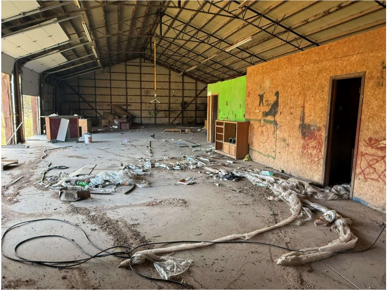
Deteriorated interior of structure located on Parcel 3.
