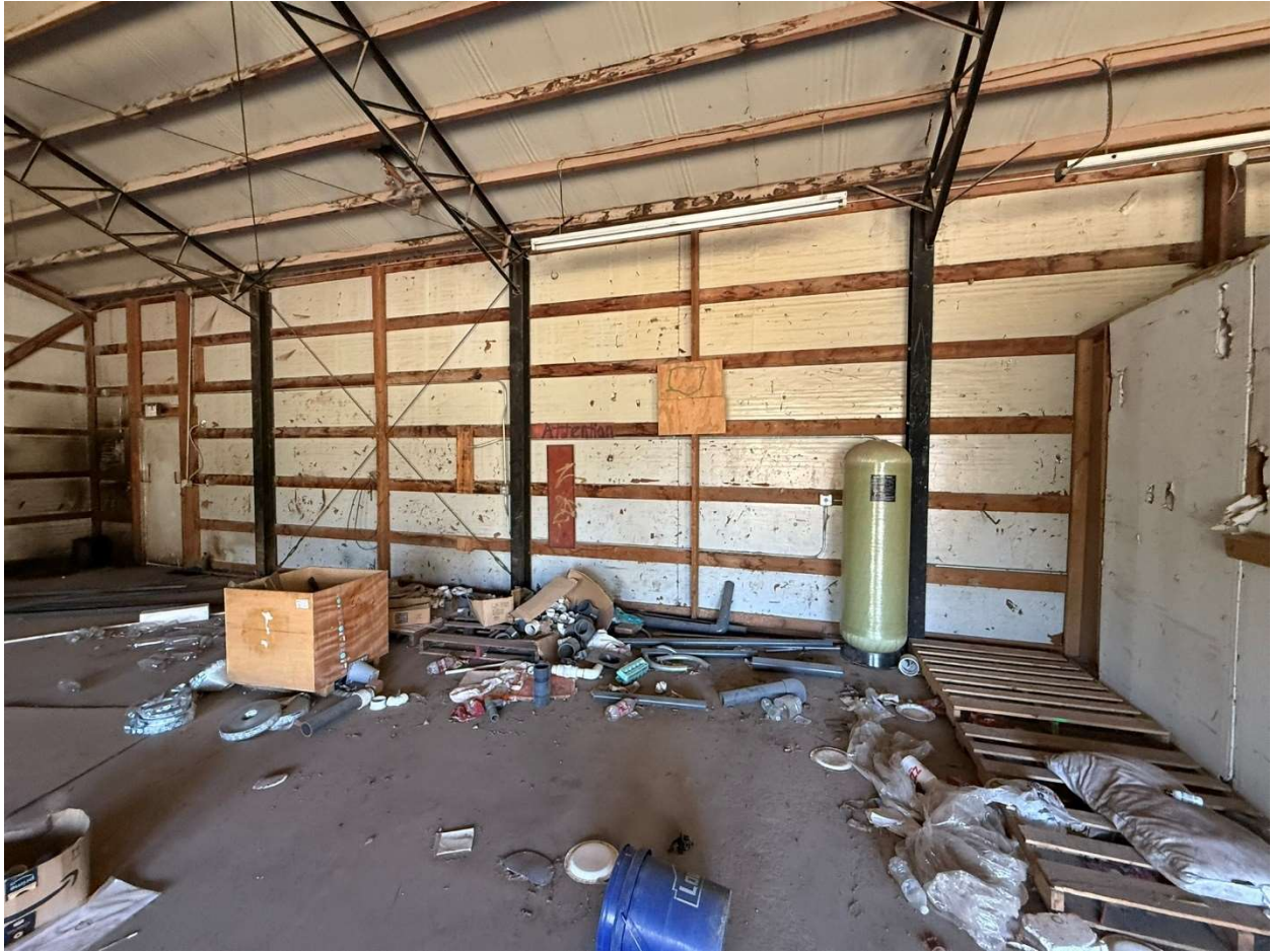
Deteriorated interior of structure located on Parcel 3.
