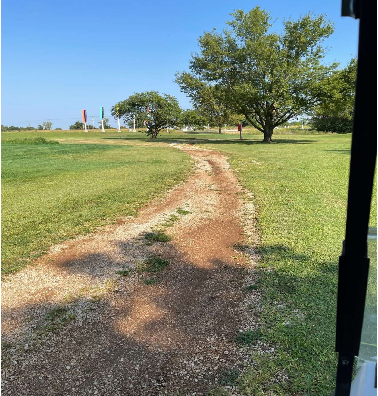
Deteriorated internal infrastructure on Parcel 2.
