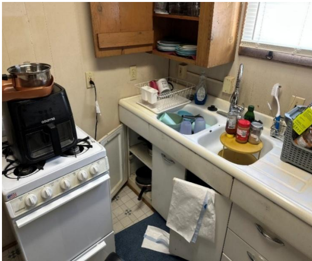
G45. The kitchen is outdated, with undersized non grounded electrical, broken appliances and worn cabinetry, and exposed plumbing.
