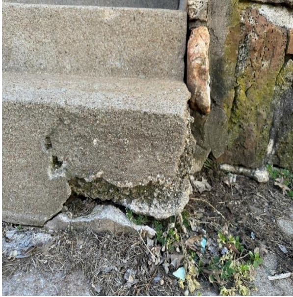
G28. The concrete step is severely deteriorated, with large cracks, crumbling edges, and exposed aggregate, creating a trip hazard and structural instability.
