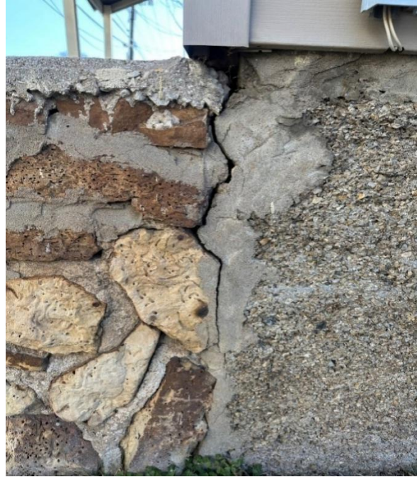
G57. The foundation has a major structural crack, posing a serious risk to the building's stability.
