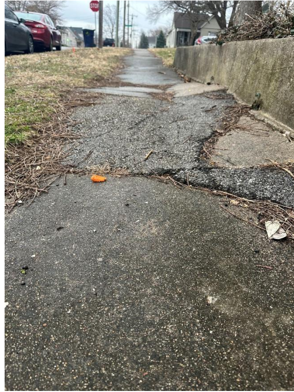
G52. This sidewalk is severely deteriorated with large cracks, uneven surfaces, and broken sections, creating a major tripping hazard.
