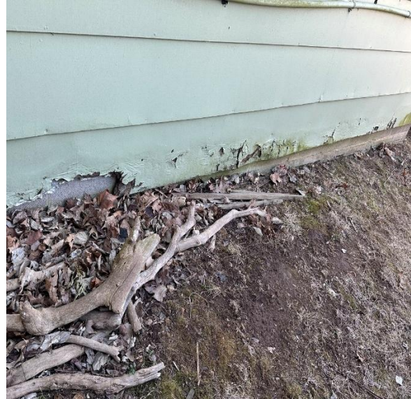
G40. The lower portion of this exterior wall exhibits severe deterioration, including rotting siding, peeling paint, and water damage, and debris accumulation, creating structural and pest intrusion risks.
