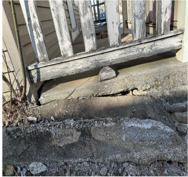
G29. The concrete porch is cracked and structurally failing. The railing is rotting and not secure.
