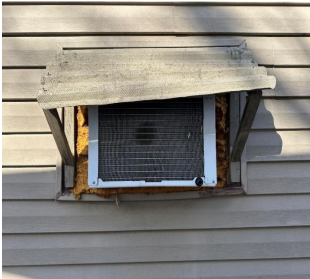
G30. The improperly installed window air conditioning unit is surrounded by expanding foam insulation, with a makeshift, deteriorating awning, creating both an unsightly and potentially unsafe condition.
