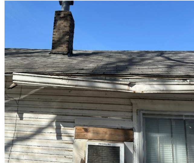
G35. The sagging and damaged gutter, deteriorating chimney and peeling paint show significant deterioration to the property.
