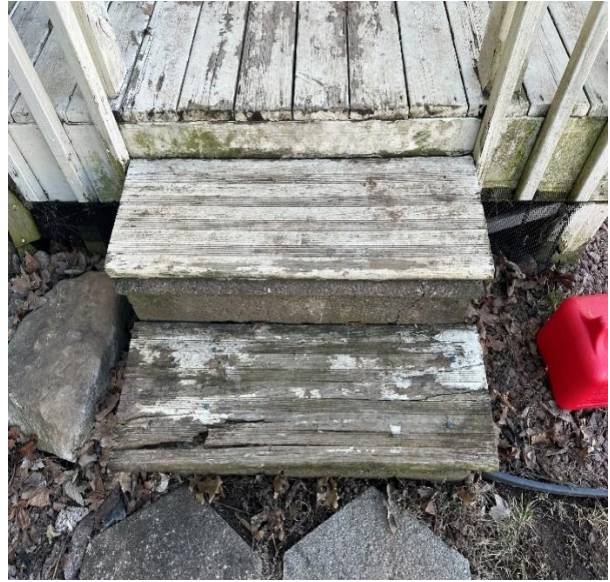
G37. The steps and decking in this image are heavily weathered, with rotting wood, peeling paint, and moss growth, creating a hazardous and unstable entryway.
