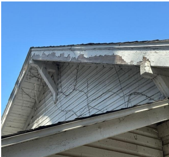
G34. The peeling paint, rotting fascia, and overgrown vines on this deteriorating gable end indicate significant concerns about potential lead-based paint hazards.
