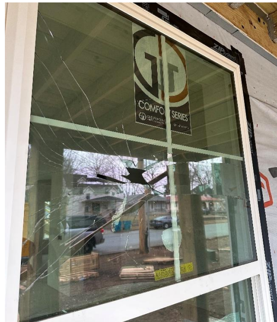
G50. This shattered window, due to vandalism, poses a serious safety hazard with sharp glass shards and compromises the security of the building.
