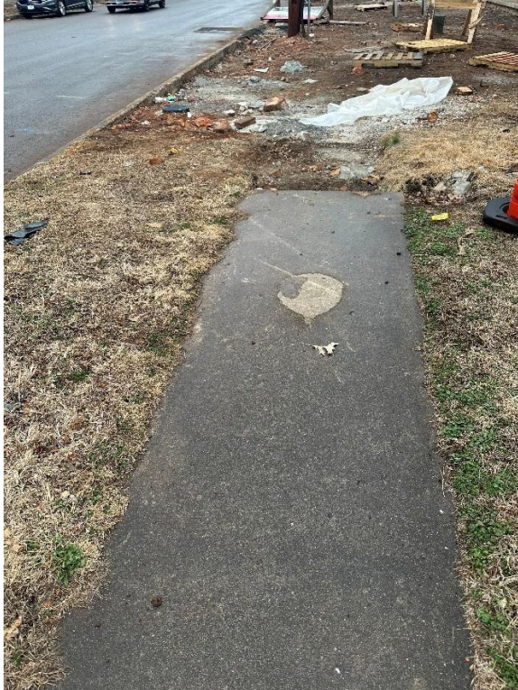
G51. The sidewalk is absent, and in need of replacement, bringing it up to ADA standards.
