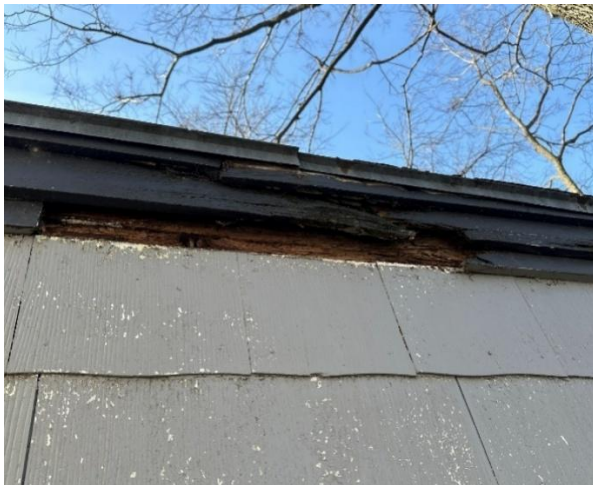
G16. The rotting fascia shows severe wood decay and structural deterioration, being vulnerable to water damage, pest infestation, and further structural compromise.
