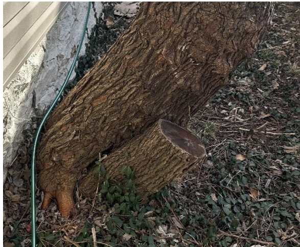
G17. The tree root system is growing through the foundation is causing serious structural concerns.
