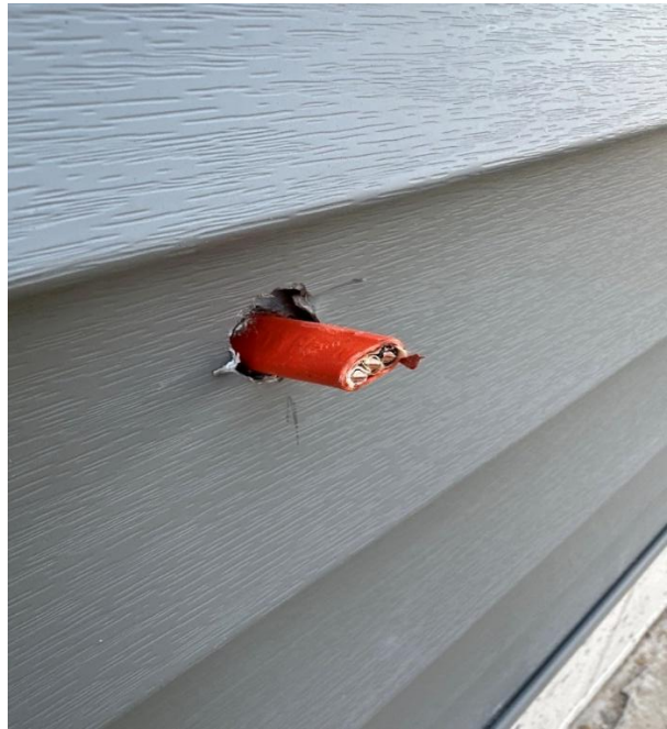
G48. The electrical wires that have been cut by vandals and left exposed, and posing a serious safety and shock hazard.
