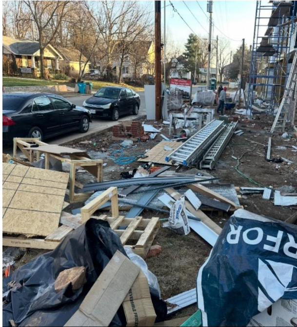
G47. The incomplete job site with construction materials, debris, and unfinished work, creating a potential hazard until its habitable.
