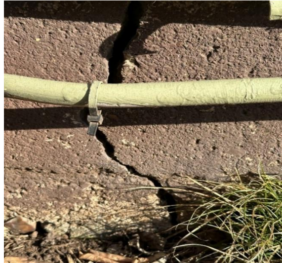
G46. The foundation has a significant crack in it, indicating structural instability, with a potentially vulnerable electrical pipe running across it.
