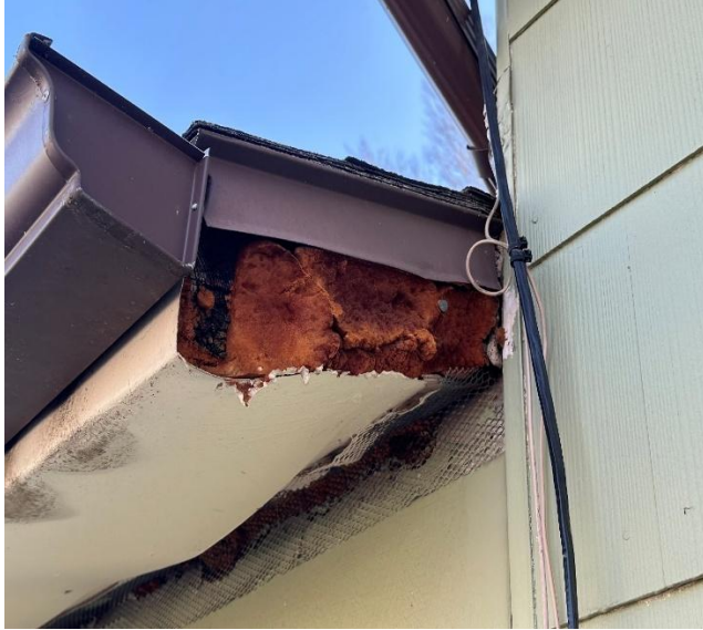
G39. The soffit is severely damaged with exposed insulation, rotting wood, and deteriorating materials, creating structural concerns and potential entry points for pests.
