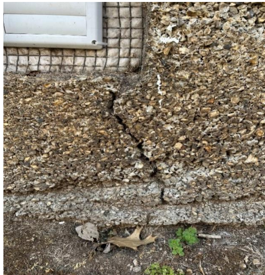
G31. The cracked foundation, is structurally failing, and a structural footing is non-existent.
