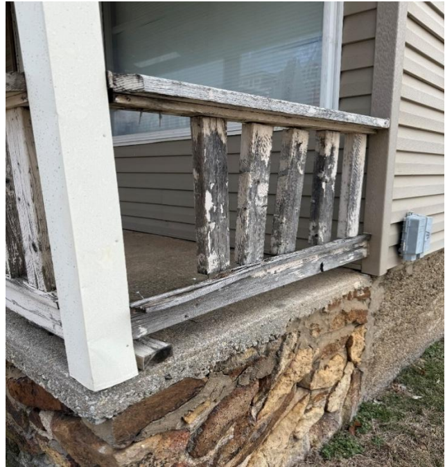
G33. The railing is broken and severely deteriorated, posing a serious fall hazard. Additionally, the chipping and peeling paint is indicative of potential lead-based paint, creating significant health and safety risks, particularly for children.
