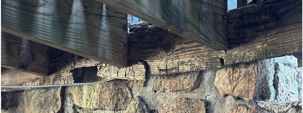
G18. The deck's rim joist is severely rotted and detaching from the wall, compromising the structural integrity of the deck and posing a serious safety hazard due to potential collapse.
