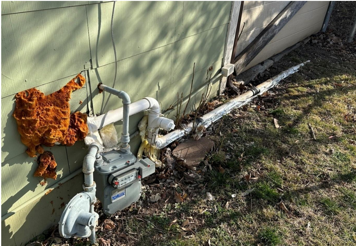
G24. The indoor plumbing is improperly routed through the exterior wall, extending directly into the ground without proper drainage infrastructure, creating potential sanitation and structural risks. Additionally, the broken asbestos siding has been inadequately patched with spray foam, which is not a safe or code-compliant repair method, further compromising the integrity of the building.
