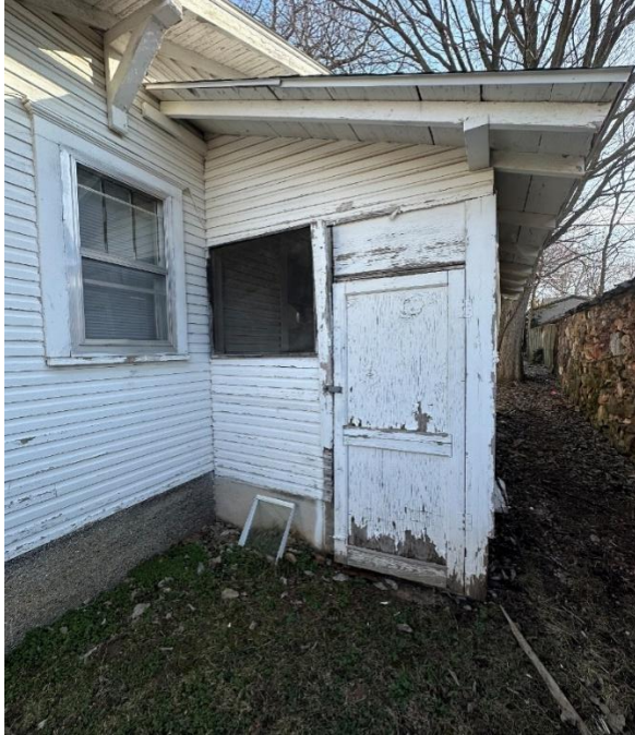
G32. The structure shows severe deterioration, with chipped and peeling paint, rotting wood, a warped door, and a missing window, all contributing to significant structural and safety concerns.
