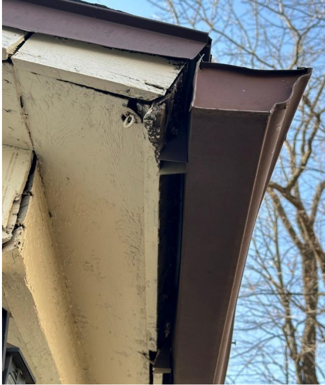
G43. The soffit and fascia are severely deteriorated with rotting wood, structural separation, creating potential for water intrusion and further damage.
