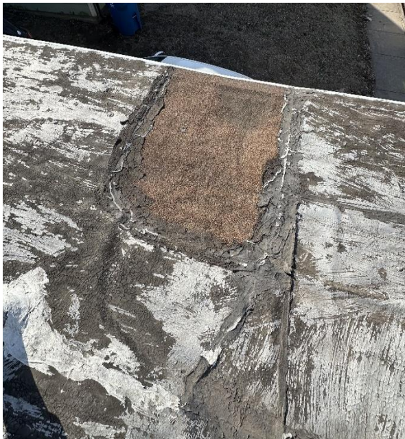
G58. The roof is severely deteriorated with extensive cracking, patchwork repairs, and failing materials, indicating it has no remaining lifespan and needs complete replacement.
