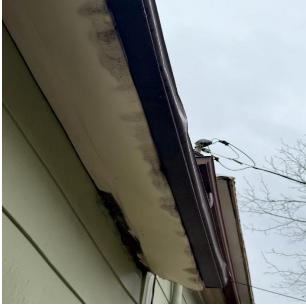
G23. The rotting wood and deteriorated soffits, along with the failing gutters, show clear signs of water damage and possible mold growth, exacerbated by gaps that allow animal and rodent intrusion.
