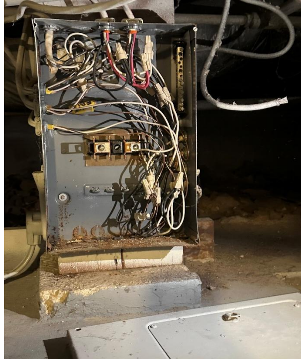
G15. This improperly wired electrical panel poses a serious fire and electrocution hazard, with unsecured connections, overloaded circuits, and a lack of proper insulation or grounding.
