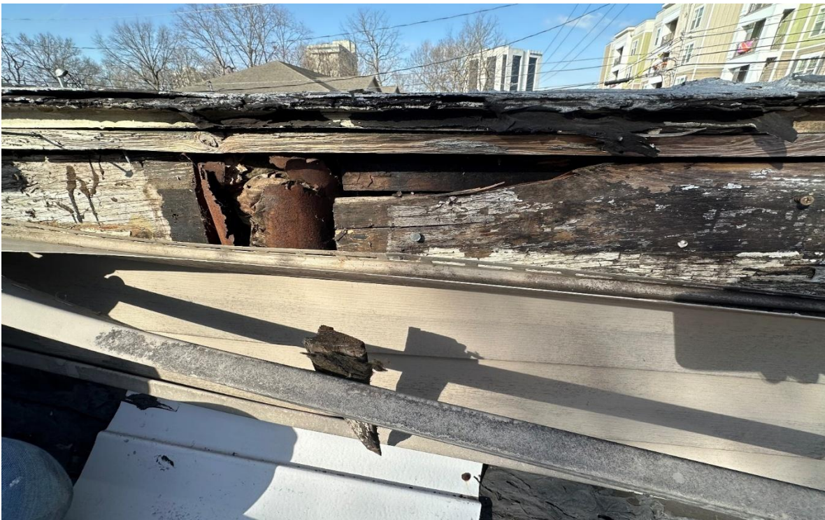
G61. This structure exhibits extreme deterioration, with severely rotted wood, rusted and damaged plumbing vent piping, and failing layers of material, indicating a critical need for immediate structural repairs.
