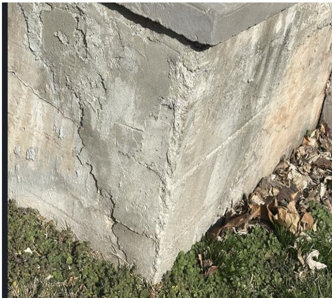
G53. This foundation corner of the porch has significant cracks, indicating potential structural issues.
