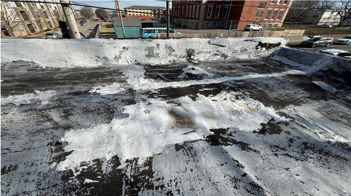
G60. This roof is in an advanced state of decay, with extreme cracking, peeling coatings, and makeshift, ineffective repairs, leaving it completely compromised and in need of full replacement.
