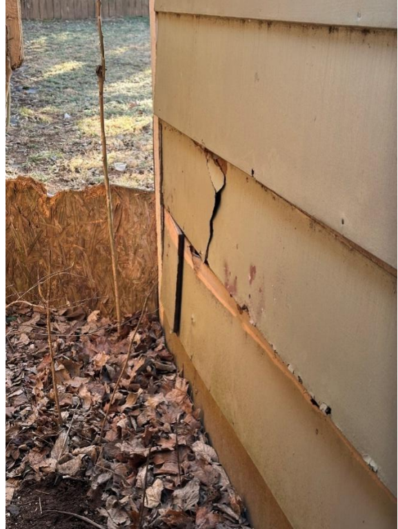
G44. The siding is severely damaged with large cracks, missing sections, and signs of decay, exposing the structure to water.
