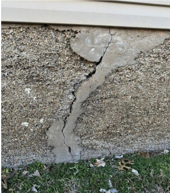
G56. The foundation has a significant structural crack, indicating foundation issues that compromise the building's integrity.
