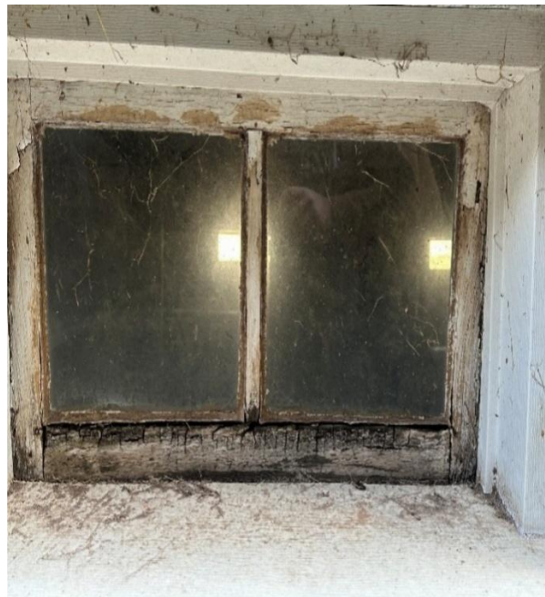
G20. The window frame is severely deteriorated, with rotting, cracked wood, and peeling paint.
