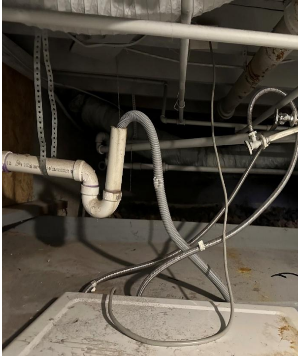
G14. The plumbing is outdated and not code compliant. Unsuitable materials, and unsecured drain connections, could lead to leaks, and water damage.
