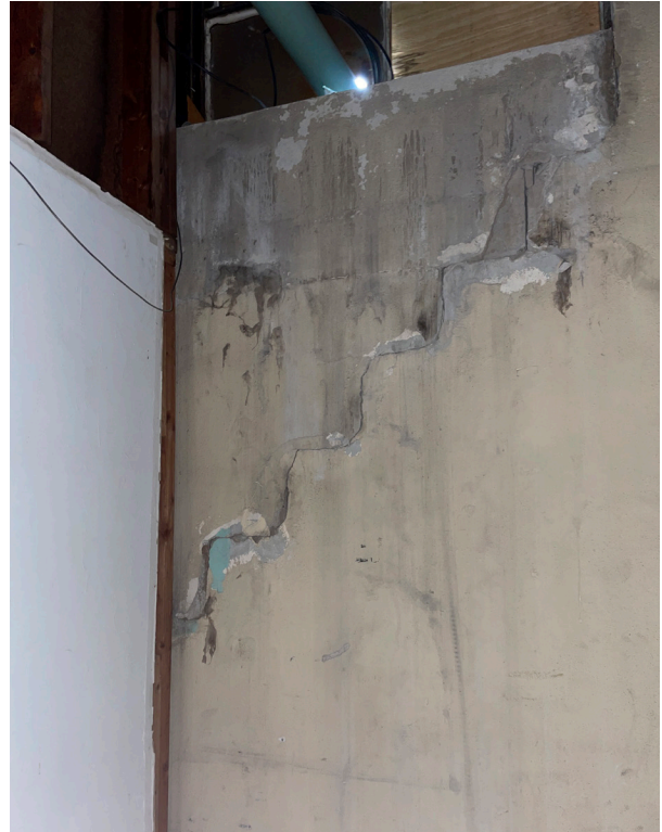
12. Large crack in an exterior load bearing wall from poor storm-water management.
