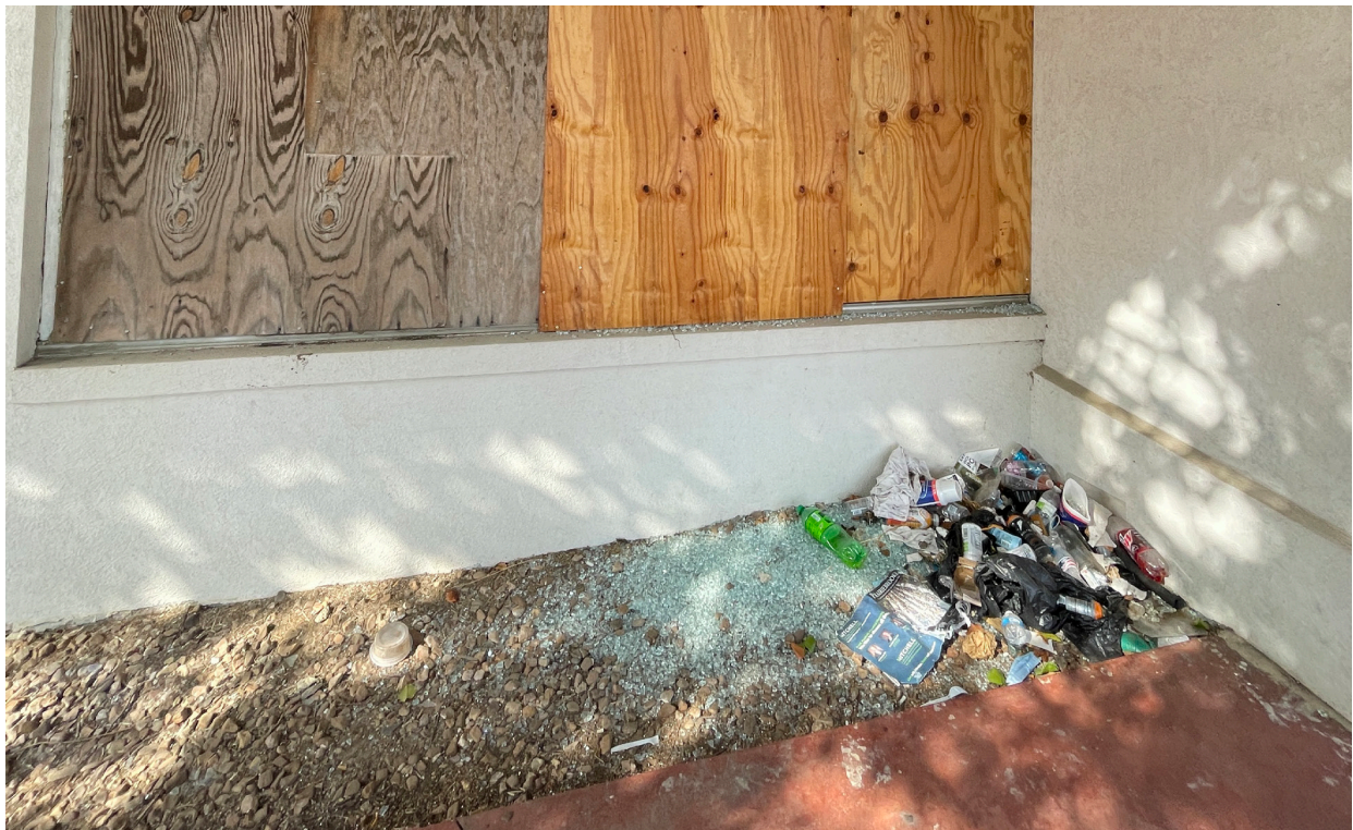
9. Broken glass from vandalism and trash from homeless individuals living on the premises.
