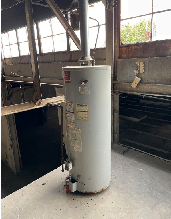
19. Water pipes into and out of the water heater have been removed. Electrical components of water heater have also been removed.
