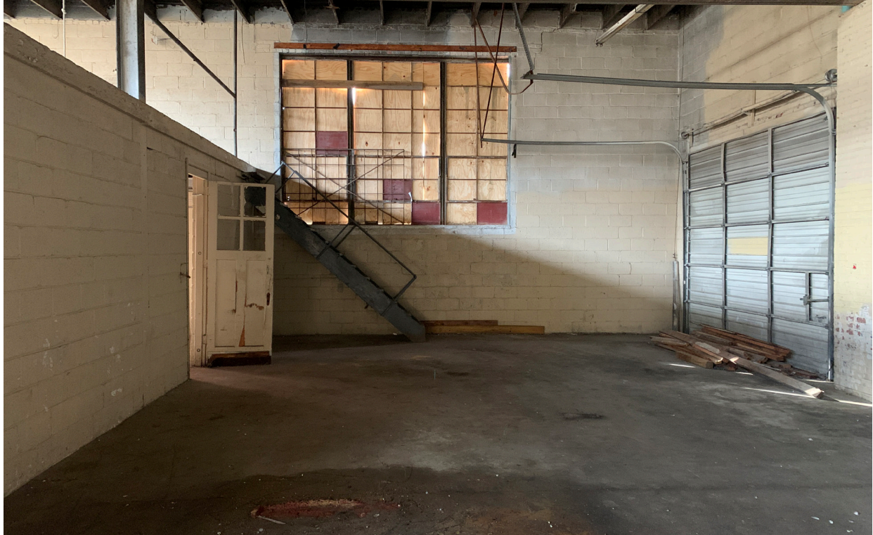
16. Broken exterior glazing; window frame is not thermally broken.
