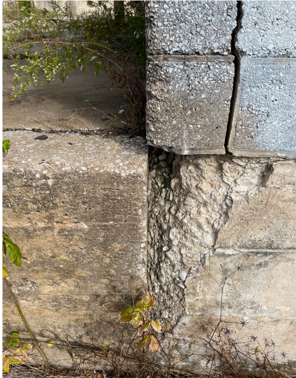
11. Cracks in the walls and foundations.
