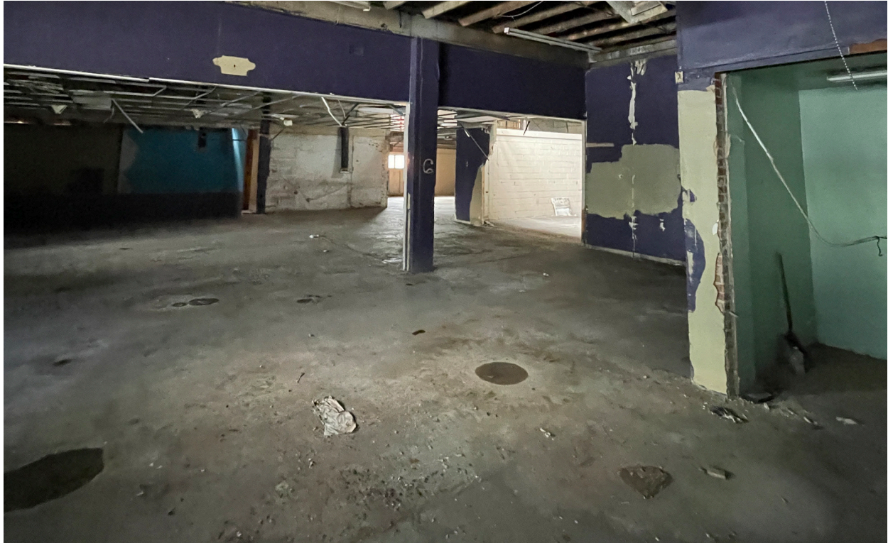
34. Existing roof is leaking resulting in areas with water ponding in the interior of the building .
