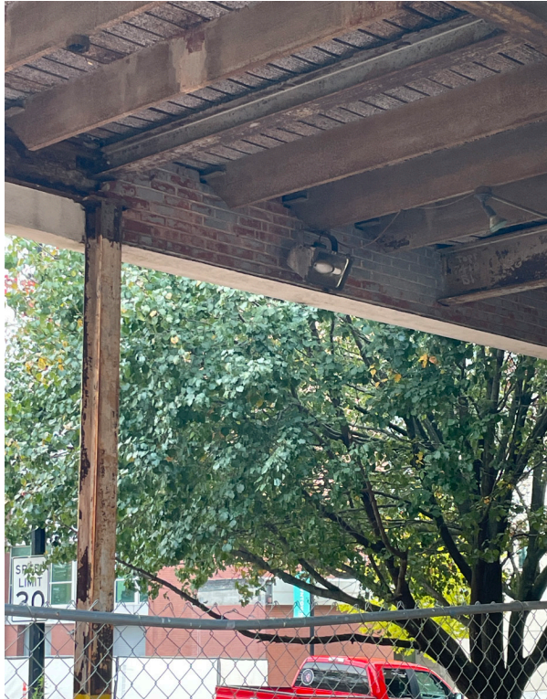
25. Existing exterior light fixture. Wire has been removed from Conduit.
