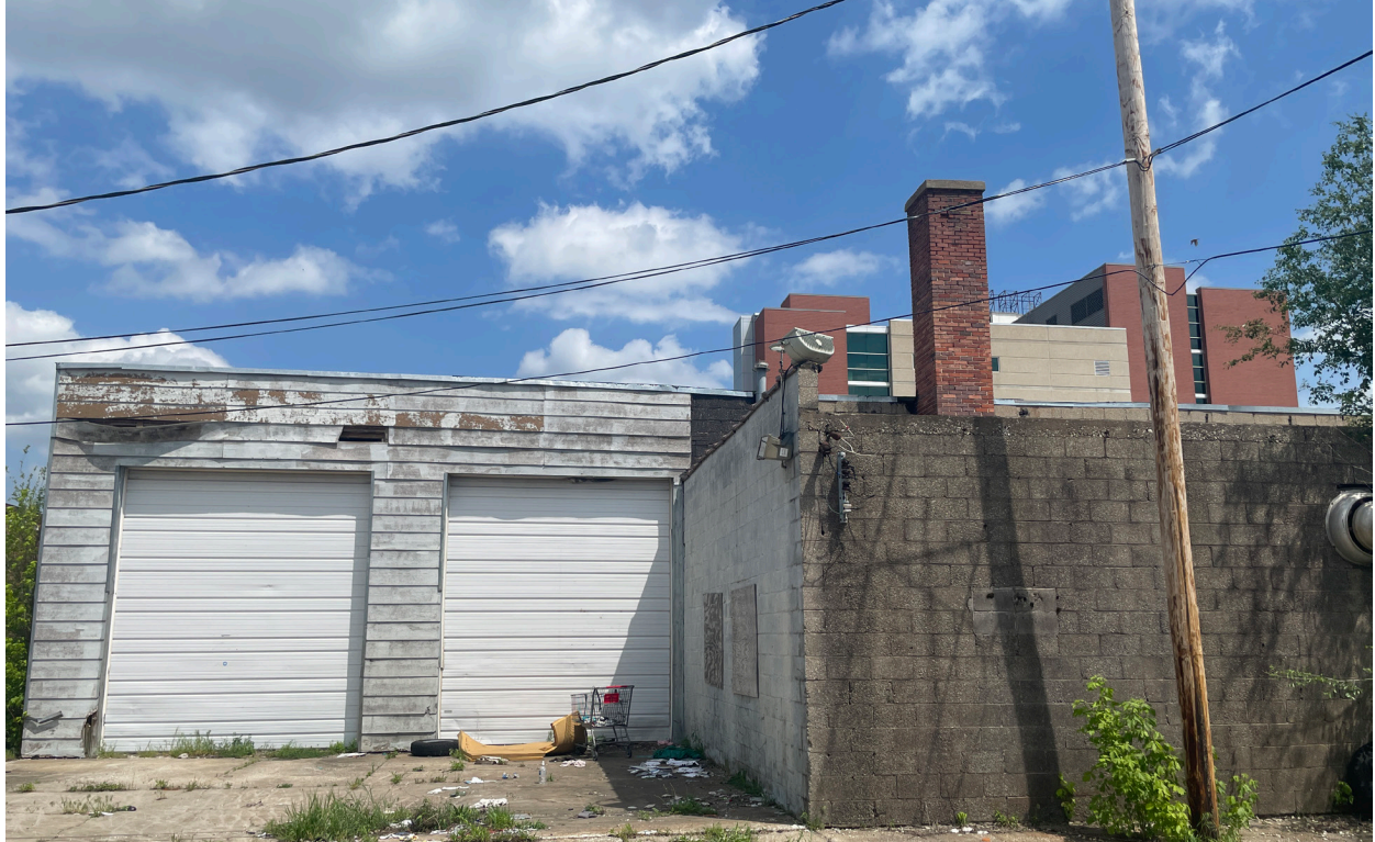
10. Low hanging power lines. Location of electrical service to the building has been removed. All electrical panel in the interior of the building have had copper electrical wires removed.
