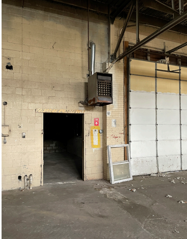
23. Existing gas heater.
