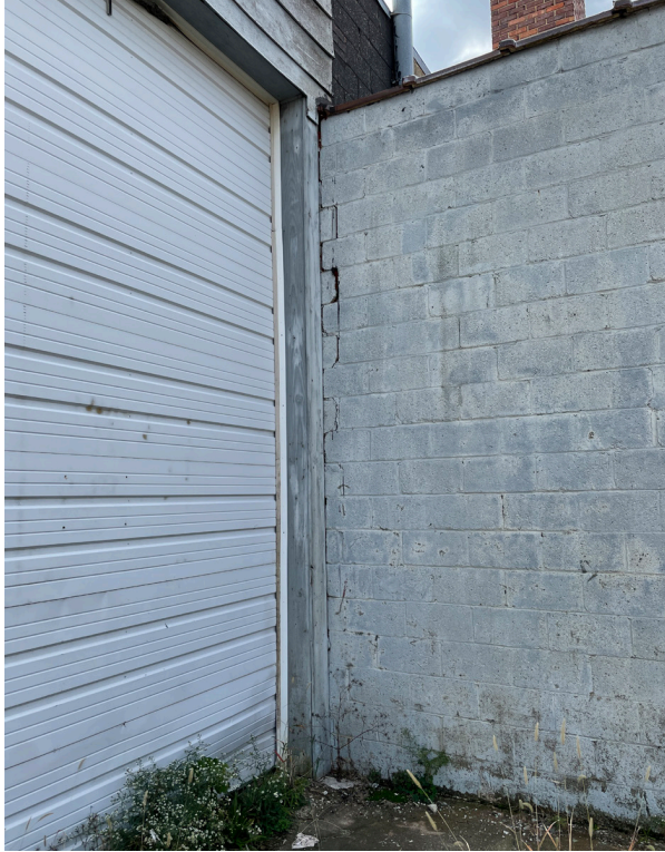
13. Large crack in wall of existing load bearing wall.
