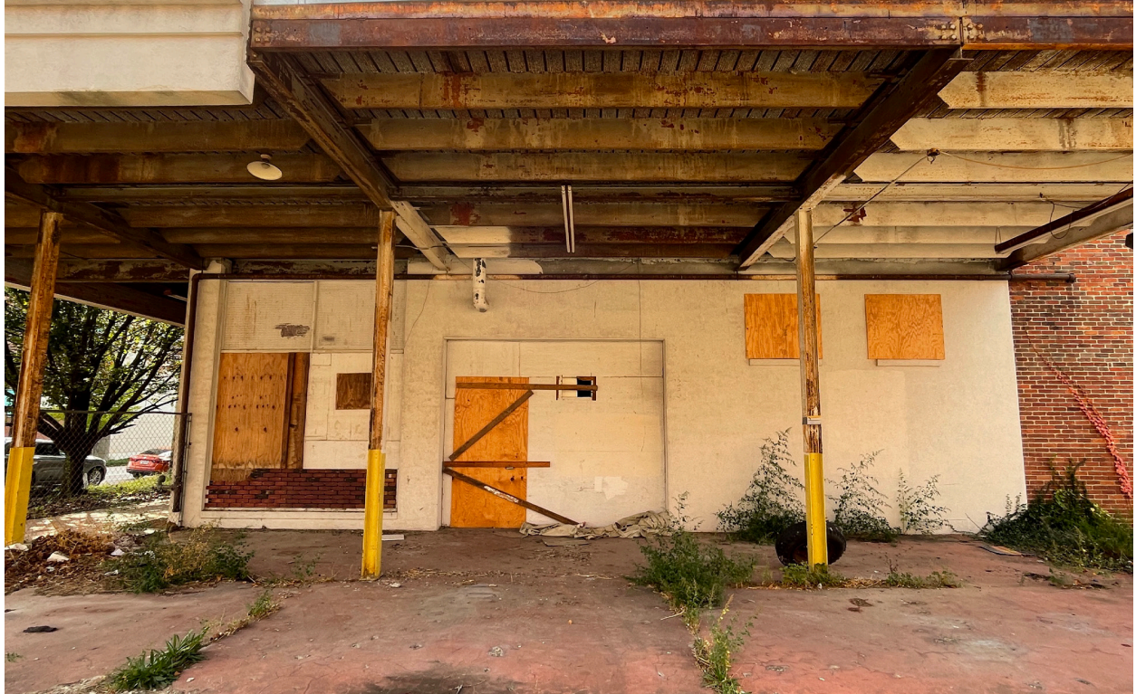
30. Boarded up windows and openings.
