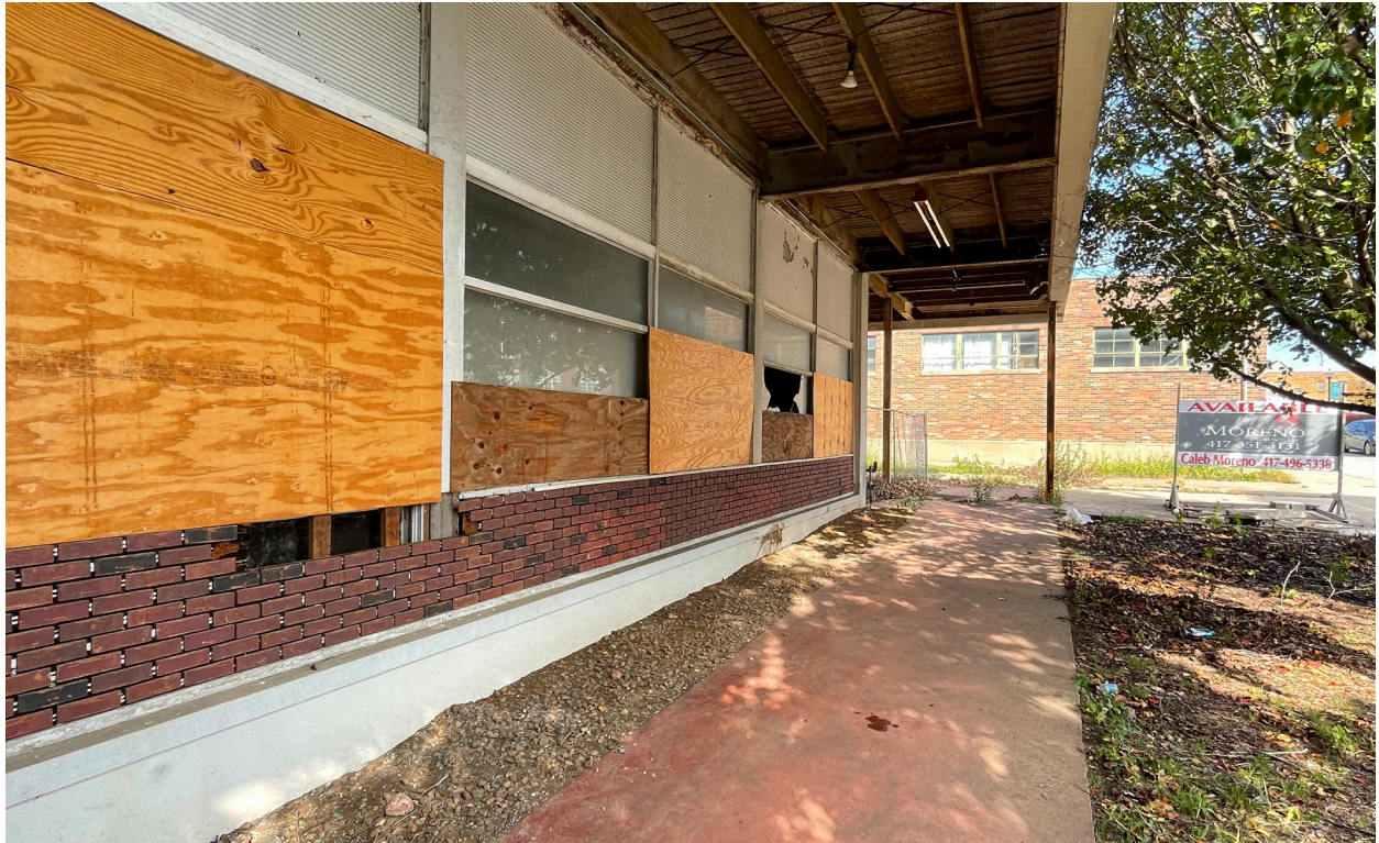
31. Boarded up windows with broken glazing. Windows are original to the building and are not thermally broken.
