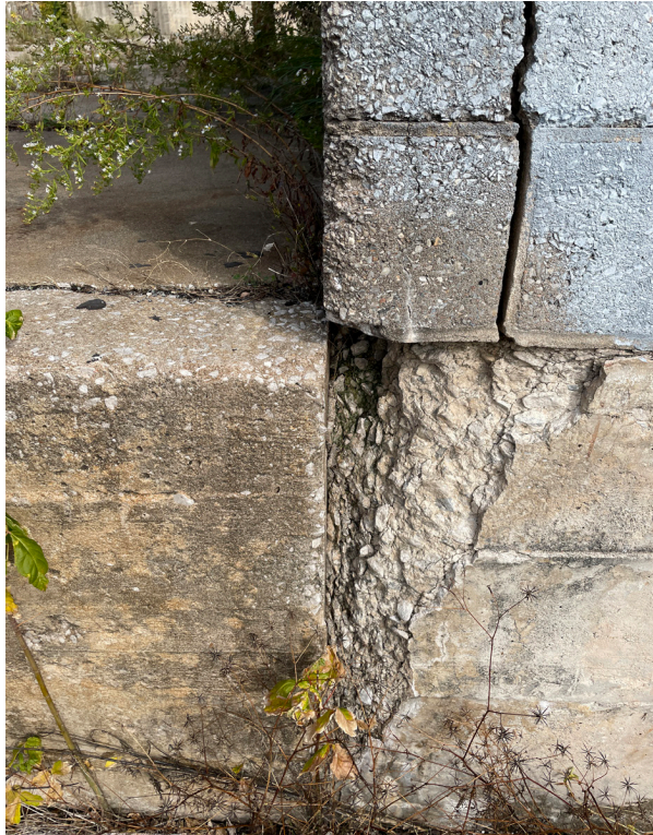
11. Cracks in the walls and foundations.
