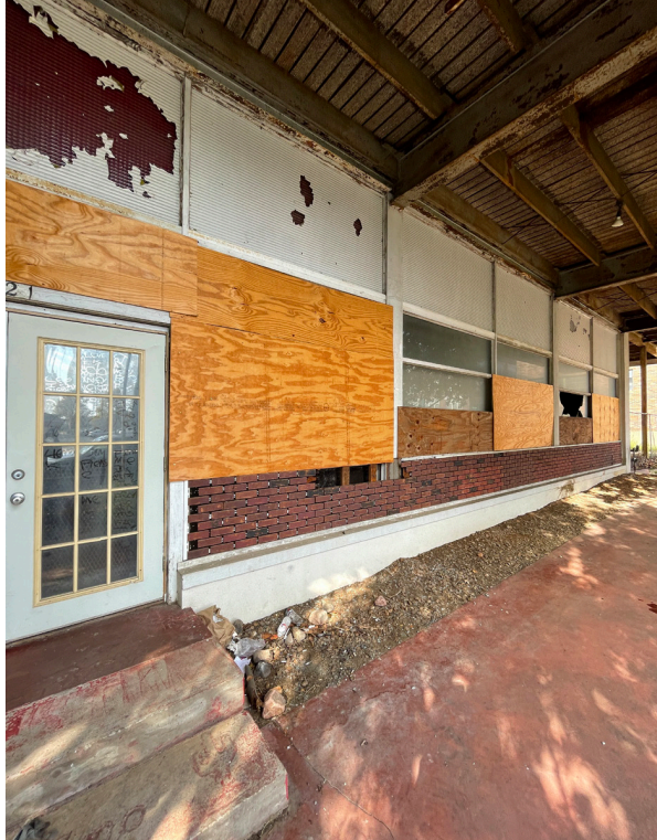
7. Trash accumulation near main entrance of the building.
