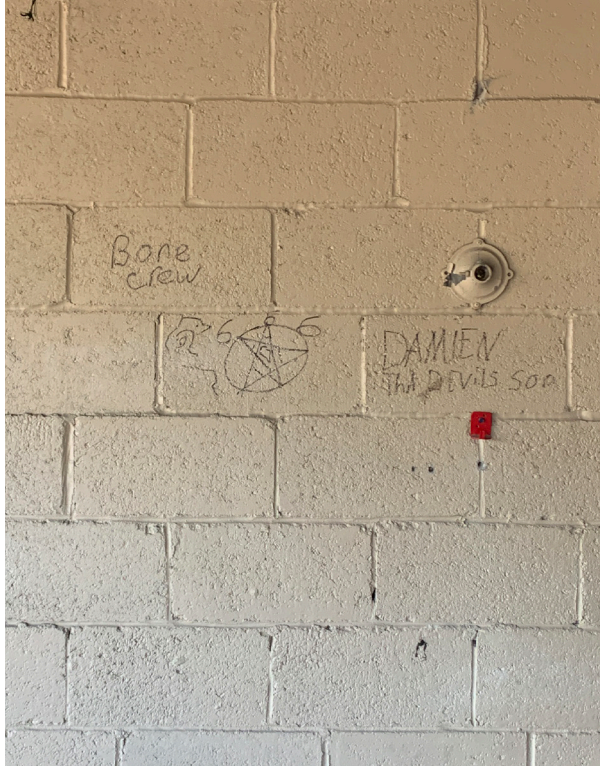
35. Vandalism inside of the building.
