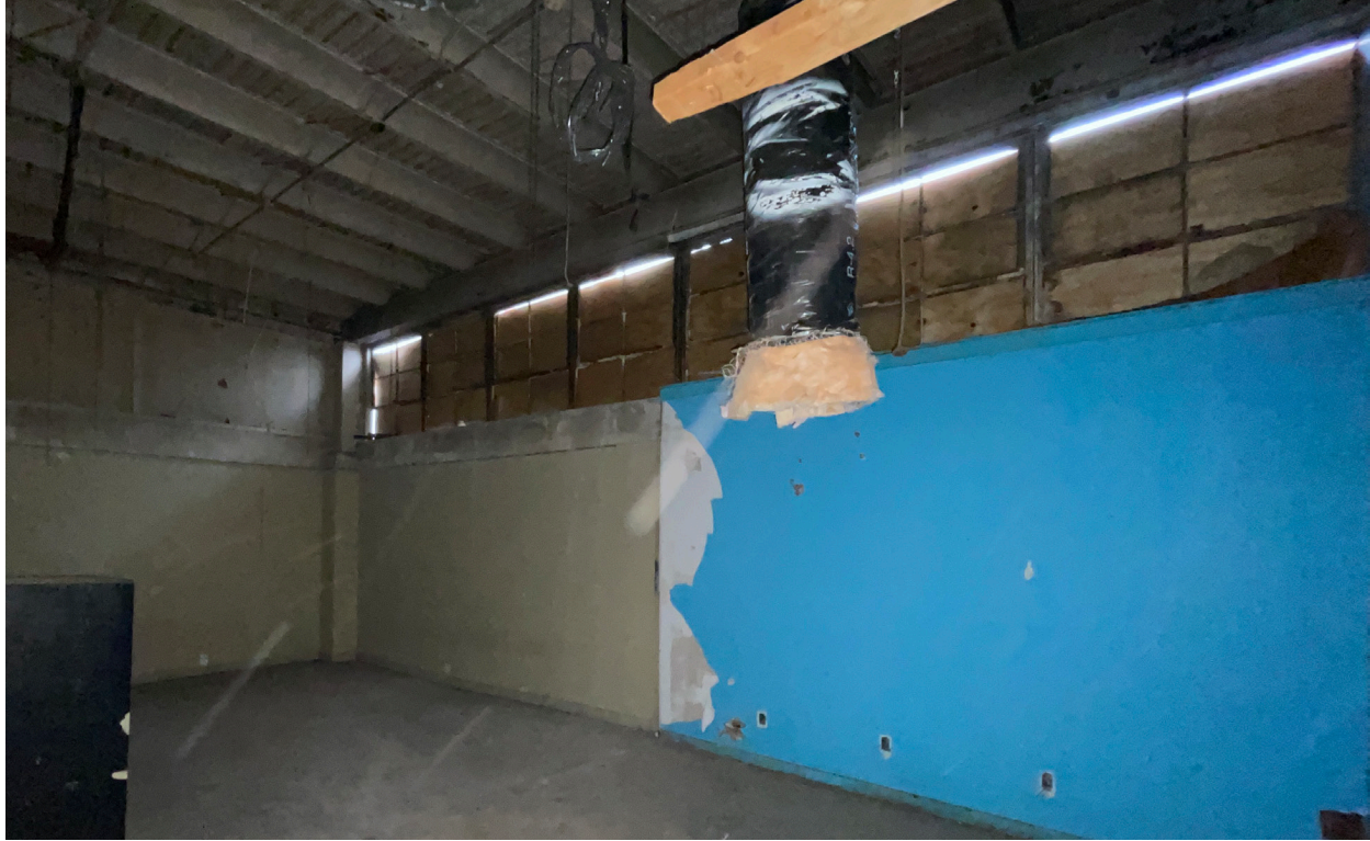
27. Original non-thermally broken steel framed windows; all glass has been broken/ removed.
