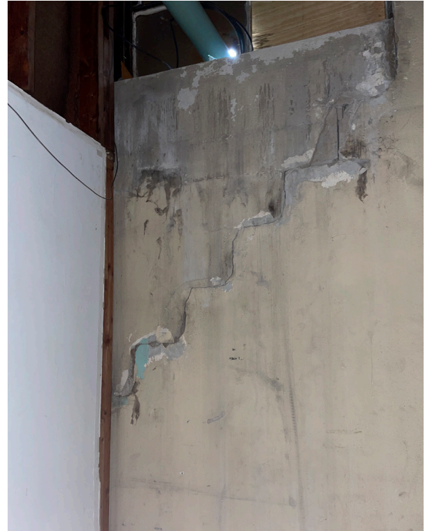
12. Large crack in an exterior load bearing wall from poor storm-water management.
