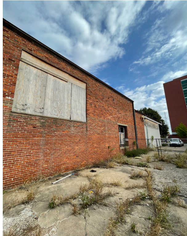
29. Boarded up windows where glass has been removed.
