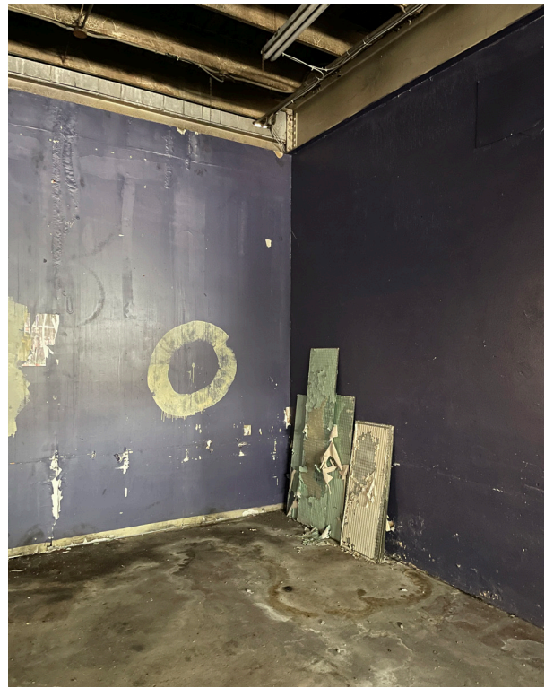
33. Sagging paint, water stains, and mold at the base of interior wall.
