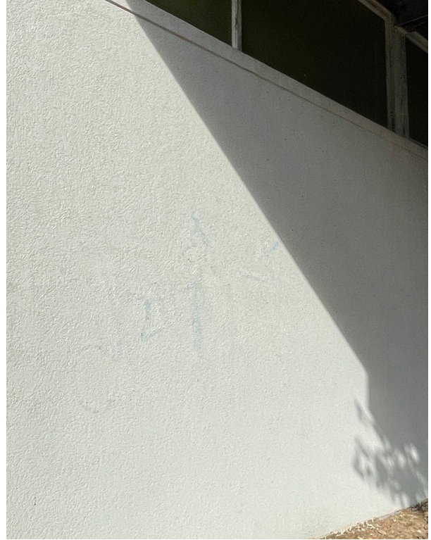
36. Graffiti showing through paint on front elevation of the building.
