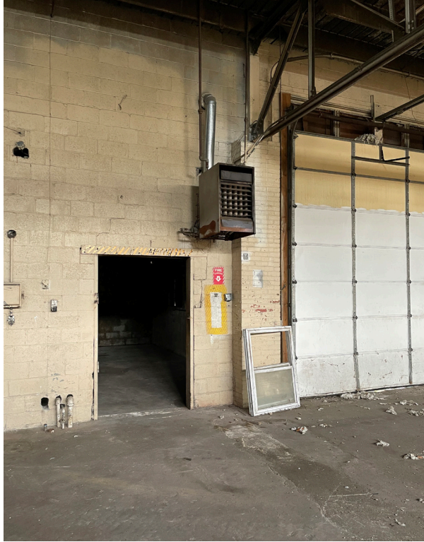
23. Existing gas heater.
