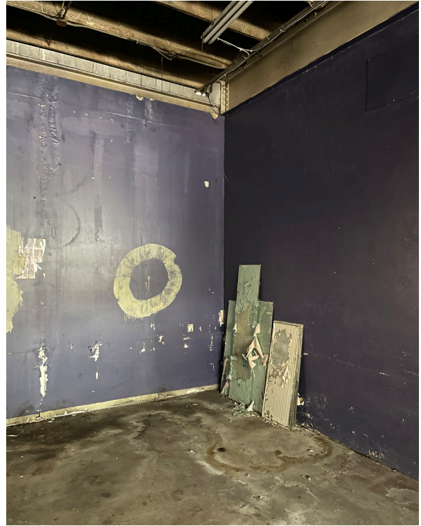
33. Sagging paint, water stains, and mold at the base of interior wall.
