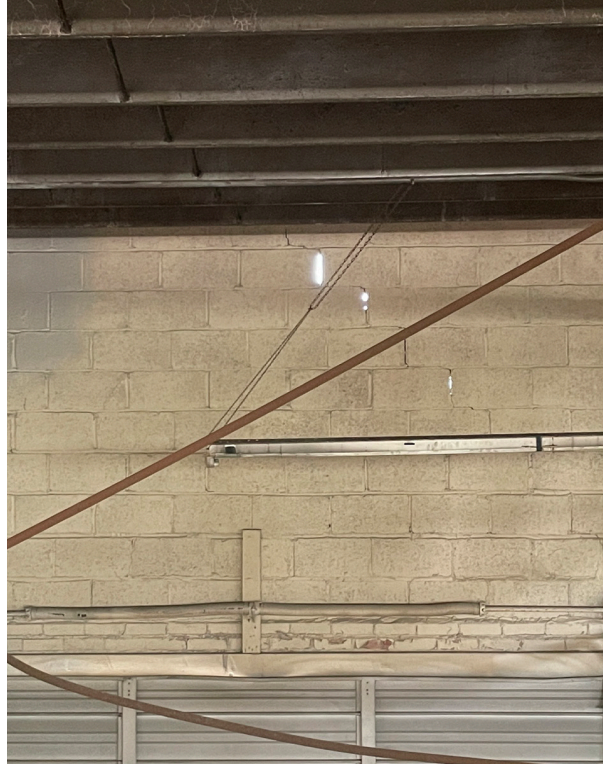
14. Sunlight can be seen through cracks the west exterior load bearing block wall.
