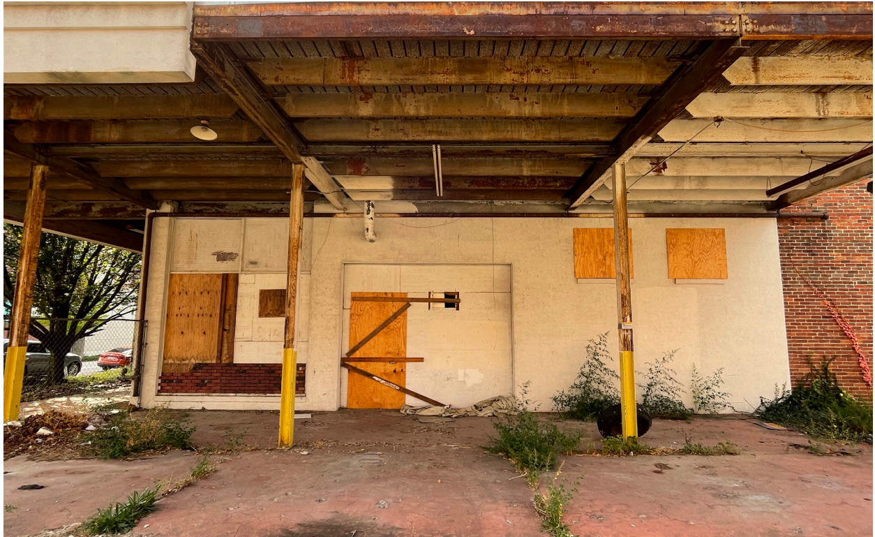
30. Boarded up windows and openings.
