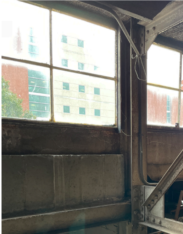
28. Original non-thermally broken steel framed windows. Several panes of glass have been broken allowing various animal to inhabit the building.
