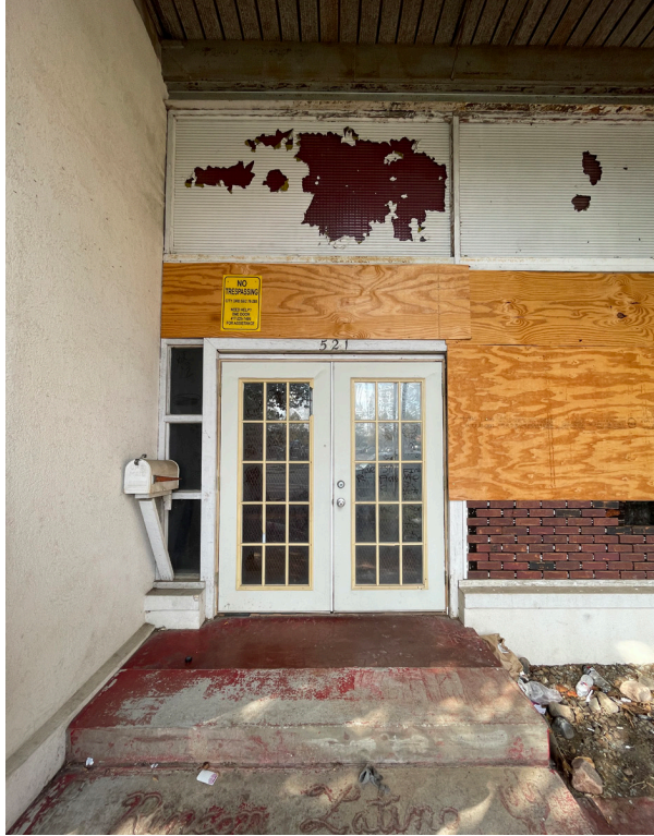
32. Main entry of the building is not handicap accessible.
