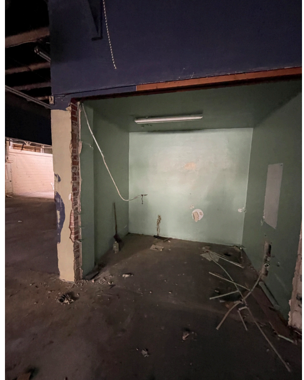
2. Trash and human waste located throughout the interior and exterior of the building. Existing sewer connection for water closet is uncovered and open to the space.
