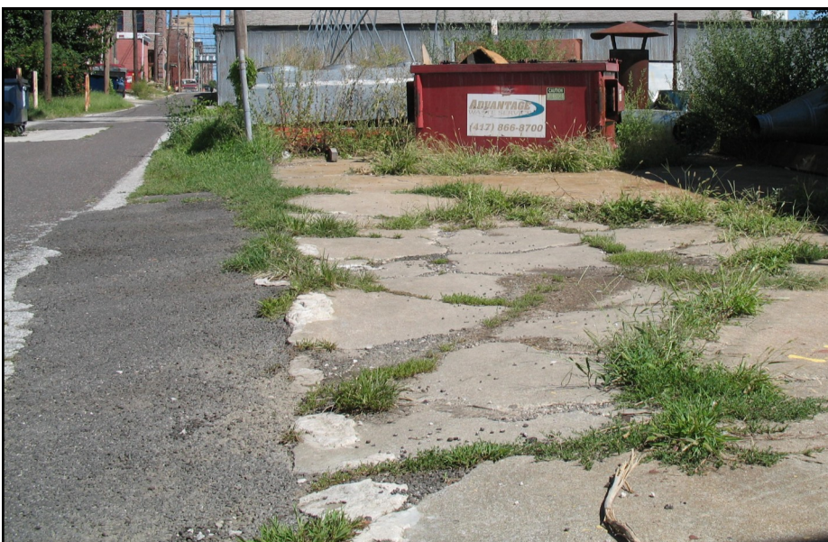
Inadequate street layout on Blaine in need of repair
