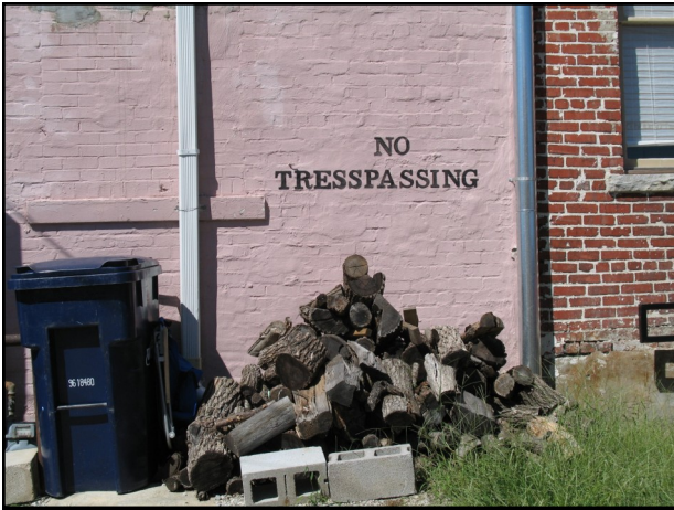
Firewood piled next to building is a health and safety Hazard and provides habitat for rodents
