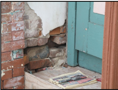
Structural damage to the foundation and missing bricks are a sign of major deterioration
