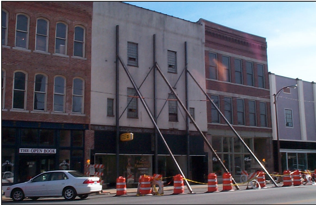
This dangerous building was at risk of falling down and required a support system to stabilize the structure until it could be repaired.
