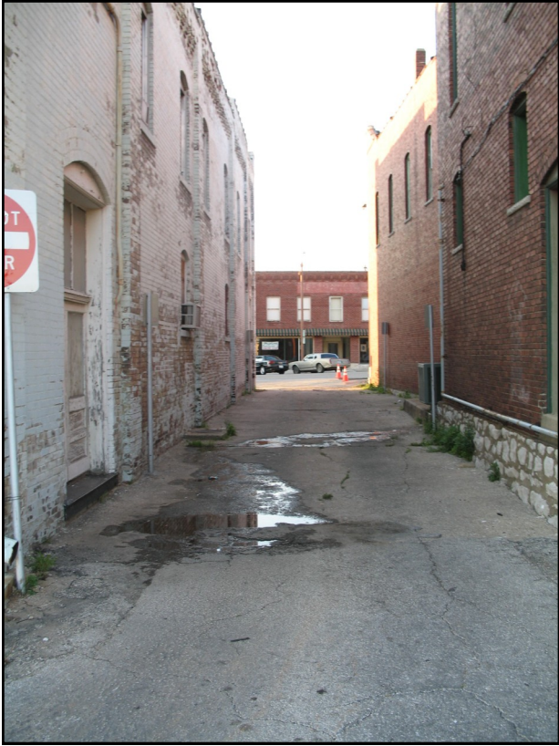
Alley with deteriorated asphalt, weeds, and buildings in need of exterior renovation
