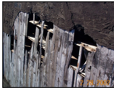
Close-up of a dangerous building with major deterioration
