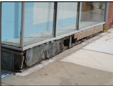
Example of structural damage to building foundation
