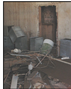
Storage of flammable materials piled inside buildings is a fire hazard
