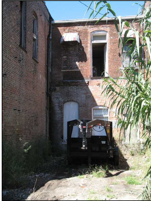
Lack of stairs from second story door
