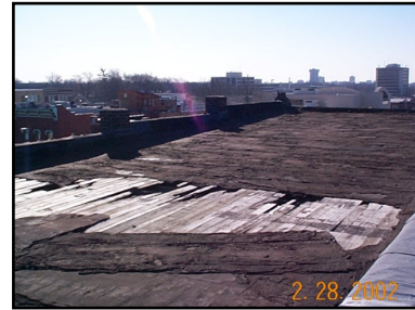
Inadequate roof systems lead to significant water damage.
