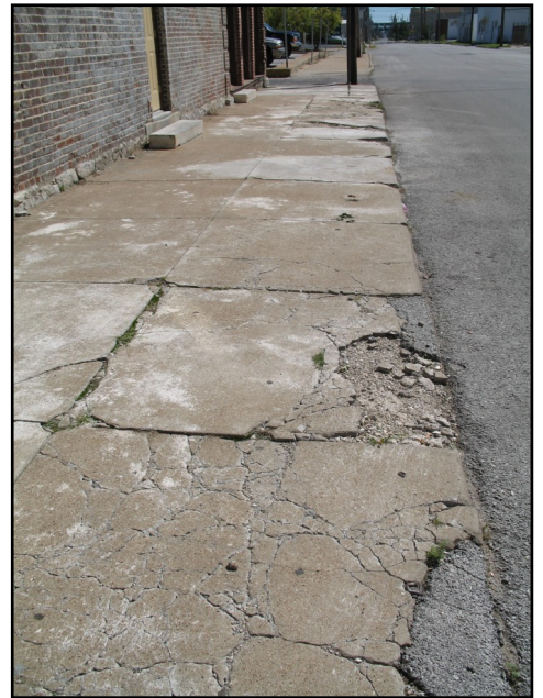
Crumbling, buckling sidewalks without curb and guttering
