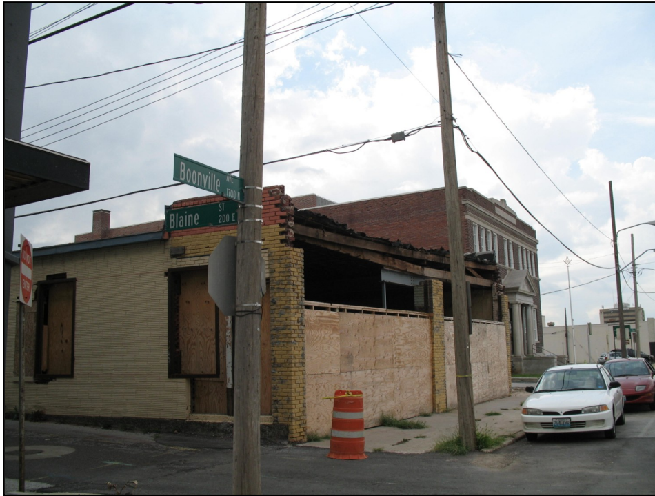
Current condition of a fire damaged structure at Blaine and Boonville within the Redevelopment Area
