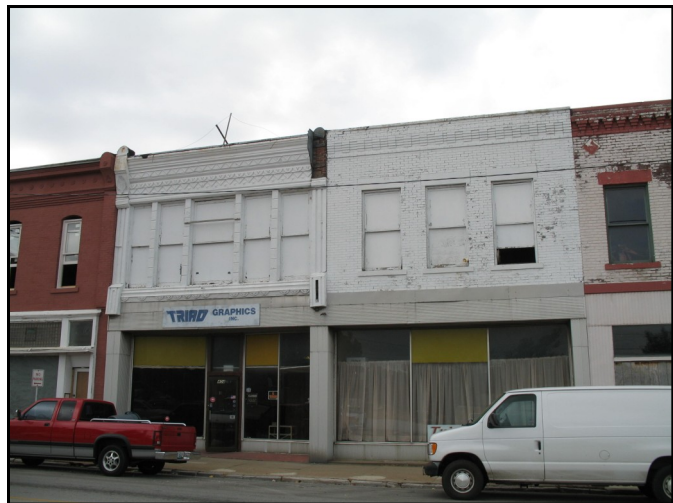
Example of one of the vacant storefronts in the Redevelopment Area. Several unoccupied structures are full of trash, litter, debris, or combustible material.
