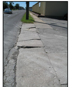
Close-up of cracked and buckling driveway
