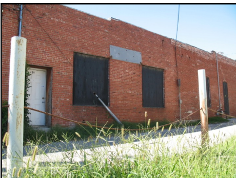
Weeds along alley show general lack of maintenance
