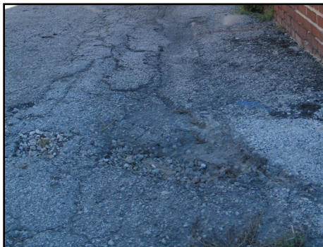
Close-up of asphalt deterioration in an alley
