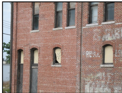
Many buildings have boarded windows like the one pictured
