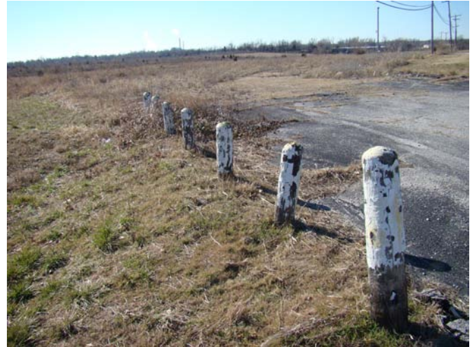
Deteriorated pavement and concrete bollards.
