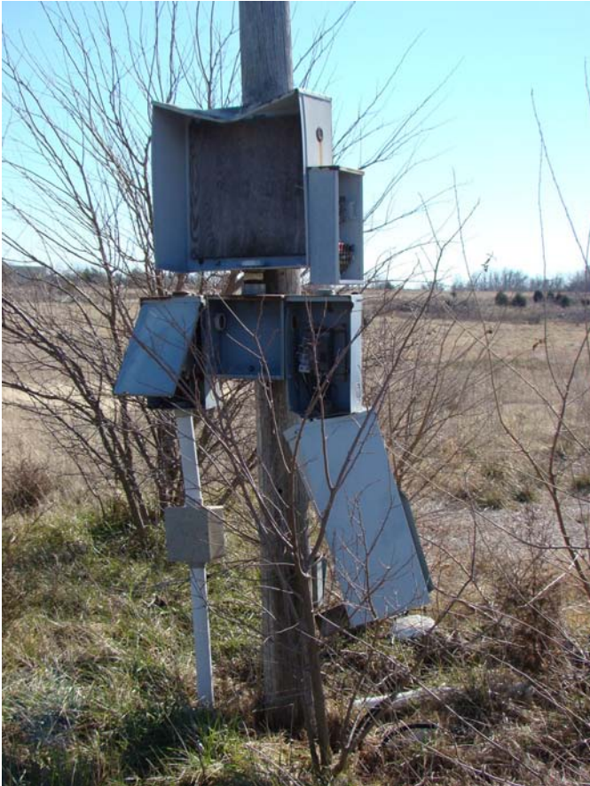
Damaged utility pole.
