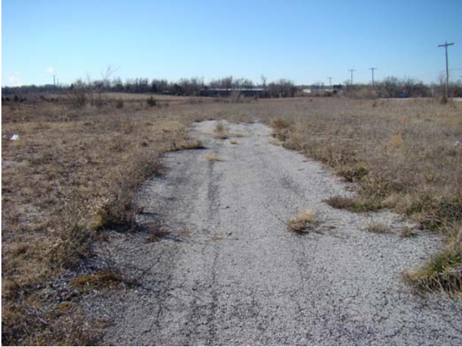
A deteriorated road-way leading into the Redevelopment Area.
