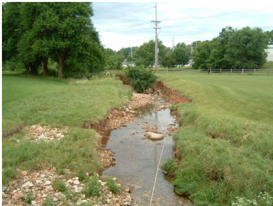
Figure 23: Ward Branch stream bank erosion
