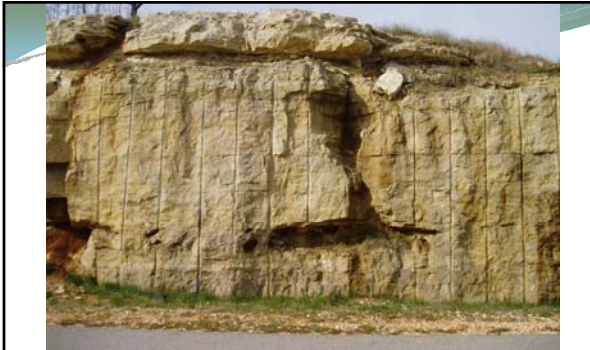
Joints and bedding planes provide weak points in the rock that, over time, become complex and intricate underground drainage systems.
