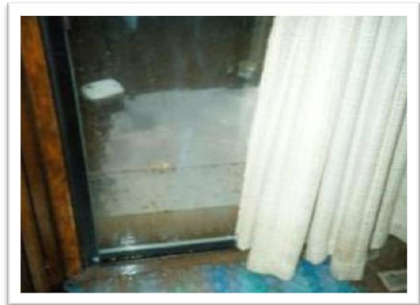
Figure 6. 2001 Flood in Hidden Valley Estates Subdivision. Note water level on sliding glass door.
