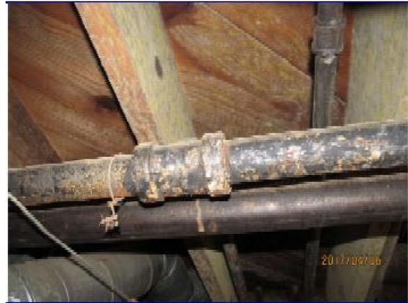
B-2.13) Metal Gas piping is corrosive and may be leaking gas into the house.
