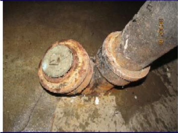
B-2.12) Sewer and Plumbing is obsolete and does not connect to city sanitation services due to a broken
