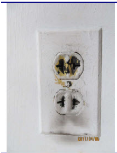
B-10) Electrical outlet has no grounding plug and appears to have been melted due to improper wiring throughout the house.
