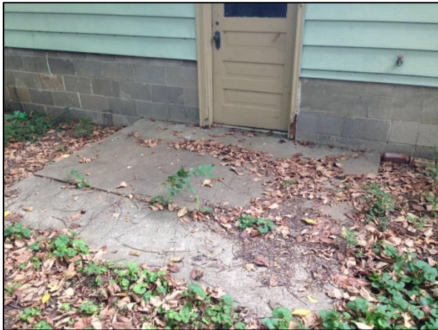
A1.) Sagging patio, and rotting exterior door jam
