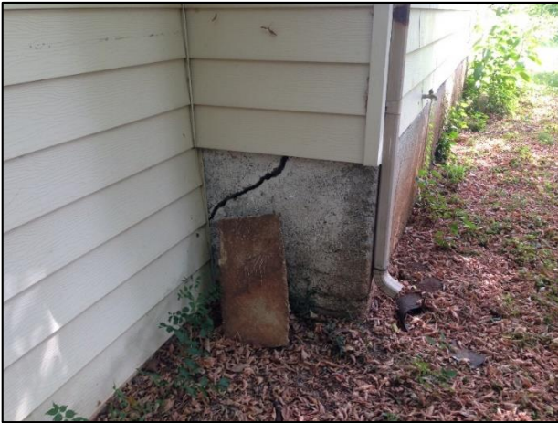
A13.) Cracked and failing foundation
