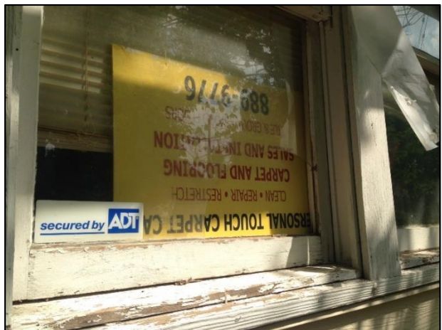
A10.) Broken windows which have been temporarily covered for quite some time
