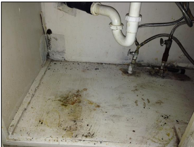
35.) Failing plumbing under the kitchen sink is a favorable environment for mold growth
