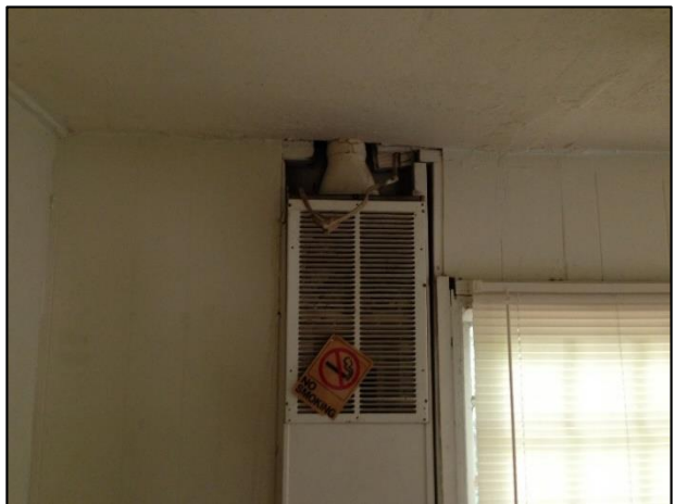
A16.) Dated wall heating system with exposed wiring
