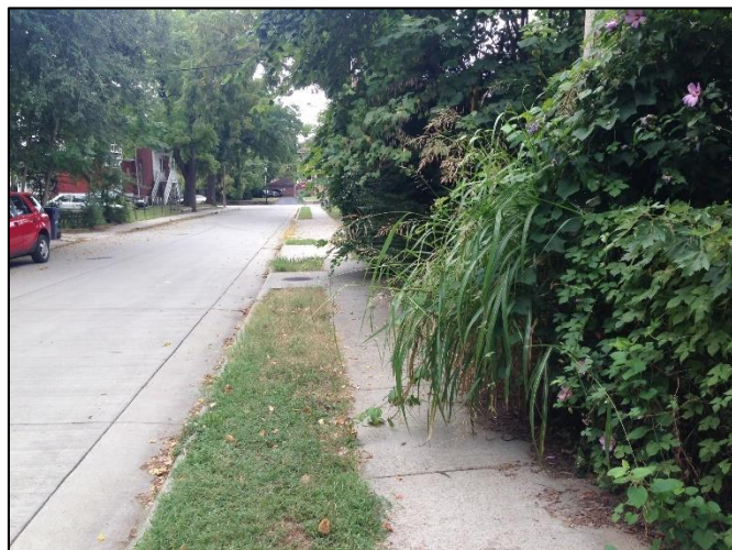
A25.) Vegetation is overgrowing the public sidewalks endangering pedestrians and bikers
