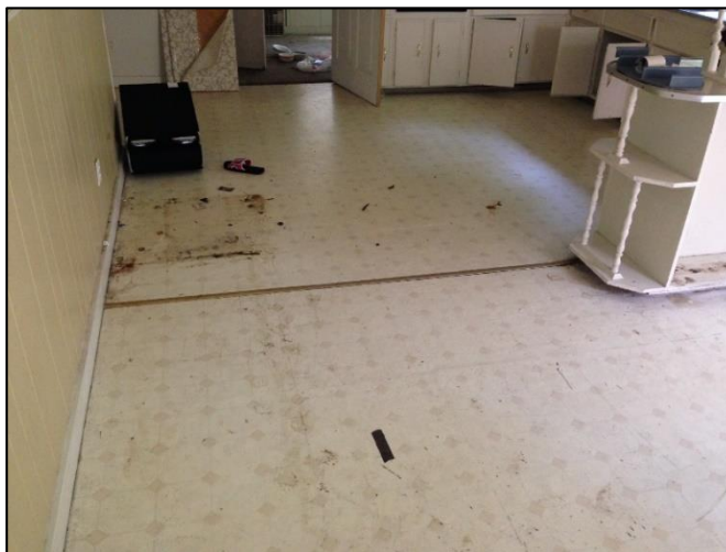
36.) Filthy interior flooring is throughout
