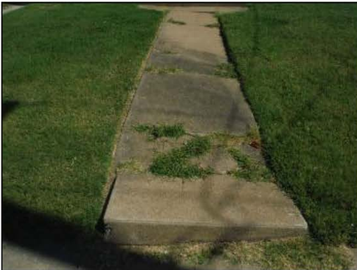
Common and larger cracks with lifting/settling to 1-2 inches, trip hazards
