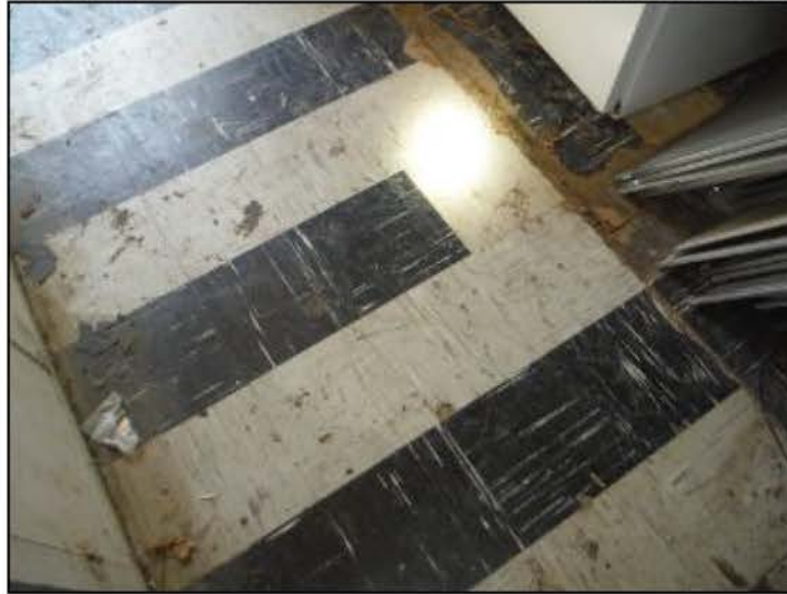
Suspect asbestos at 9"x9" tiles
