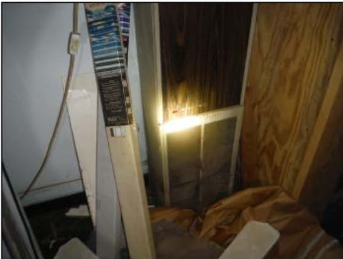
Old rusty unit needs to be replaced
