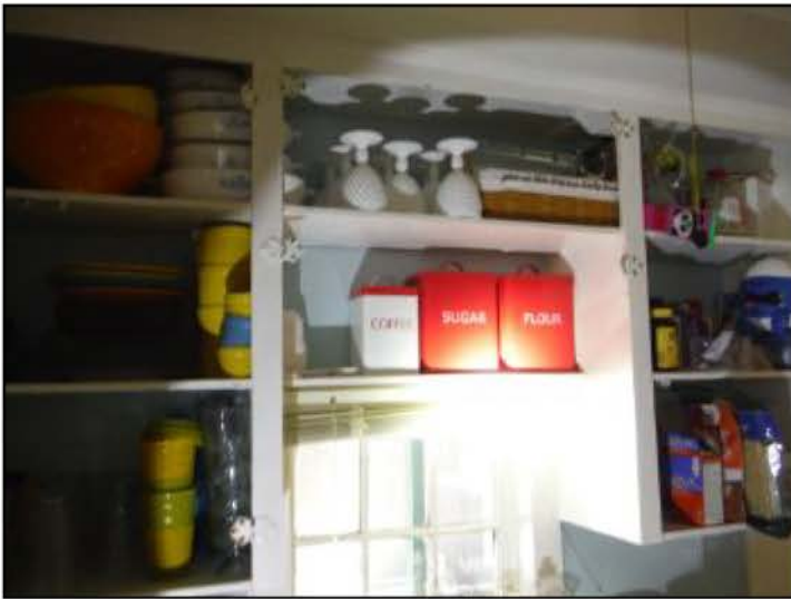
Missing cabinet doors
