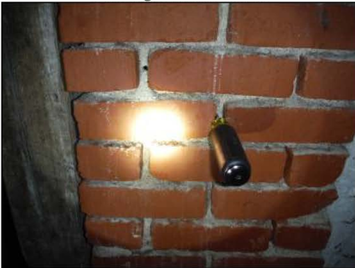
Deteriorated mortar at basement
