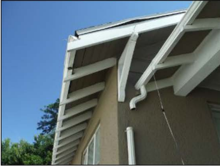
Rusted/damaged/incomplete guttering needs removal/replacement
