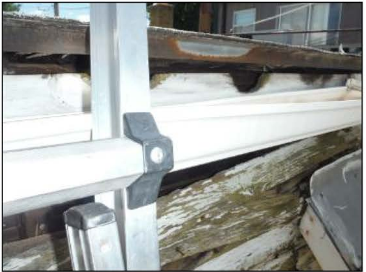
Lone gutter needs maintenance
