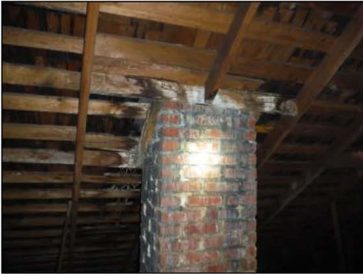
Stains appear dry
