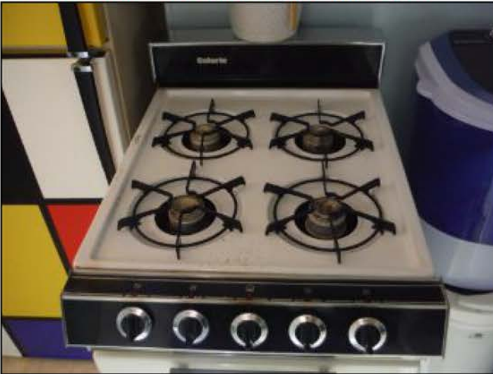
Did not self light, safety hazard, needs immediate repair
