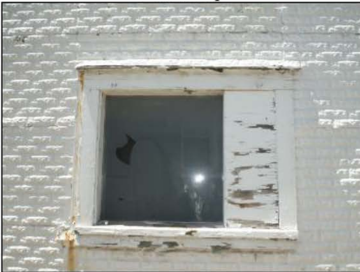
Broken unit/s are potential liability
