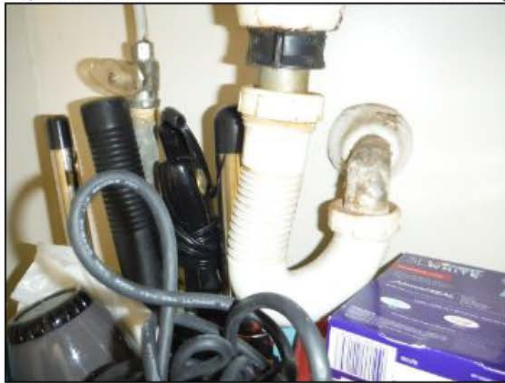
Tiny leak at loose trap
