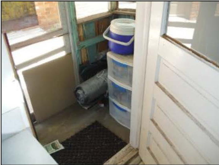
Uneven/cracked concrete floor noted
