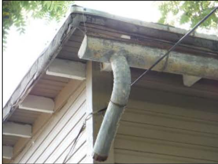
Partial system needs maintenance
