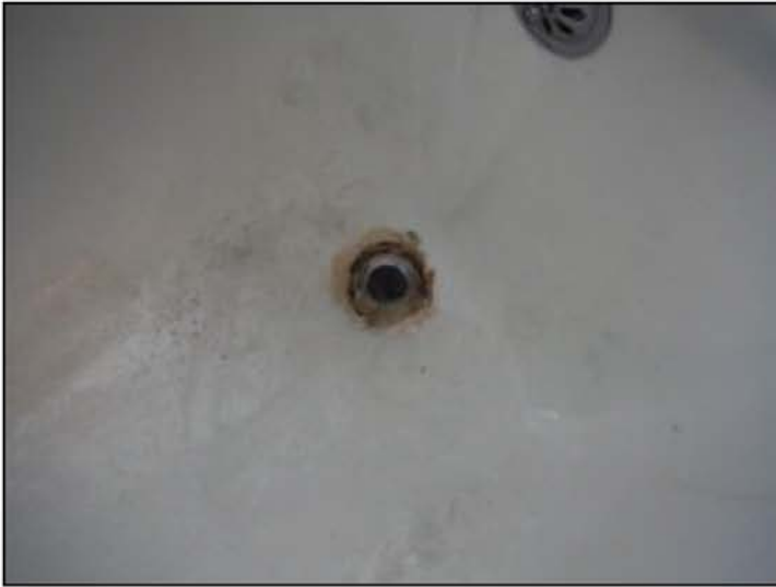
Serviceable though stopper missing and stains/wear noted
