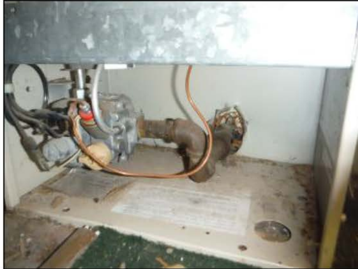
Untested older unit needs upgrade/replacement
