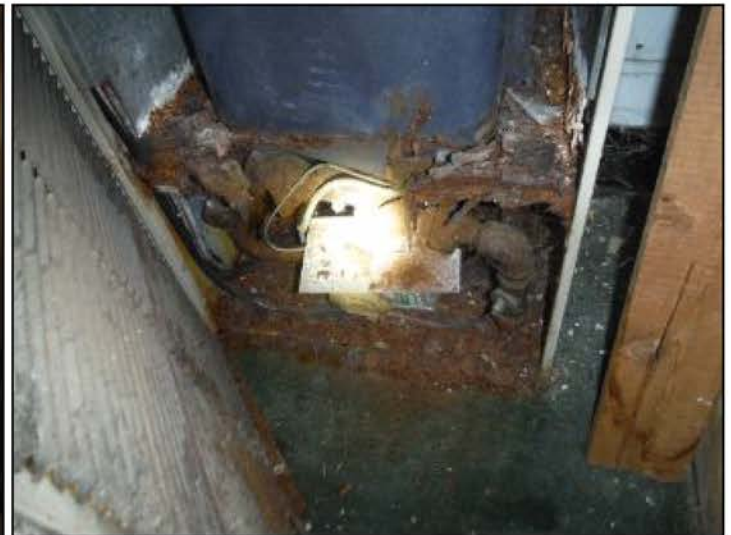
Old rusty unit needs to be replaced
