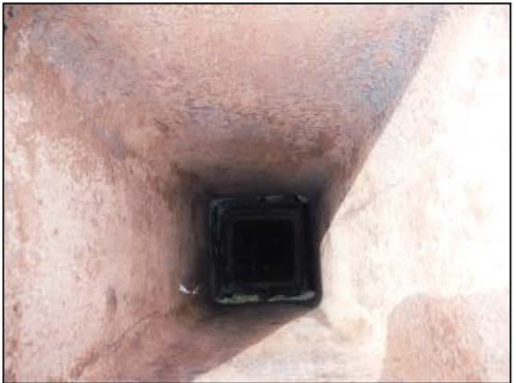
Flue is clean
