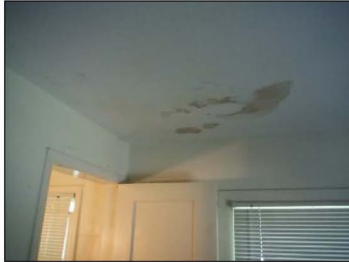
Stains appear dry
