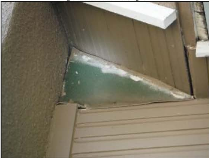
Missing wood lap siding at back eave
