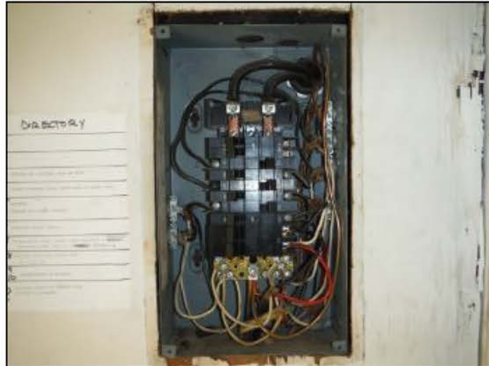
Serviceable older 100 Amp breaker panel
