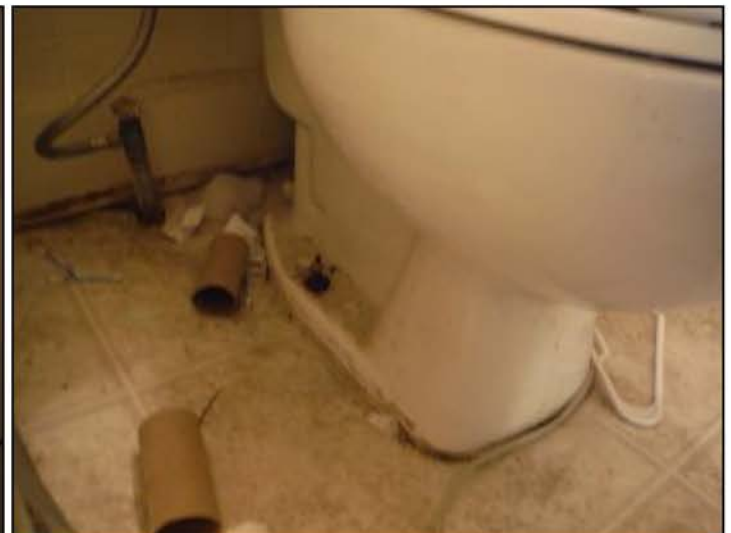
Loose at floor, needs resetting by plumber
