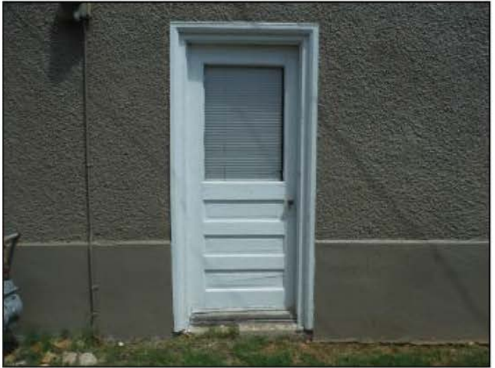
Untempered glass not to current standards
