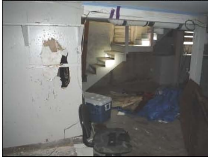
Damaged finish limits inspection
