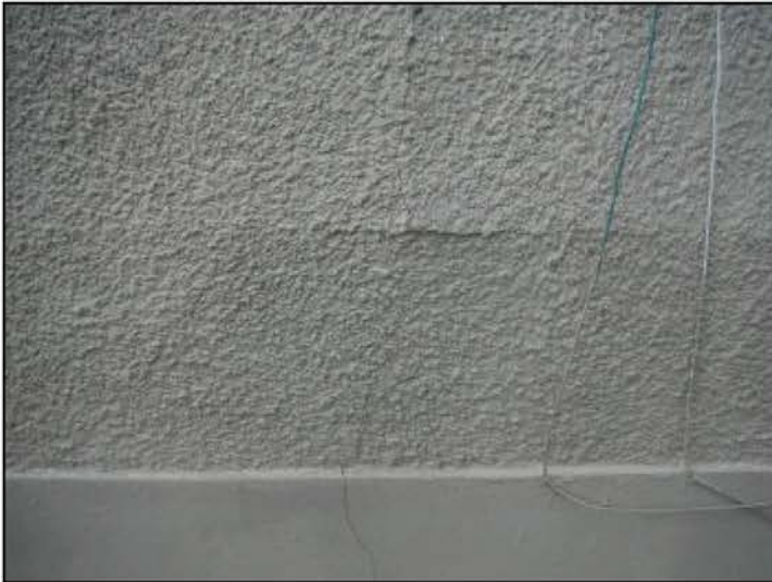
Loose/bulged at east side, refer to qualified stucco plasterer (closeup)
