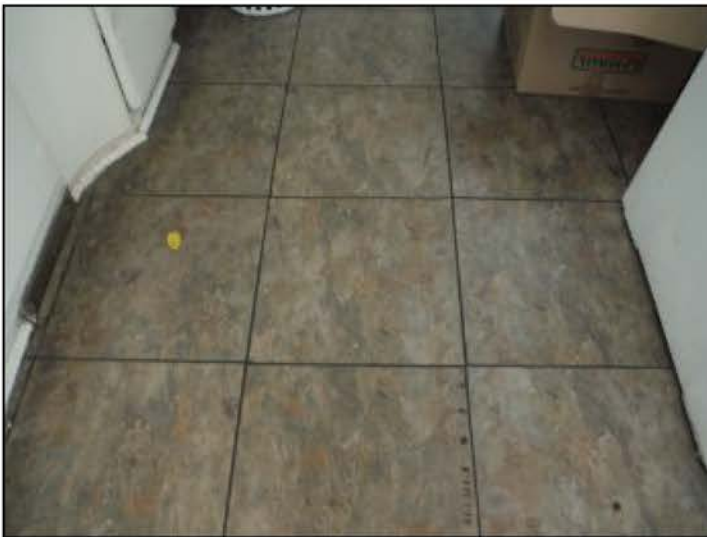
Uplifted vinyl tiles at kitchen
