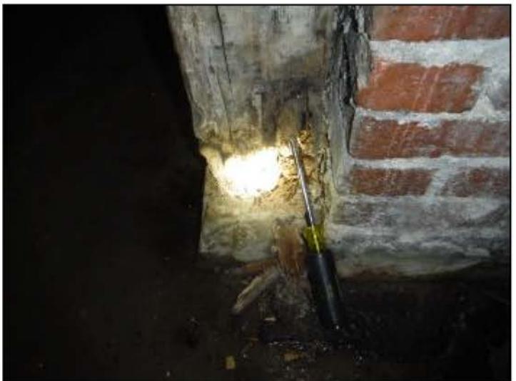
Rotted posts, refer to termite inspection report
