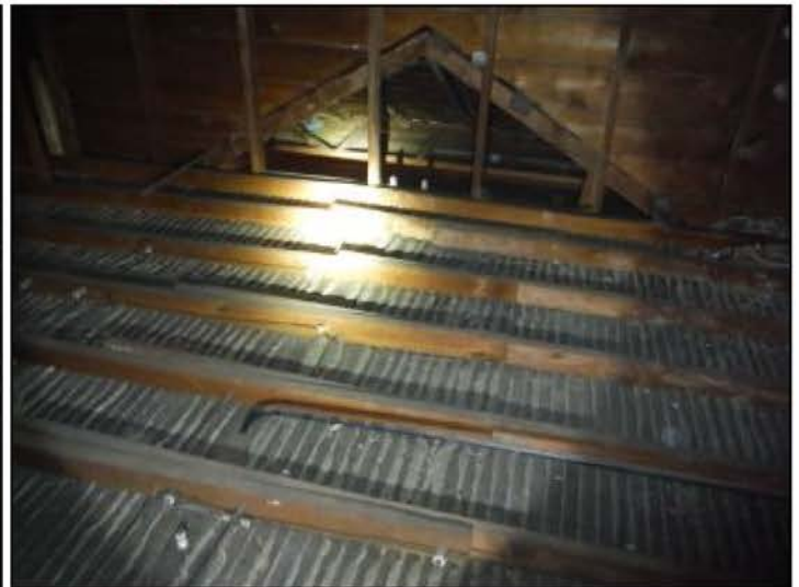
Active knob and tube wiring needs upgrading prior to adding insulation
