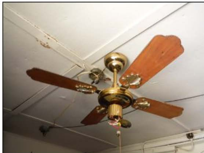
Inoperative fan (or switch not found)
