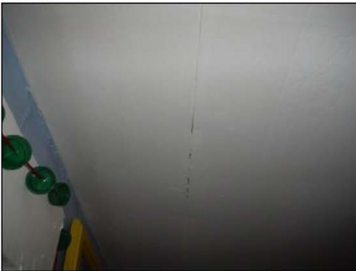
No access at ceiling, patched areas noted
