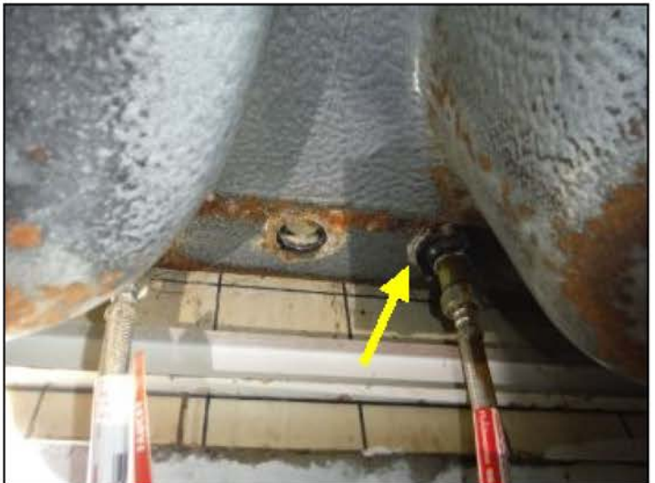
Leak/s at supply/faucet below, refer to plumber
