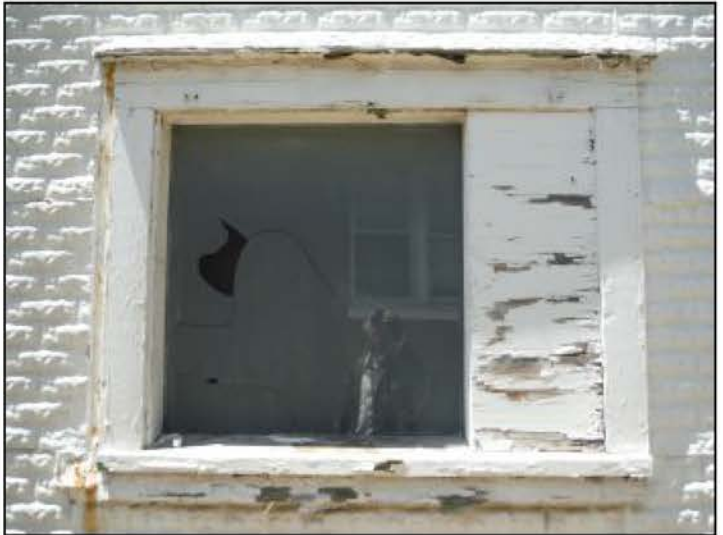
Broken unit/s are potential liability
