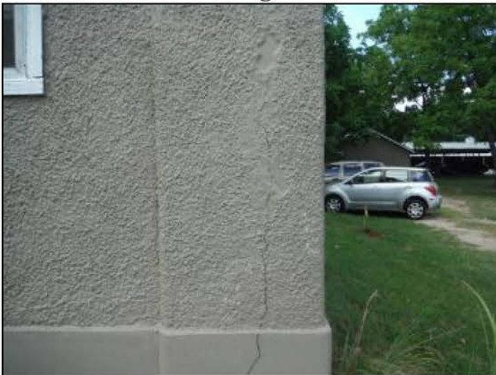
Common cracks at stucco
