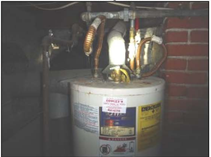
Vents gas water heater and furnace, old standard may not be allowed
