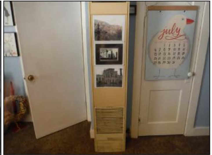
Older wall heater has limited economic lifespan, is fuel inefficient, hazardous and obtrusive
