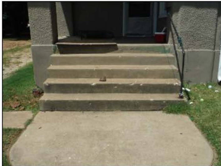
Hand railings not to current standards
