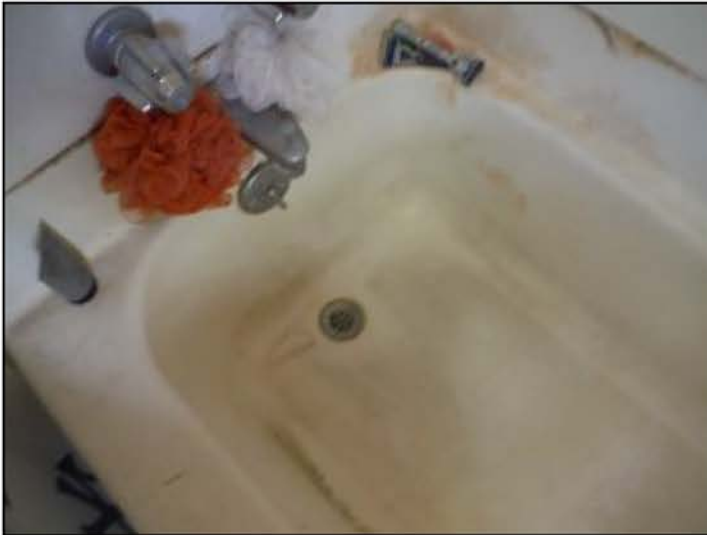
Stains, missing stopper
