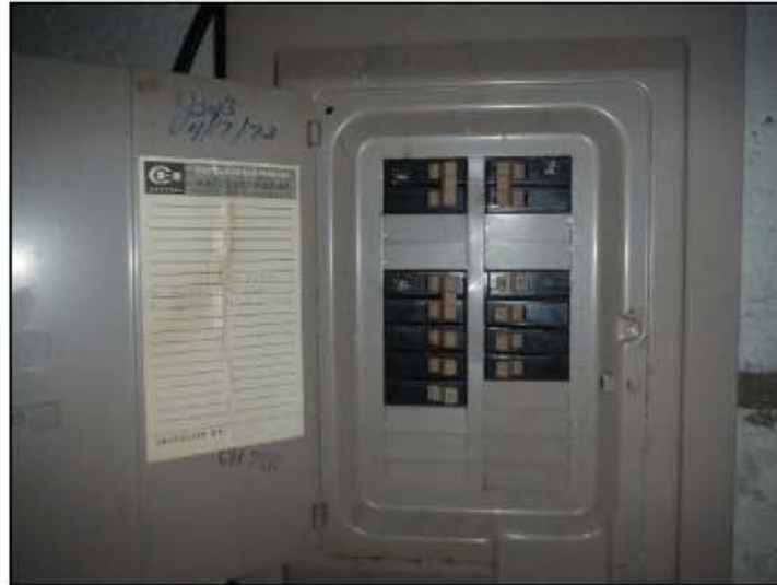
No main breaker, lug type panel (old school as installed)
