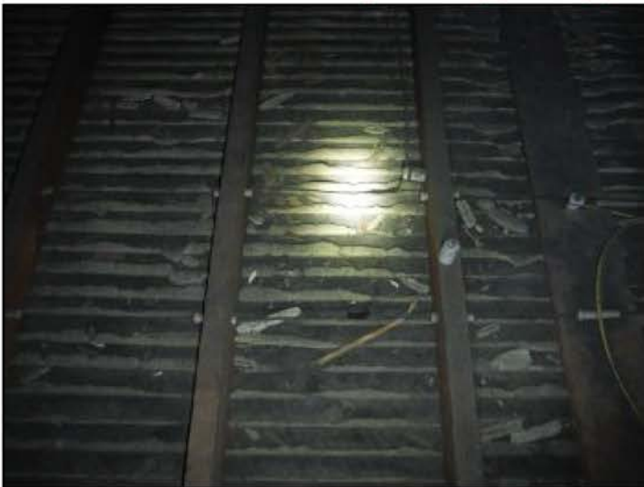
Active knob and tube wiring confirmed at attic, refer to qualified electrician to update
