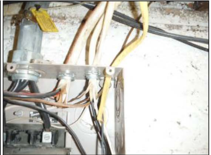
Missing wire clamps as installed
