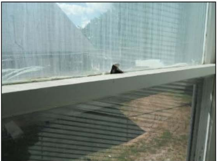
Broken window is hazard/liability
