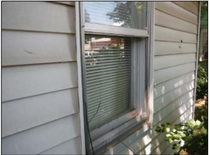
Most windows are inoperative or have serviceability issues
