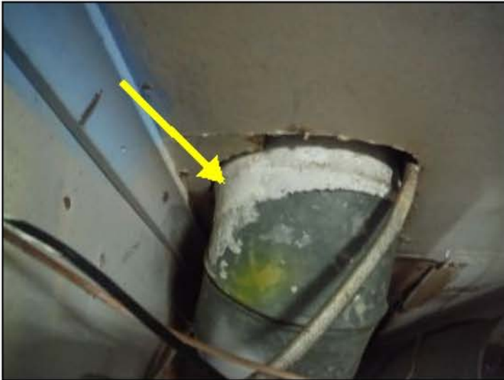
Suspect asbestos tape at ductwork noted
