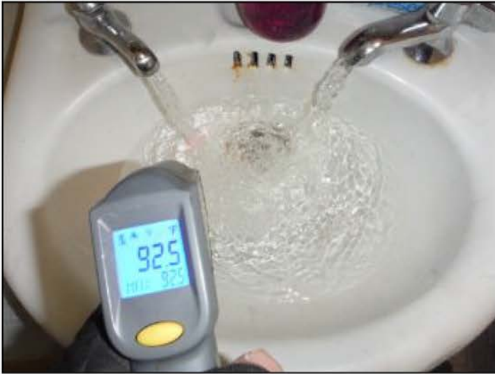
Not mixer valves, hot on left
