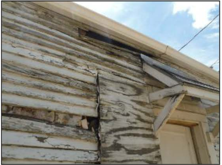
Closeup of deteriorated wood siding at back
