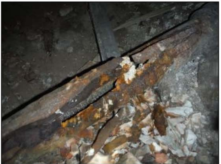
Wood debris needs removal (refer top termite inspection report)
