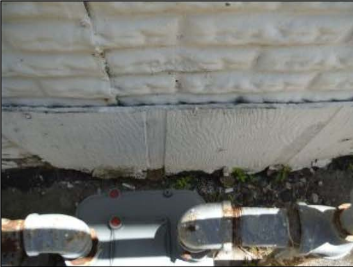
Skirting/siding conceals access at back
