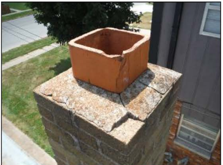
Refer to mason, deteriorated crown and top tile noted
