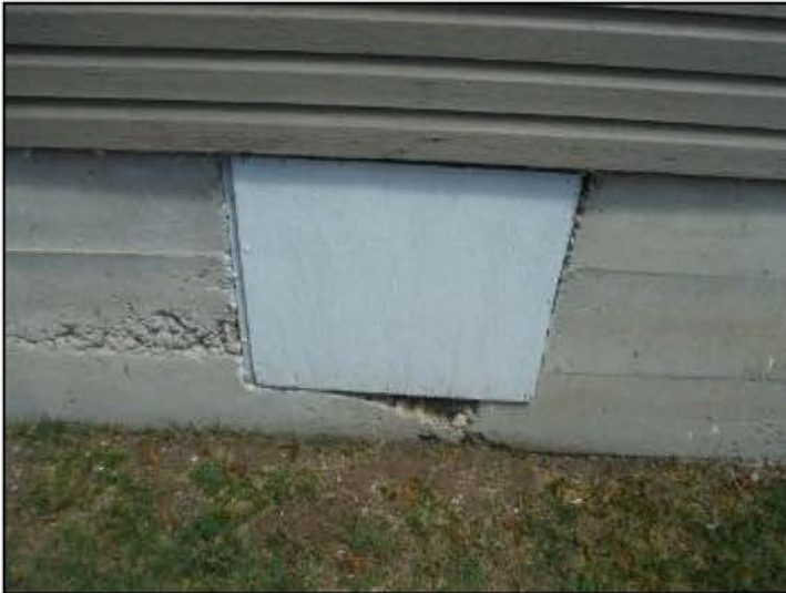
Access cover is secured
