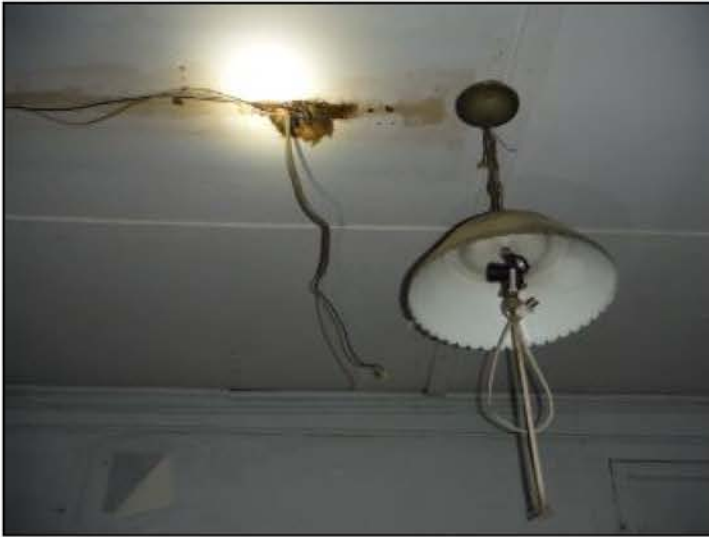
Unsecured wiring, refer to electrician
