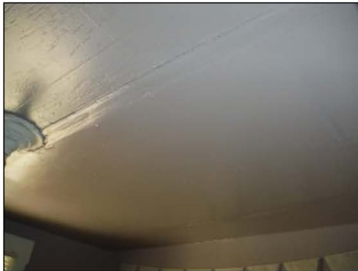
No attic access at ceiling, patched areas noted
