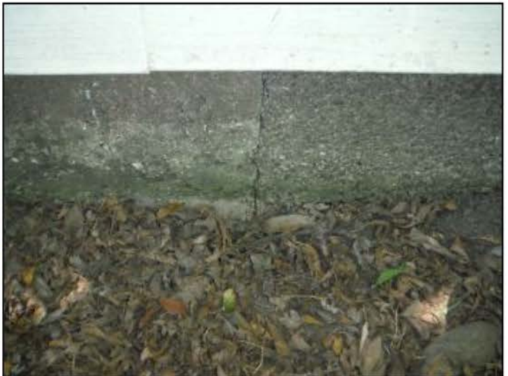
Cold joint means half is an addition
