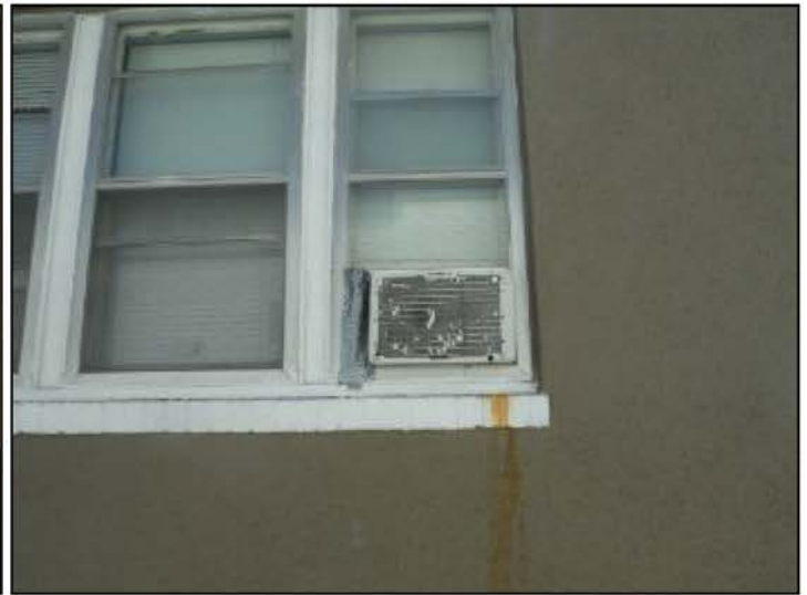
Missing screens/sashes noted
