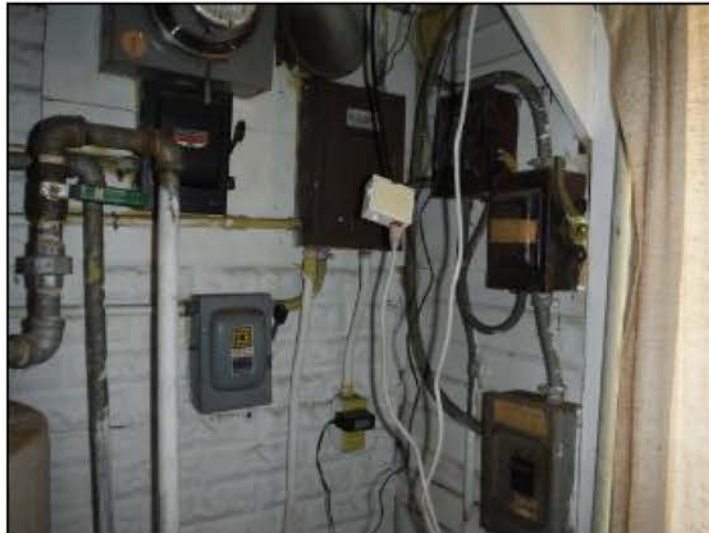
Multiple fuse panels/subpanels, not to current standards for commercial property
