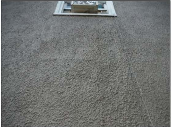
Loose/bulged at east side, refer to qualified stucco plasterer
