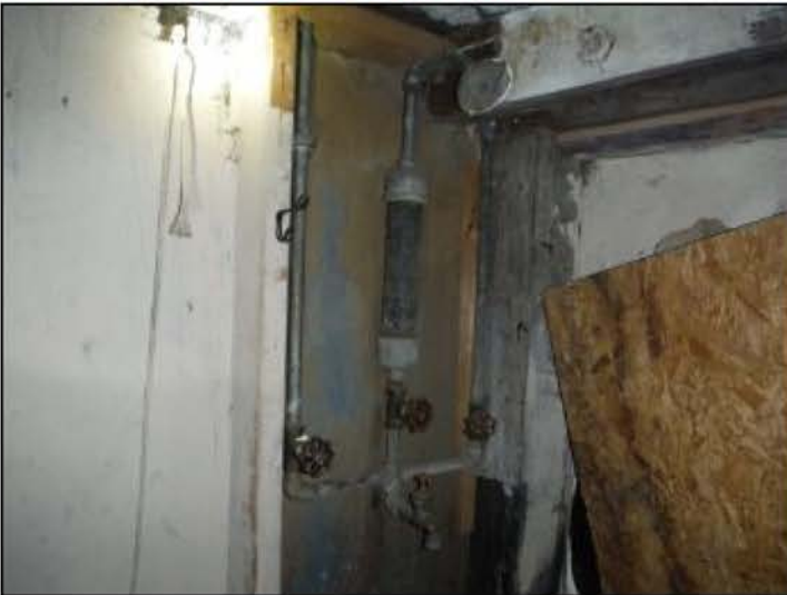
Untested abandoned shower in basement
