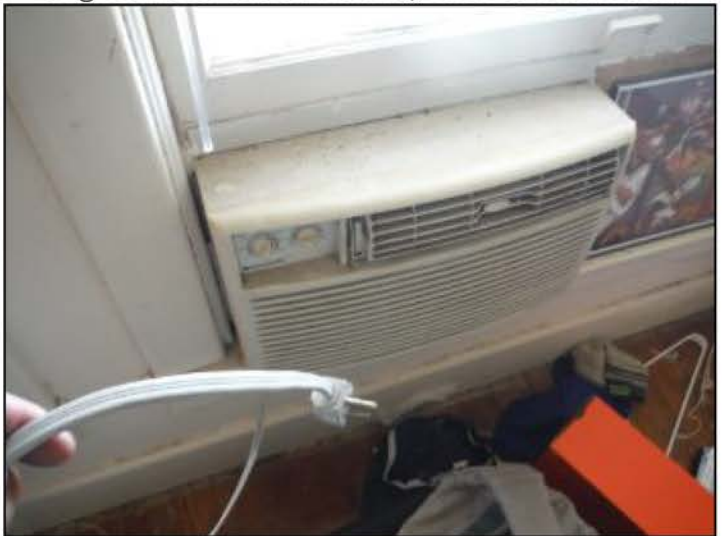
This A/C unit requires extension cord, no outlet nearby
