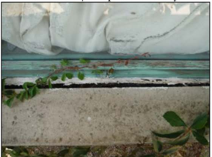
Broken unit/s are potential liability
