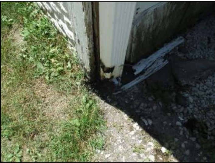
Lone downspout needs splash block
