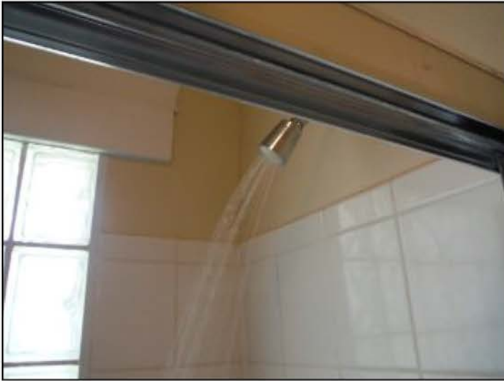
Low head clearance noted at top door track
