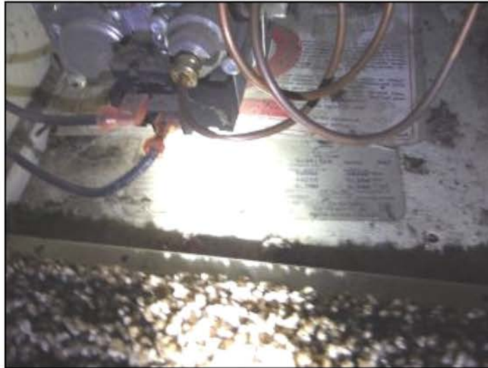
Burns room/conditioned air (inefficient)
