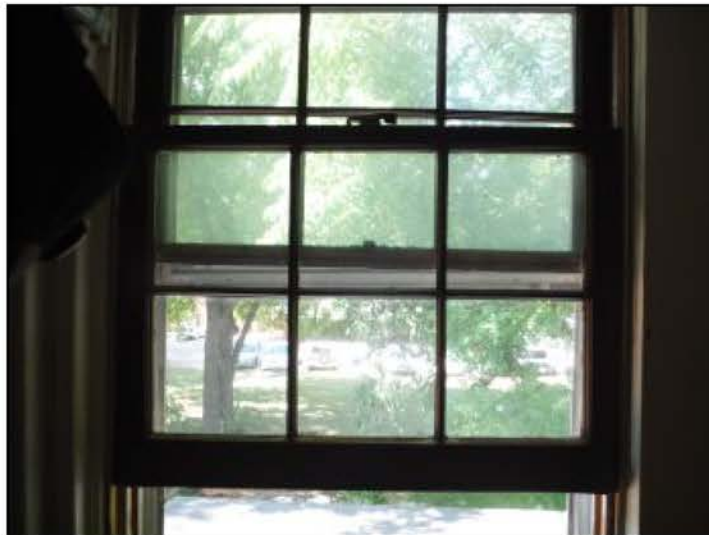
Window needs maintenance repairs
