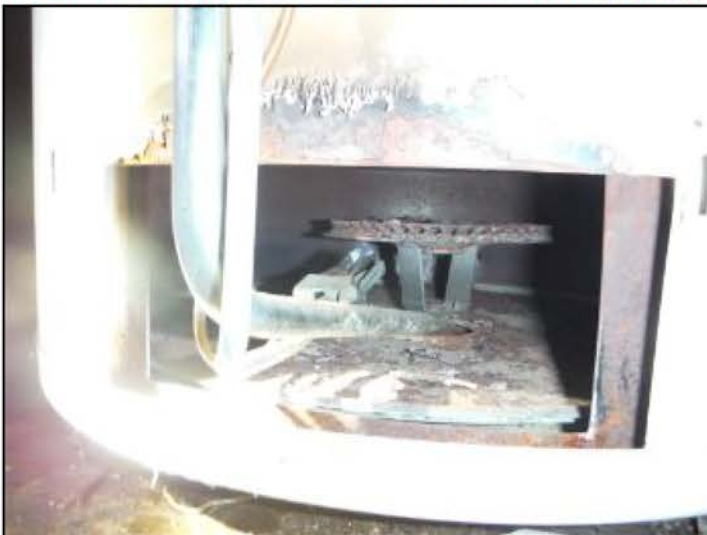
Rusted older unit has limited life
