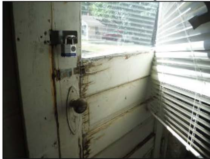
Basement unit is moisture damaged
