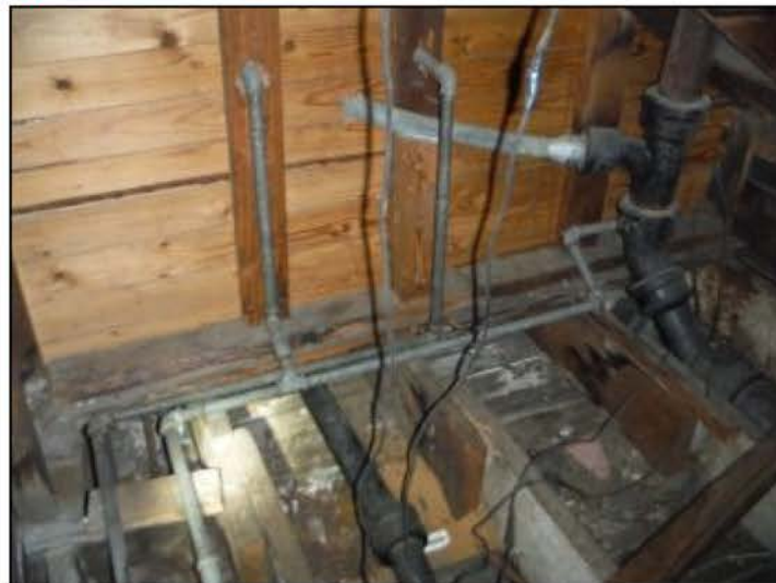
Plumbing needs insulating
