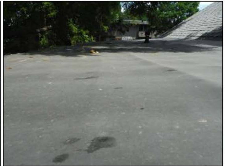
Spongy, stains are sign of ponding
