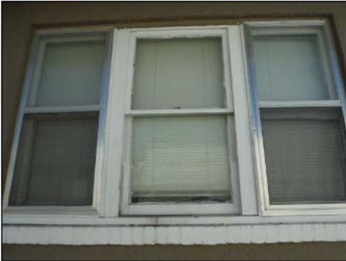
Refer to window specialist, need either upgraded with replacement windows or much overdue maintenance for serviceability
