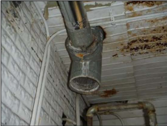
Disconnected (abandoned status)
