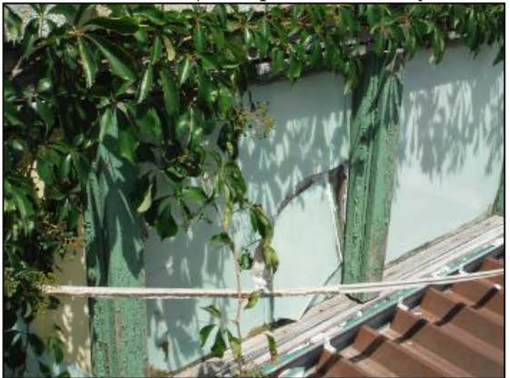
Broken unit/s are potential liability
