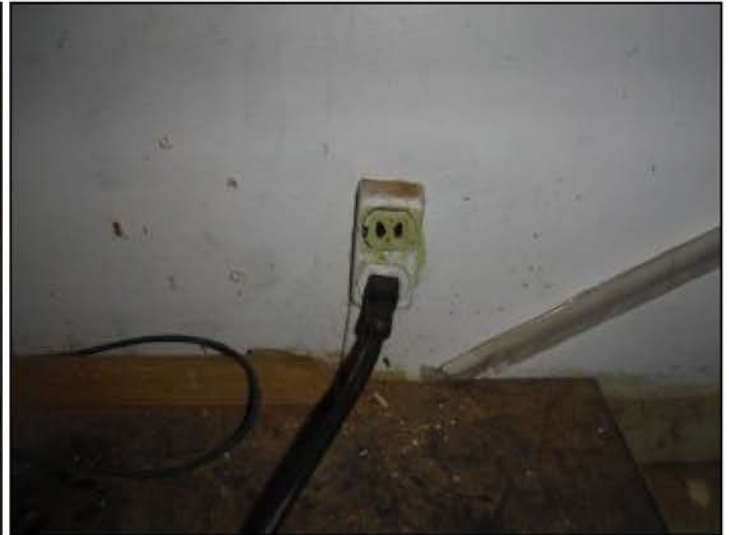
Dated two wire system, not to contemporary standards for commercial property
