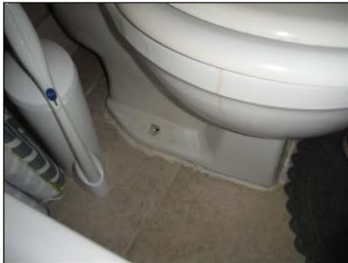
Caulked base not preferred
