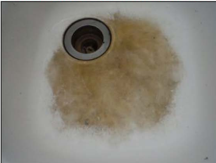
Serviceable unit, stains/wear noted
