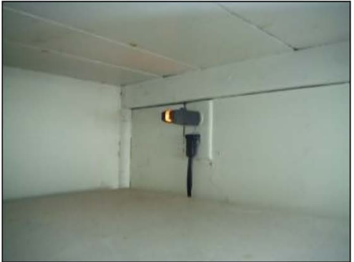
Ungrounded outlets found, refer to electrician
