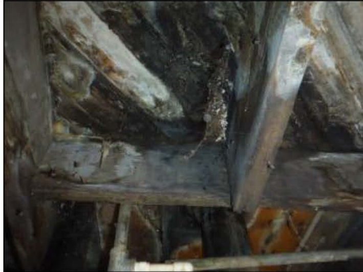
Unrepaired minor damage below half bath observed
