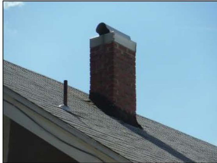
Vents water heater and floor furnace
