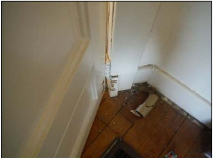
Damaged upstairs unit
