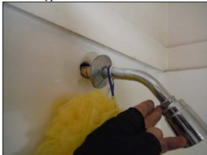
Showerhead is loose, leaks
