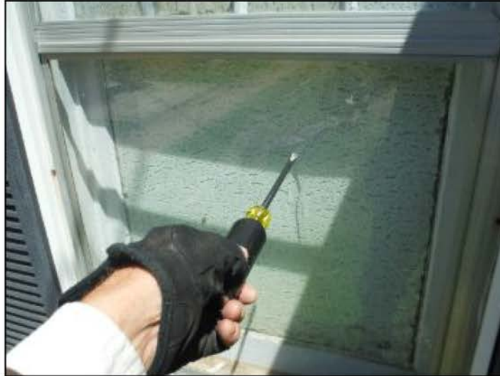
Cracked glass needs repair
