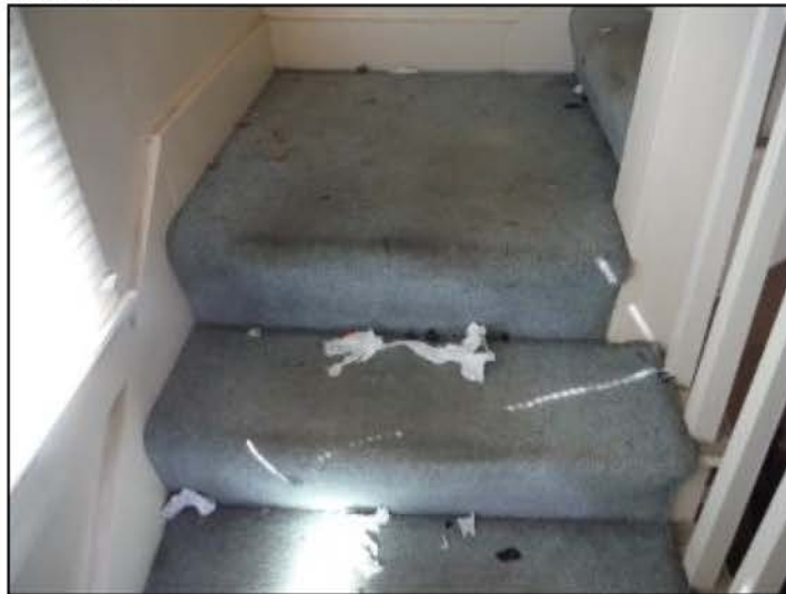
Damaged carpet at main stairs is trip hazard issue, needs correction
