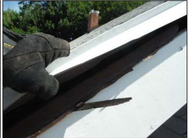
Multiple layers: Two or more composition overlay original wood shingles (which with gapped sheathing are substrate for composition)
