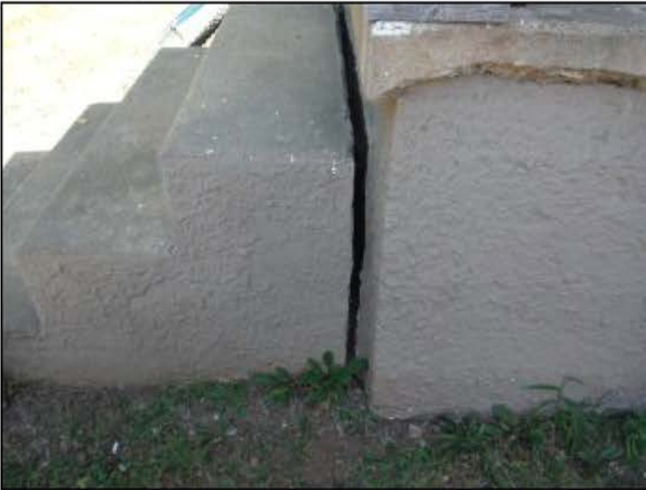
Settling has caused wide gap to develop at stoop, no action needed
