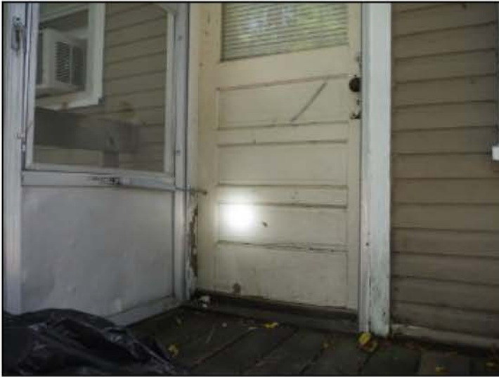
Untempered glass not to current standards
