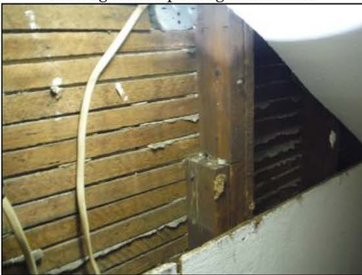
Uninsulated, old standard not yet upgraded
