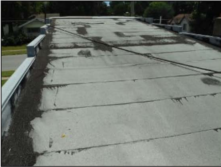
At end of life, needs stripping and replacement ASAP
