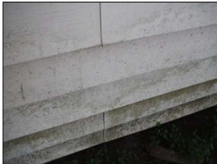
Fungal stains at vinyl siding need cleaning
