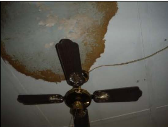
Stains and water damaged ceiling, sign of roof issues
