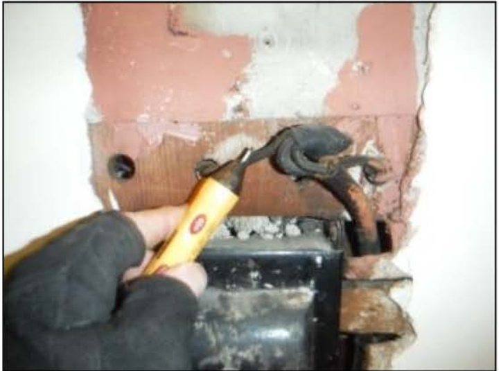
Unsecured wiring (exposed wiring/splices/open junction boxes) observed at basement stairwell, refer to electrician to cleanup/secure
