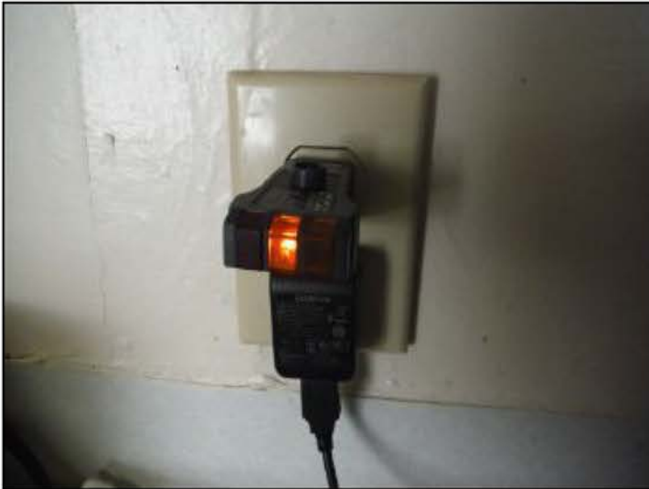
Ungrounded outlets found, refer to electrician
