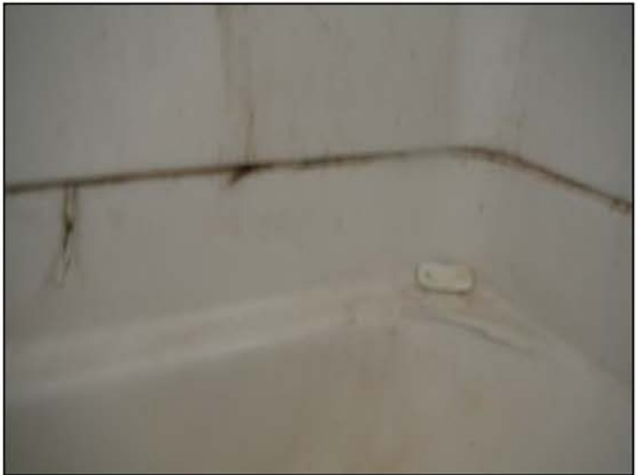
Seam needs recaulking
