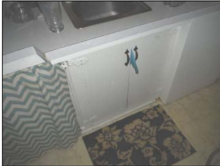
No toe space at sink cabinet
