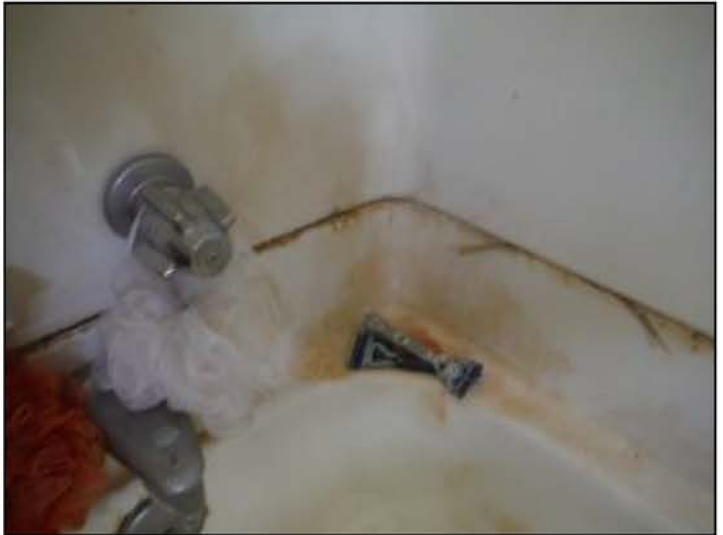
Seam needs recaulking
