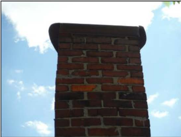
Refer to qualified mason for maintenance
