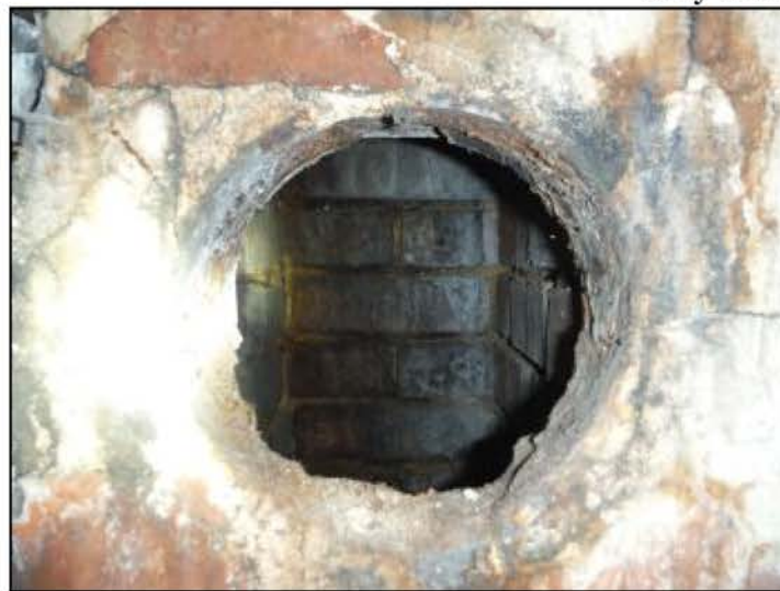
Open flue connection, needs capping off at attic (fire hazard)
