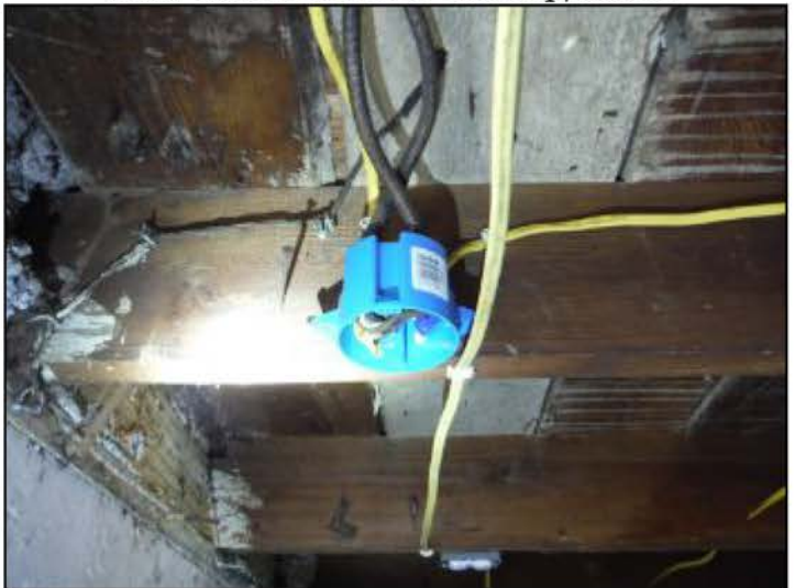
Unsecured wiring (exposed wiring/splices/open junction boxes) observed at basement and attic, refer to electrician to cleanup/secure
