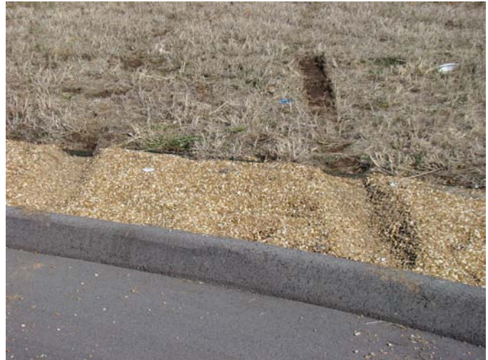
Evidence that motorists ignore paved roadways and create their own paths into or through the Redevelopment Area.
