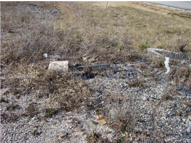
Deteriorated pavement left from demolition which occurred more than three years ago.
