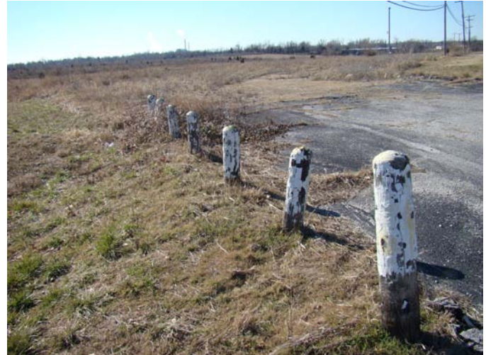
Deteriorated pavement and concrete bollards.
