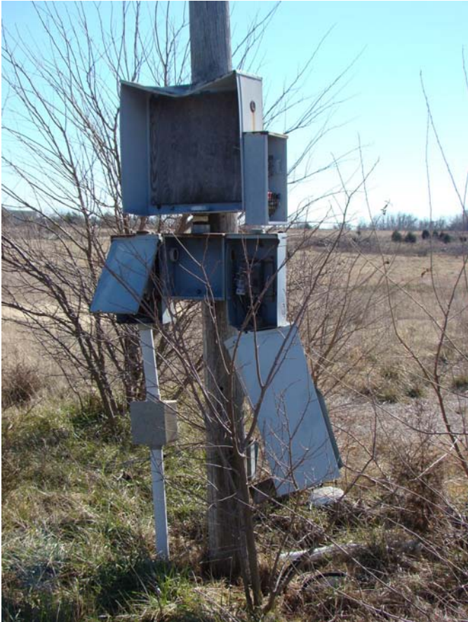
Damaged utility pole.
