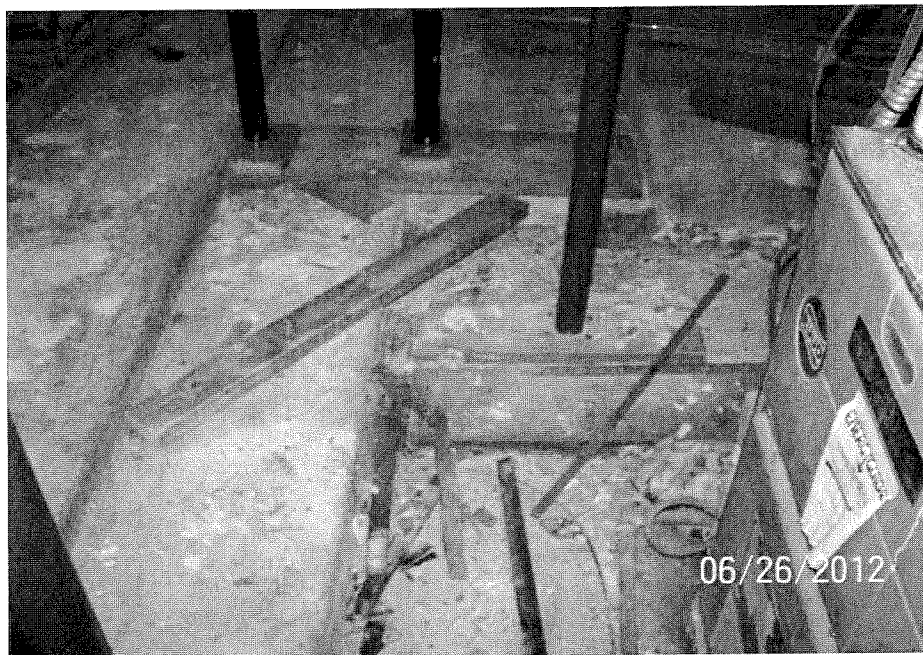
920 S. National – Basement debris, peeling paint, Previous structural repairs
