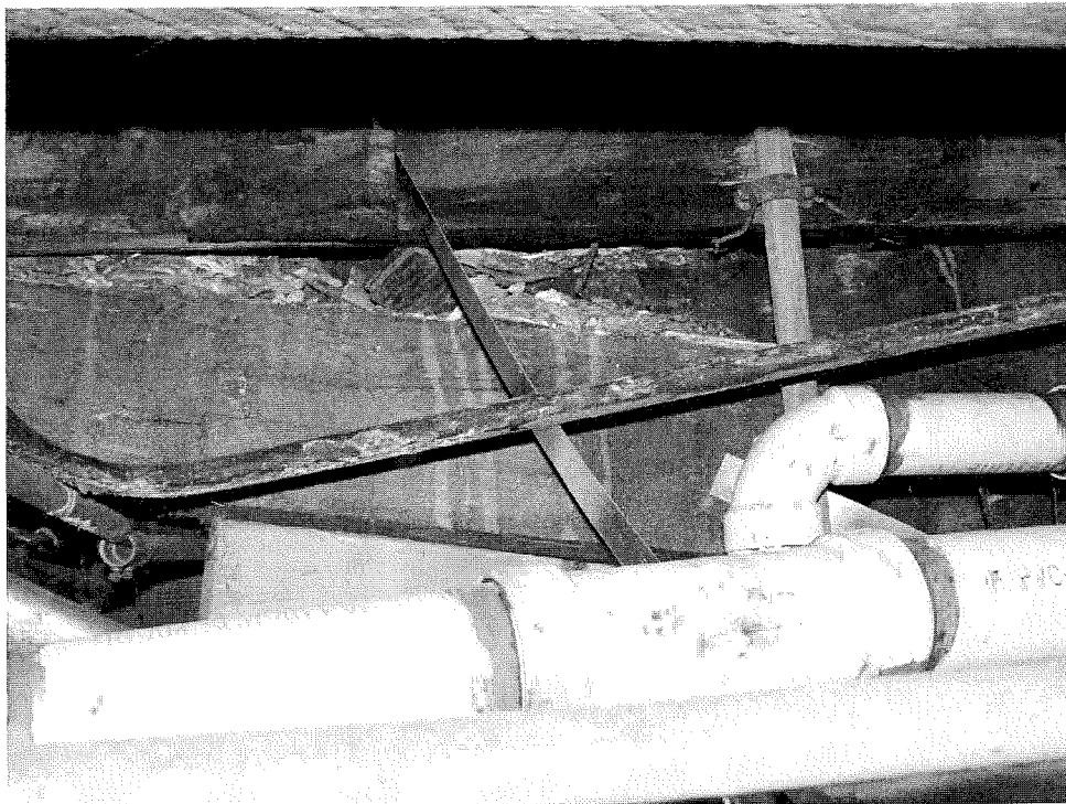
920 S. National – Broken floor joist, damaged pipes, exposed plumbing
