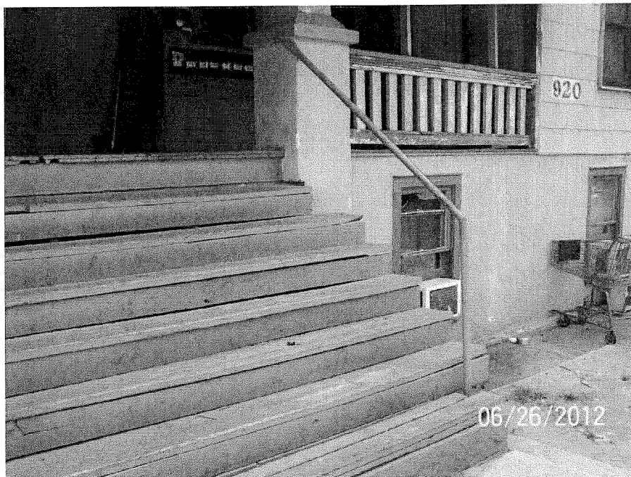
920 S. National – Front (West) Damaged, unsafe stairs
