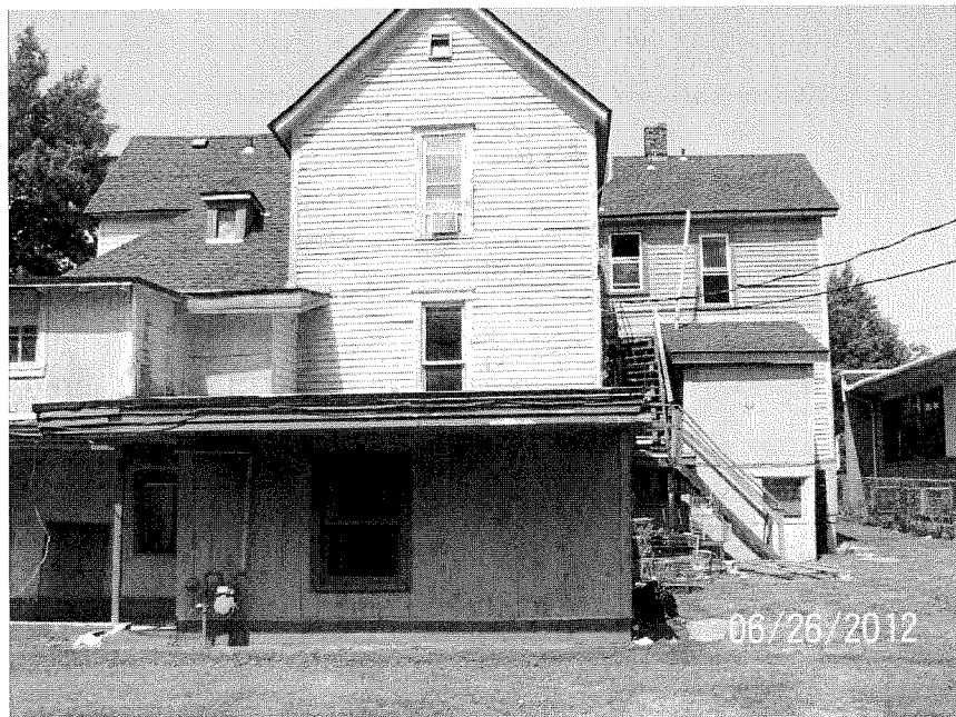
920 S. National – Back (East) Unsafe stairs
