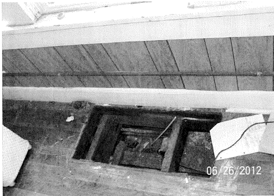
920 S. National – Damage to floor, hole to basement
