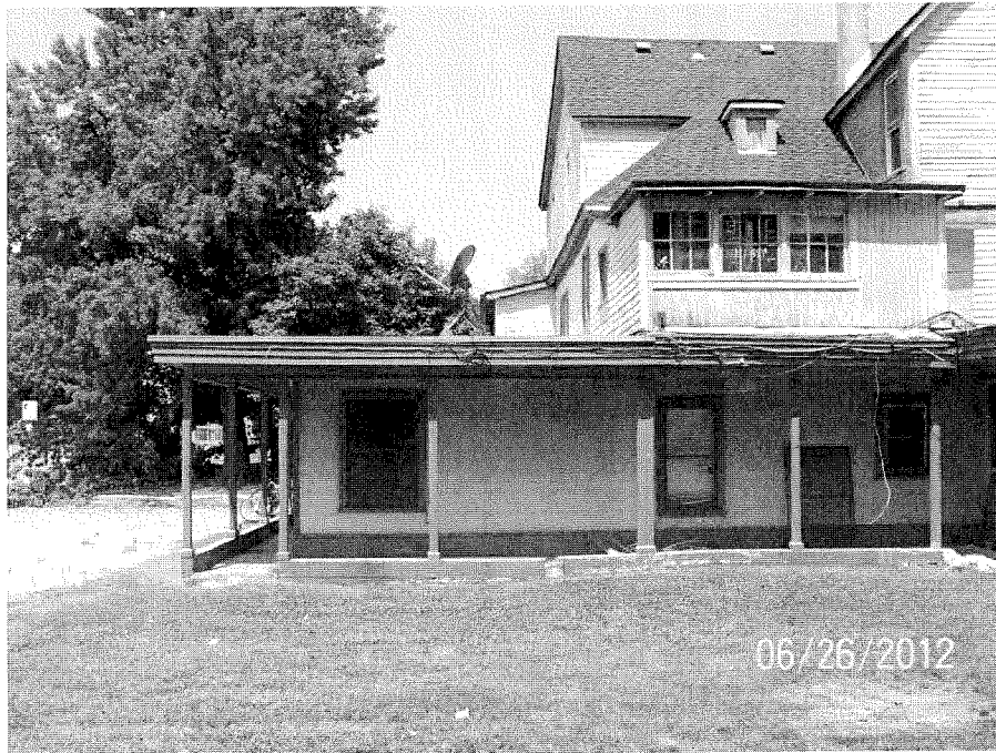
920 S. National – Back (East) Exposed wiring
