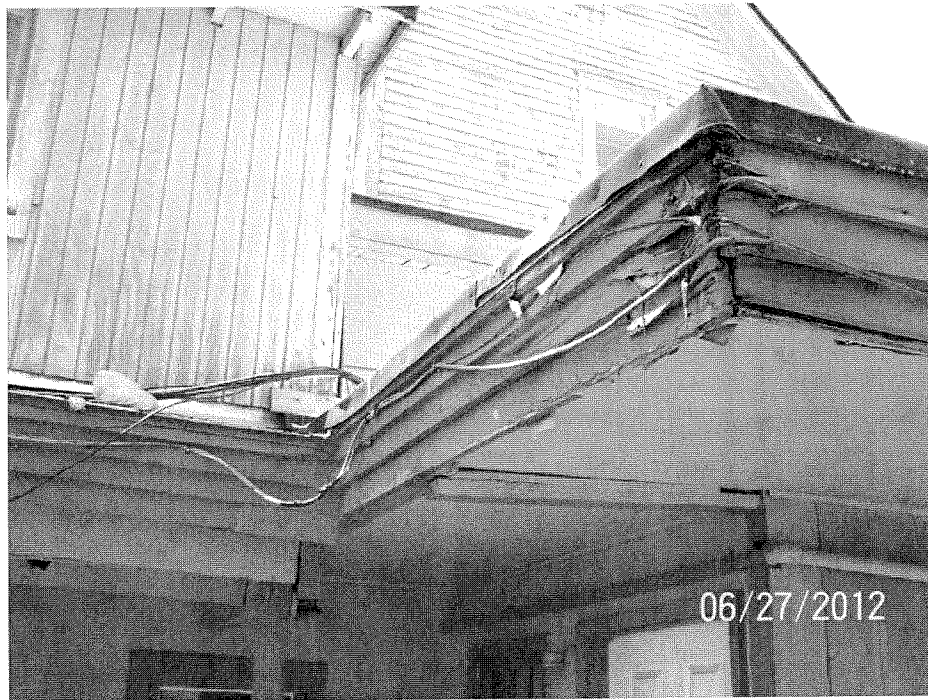
920 S. National – Back (East) Paint peeling, exposed wiring, damage soffit and fascia.
