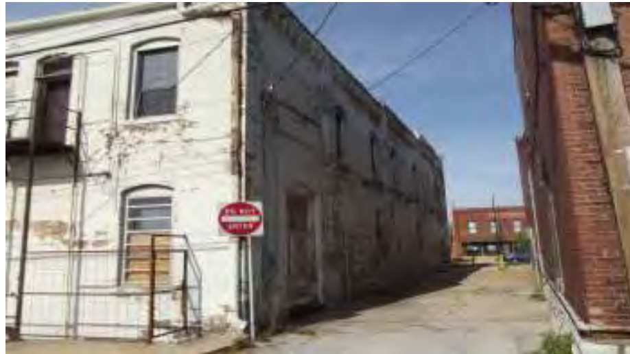
Existing Door to Be Replaced (2 nd Floor)
