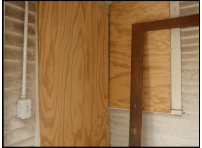
Boarded up doors/windows
