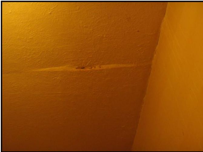
Unit #1 Sign of a Leak
