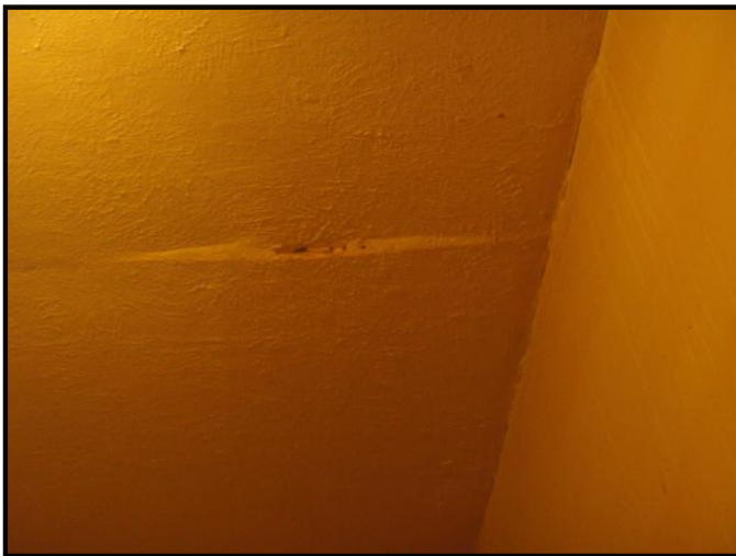
Unit #1 Sign of a Leak
