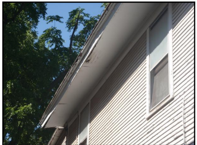
Rotting Soffit &amp; Fascia
