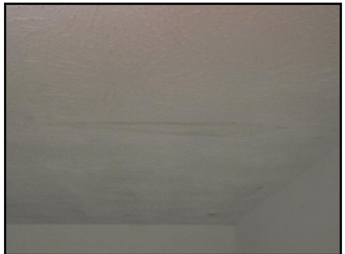
Unit #4 ceiling leak
