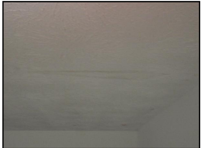
Unit #4 ceiling leak
