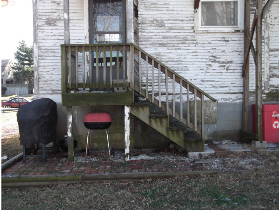
Foundation View from the North (shows foundation crack below crawl space entrance)
