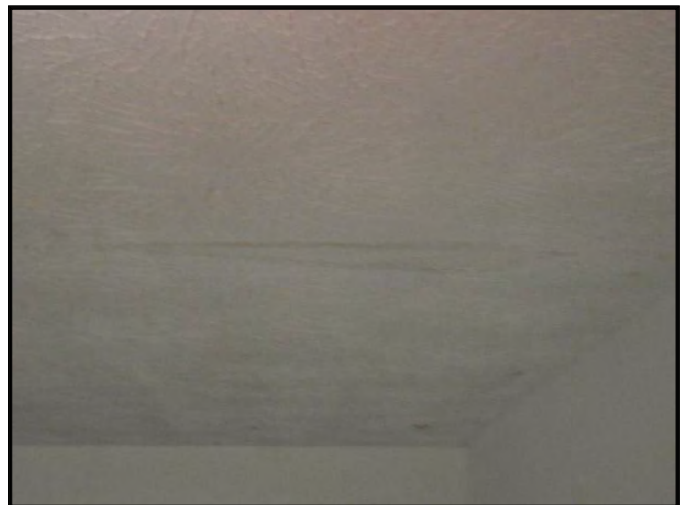
Unit #4 ceiling leak
