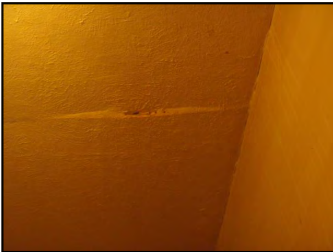
Unit #1 Sign of a Leak
