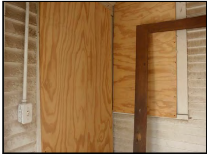
Boarded up doors/windows
