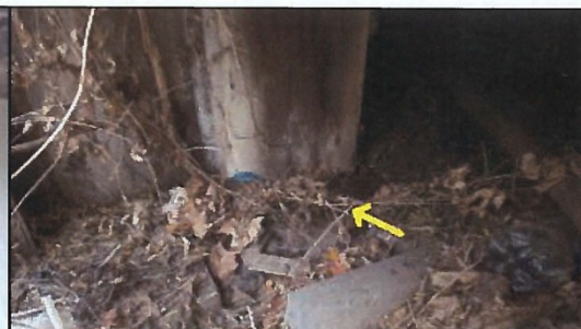
Wood to earth contact
