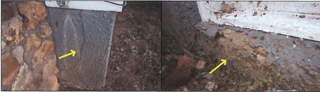
Crack at SE corner (1/2" displacement)
