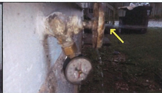
Rear faucet leaks
