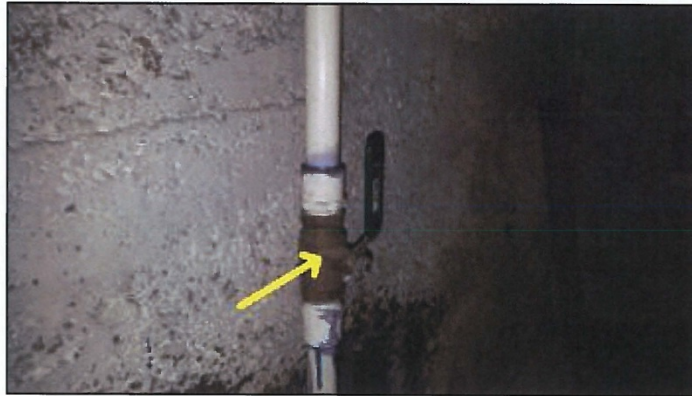
Main water shut off
