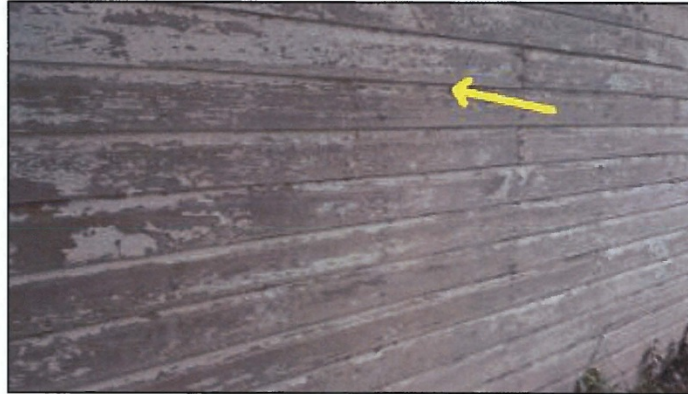
Worn paint on exterior
