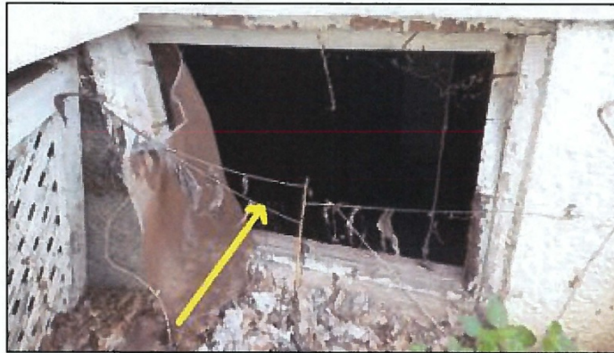
Missing basement window bear back porch.
