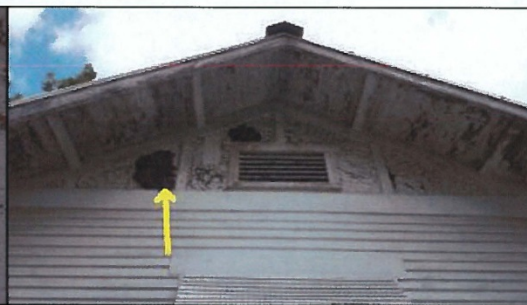
Holes in asphalt paper on West gable
