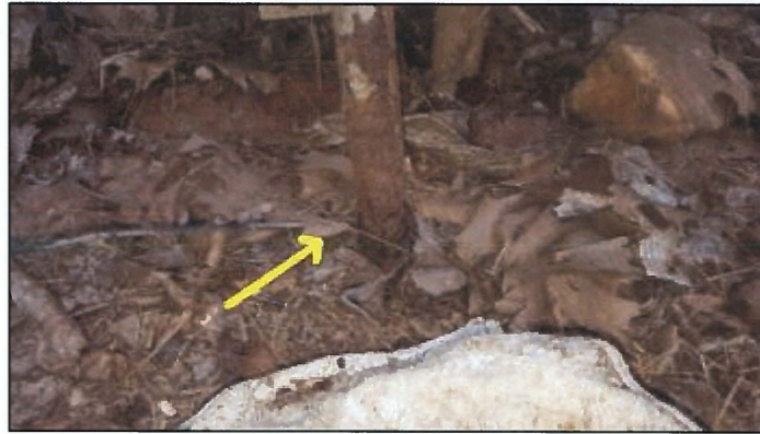
Heavily deteriorated main gas line
