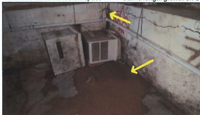
Signs of moisture penetration at NE corner (below downspout)
