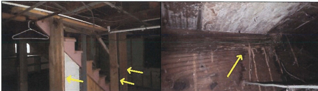
Floor and interior basement stairway poorly supported
