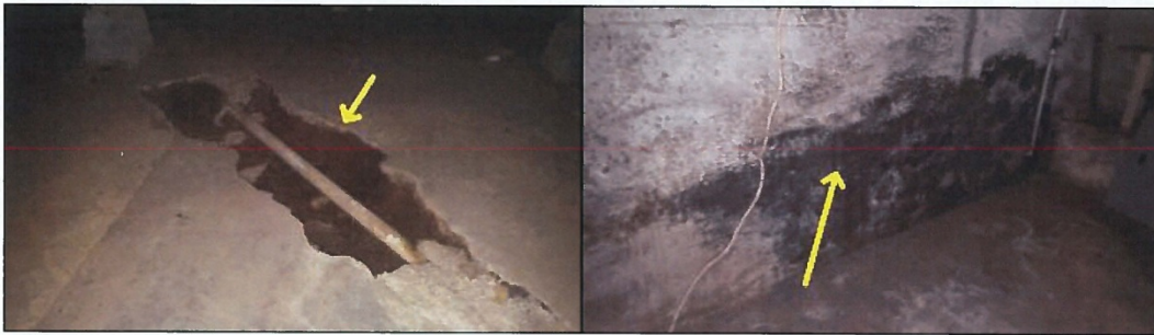
Large hole in concrete floor
