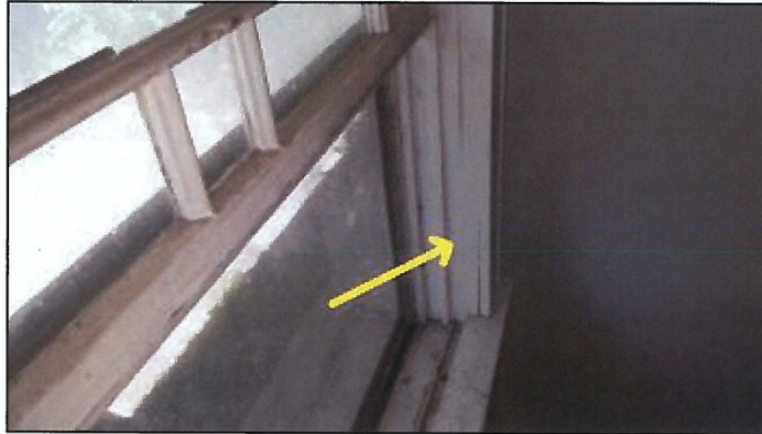
Lower dining room window is missing
