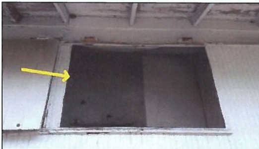
Missing shutter noted
