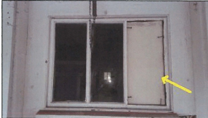
Missing glass at front door
