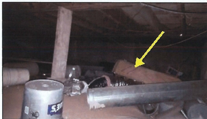
Construction debris in crawlspace
