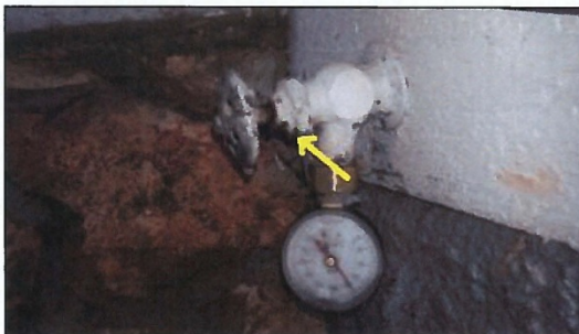
Front faucet leaks under pressure
