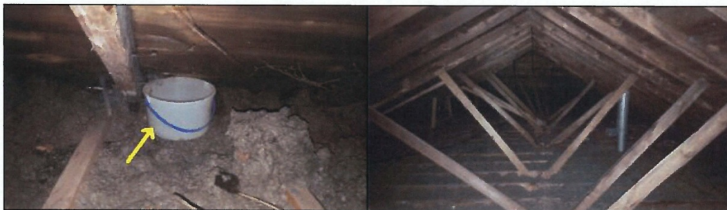
Bucket indicating past leak
