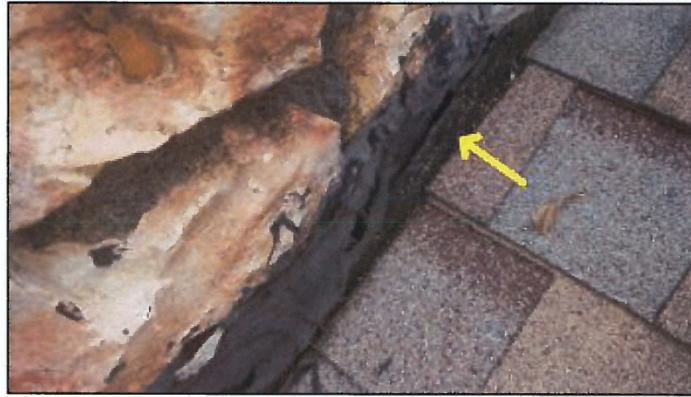
Improper and loose flashing at front chimney
