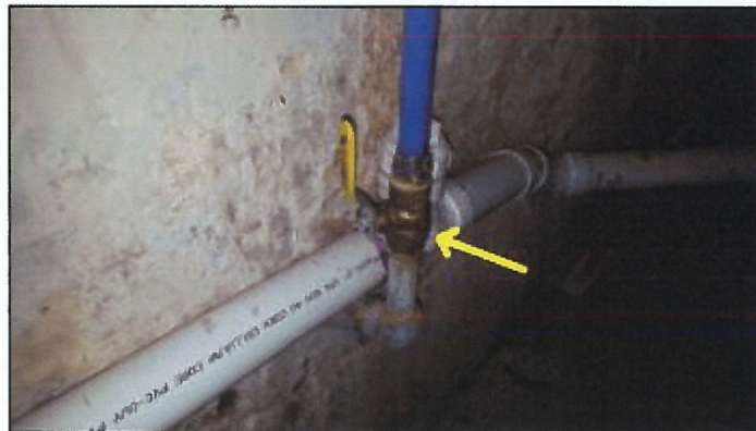
Main water shut off
