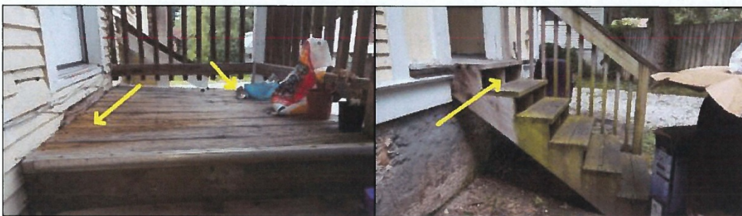
Landing has settled - Unit 3
