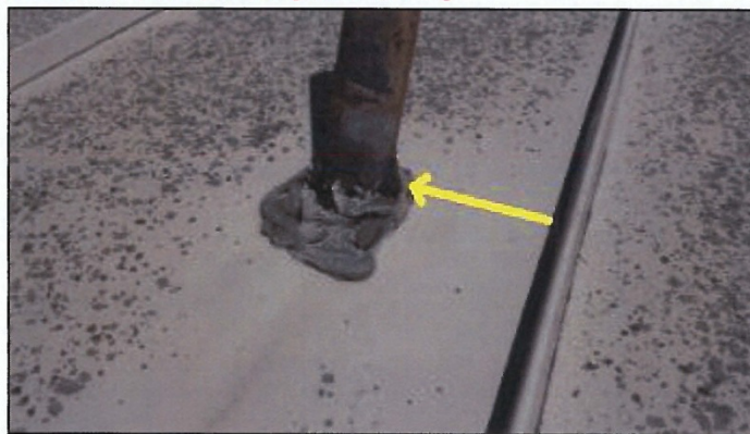
Kitchen plumbing vent
