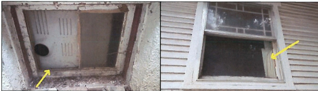
Missing window on back wall of basement
