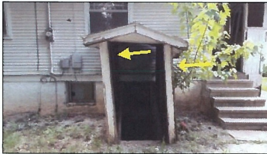
Stairway covering damaged and leaning
