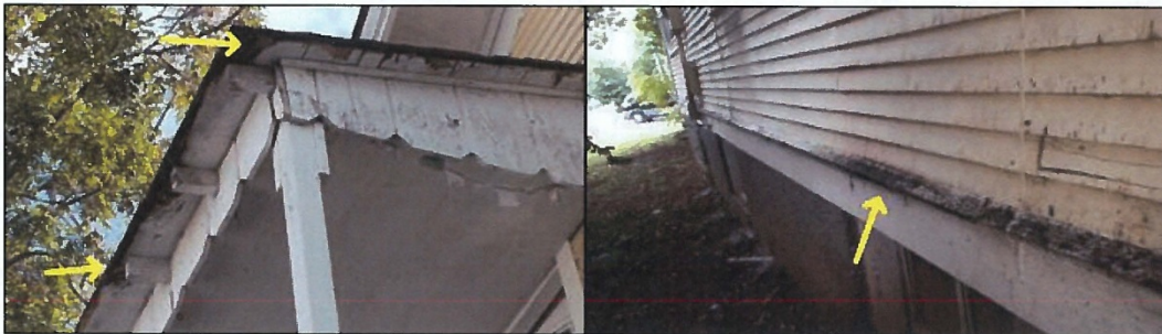
Deterioration above door to unit three
