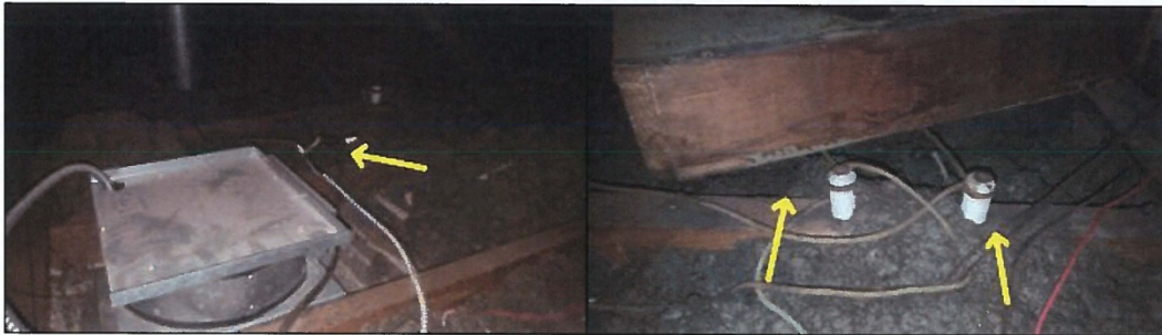
Exposed splice near access
