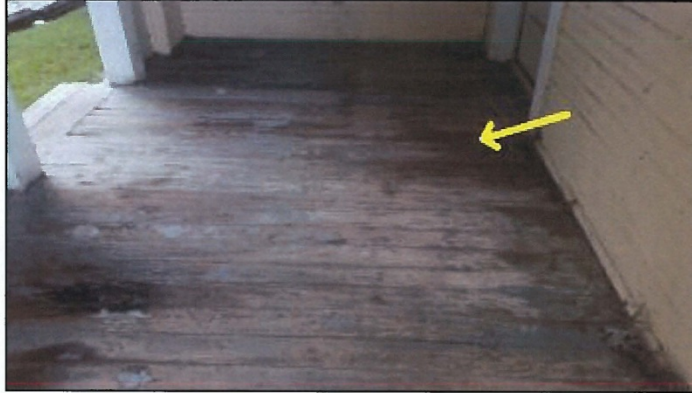
Back porch needs maintenance
