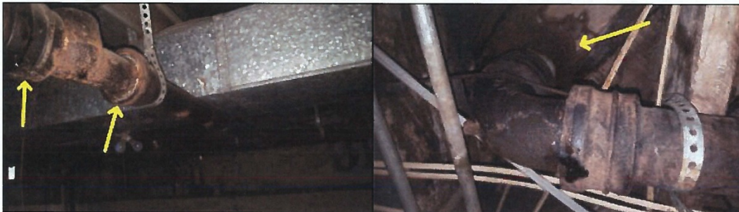
Several unions leak in basement.
