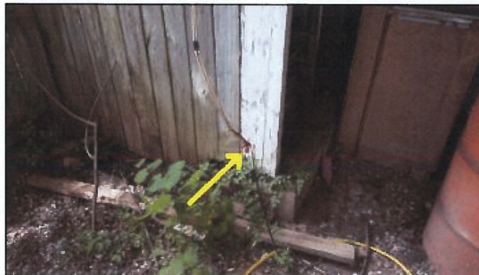
Cord with exposed splice powers garage
