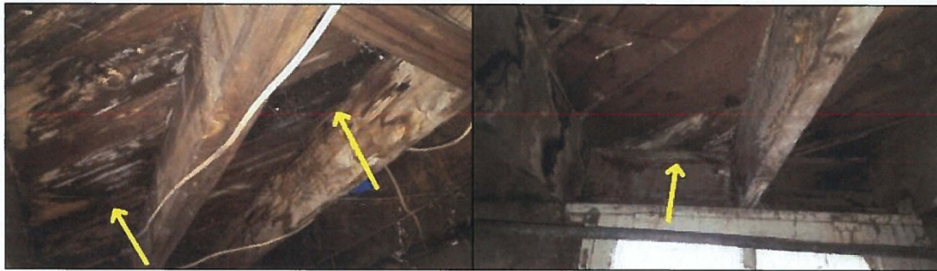
Fungal growth and damaged subfloor in NW portion of basement
