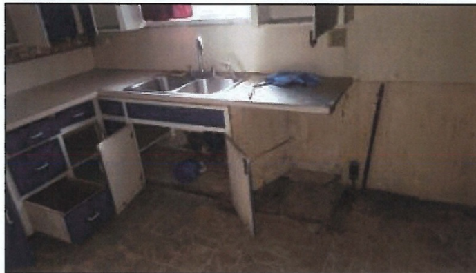
Kitchen is in poor condition overall.
