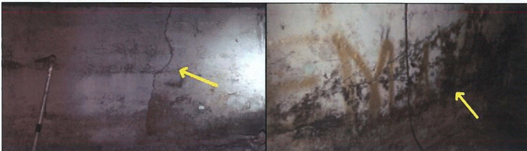
Small crack in SW corner of basement/crawlspace
