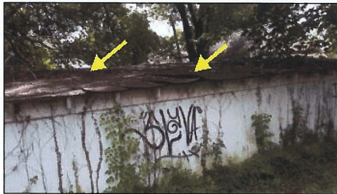
Garage roof in poor condition and covered with branches/debris
