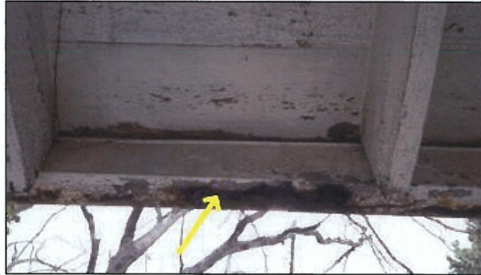
Gutters rusted through
