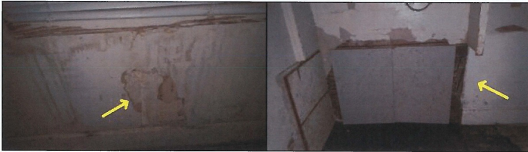
Moisture stains and cracks
