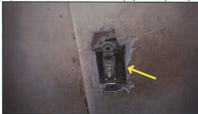
Outlets and switches missing plates l'm various locations.
