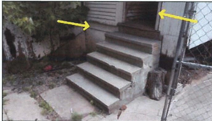
Handrail needed at back steps
