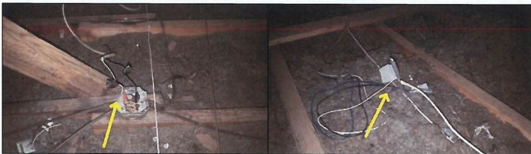
Exposed splice in center of attic
