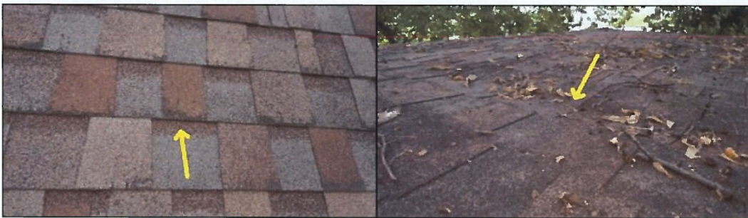
Granular loss and wear
