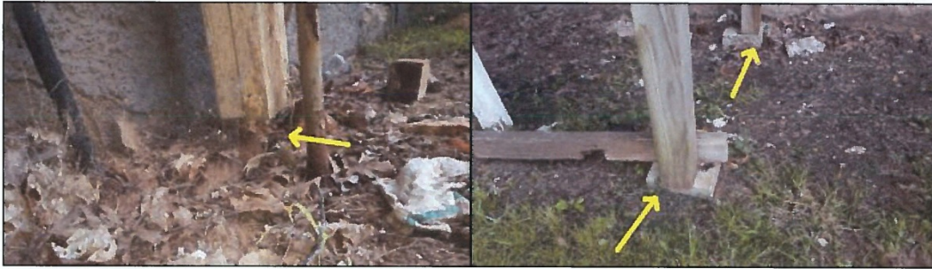
Missing footing below stairway - Unit 3
