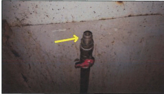
Open gas line behind stove
