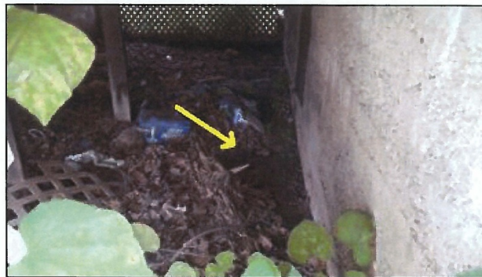
Poor drainage below front porch
