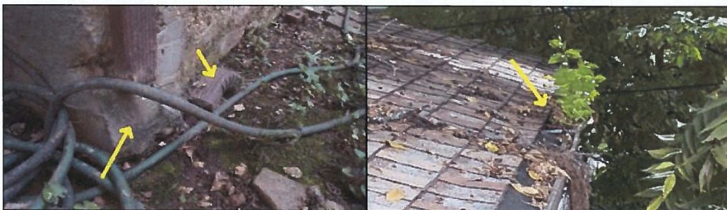
Missing downspout elbow
