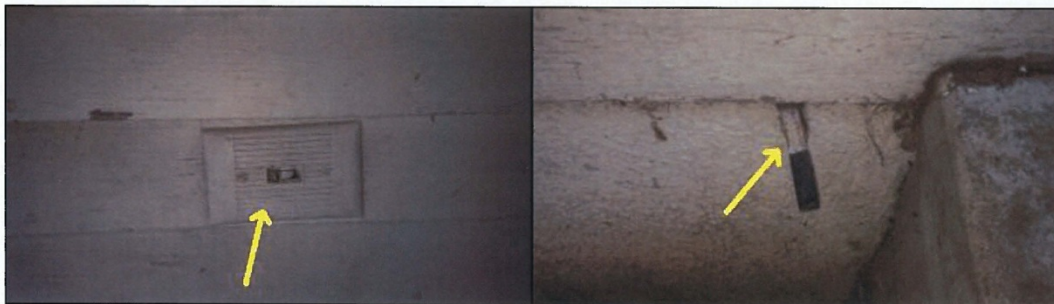
Broken switch at back porch
