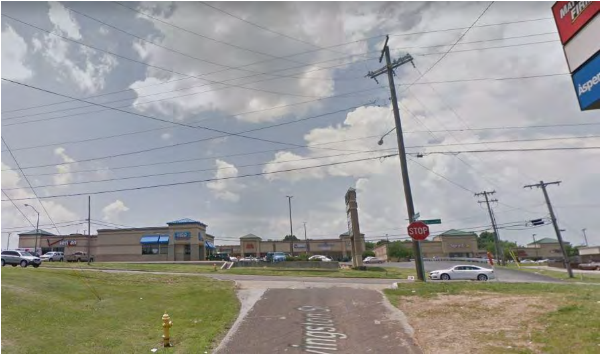
Powerlines at W. Livingston & N. Kansas Expwy
