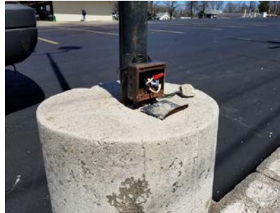
Figure 28 – Site lighting w/ open junction box & exposed wires, 1000 block E Kearney St, north side
