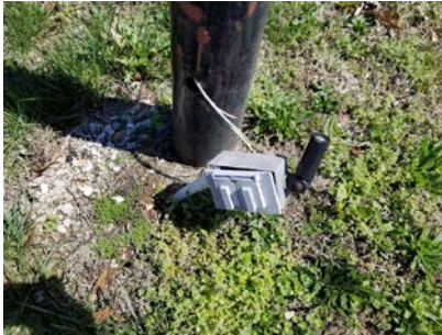
Figure 27 – Deteriorated signage w/ exposed wires, 800 block W Kearney St
