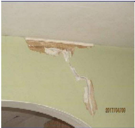
B-2.14) Structural cracks and structural issues are seen throughout the house.
