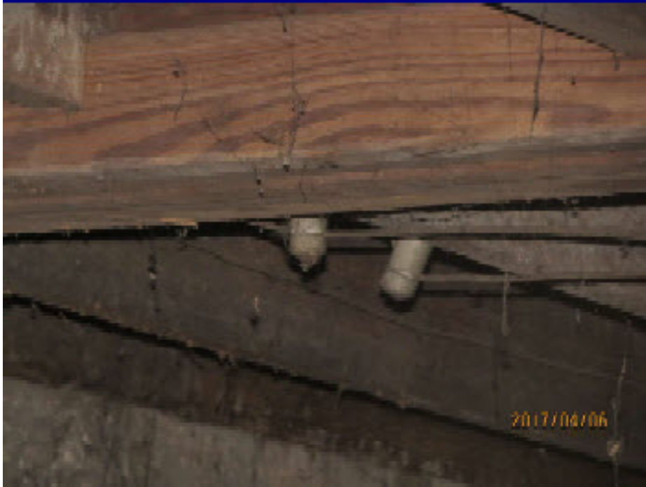
B-2.24) Electrical knob and tube is exposed below lath and plaster. The outdated wiring is at High Risk of causing a fire.
