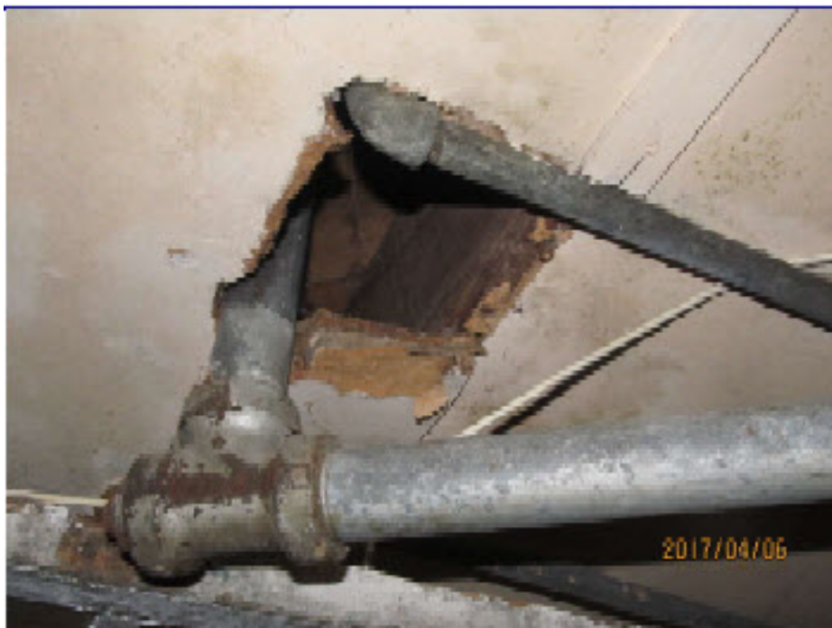
B-2.25) Exposed gas and water pipes throughout the house.
