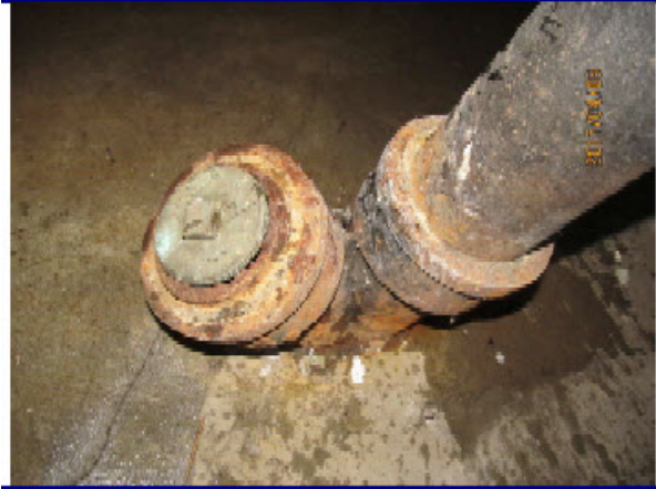
B-12) Sewer and Plumbing is obsolete and does not connect to city sanitation services due to a broken sewer line.
