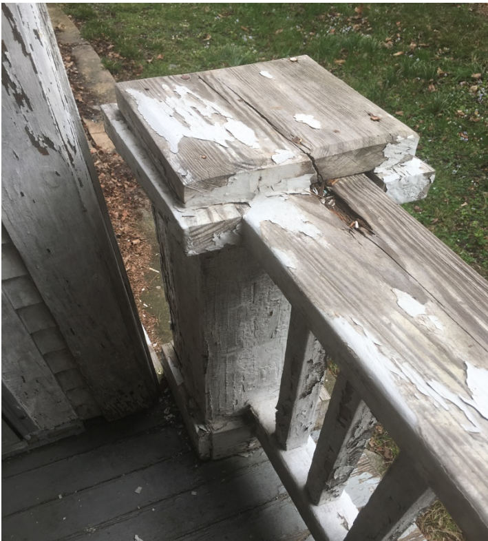
B-1.25) Structural Columns are decaying and has caused an sever structural porch danger.
