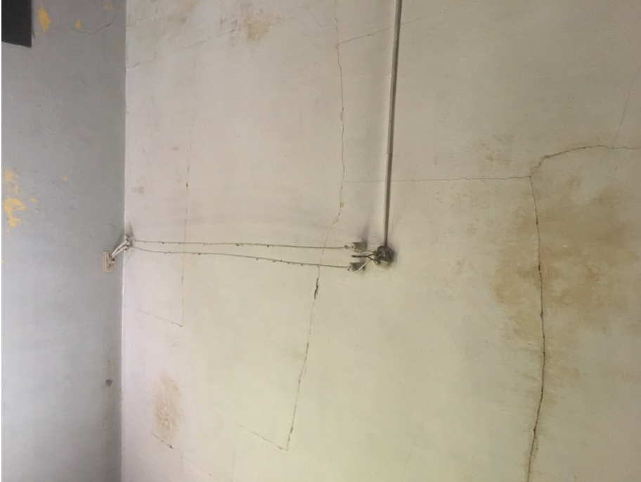
B-1.9) Electrical knob and tube is exposed below lath and plaster. The outdated wiring is at High Risk of causing a fire.
