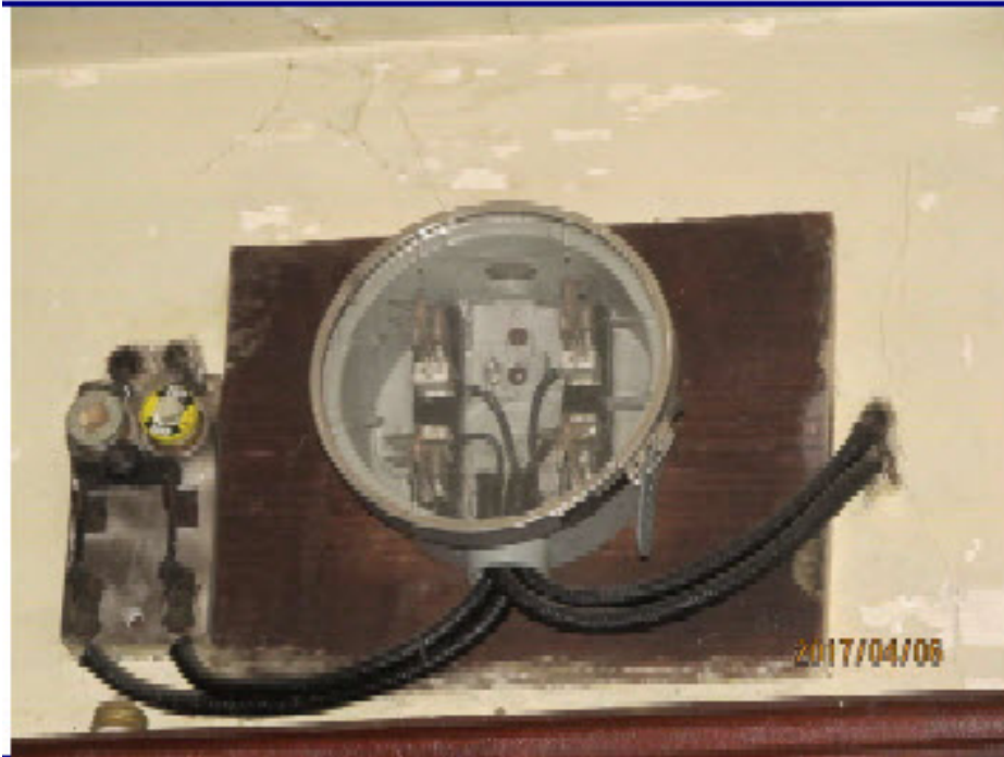
B-1.8) Electrical Fuse Box is outdated and is at High Risk of causing a fire.
