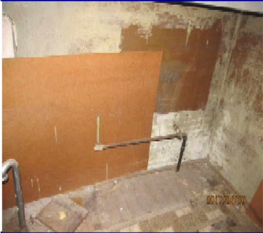
B-1.5) The Kitchen cabinets appear to have been removed and possible stolen from the house by vagrants.
