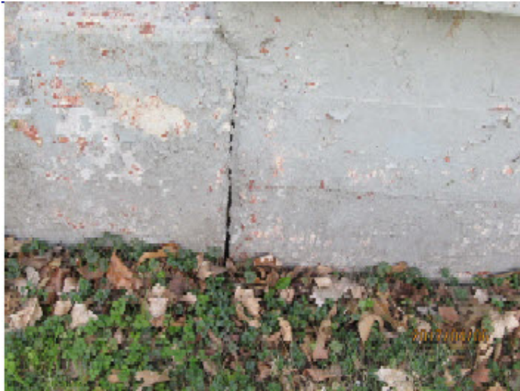
B-2.3) Cracks in the foundation are causing structural issues.
