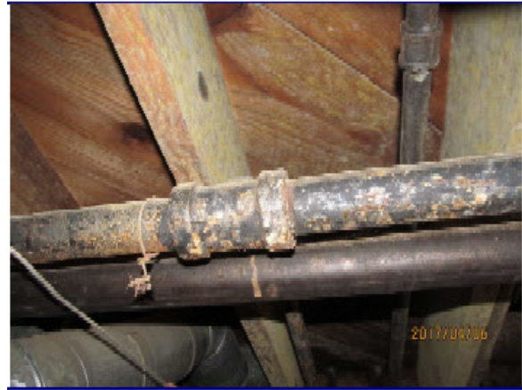
B-13) Metal Gas piping is corrosive and may be leaking gas into the house.
