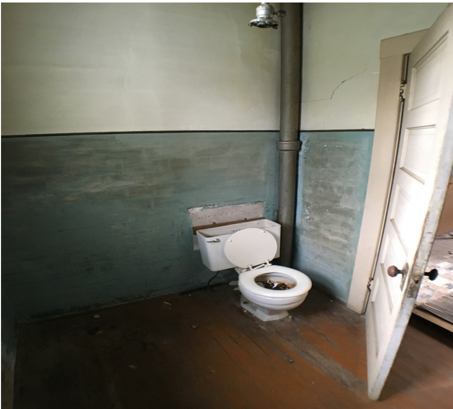
B-1.7) The bathroom has signs of vagrants utilizing the remaining toilet that is in non working order. The rest of the bathroom is in disarray.
