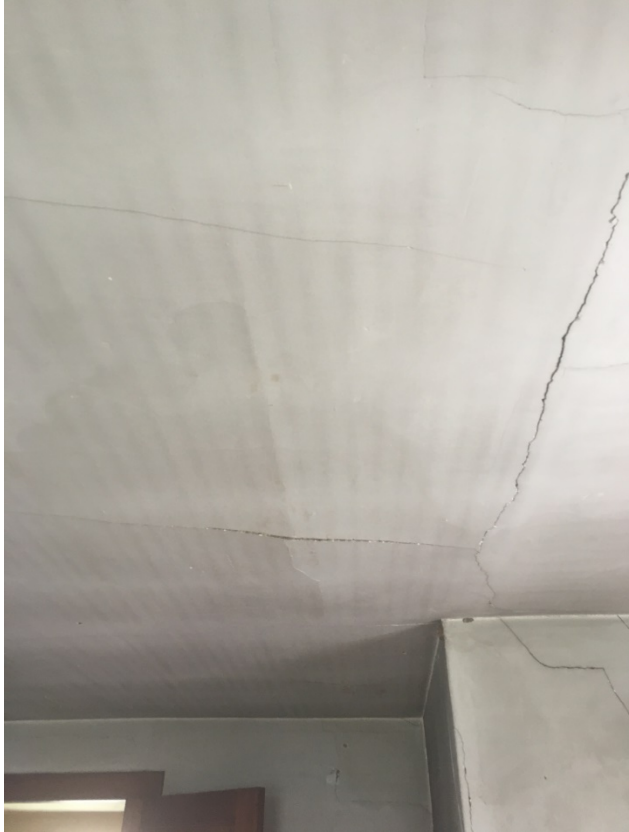
B-1.16) Structural cracks and structural issues are seen throughout the house.
