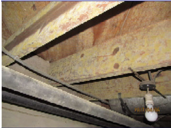
B-8) Fungi growth is prevalent on flooring joist in basement.
