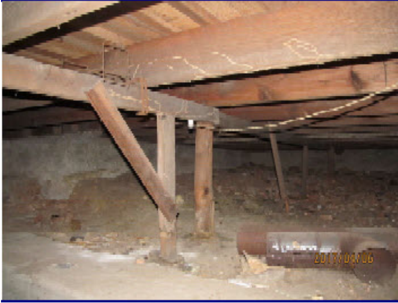
B-1.13) Girders and structural beams are undersized for weight of existing structure.
