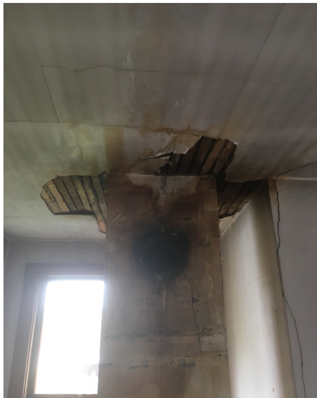
B-1.18) Dilapidated roofing has caused major interior damages around the fireplace.
