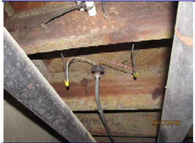
B-9) Electrical throughout the house is outdated, improperly installed, and is at High Risk of causing a fire.
