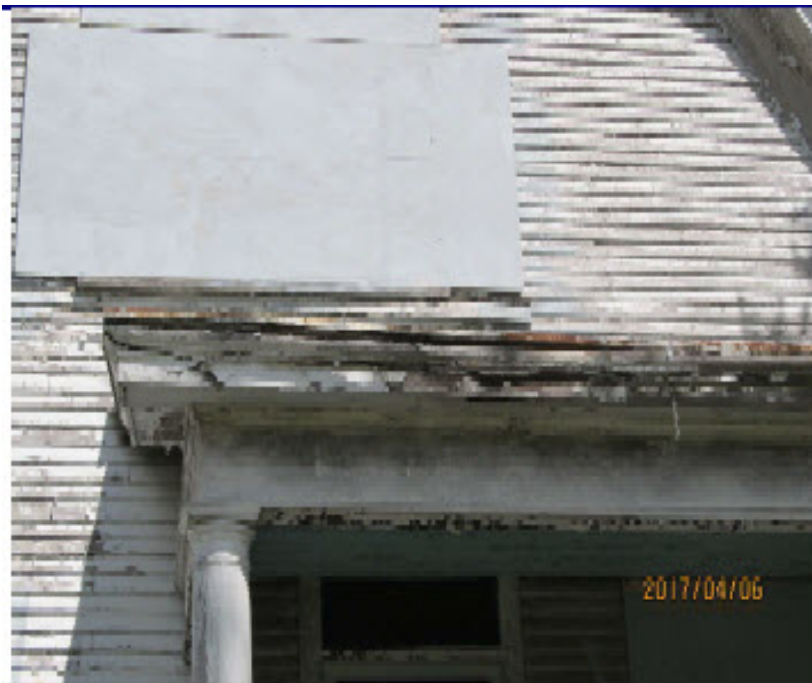
B-1.6) Guttering around the house is deteriorating and causing water damage to soffits areas and structural damages to porch.
