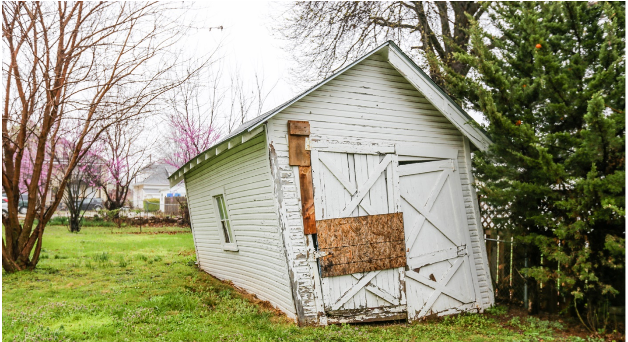
B-3.1) Exterior structure garage is falling over and unsecured. Vagrants have broken into the structure.
