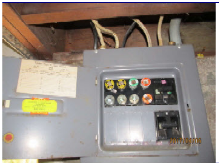
B-11) Electrical Fuse Box is outdated and is at High Risk of causing a fire.
