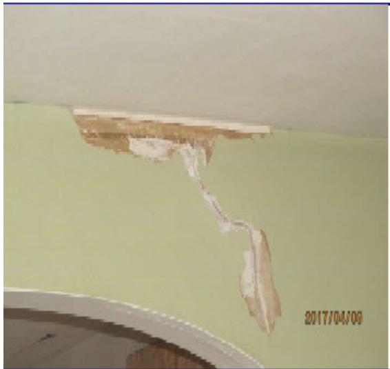
B-14) Structural cracks and structural issues are seen throughout the house.
