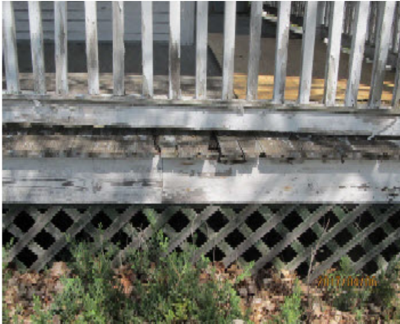
B-1.4) Porch flooring is rotted through and dangerous to the structure falling in.
