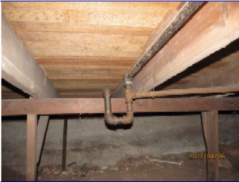
B-1.14) Metal Gas piping is corrosive and may be leaking gas into the house.
