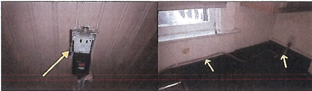
Missing plate in bathroom - Unit 3
