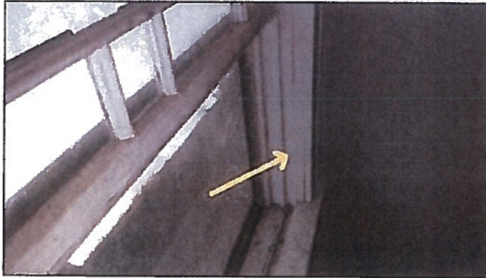
Lower dining room window is missing
