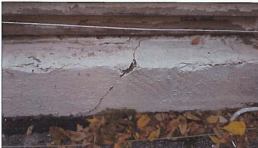
Typical foundation cracks - West side
