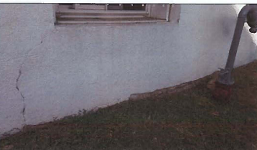
Cracks and deterioration - East Side
