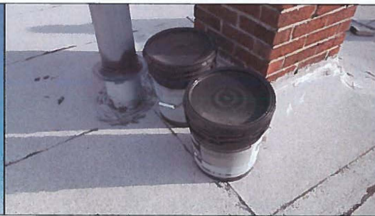
Buckets of sealant observed on roof indicating prior repair
