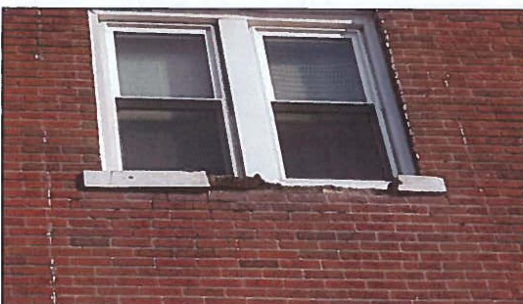
Deteriorated window ledges - Front, top floor
