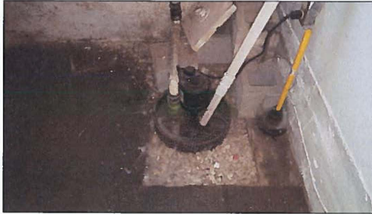
Sump pump installed
