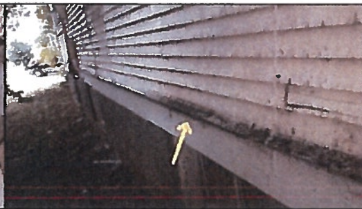
Deteriorated paint and trim below air conditioners.
