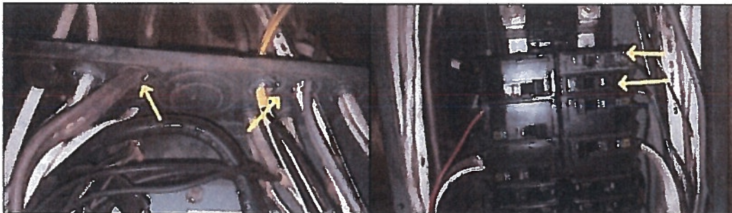
Missing protective clamps
