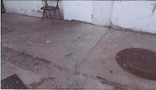
Poor drainage at rear of building
