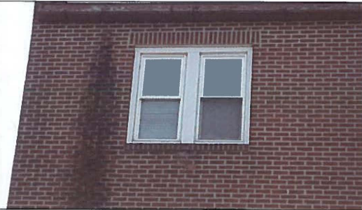
Signs of gutter leakage - Rear
