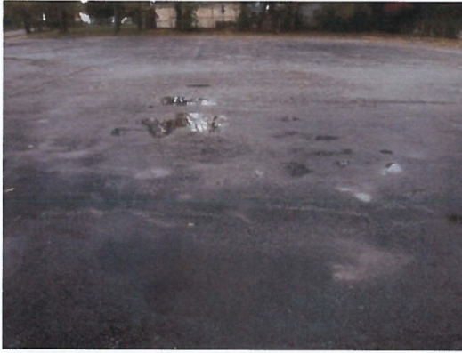
Parking lot has several low areas and ponding water
