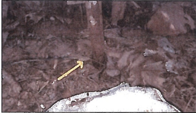
Heavily deteriorated main gas line
