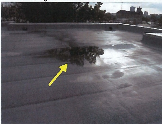
Ponding water at middle east part of roof
