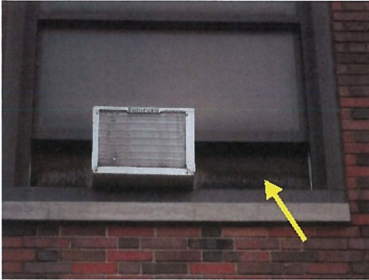
Mold growth on back of material at upper front east A/C unit
