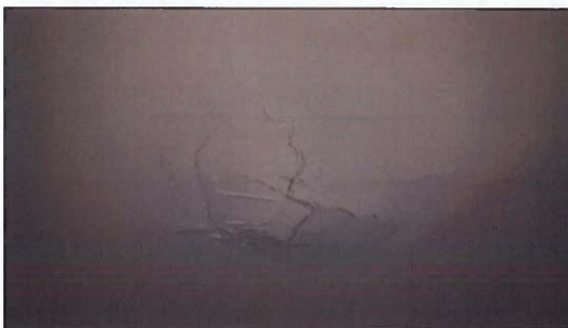
Damaged ceiling at back storage room
