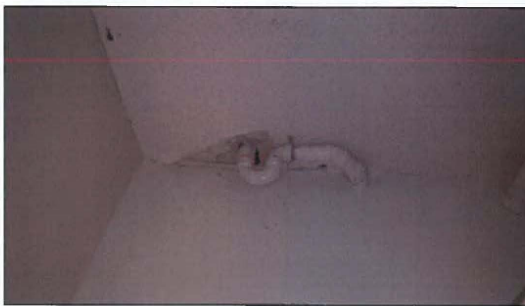
Moisture damage - Unit 13 Bath
