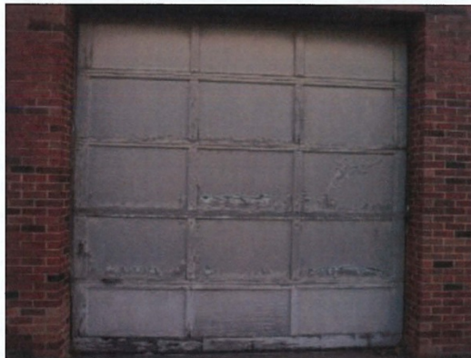
All vehicle doors have some flaking/peeling paint
