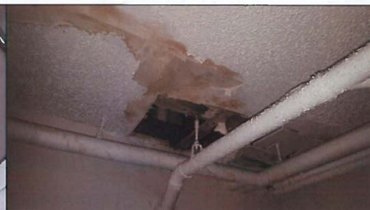
Moisture damage - Basement TV room
