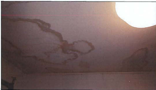
Moisture stains in laundry room
