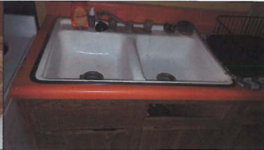
Missing drawer - Unit B kitchen
