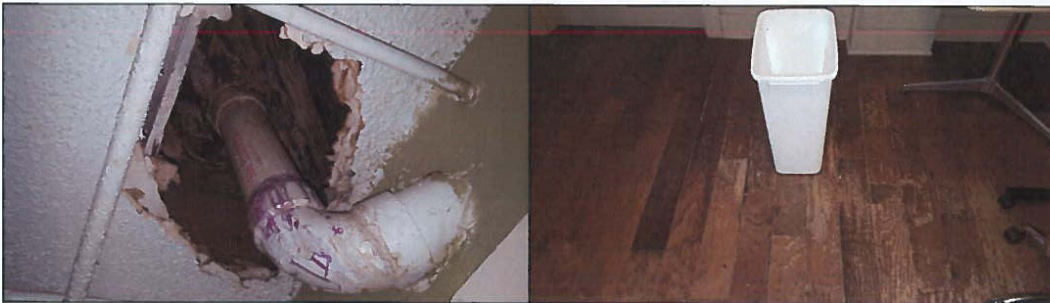
Mold fungal growth and moisture damage - Game room bath Bucket and moisture damage - Learning center
