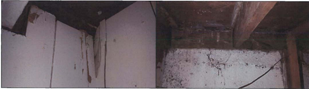
Termite shelter tubes near basement stairway
