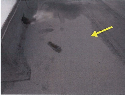
A pile of granules are present near the middle east roof drain
