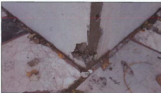
Damaged stem wall at back
