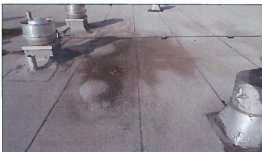
Signs of ponding on roof
