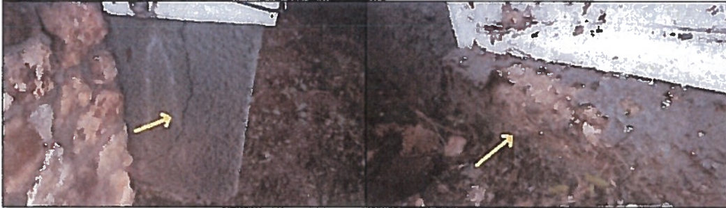
Crack at SE corner (1/2" displacement)
