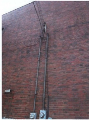
Electric service does not appear adequate for a building of this size
