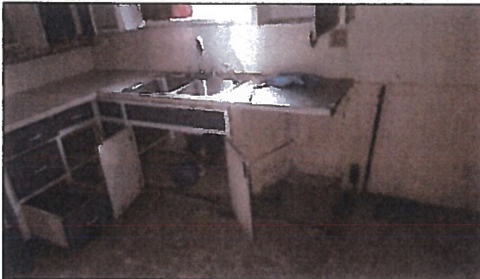
Kitchen is in poor condition overall.
