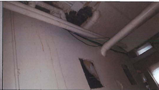
Holes/damage - Linen Storage
