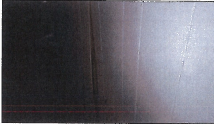
Loose paneling in living room. Unit 1
