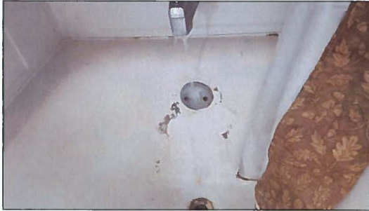
Tub faucet leaking - Unit B
