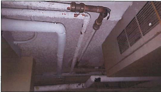
Past/Improper plumbing repairs - Main Laundry
