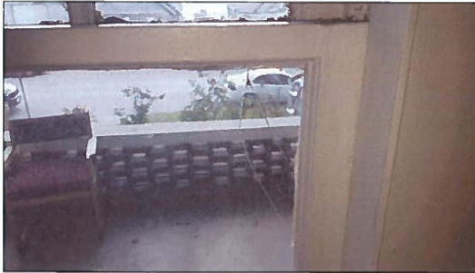
Broken window near front door
