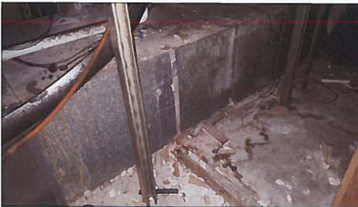
Moisture stains below AC coil Heat #1
