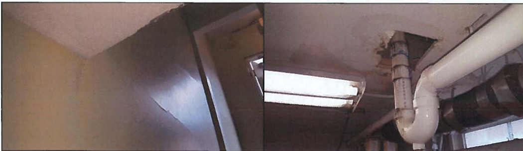
Loose plaster - North basement stairway
