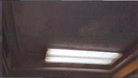
Moisture damage - Main kitchen ceiling
