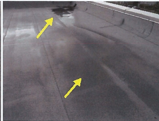
Standing water at west end near SW corner
