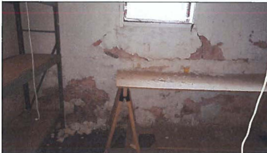
Moisture penetration/damage in SW room of basement
