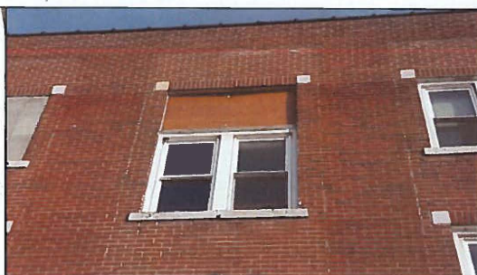
Boarded up window - Front, top floor
