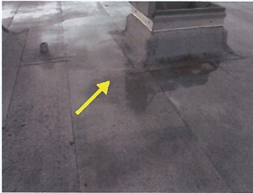
Ponding water around the roof access
