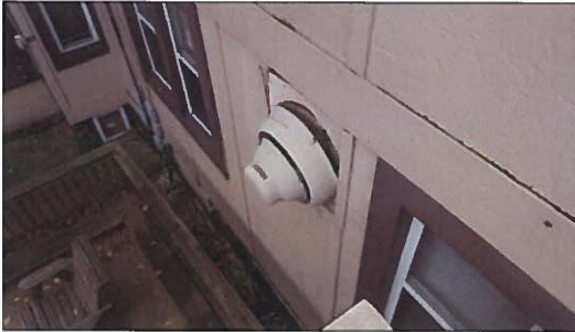
Loose exhaust fan on East side
