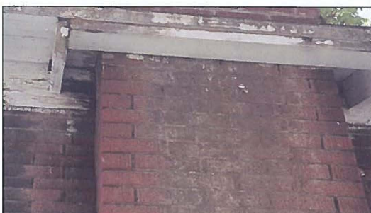
Damaged fascia at chimney
