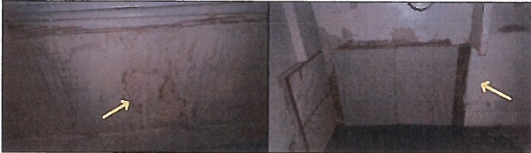
Moisture stains and cracks
