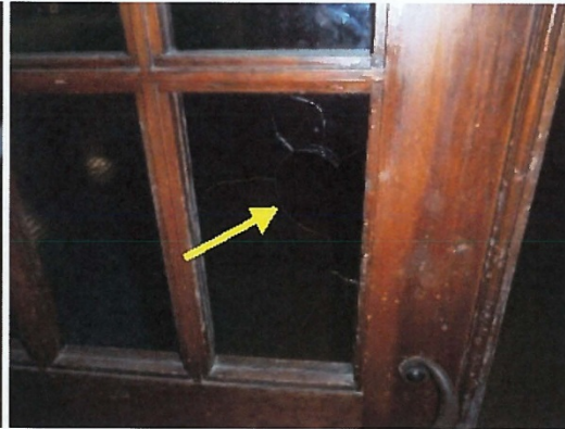
Broken glass panes on the doors to the gym
