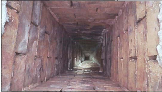
West chimney is unlined
