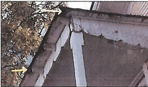
Deterioration above door to unit three
