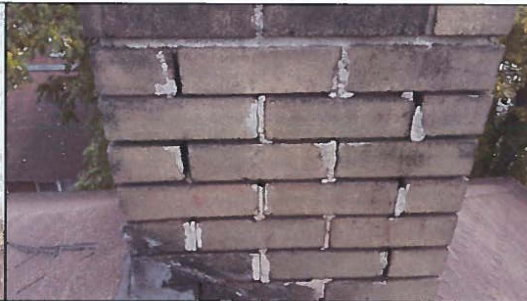
Spalling/missing mortar on chimneys
