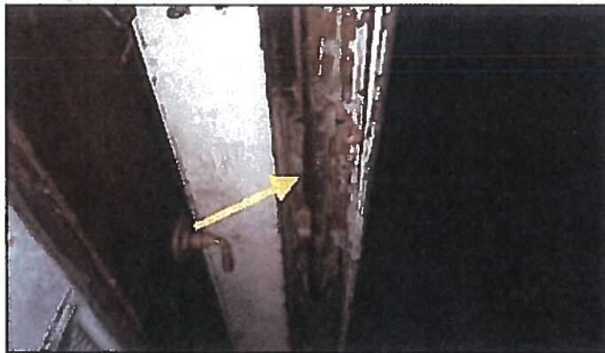
Unit 1 - Front door jamb is damaged
