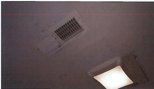
Mildew/fungal growth upstairs bathroom
