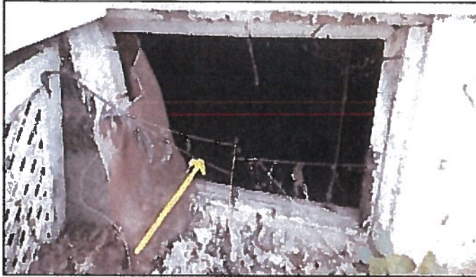
Missing basement window bear back porch.
