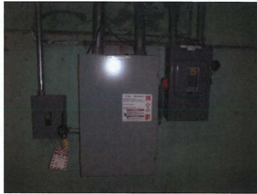
Main disconnects are located on the north wall in the NW basement room
