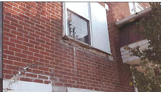
Deteriorated window ledge - Front
