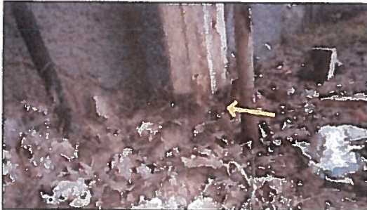
Missing footing below stairway - Unit 3
