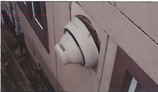
Loose/abandoned fan on East side
