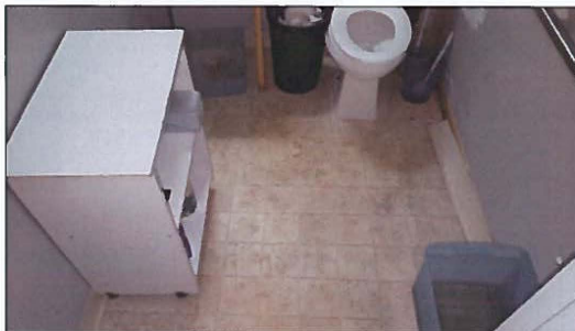
Tubs below plumbing leaks - Staff Bathroom
