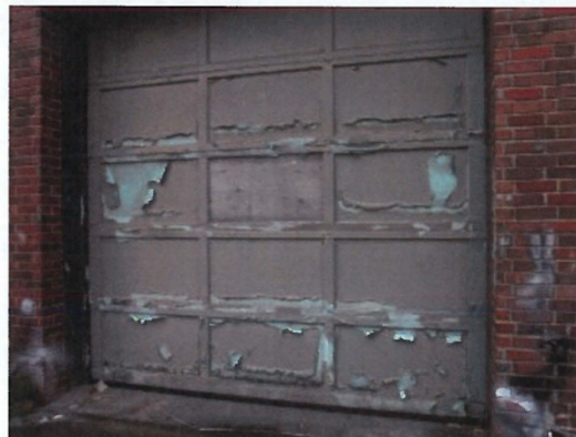
Heavy flaking/peeling paint on the roll up door on back of the gym
