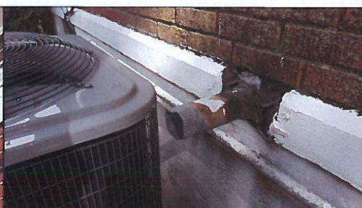
Vent pipe directed at AC unit
