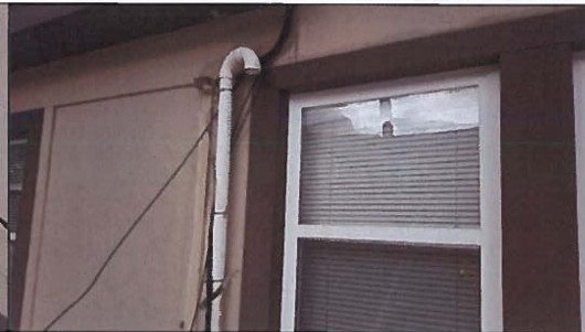
Vent too close to widow on East side
