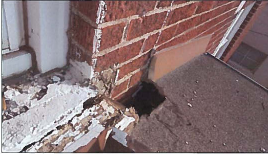
Holes in entry roof - Both sides of windows
