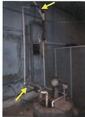
The sump pump dispels improperly into the sanitary sewer system
