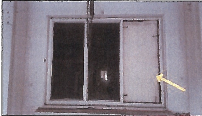
Missing glass at front door
