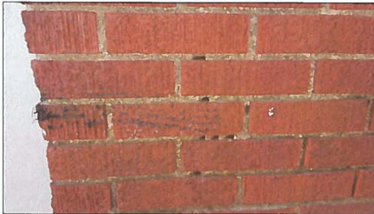
Spalling mortar at chimney
