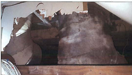
Likely asbestos containing tape on abandoned ductwork in basement.
