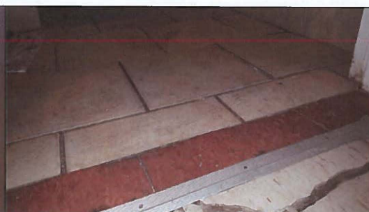
Damaged floor - Bath C
