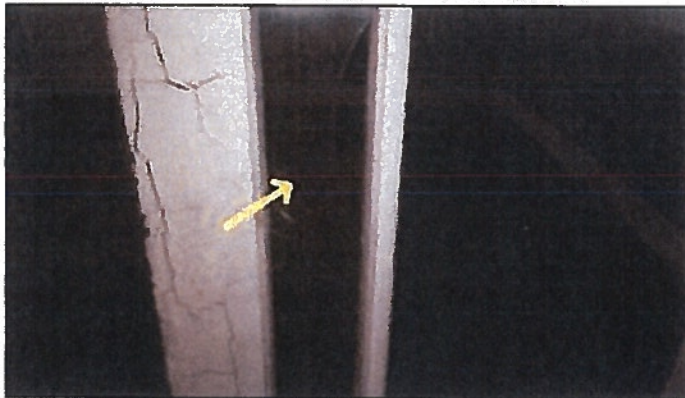
Broken glass in main living area doors.
