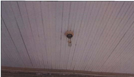
Missing globe at front porch
