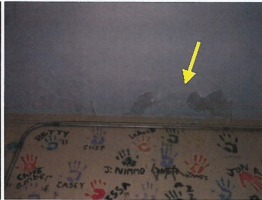
Water damage to ceiling at upper north hallway
