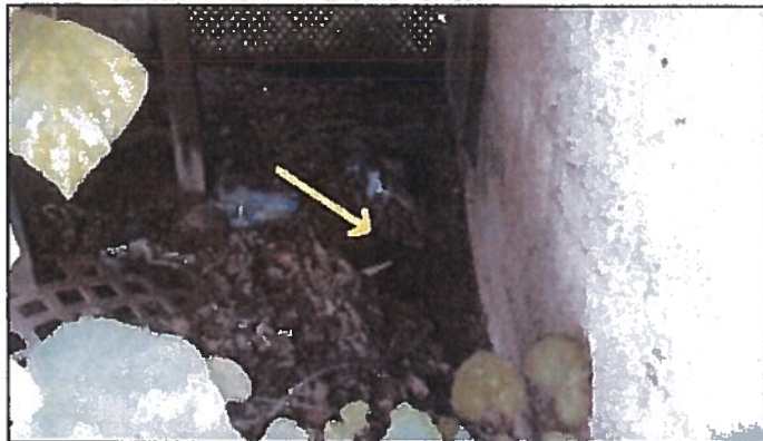
Poor drainage below front porch
