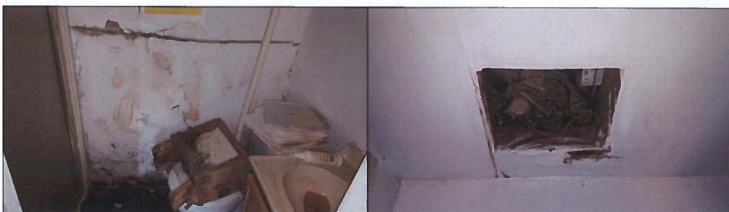
Heavy moisture damage in basement bath
