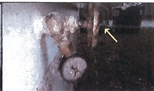
Rear faucet leaks
