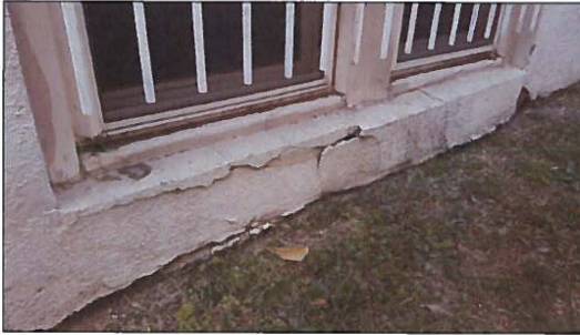
Deteriorated sparging - East side
