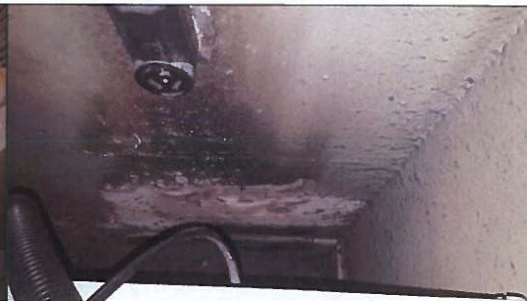
Evidence of past lint fire - NW corner of main laundry
