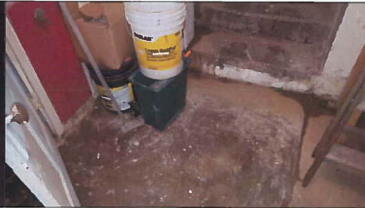
Signs of moisture penetration near basement stairway
