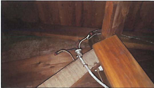
Exposed/improper splice above attic access
