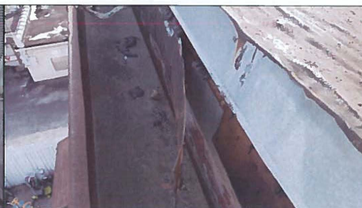
Loose flashing at rear gutter
