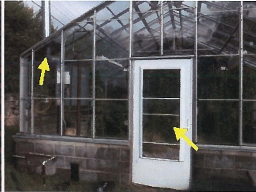
Broken glass in door and upper SW corner
