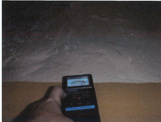
Abnormal moisture at south wall in the east entry
