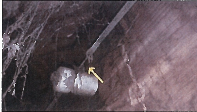
Knob and tube wiring with deteriorated insulator in SE portion of basement.
