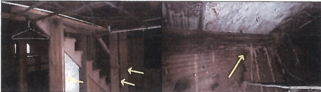
Floor and interior basement stairway poorly supported
