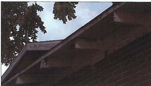
Damaged eaves on West side
