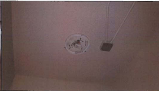
Missing light - Unit 13 Closet
