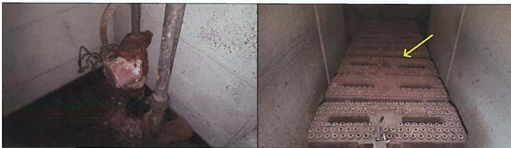
Heavy corrosion on water recirculation pump in boiler room
