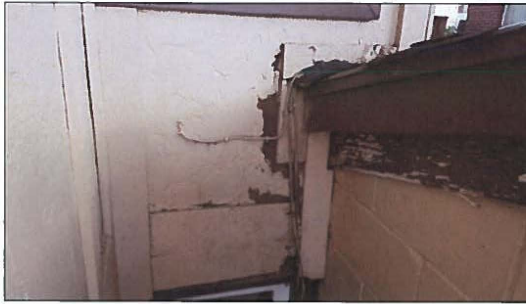
Moisture damage at basement stairway connection
