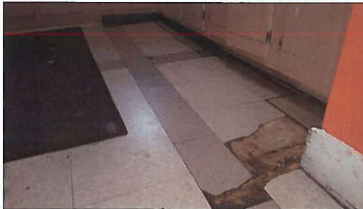
Flooring damage - Dining area
