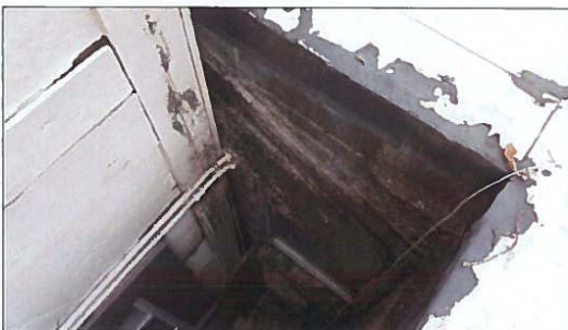
Moisture damage between sections on East side
