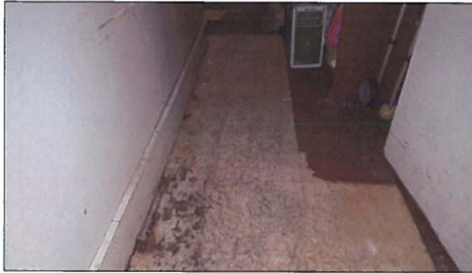
Flooring damaged/missing - Linen Storage
