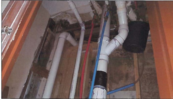
Mold and Improper plumbing repairs - Oasis room closet
