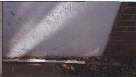
Typical cracks in foundation stem walls
