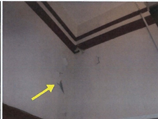
Peeling paint at SE corner of office area
