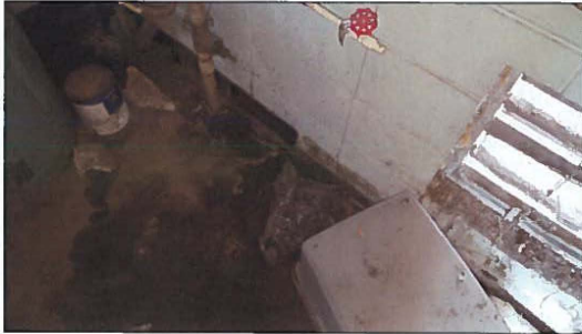
Leak in boiler room
