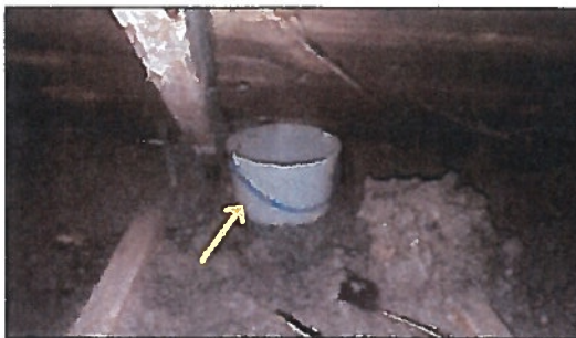
Bucket indicating past leak
