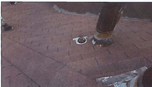
Improper height on plumbing vent
