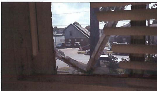
Broken window at front office
