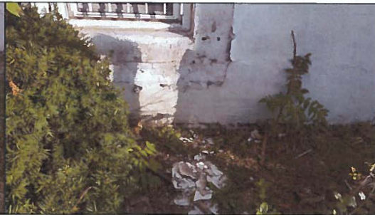
Spalling surfaces - Front
