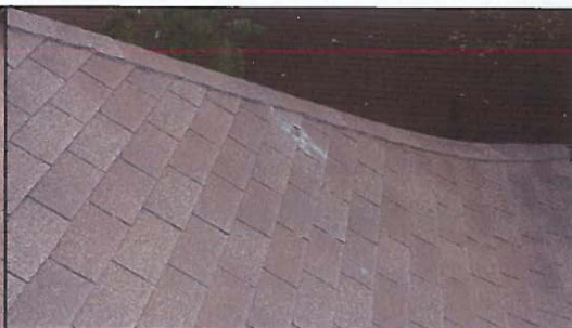
Damaged shingles near SE corner
