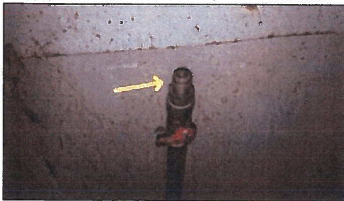
Open gas line behind stove
