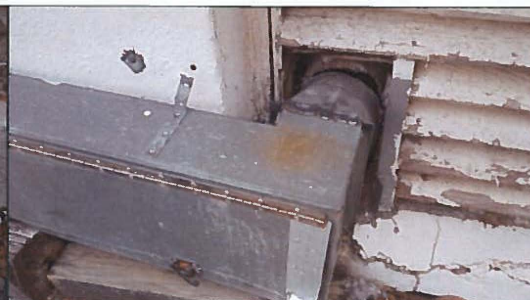
Disconnected dryer duct - West side
