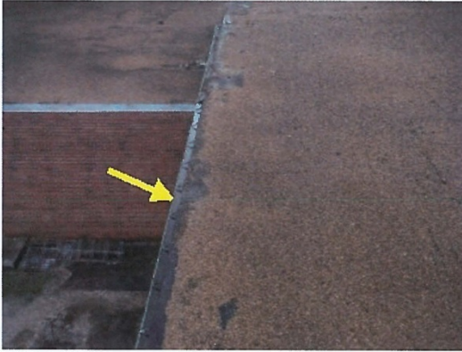
Guttering on back of gym is full of rock and water at time of inspection
