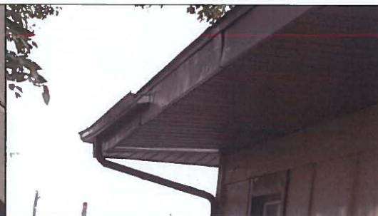
Majority of gutters have been removed
