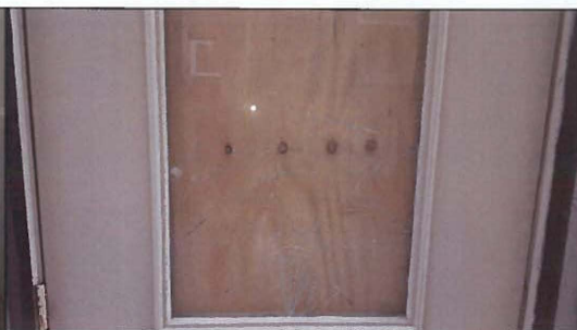
Broken window on west side
