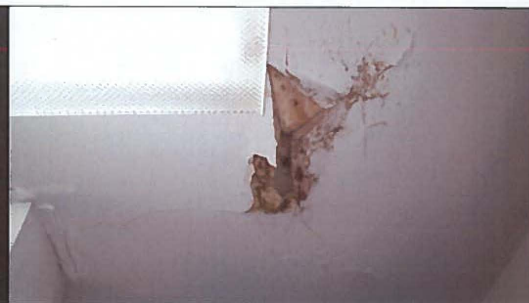
Moisture damaged ceilings
