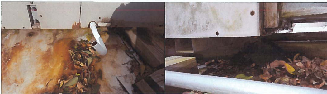
Condensation drains onto roof AC 3
