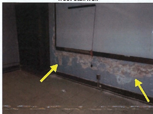
Delaminating plaster at SE corner of upper SE classroom
