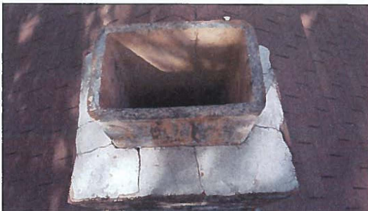
Cracks in crown and flue tile at West chimney
