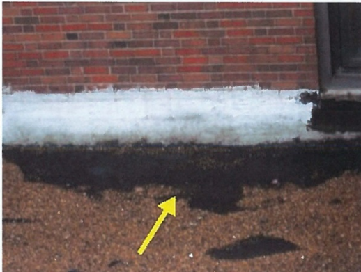
Missing gravel at SW corner of the gym roof
