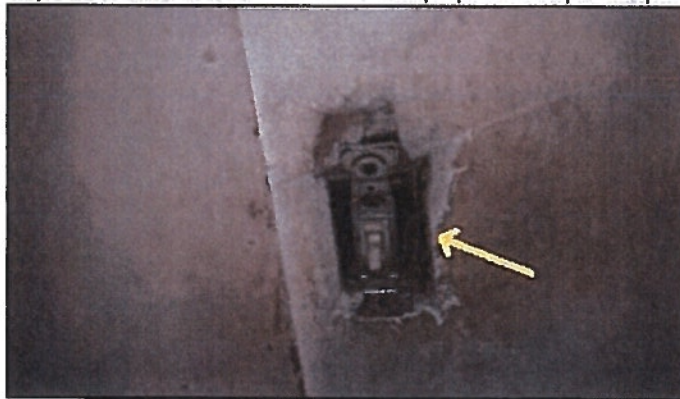
Outlets and switches missing plates in various locations.
