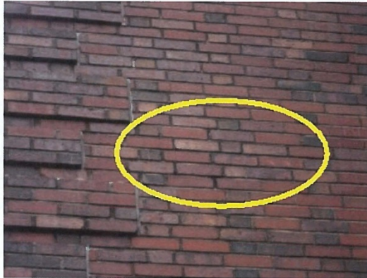
Area of tuck pointing needed at upper front west entry
