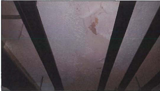
Moisture damage ceiling - 3rd Hall
