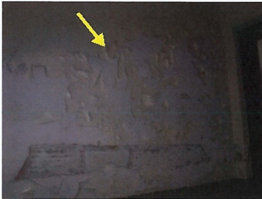
Heavy peeling finish at middle part of east stairway
