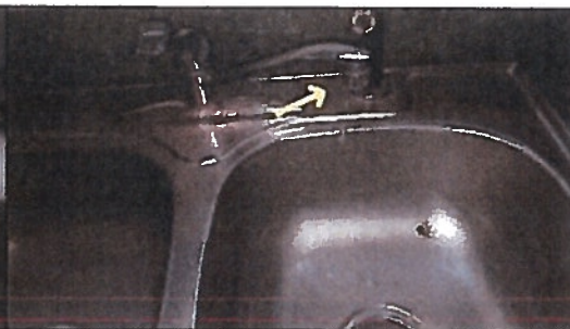
Leaky and loose faucet - Unit 2
