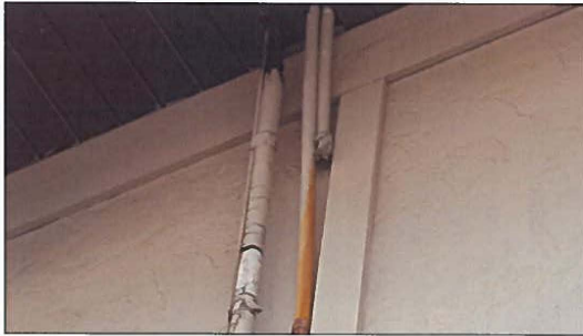
Condensation leaking from overflow on West side
