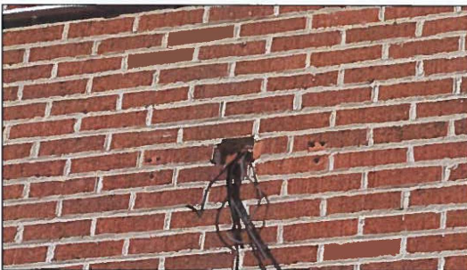
Hole in brick - East Side
