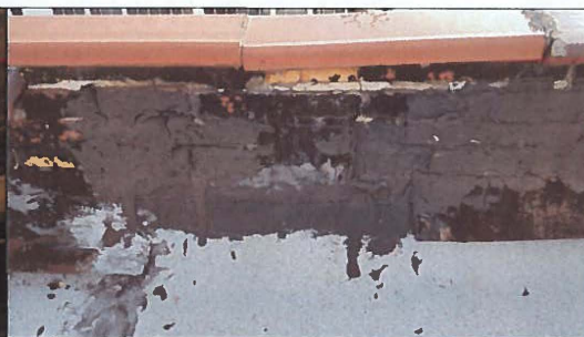
Deterioration and sealant on parapet wall
