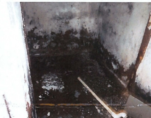
Water was leaking into the small cubby at the north wall in the basement
