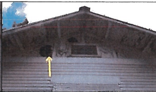
Holes in asphalt paper on West gable
