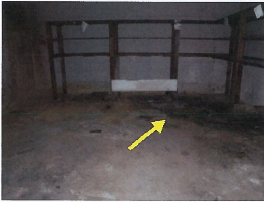
Stains from past water penetration at the NE basement room
