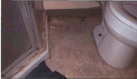
Standing water and damaged floor - Bath G
