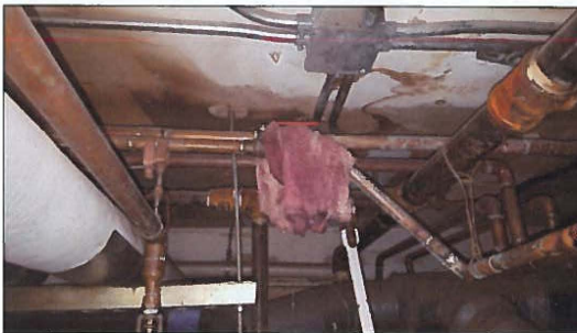
Multiple Plumbing leaks - boiler room
