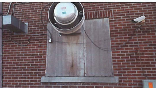
Boarded up window - Rear
