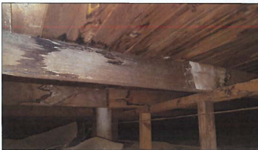
Moisture stains throughout attic
