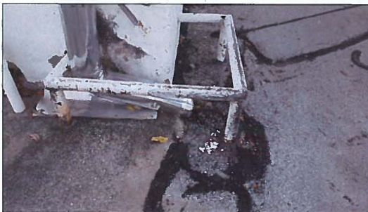
Gutter drains onto Driveway, will cause deterioration and ice buildup.
