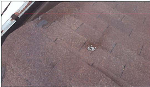
Damage at North end of ridge
