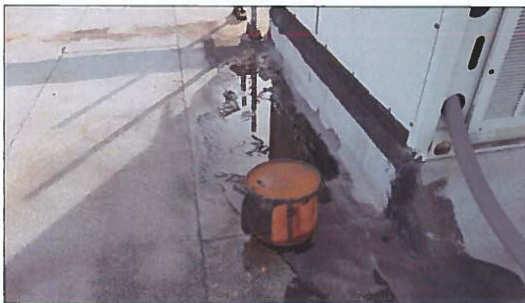
Ponding near water cooler on roof
