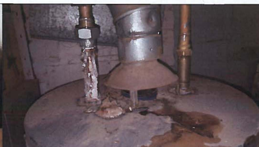
Corrosion at front water heater
