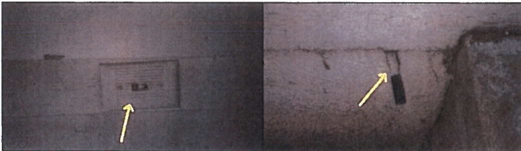
Broken switch at back porch
