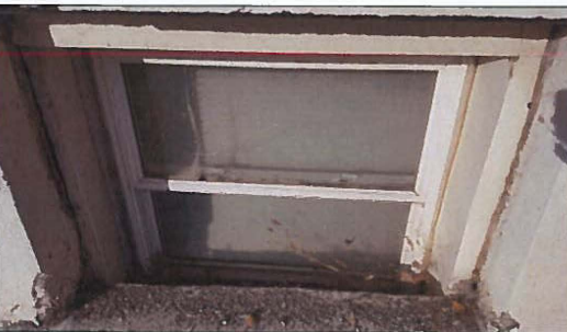
Broken window - East, Basement
