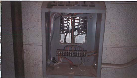
Missing cover and loose wiring at boiler subpanel
