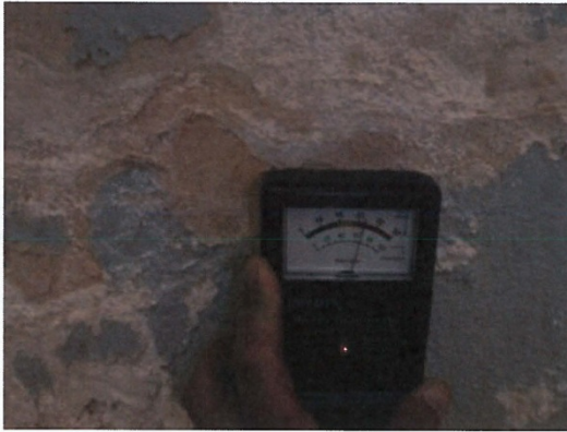
Abnormal moisture at water damaged wall in the upper SE classroom
