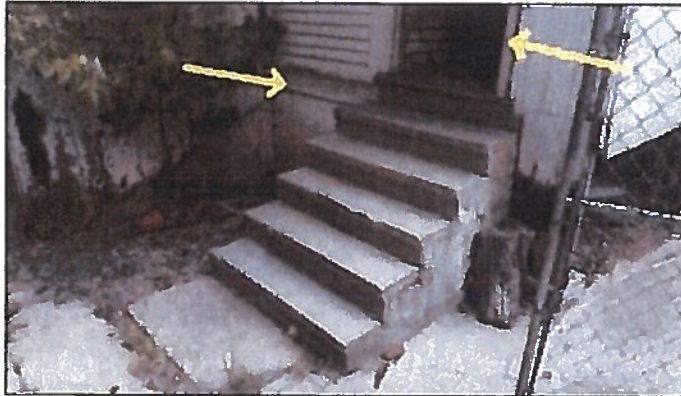
Handrail needed at back steps
