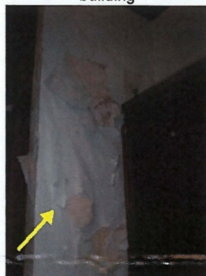
Water damage at SW corner of the upper middle classroom
