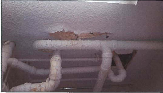
Moisture damage - Main kitchen ceiling
