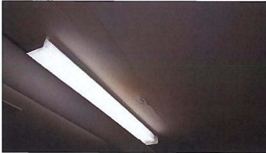
Moisture stains ceiling and floor 209
