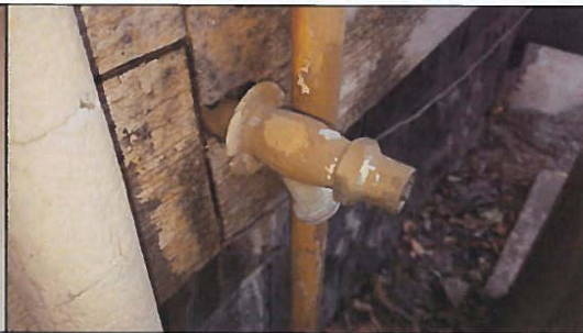
Faucets missing handles, not tested
