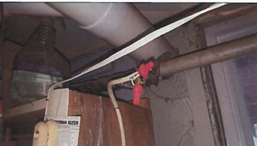
Exposed splices throughout basement
