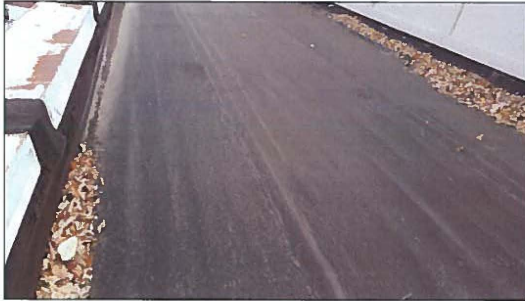
Middle section of roof dear end of lifespan
