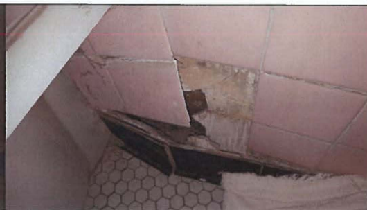
Moisture damage around shower
