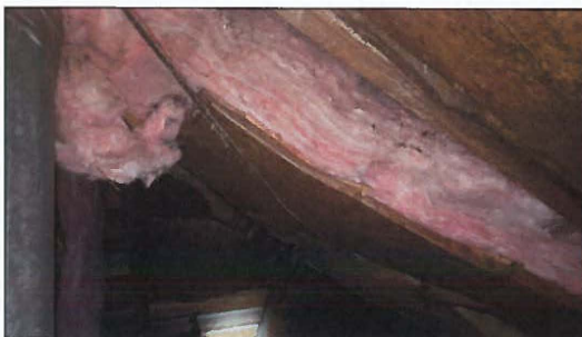
Knob and tube wiring touches insulation in attic
