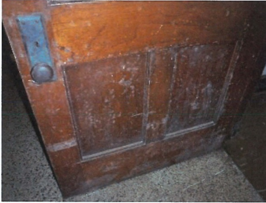
Mold growth on several doors
