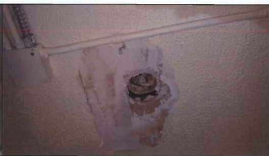
Missing light - Bath E
