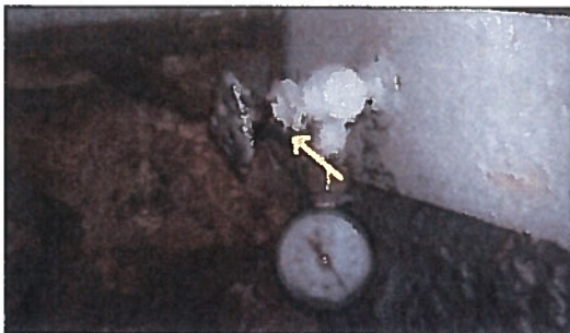
Front faucet leaks under pressure
