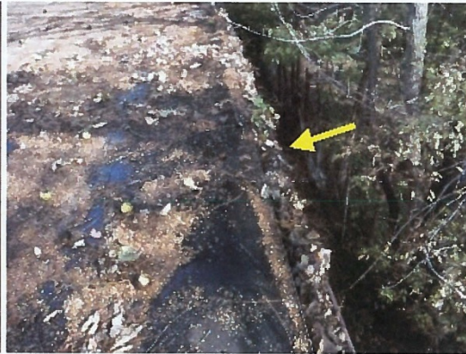
Guttering on back of addition is full of leaves/debris
