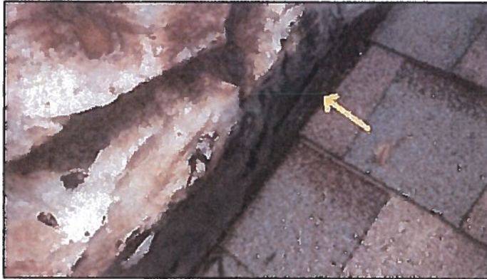
Improper and loose flashing at front chimney
