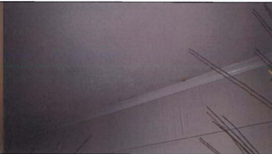
Moisture stains in main living area
