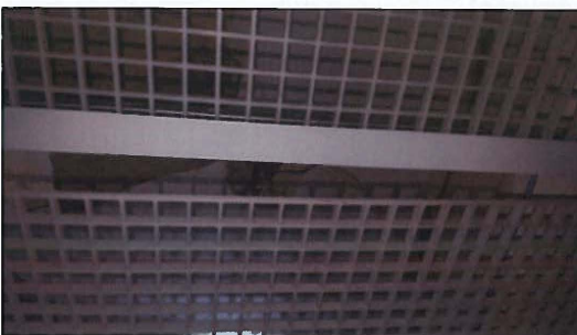
Exposed splice above grid in main hall
