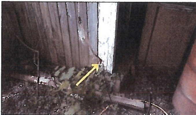
Cord with exposed splice powers garage
