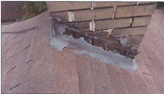
Improper flashing at east chimney
