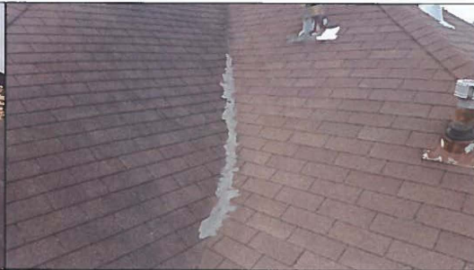
Past repair in rear valley
