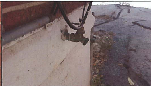
Leaky faucet at NE corner
