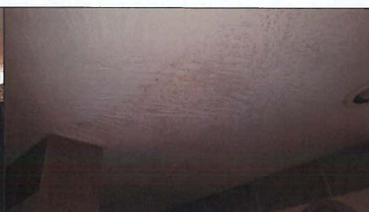
Mold/Mildew - Oasis bathroom ceiling
