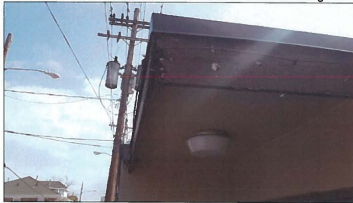
Damaged fascia at back of addition
