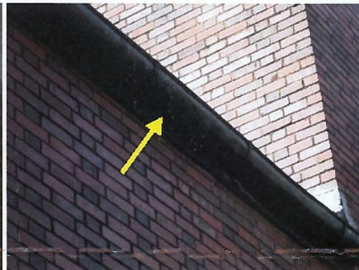
Water was running over at the guttering on back of the gym
