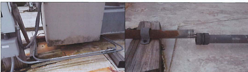
Condensation leaking from bottom of unit AC 3
