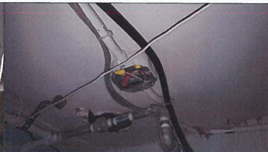
Missing junction box covers in basement
