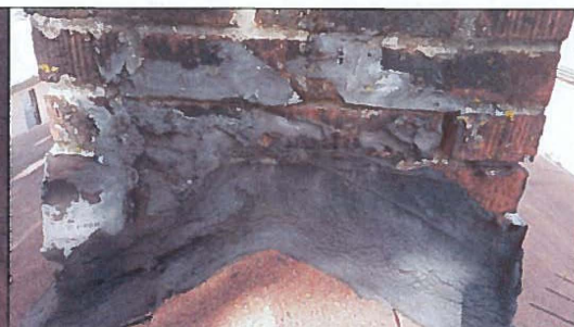
Improper/loose flashing and missing mortar at West chimney
