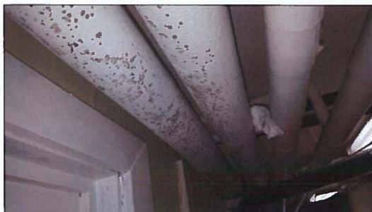
Mold/Mildew - 2nd floor hall pipe insulation
