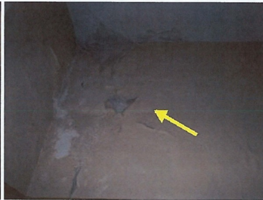
Moisture damaged plaster at the SE corner of the east entry
