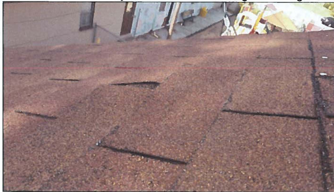
Raised shingles at North end of ridge
