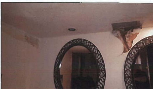
Heavy moisture damage & current leak - Oasis Room Bathroom
