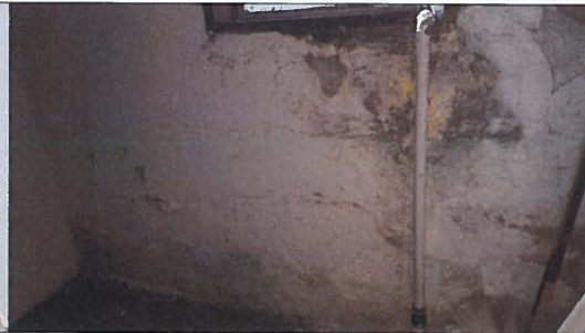
Moisture penetration/damage in main room of basement
