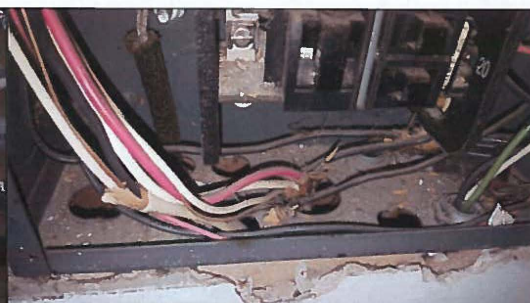
Missing protective clamps in panel
