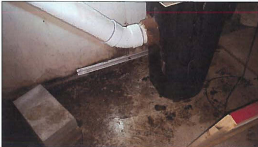
Leak at sewage lift pump
