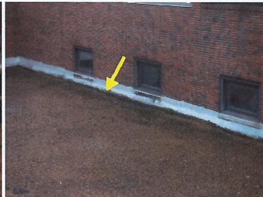
Prior patching/repair all along the roof wall connection
