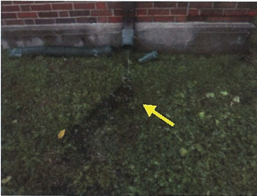
Poor drainage at SW corner of building
