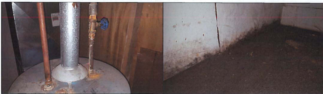
Corrosion at water heater supply
