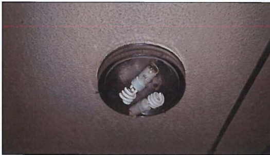
Missing globe - Unit B Kitchen (Typical throughout)
