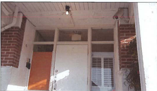
Boarded up window - Entry
