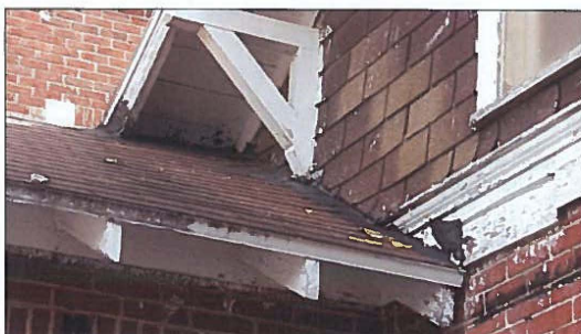
Improper flashing and heavy sealant at back of roof
