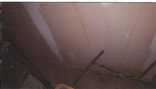
Mildew and moisture stains - Furnace room
