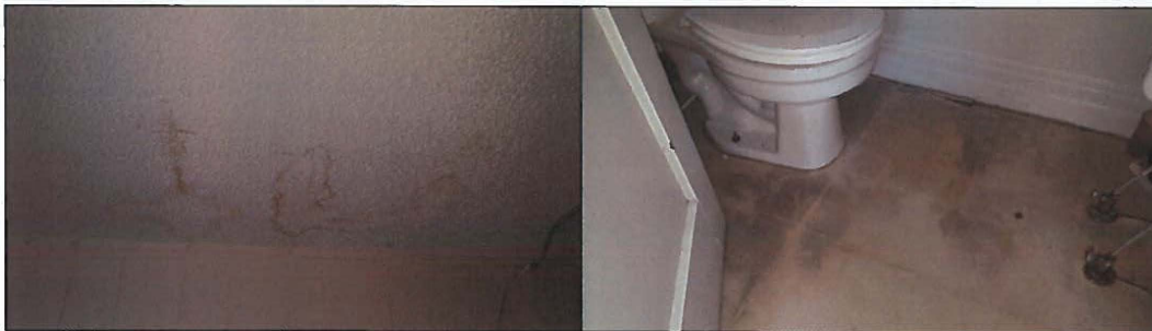
Moisture Damage/Stains ceiling - Unit H
