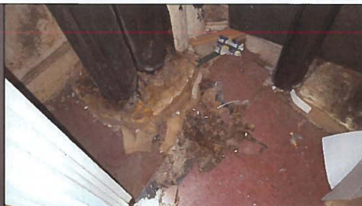
Floor damage - Unit 26 Closet
