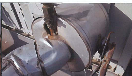
Corrosion on valves and fittings on roof water cooler
