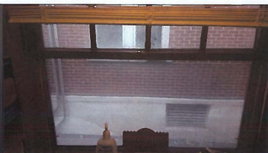
Broken Windows - Kitchen
