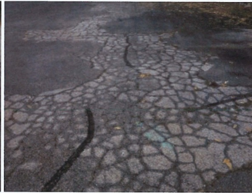
Asphalt parking lot is in poor condition; surface is alligating
