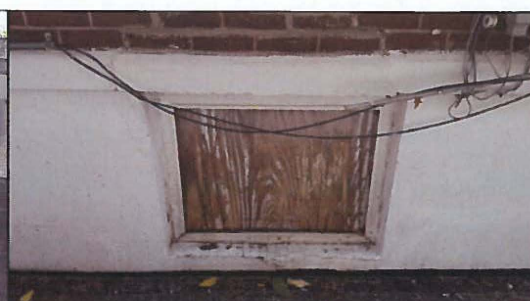
Basement windows have been replaced with plywood
