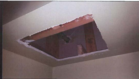
Missing access panel in NE hall
