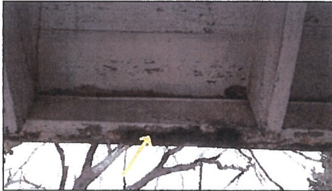
Gutters rusted through
