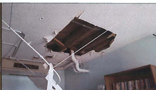
Moisture Damage - Library Ceiling
