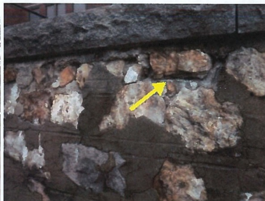
Areas of deterioration in a few areas of retaining wall
