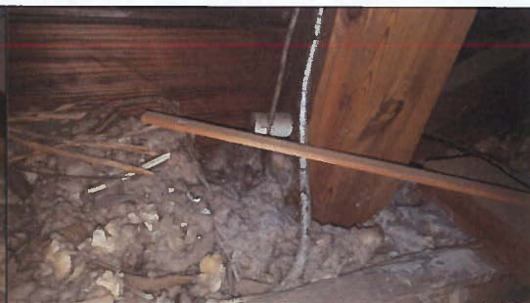
Knob and tube wiring in attic
