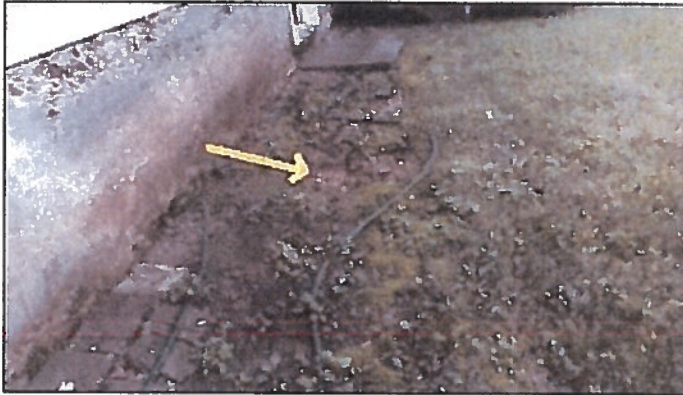
Erosion from overflowing gutter at back of home
