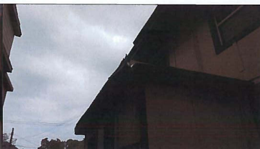
Damaged gutter on West side
