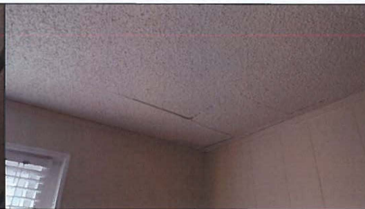
Loose plaster on ceiling - Unit F
