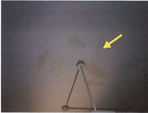
Old stains on ceiling in the upper SW classroom
