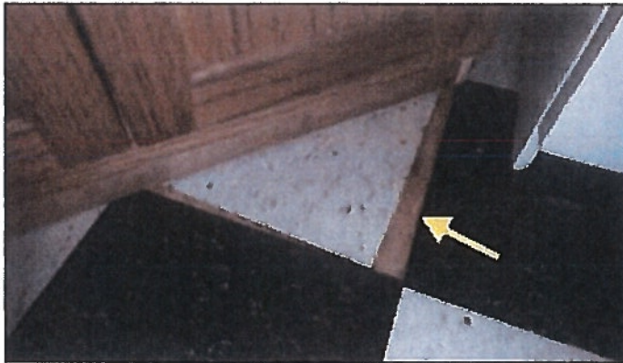
Loose tile below sink - Unit 1
