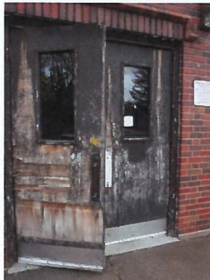
West exterior doors are damaged and delaminated
