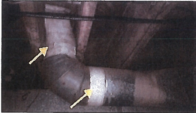
Tape on ductwork likely contains asbestos
