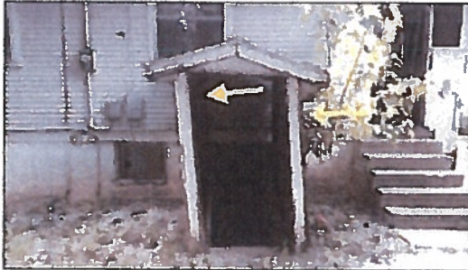
Stairway covering damaged and leaning
