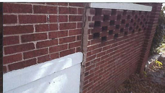
Settlement at front porch
