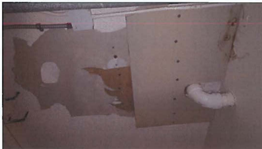
Moisture damage - Bath 23/25
