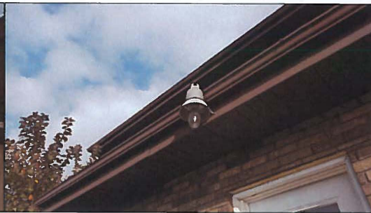
Missing globe at front door
