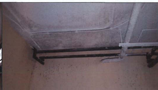
Mold/Mildew ceiling and walls - Bath G
