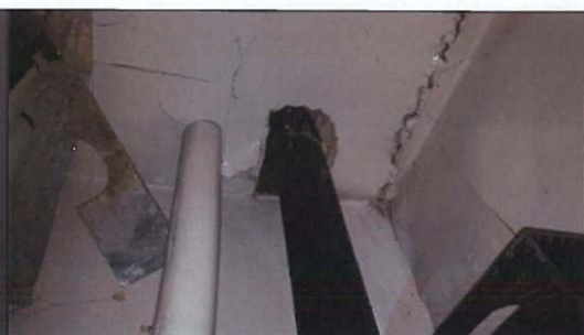
Moisture damage - Unit 8 Closet
