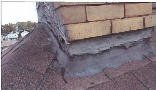
Loose/improper flashing at West chimney
