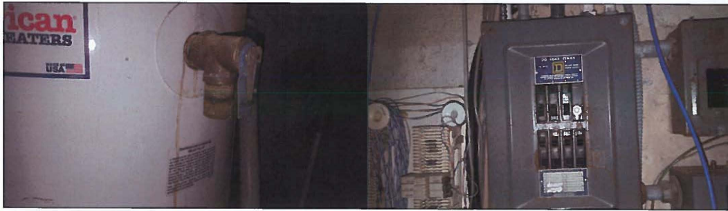
Missing TPR pipe at front water heater
