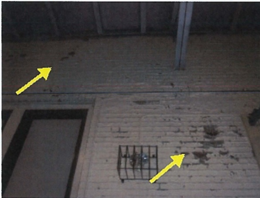
Peeling paint on the north gym wall
