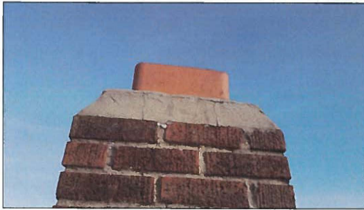
Cracks in crown and missing rain cap
