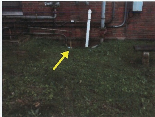
Low spot at the rear west end of the building
