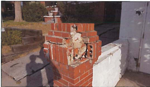
Damaged column on retaining wall - Front
