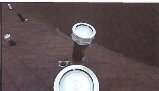
Leaning flue pipe
