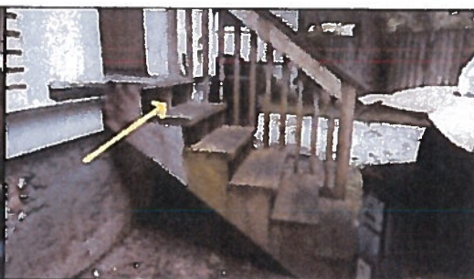
Handrail missing at back steps
