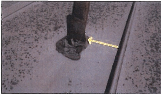
Kitchen plumbing vent
