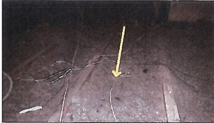
Attic poorly insulated
