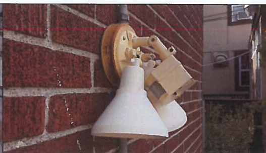
Damaged light at back porch
