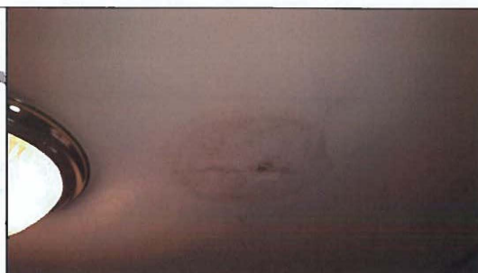
Moisture damage in office 202
