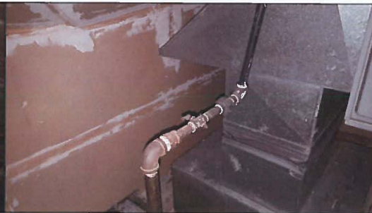
Leak detected on gas line near attic furnace
