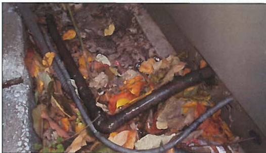
Missing/damaged insulation on South AC lines
