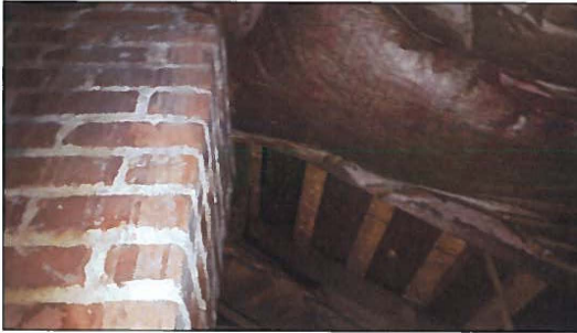
Moisture detected below chimney at front of building
