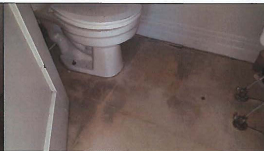
Moisture damaged floor - Unit H
