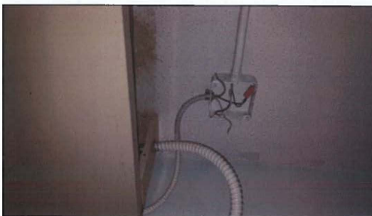
Exposed wires - Unit A
