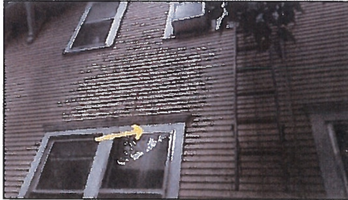
Condensation dripping down walls and window
