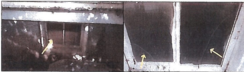
Boarded up basement windows
