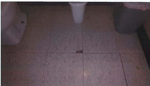
Damaged flooring in nursery bath
