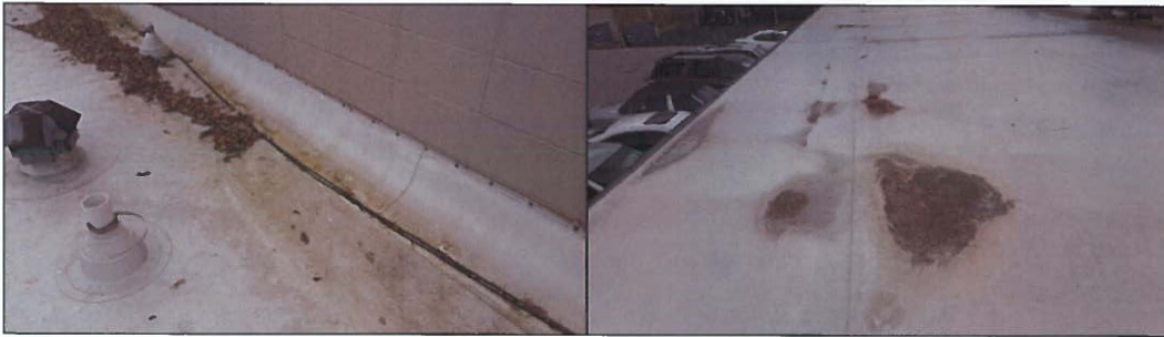
Signs of ponding/poor drainage at rear addition roof
