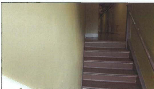
Bowed/loose plaster - South stairway wall 2nd/3rd
