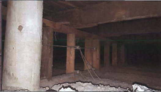
Knob and Tube wiring observed in attic
