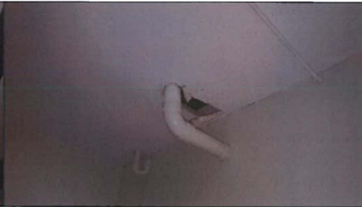
Ceiling damage - Bathroom 12
