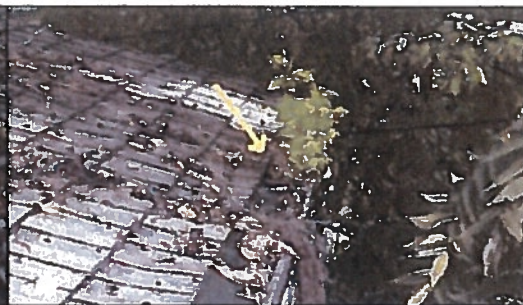
Missing gutter guard at SE corner
