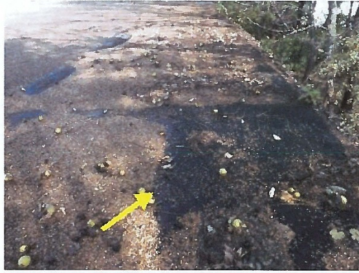
Missing granulars at middle east part of the storage building roof
