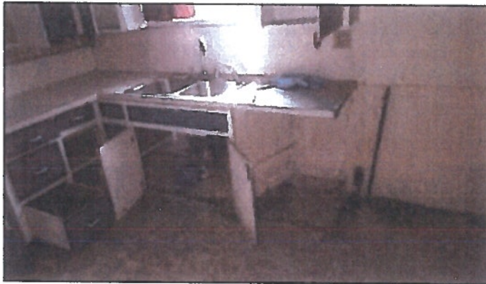
Kitchen is in poor condition overall.
