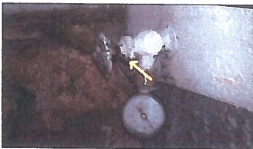
Front faucet leaks under pressure
