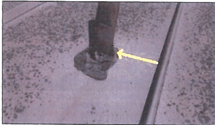
Kitchen plumbing vent
