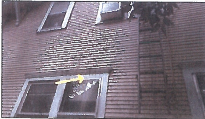
Condensation dripping down walls and window
