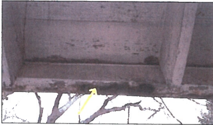
Gutters rusted through
