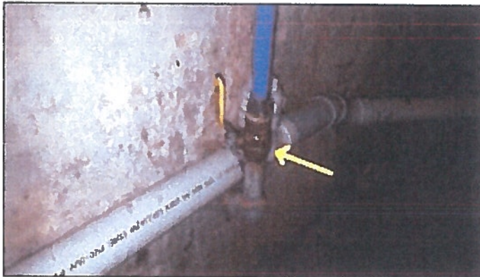
Main water shut off
