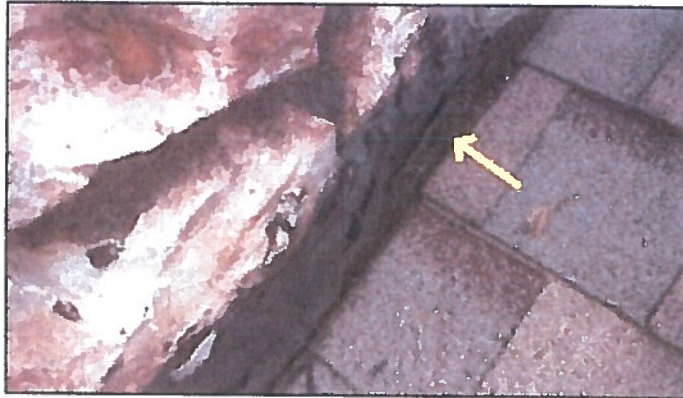
Improper and loose flashing at front chimney
