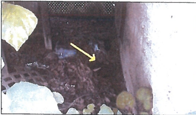
Poor drainage below front porch
