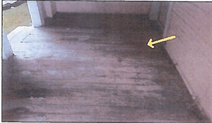
Back porch needs maintenance
