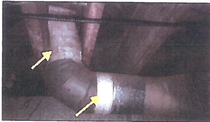
Tape on ductwork likely contains asbestos
