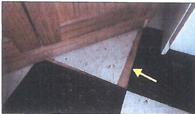
Loose tile below sink - Unit 1
