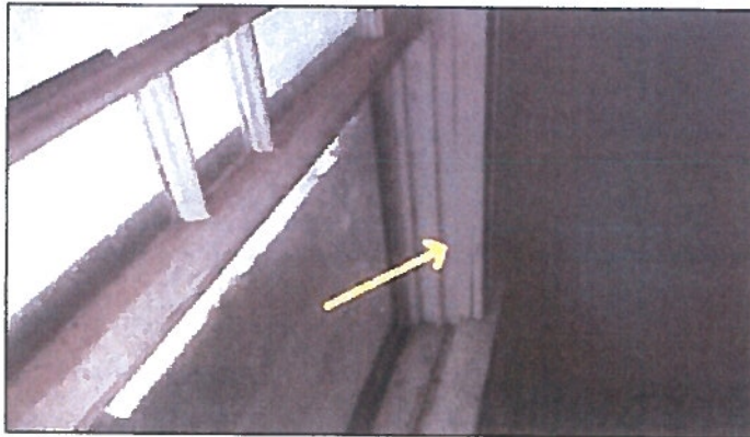
Lower dining room window is missing
