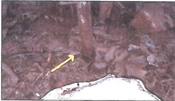
Heavily deteriorated main gas line
