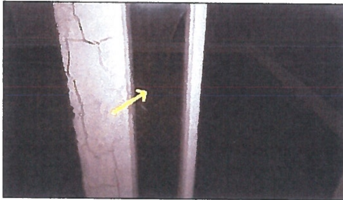
Broken glass in main living area doors.
