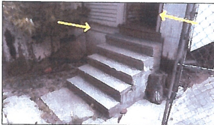
Handrail needed at back steps
