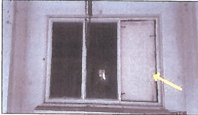
Missing glass at front door
