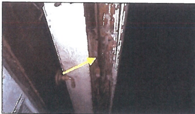
Unit 1 - Front door jamb is damaged
