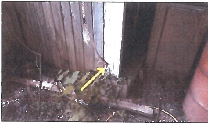
Cord with exposed splice powers garage
