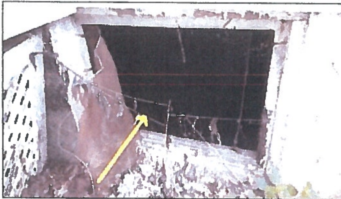
Missing basement window bear back porch.
