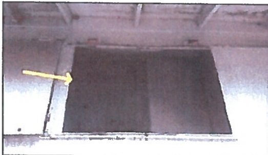
Missing shutter noted
