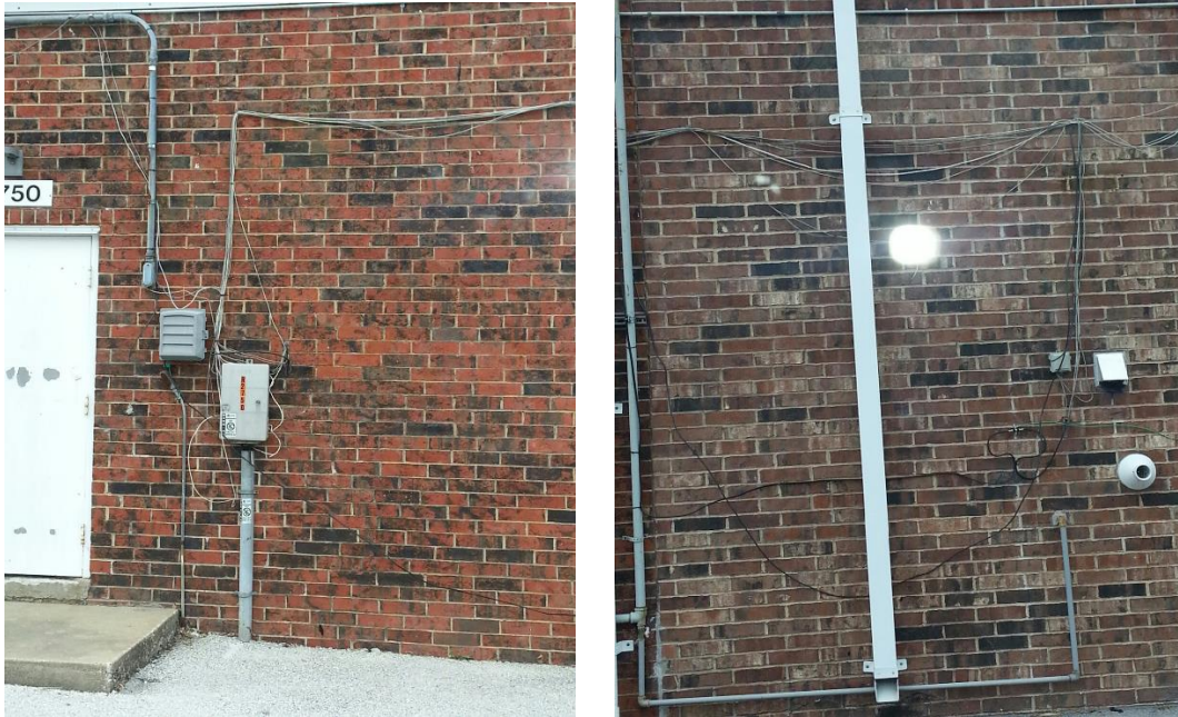
Photo 27-28: Example of various loose wiring on the rear of buildings.
