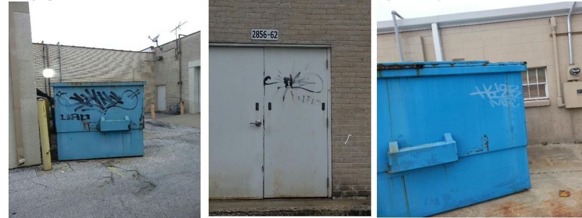
Photos 6-7-8: Sample of area graffiti damage.
