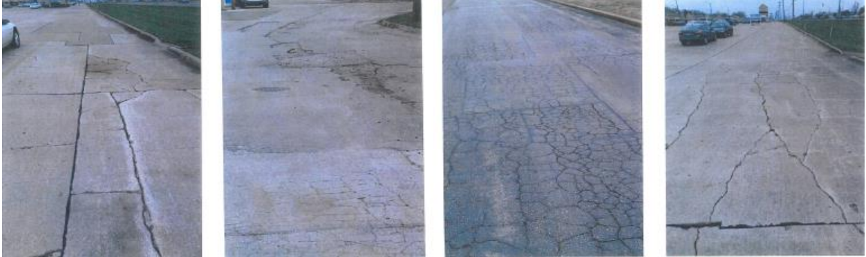
Photos 12-13-14-15: Demonstrate deteriorating conditions of driving lanes and parking field that require removal/replacement.
