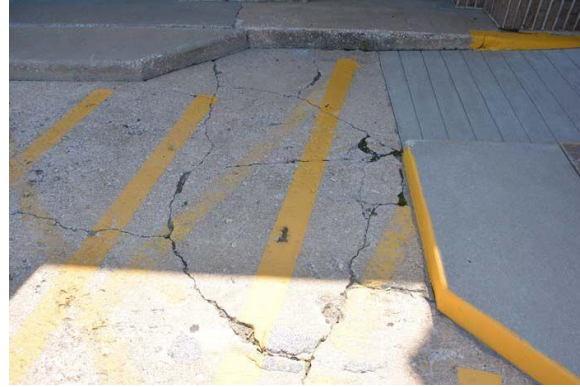
Photo 5: Example of non-ADA compliant sidewalk access.
