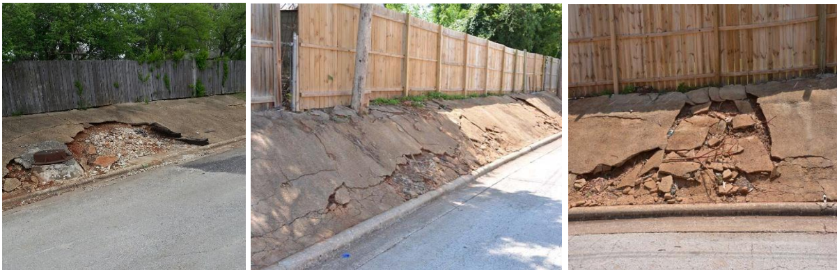
Photos 18-19-20: Examples of damaged soil retention along rear of Study Area.
