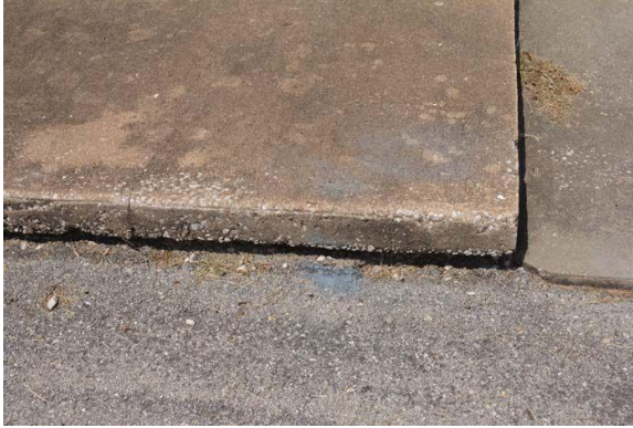
Photo 4: Example of sidewalk displacement between slabs.
