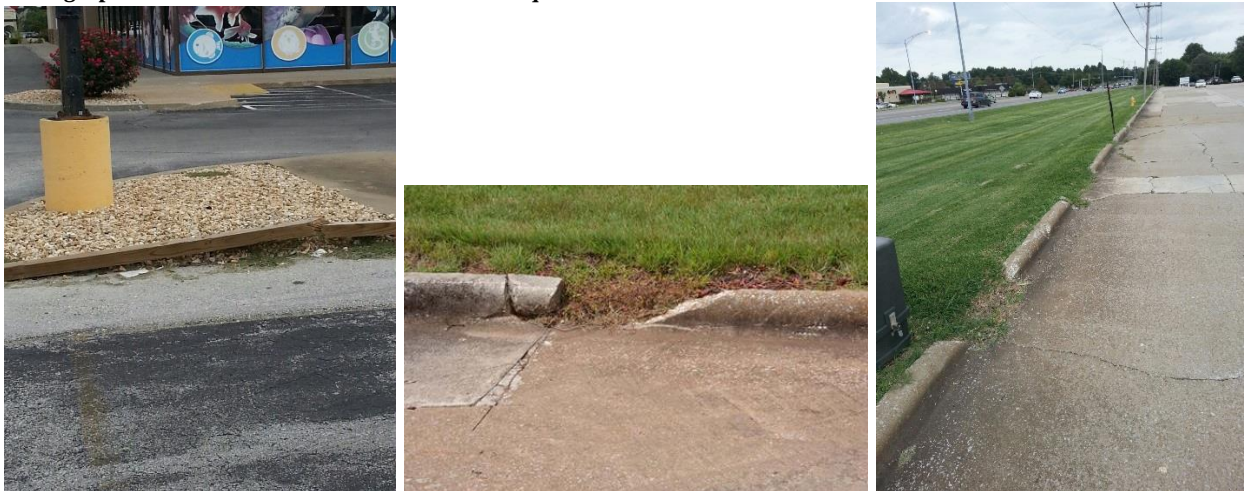
Photo 1-2-3: In addition to several others, these photos provide a sampling of locations damaged and missing curbing.
