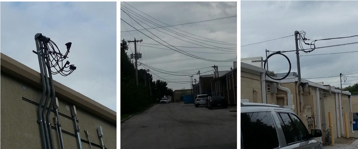
Photos 9-10-11: Demonstrate a myriad of messy, low hanging wires with a history of being torn off the buildings by service vehicles resulting in a danger of creating fires, electrical disconnections, etc...
