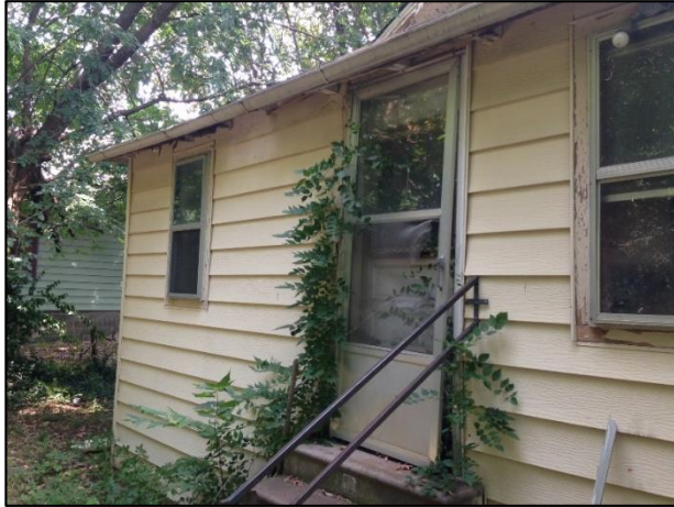
A23.) Vegetation growing through the back door and into the structure
