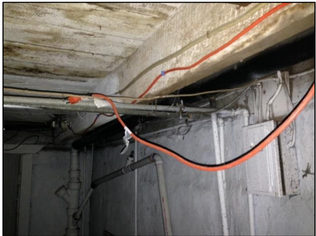
A20.) Extension cord being used for permanent wiring
