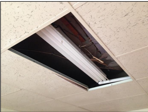
A15.) Exposed wiring throughout living areas
