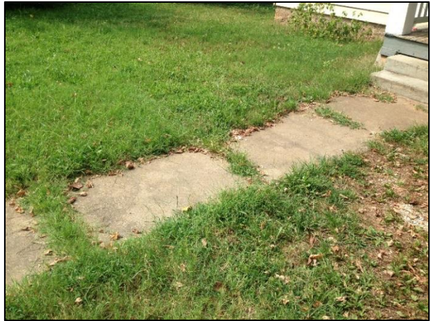
A14.) Overgrown and un-level sidewalk
