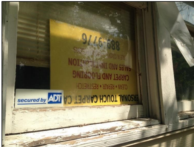
A29.) Broken windows create an easy access point for intruders
