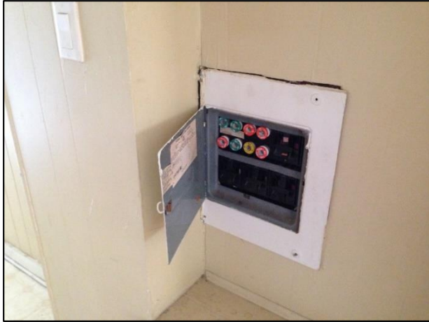
A17.) Outdated electrical system
