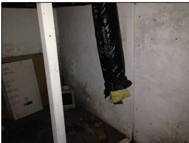
A21.) Detached ductwork
