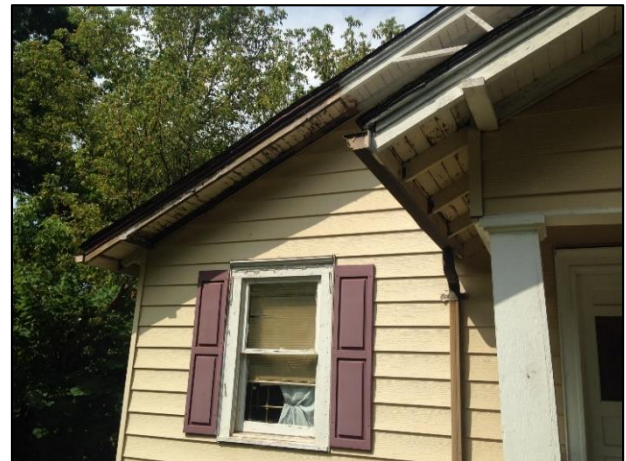
A4.) Exposed raw wood in fascia and rotting window with chipping paint
