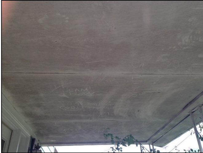
A28.) The dirty front porch ceiling has been graffitied
