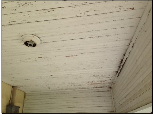
A6.) Chipping paint on front porch
