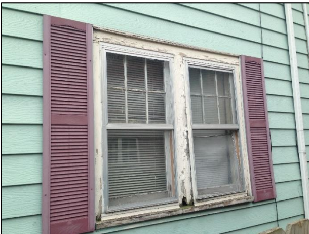
A3.) Rotting window framing and chipping paint
