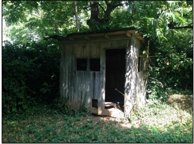
A12.) Out building is deteriorated and door has been kicked in by a vagrant.
