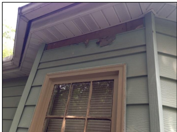
A22.) Failing/missing siding
