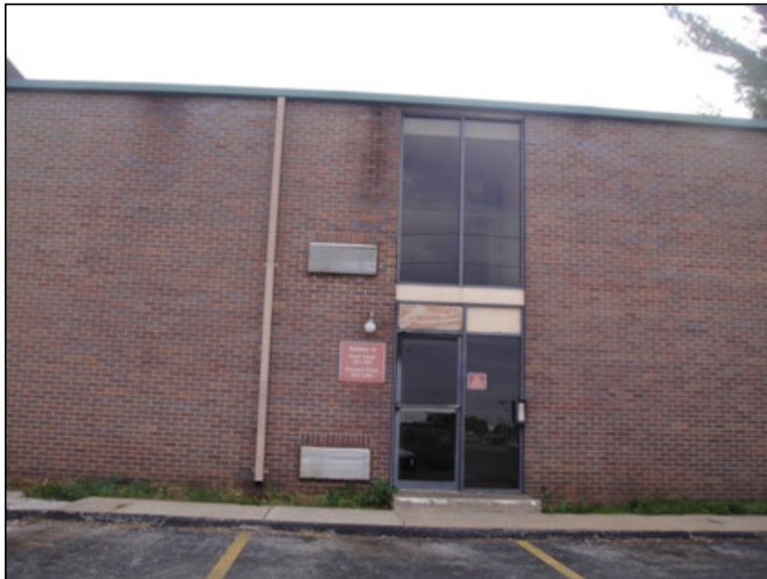
Failure of exterior systems (Water penetration down brick mortar joints, shown as dark vertical lines) Also note, boarded/compromised window above doorway.
