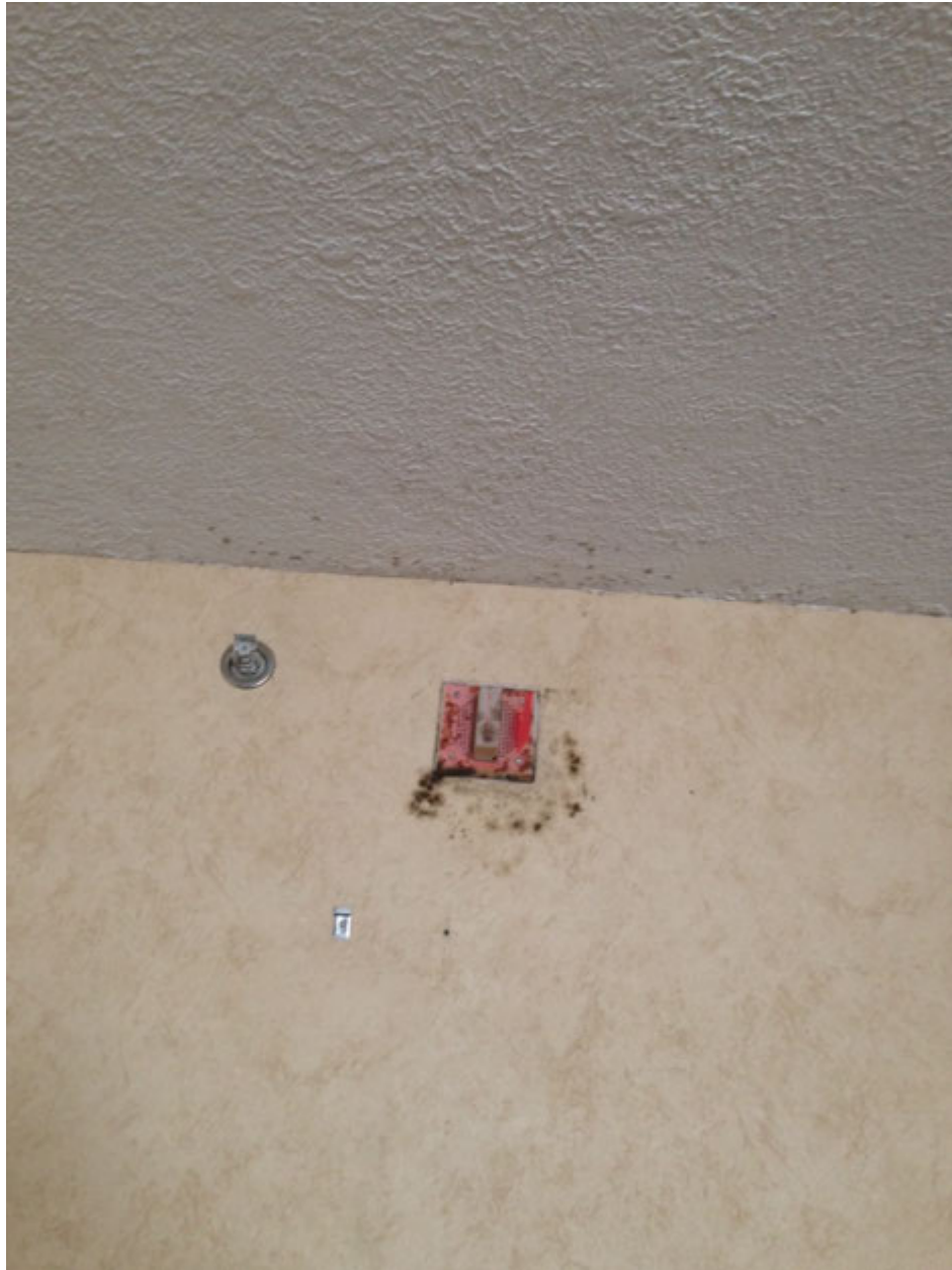
Suspect Black Mold growth on interior walls of rooms.
