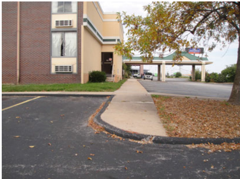
Deteriorated sidewalks and curb cuts
