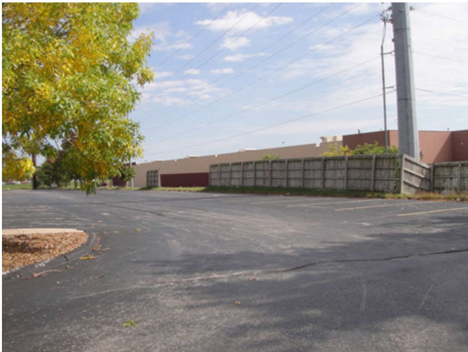
Deteriorating Site Improvements (Broken Fencing)
