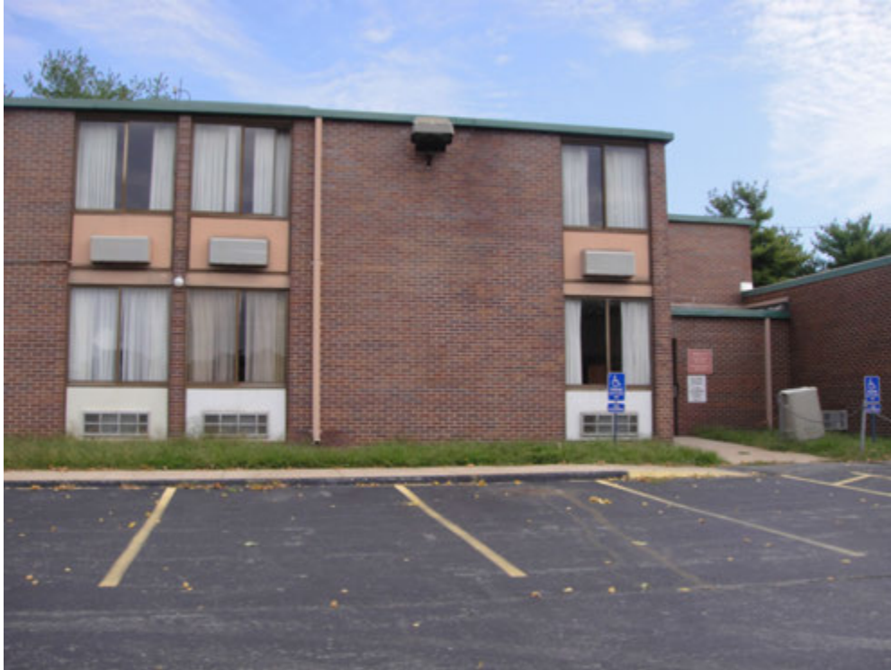
Deteriorating façade (Water Damage)
