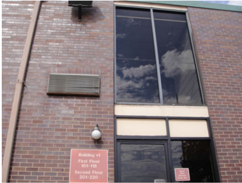
Deteriorated window moldings
