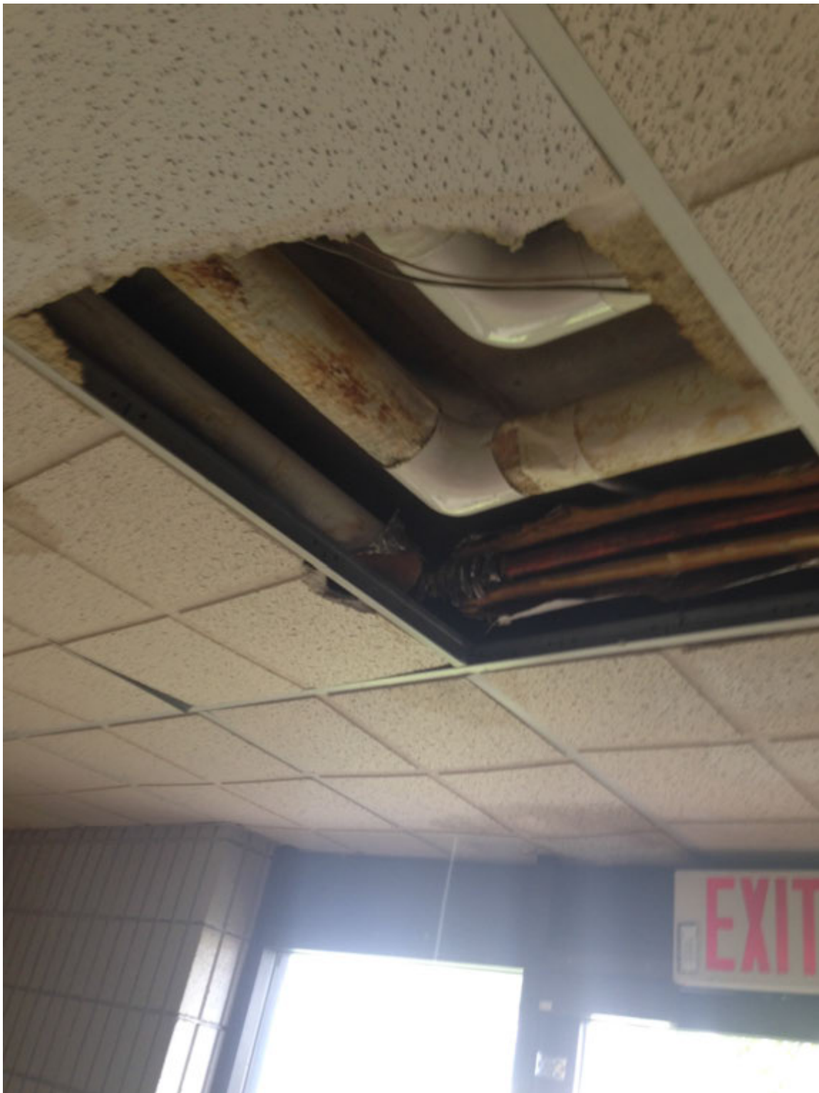
Deteriorating Plumbing Infrastructure
