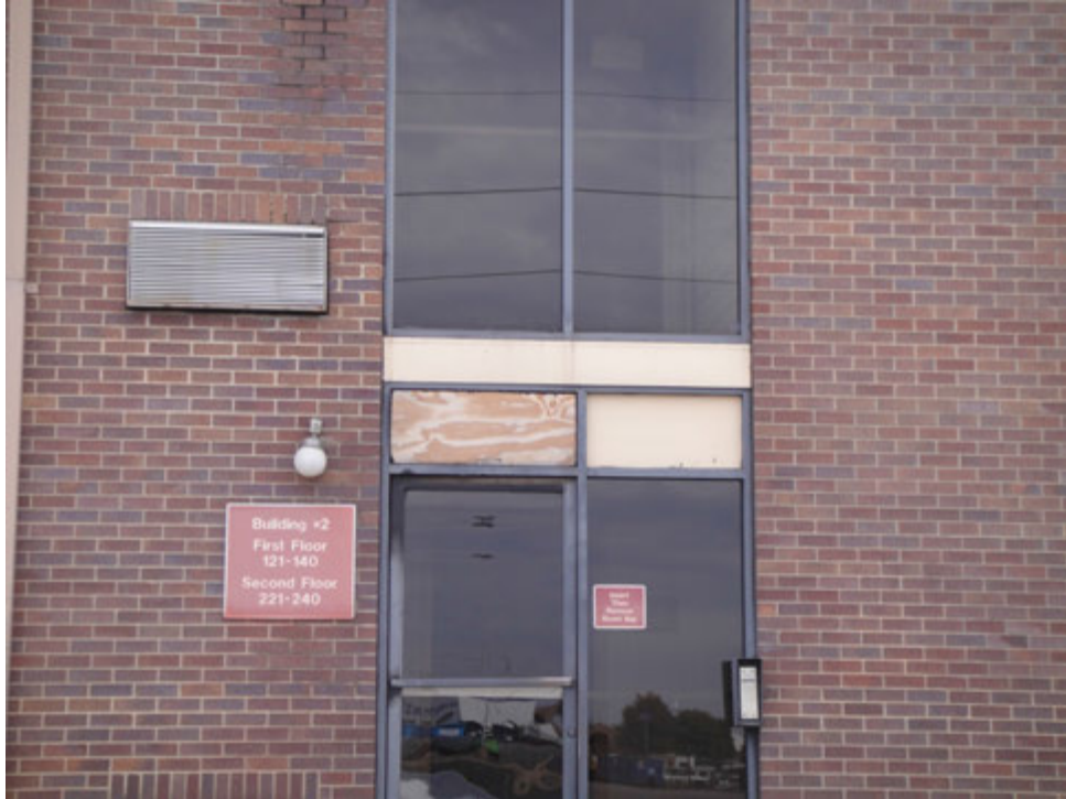
Deteriorating Site Improvements (Broken Windows)
