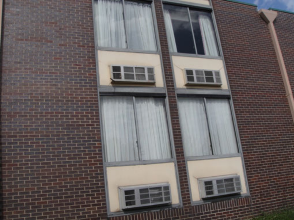
Deteriorating Exterior Building Envelope
