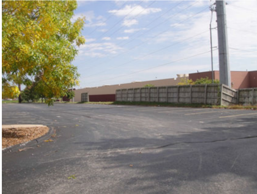
Missing Fencing Segments
