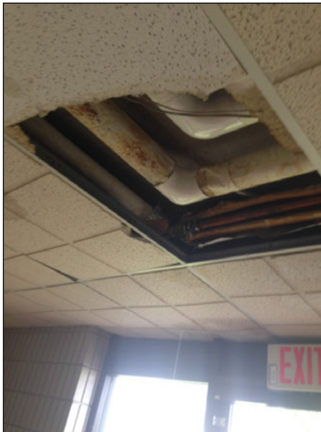
Deteriorated plumbing infrastructure
