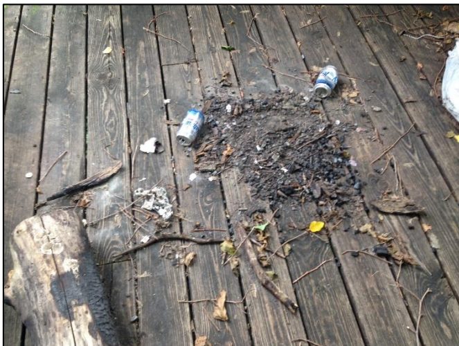
37.) Vagrants have lit a fire on the rear deck of one of the structures.
