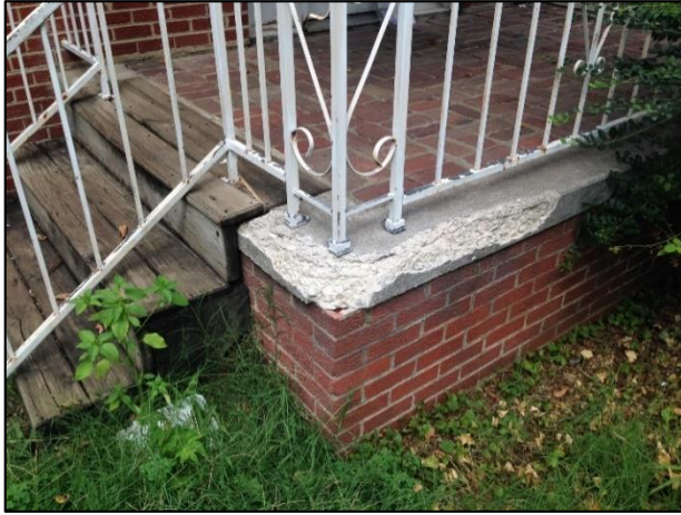
A5.) Failing porch foundation and deteriorated Front entry stairs
