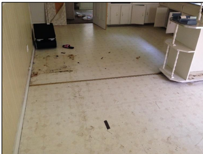
36.) Filthy interior flooring is throughout
