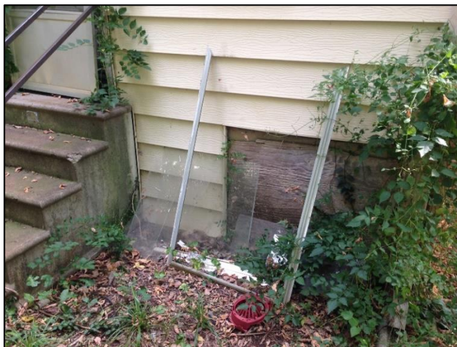
A30.) Broken glass on the ground near the rear steps from an old storm window which has been removed.
