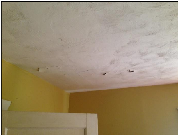
A7.) Failing sheetrock from squirrels living in the attic space
