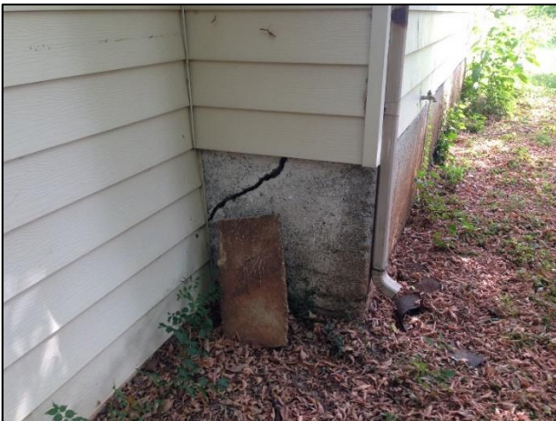
A13.) Cracked and failing foundation
