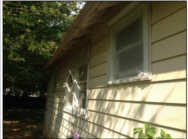
A2.) Failing windows have been covered in plastic
