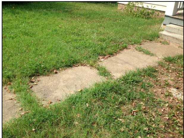
A14.) Overgrown and un-level sidewalk
