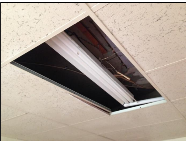
A15.) Exposed wiring throughout living areas
