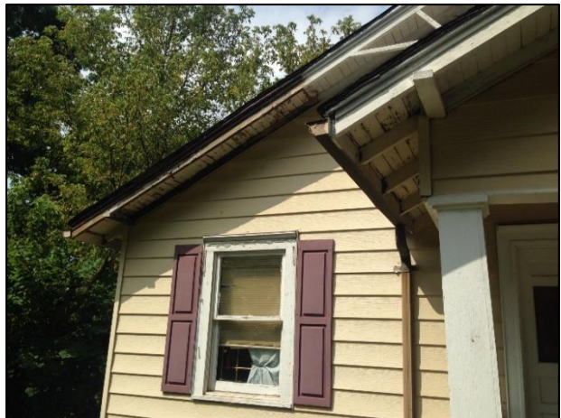
A8.) Soffit and Fascia is deteriorating
