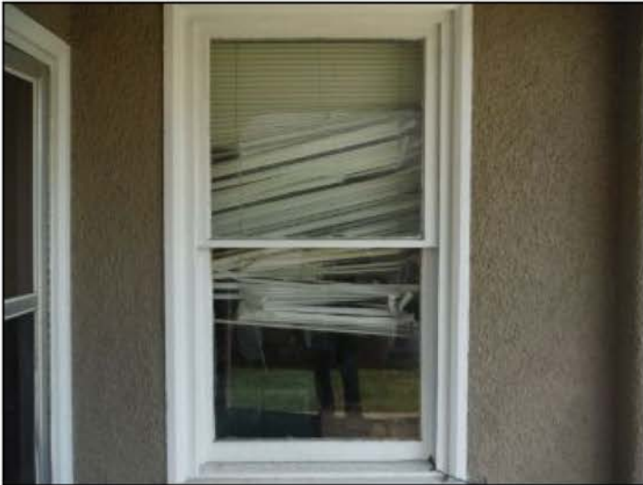
Recommend replacement of older wood units, missing storms/screens noted
