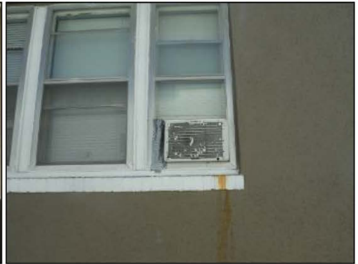
Missing screens/sashes noted
