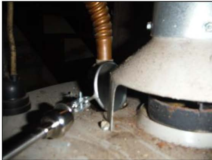
Persistent back drafting, related to being vented into masonry chimney
