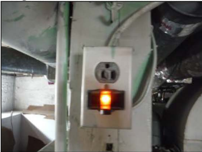
Ungrounded outlets found, refer to electrician
