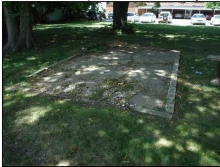
Deteriorated concrete parking pad is past garage floor/foundation
