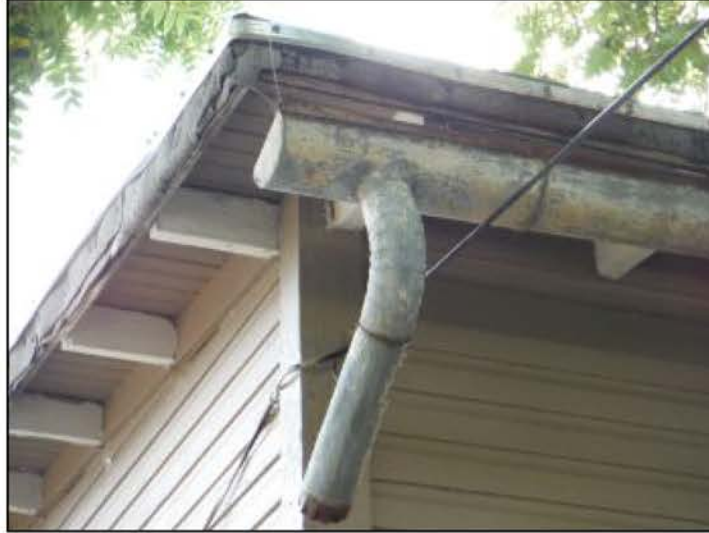
Partial system needs maintenance
