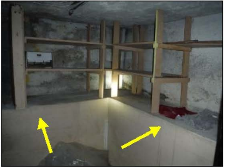
Chicago shelving (concrete)
