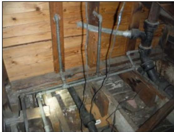
Plumbing needs insulating
