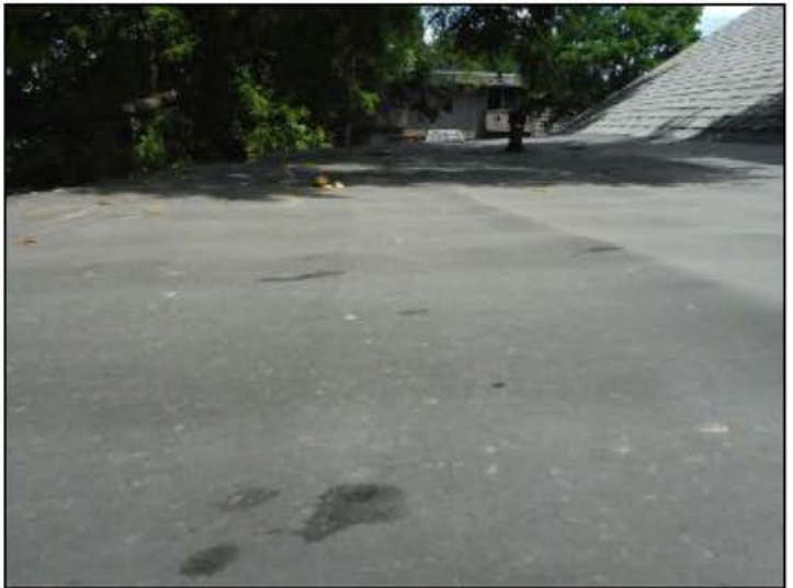
Spongy, stains are sign of ponding
