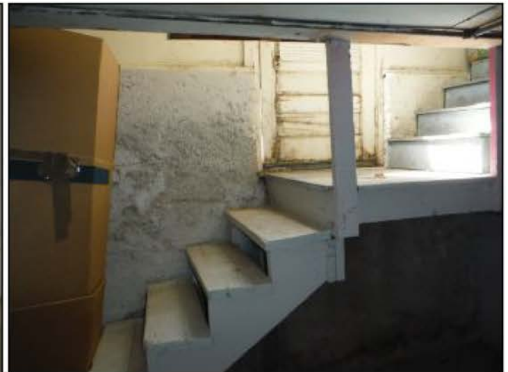
Older standards, low head clearance, under lighted, no hand rails and blocked by basement partition
