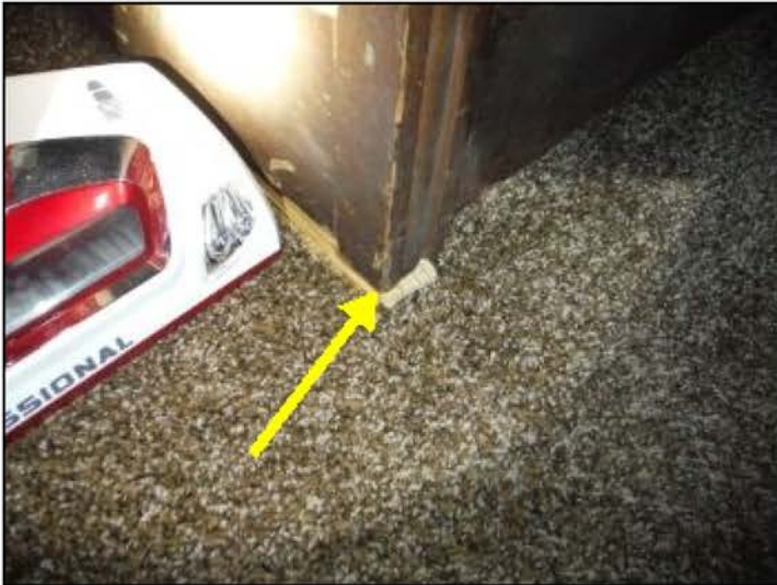
Uneven/sloped areas, photo is shim at tenants furniture
