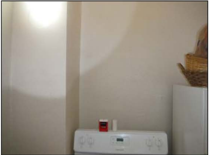
No exhaust hood provided
