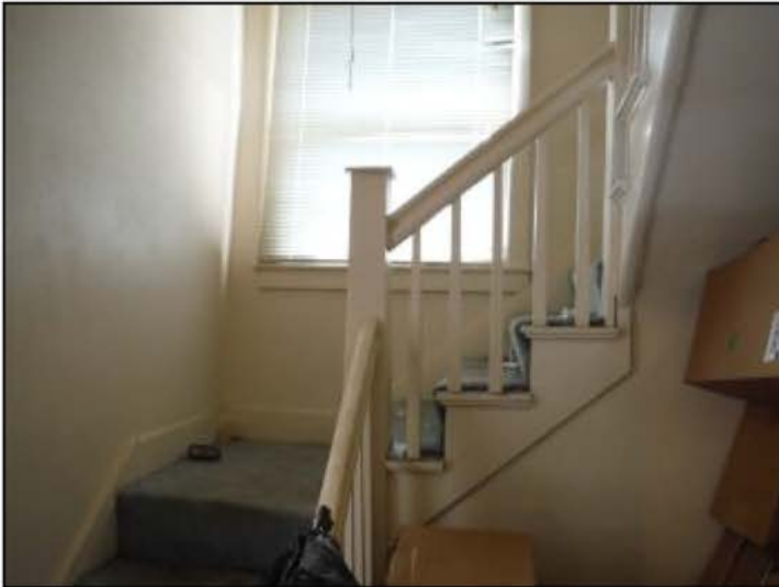
Winding stairs are to older standards, low head clearance noted
