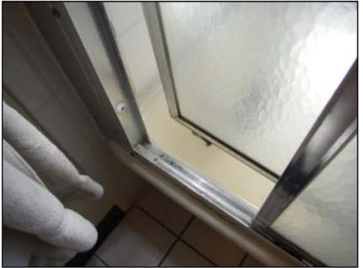
Missing guide needed
