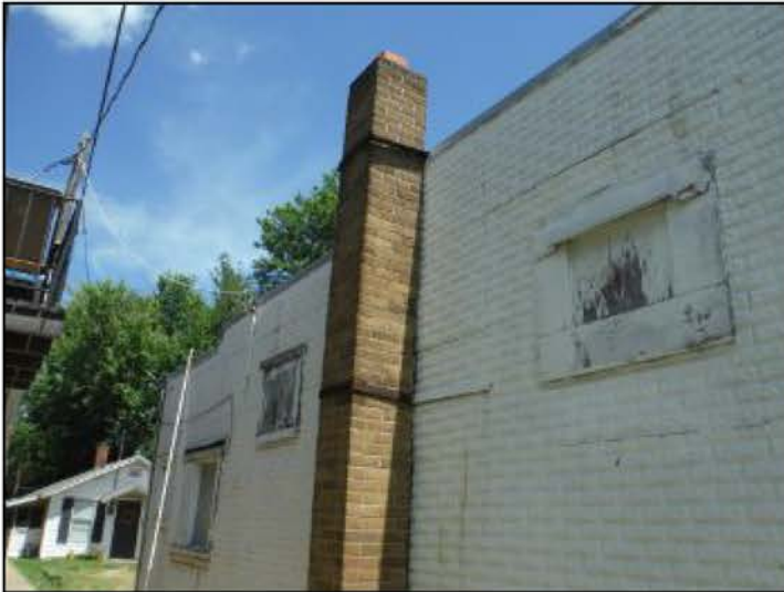
Deteriorated masonry, note gaps at wall and rusted steel anchoring
