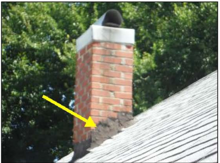
Mastic coated chimney flashing needs periodic recoating
