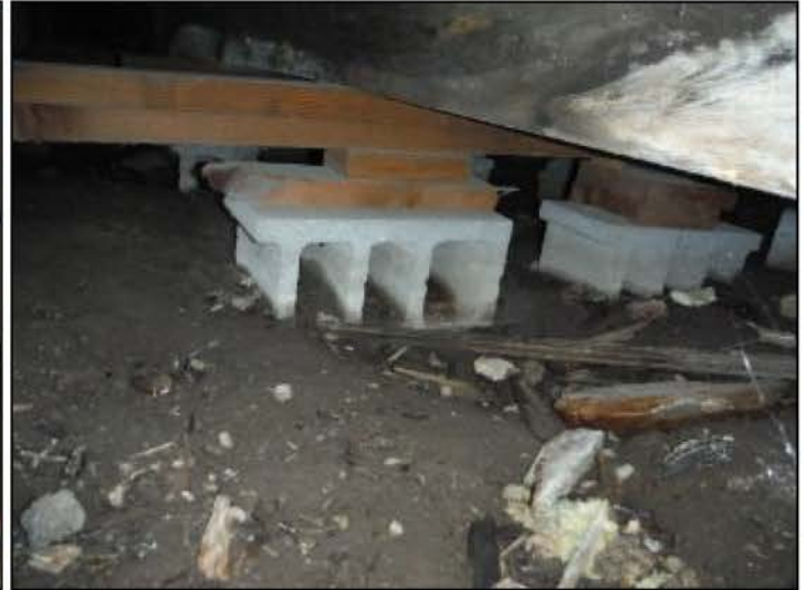
Too low to crawl, this view from damage/hole
