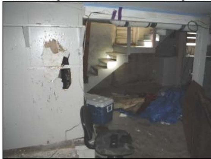
Damaged finish limits inspection
