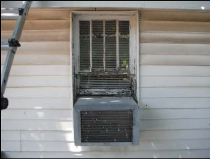
Older package air conditioner has limited life
