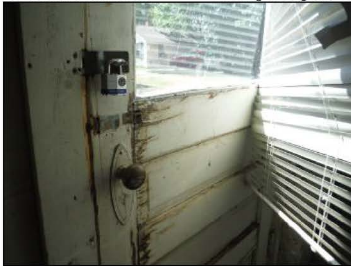
Basement unit is moisture damaged
