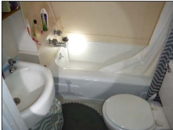
Undersized area/room, not universally accessible
