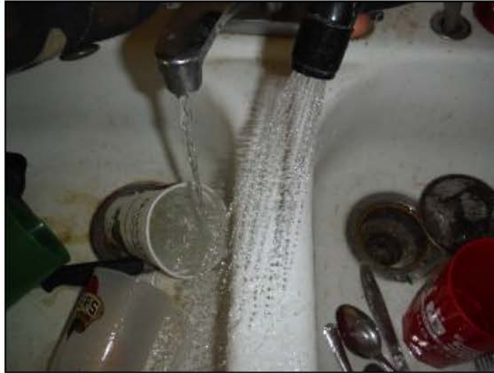
Worn sprayer diverter
