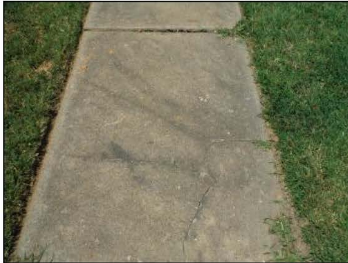
Trip hazards noted
