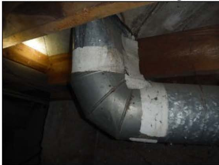
Suspect asbestos tape at ductwork noted
