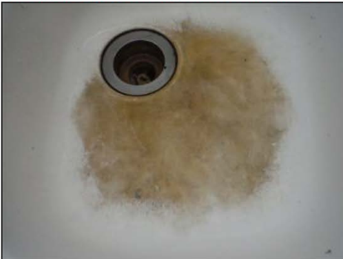
Serviceable unit, stains/wear noted
