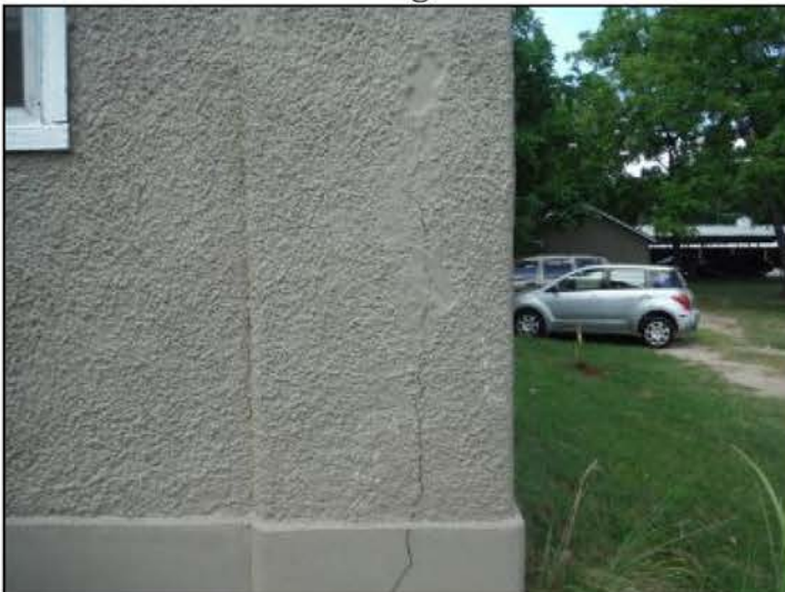
Common cracks at stucco
