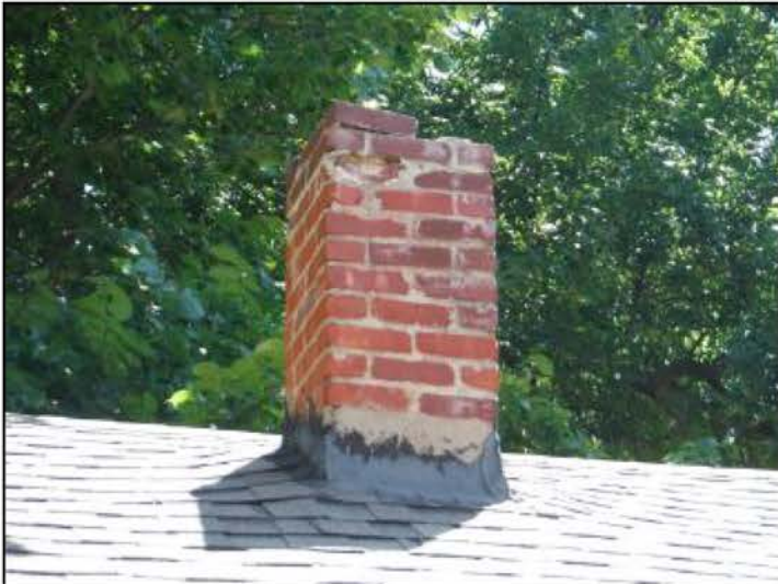
Very deteriorated, appears unlined brick masonry
