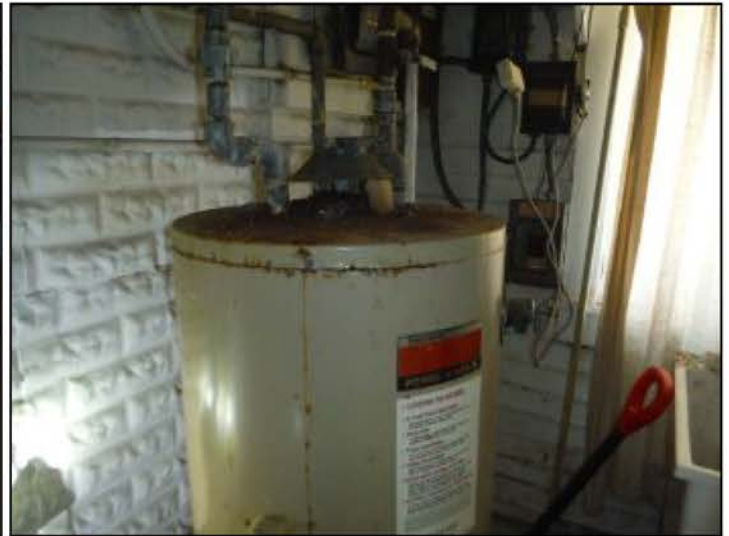
Disconnected (abandoned status)
