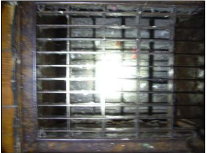
Some original ductwork needs cleaning
