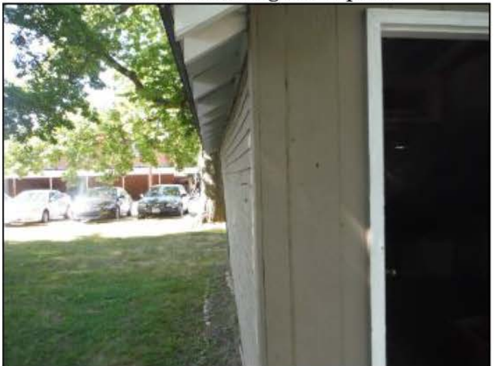
Side walls are leaning (building is wind racked)
