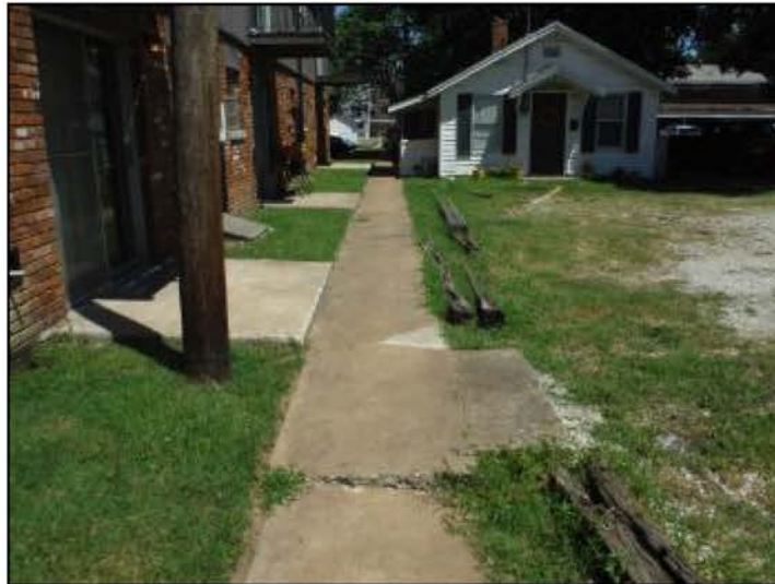
Very deteriorated, trip hazards
