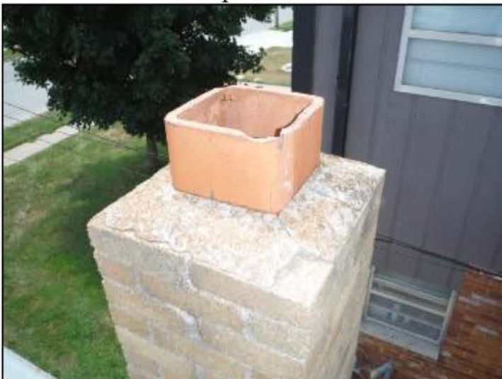
Missing rain cap and screen, water and birds can enter
