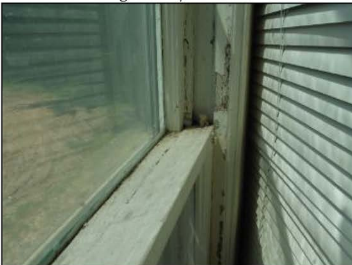
Missing sash cords, old style counterweight system
