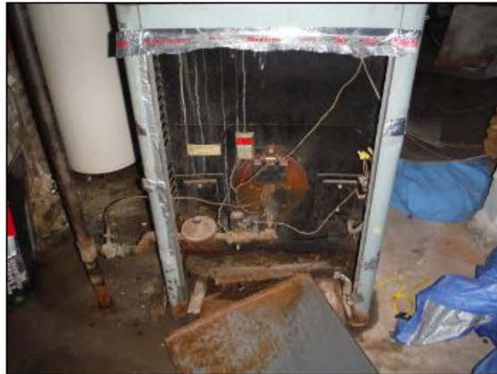
Poor maintenance, refer to HVAC technician
