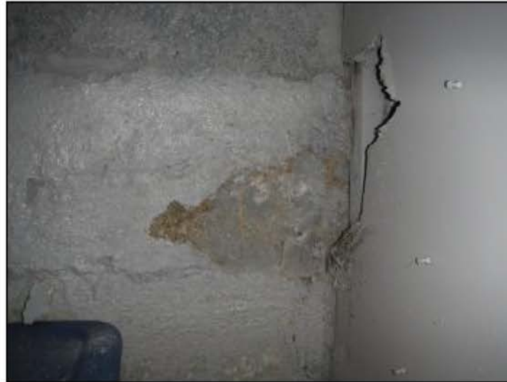
Peeling finish/stains are sign of moisture
