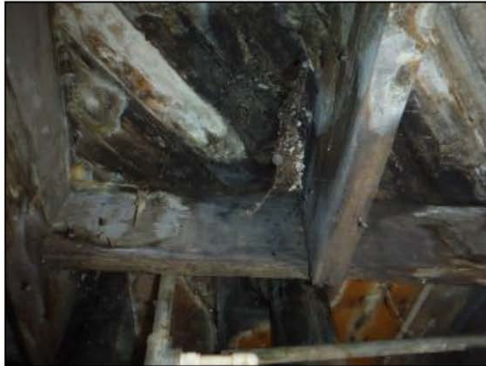
Unrepaired minor damage below half bath observed
