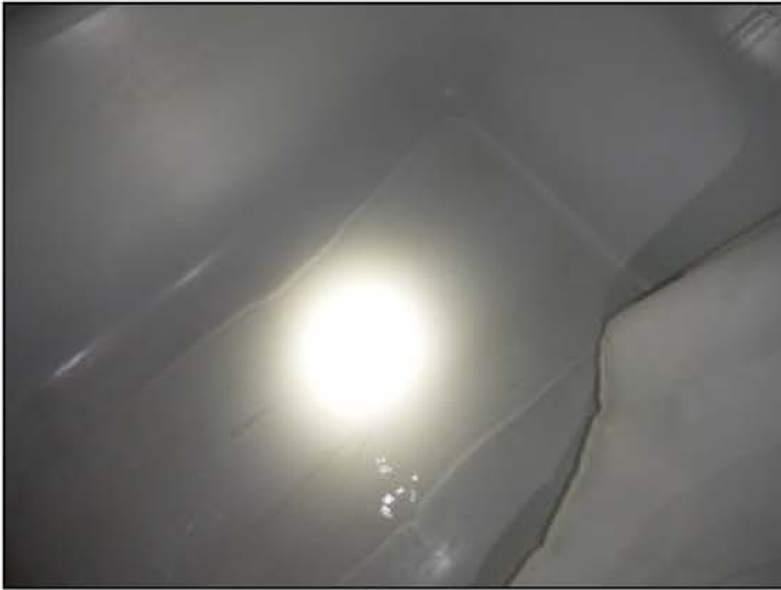
Does not drain properly, unit not level
