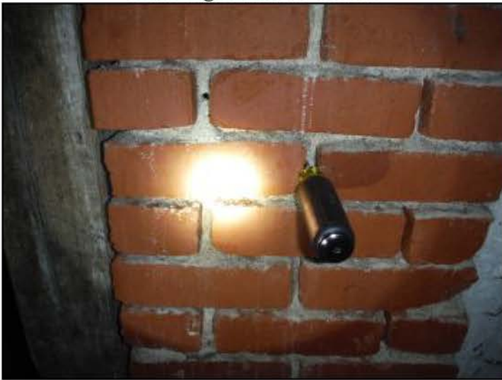
Deteriorated mortar at basement
