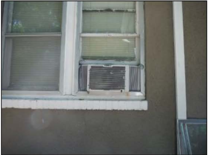
Older window air conditioners beyond scope
