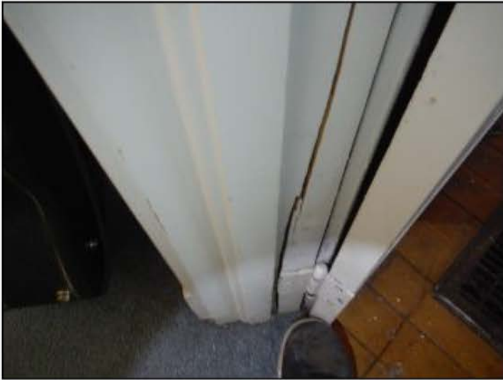
Damaged upstairs unit
