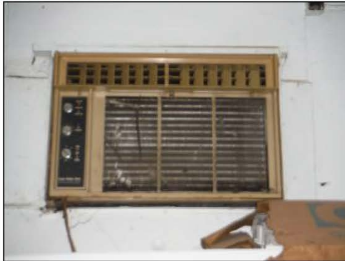
Inoperative older package/wall air conditioner
