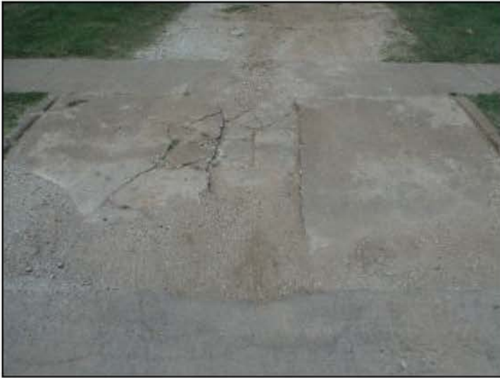
Deteriorated approach at shared driveway
