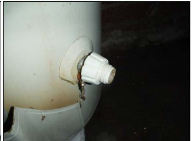
Tank drain valve leaks, needs a cap
