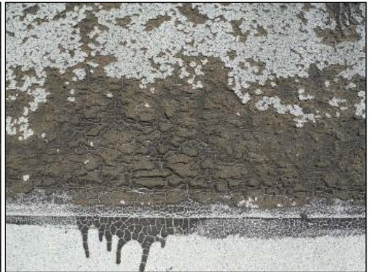
At end of life, needs replacement when reroofed
