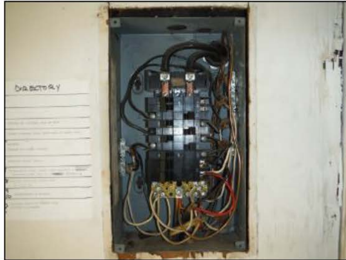
Serviceable older 100 Amp breaker panel
