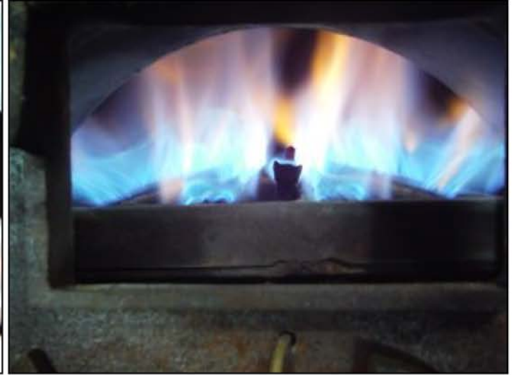
Rusty barrel type heat exchanger might be 50% efficient
