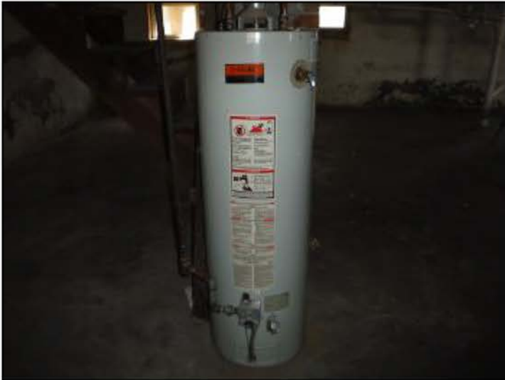
Old standard, burns basement air, suggest upgrade
