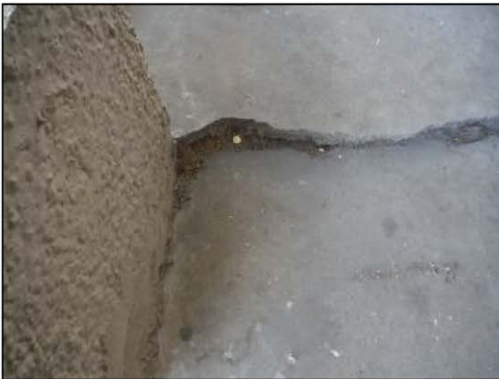
Serviceable concrete is cracked and settled (apx. one inch, both sides)
