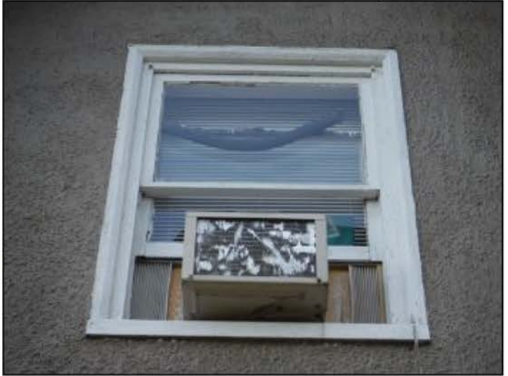
Window air conditioner untested, beyond scope
