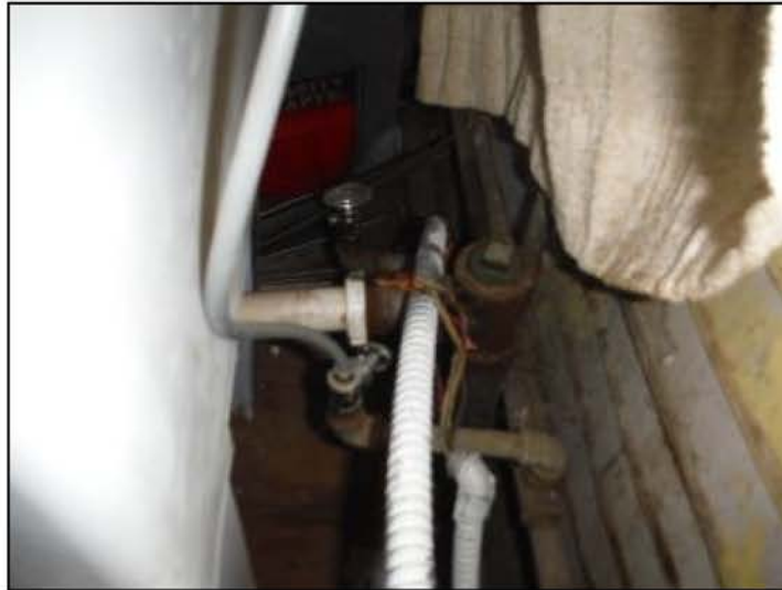
Older waste piping untested, water off
