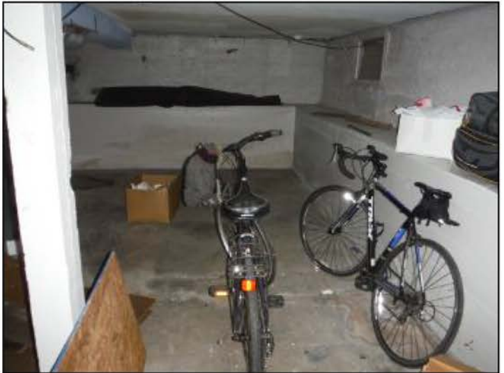
Dry today, signs of past dampness
