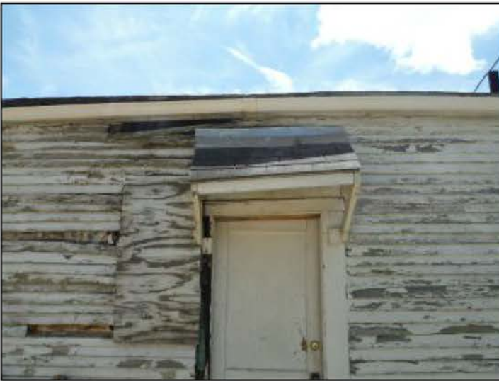
Damaged siding needs repair, moisture entering wall/s
