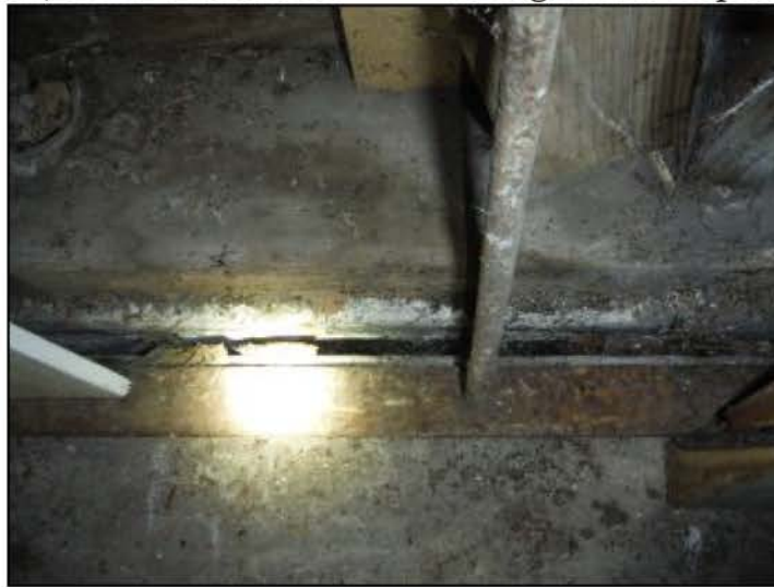
Refer to termite inspection report
