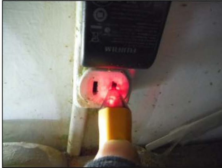
Miswired outlets, refer to electrician
