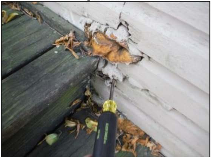
Rotted siding observed
