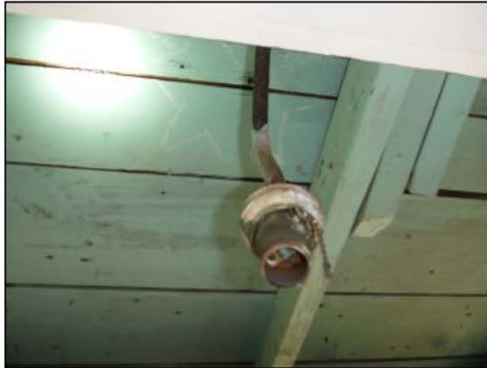
Old school light fixture is shock hazard
