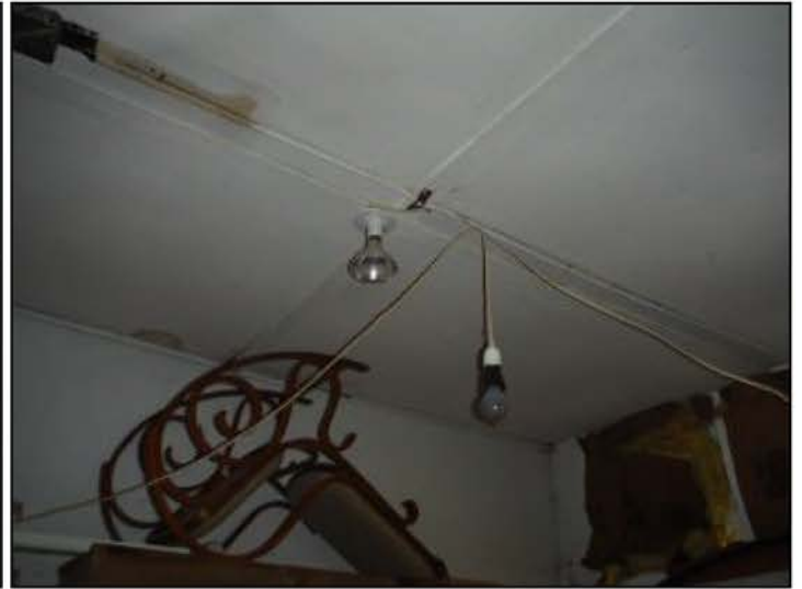
Unsecured wiring, refer to electrician
