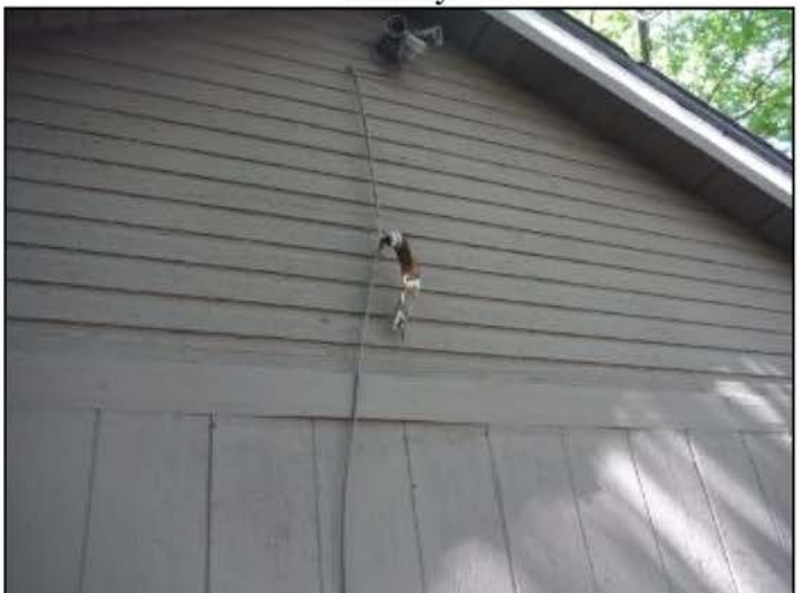
Disconnected out to detached garage (no power there)
