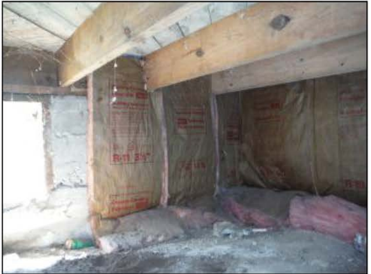
Insulation limits inspection
