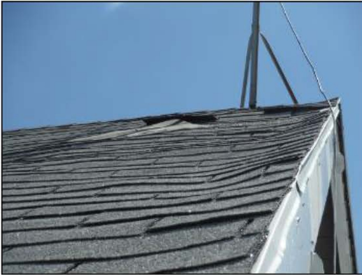
Refer to qualified roofer to do maintenance, replace missing shingles, seal flashing as needed
