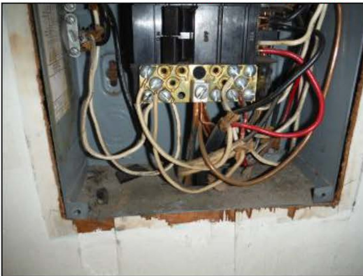
Most is two wire romex, cannot have grounded outlets unless rewired
