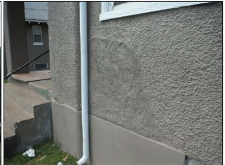
Patched stucco observed
