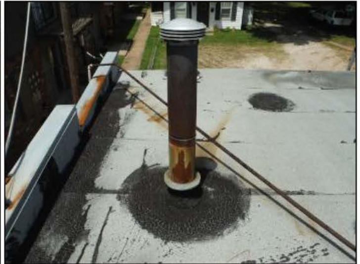
Disconnected (abandoned status)
