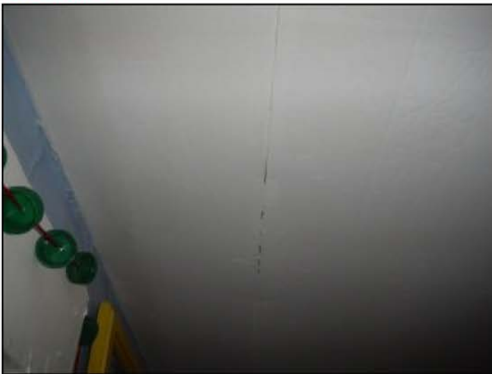
No access at ceiling, patched areas noted
