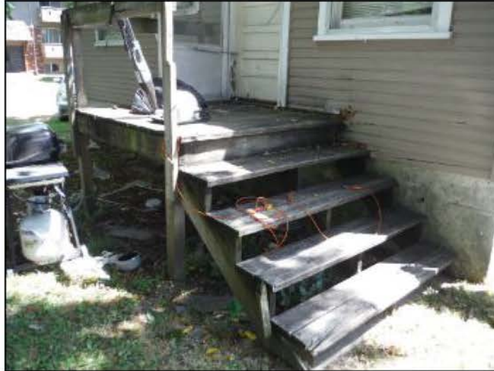
Missing railings, not to current standards
