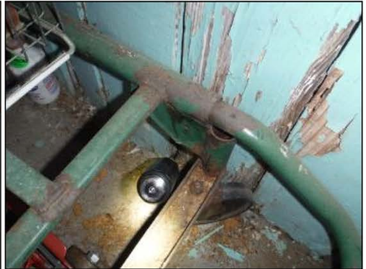
Rot measured at wood walls of screened porch
