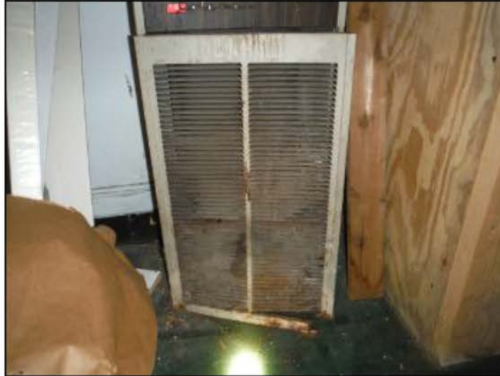
Old rusty unit needs to be replaced
