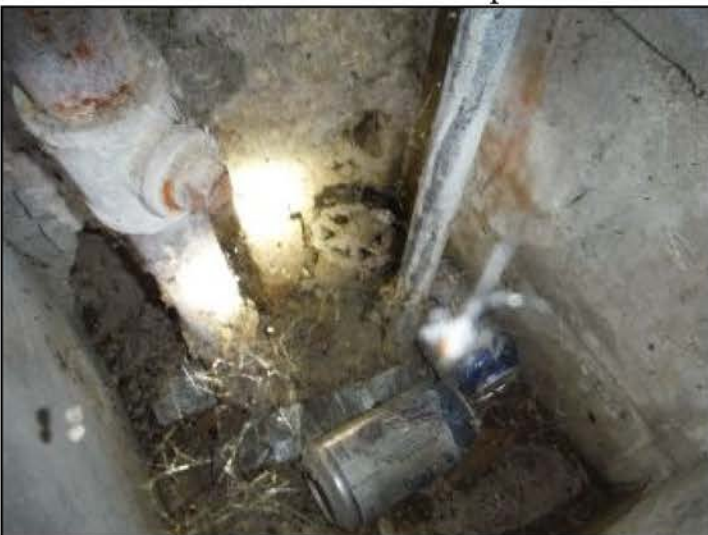
Older sump pump has limited life
