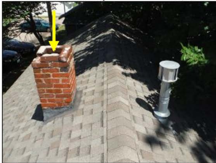
Water and birds can enter chimney
