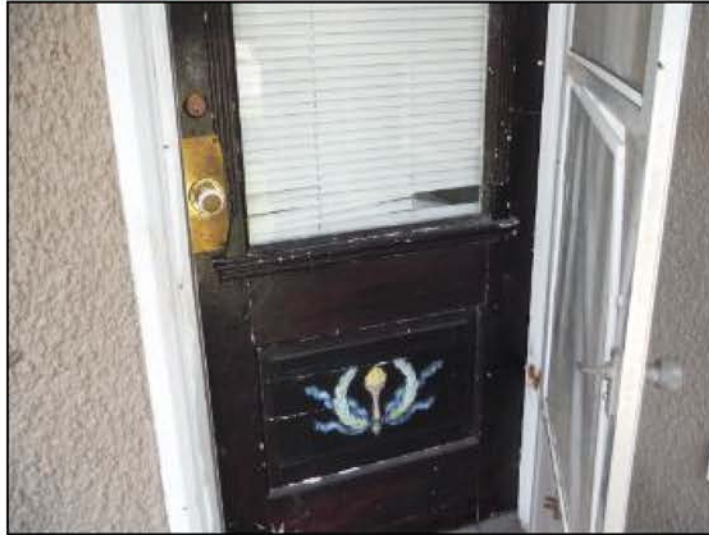
Untempered glass not to current standards
