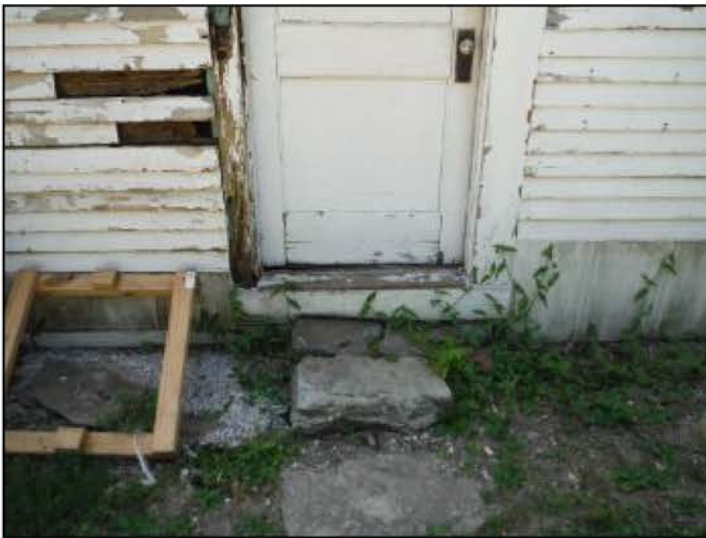
Trip hazards at back door, no proper stoop
