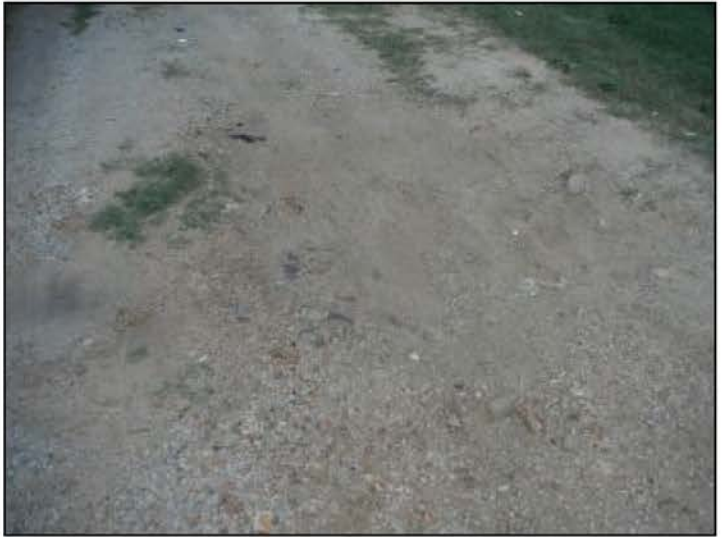
Eroded gravel at shared drive
