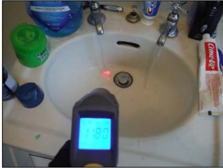
Old standard, separate hot/cold faucets
