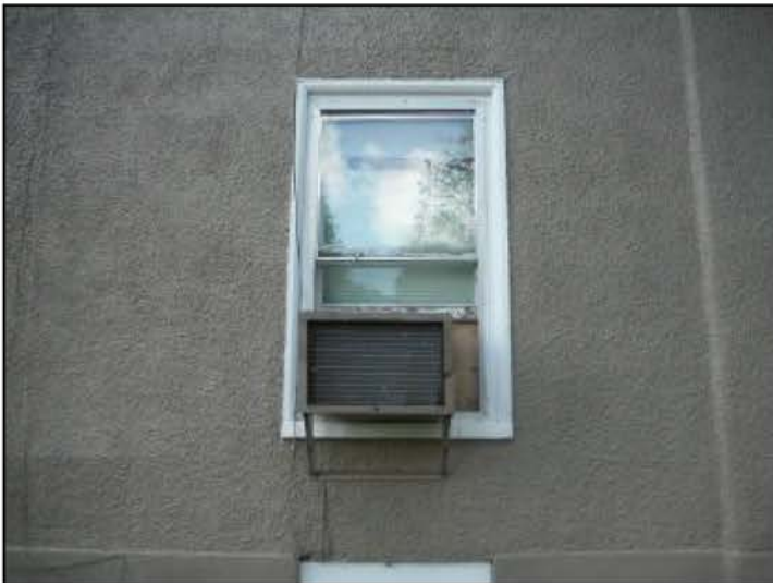
Window air conditioner untested, beyond scope
