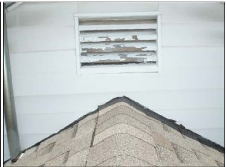
Limited view at gable vents
