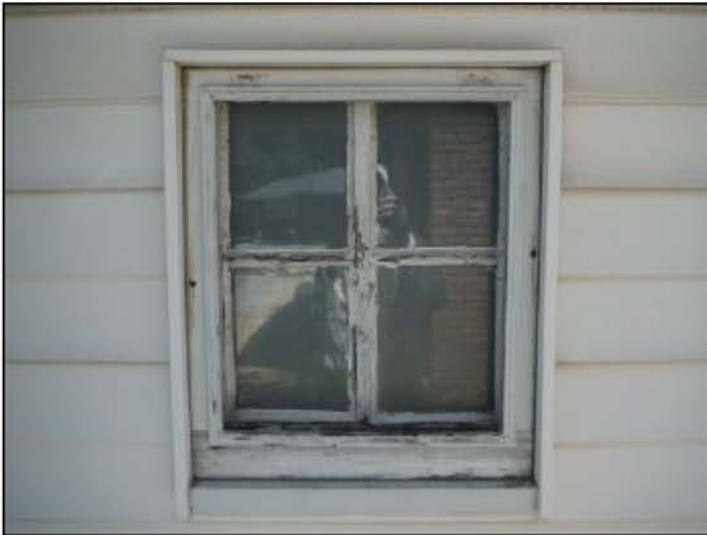
Older wood units need paint maintenance
