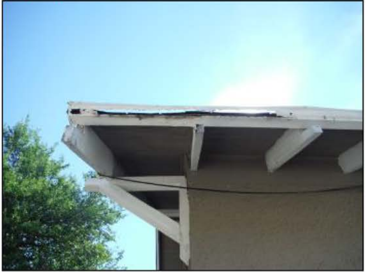
Rusted/damaged/incomplete guttering needs removal/replacement
