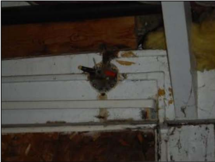
Unsecured wiring, refer to electrician
