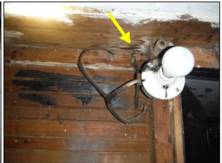
Active knob and tube wiring confirmed at basement and attic, refer to qualified electrician to update
