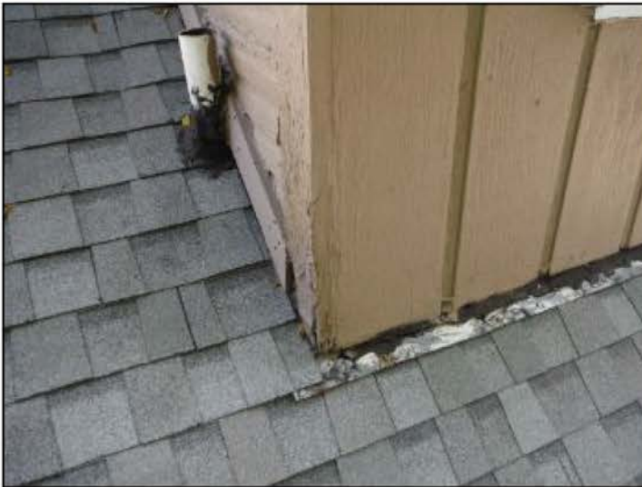
Refer to qualified roofer to seal/repair/maintain pipe/transition/chimney flashing
