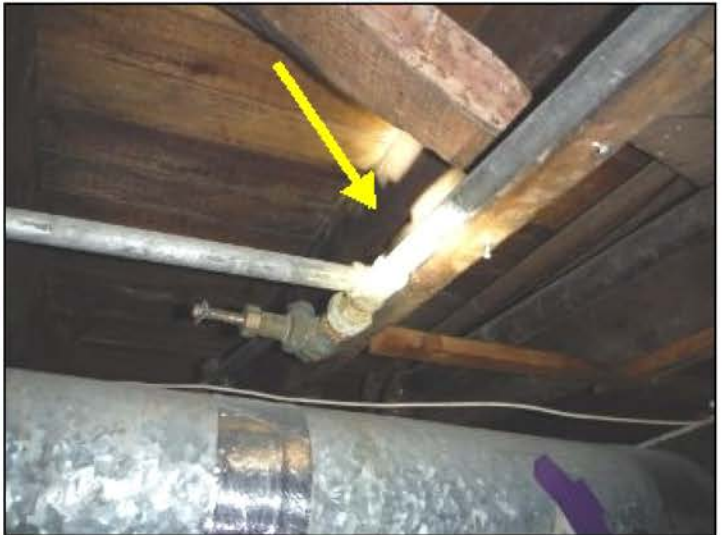
Leaking at basement, refer to plumber
