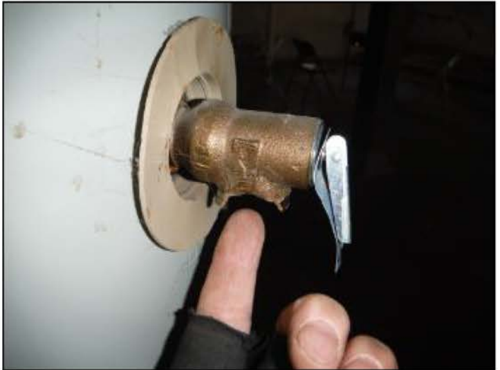
Missing overflow pipe at TPR valve
