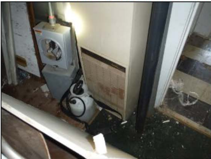
Untested older unit needs upgrade/replacement
