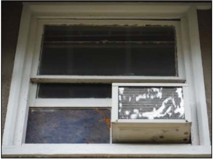
Window air conditioner untested, beyond scope
