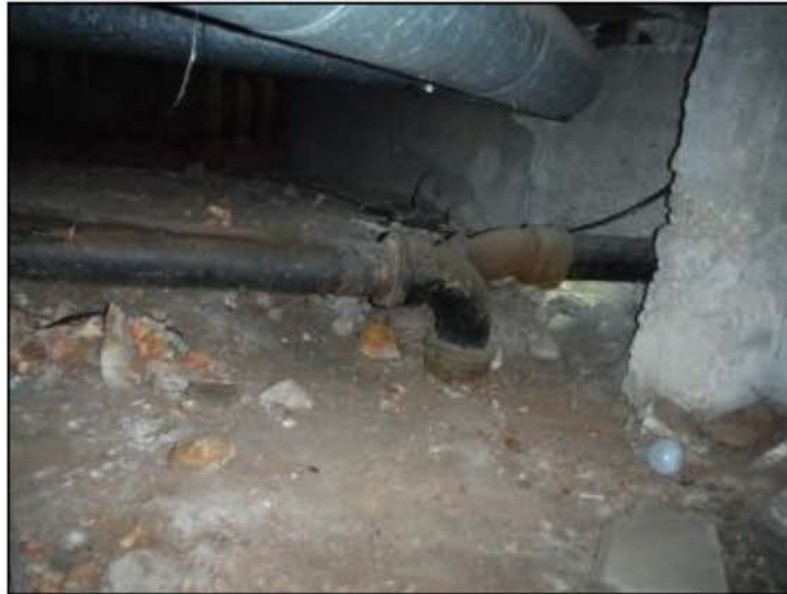
Most is older cast iron
