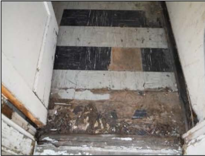
Damaged at back door
