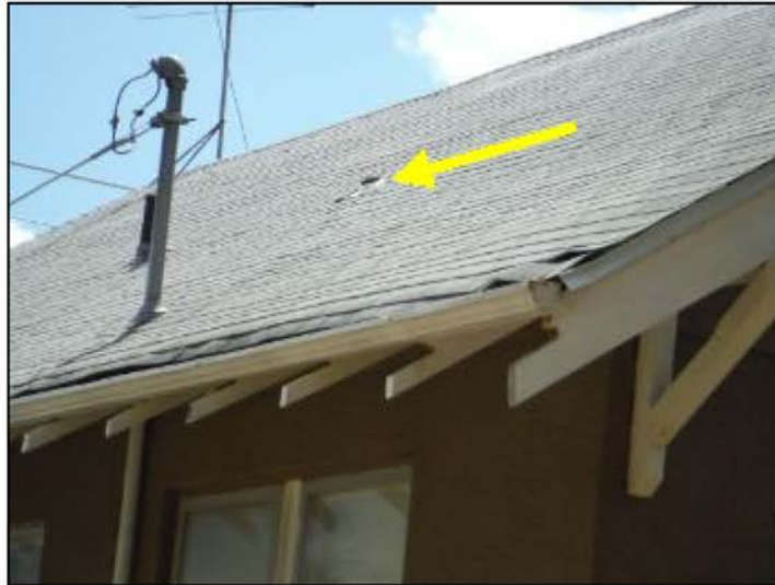
Plumbing vent and/or flashing need/s attention
