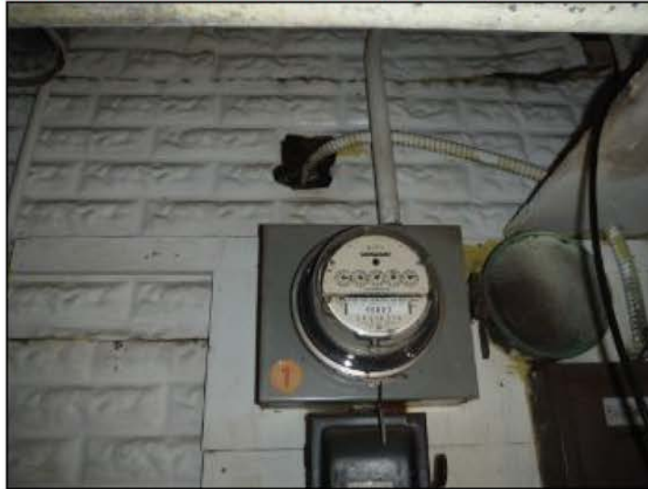
Meter inside, not to current standards for commercial property
