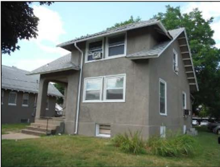
Real stucco needs regular maintenance
