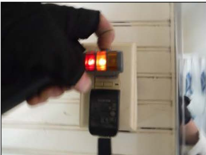
GFCI did not trip
