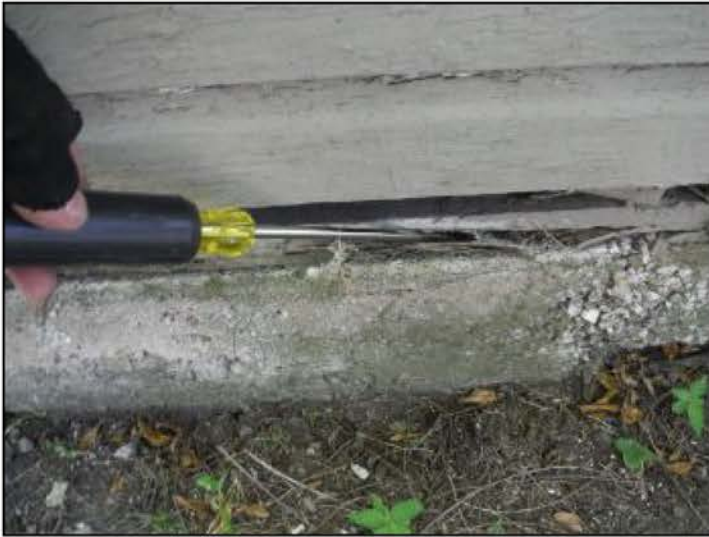
Refer to termite inspection report
