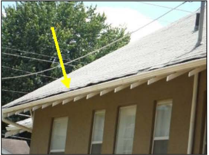
Unsightly curl at eaves/gutters noted (no drip edge flashing, shingles unsupported)
