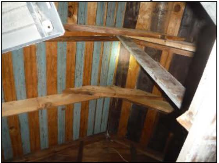
Has newer bracing and repairs
