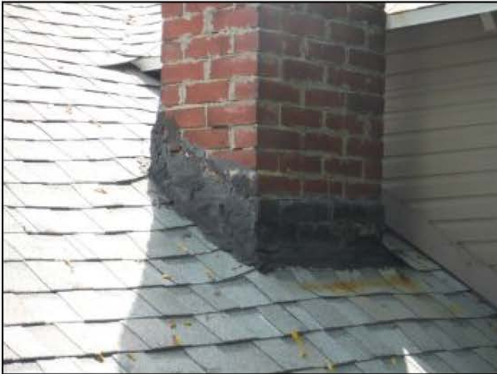
Flashing is mastic coated
