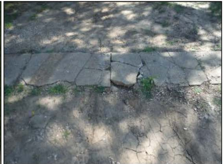
Older/deteriorated concrete walks are at/near end of normal life
