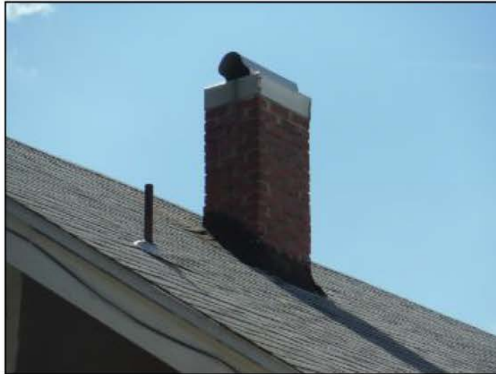
Vents water heater and floor furnace
