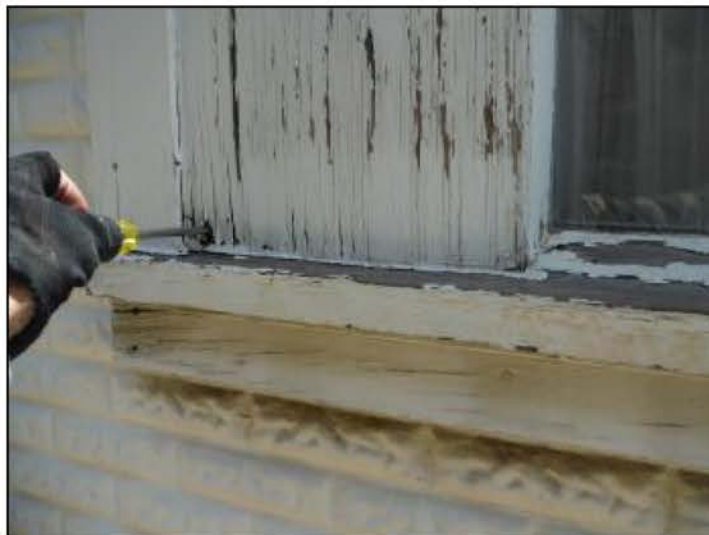
Wood trim needs a good paint job, rot in places
