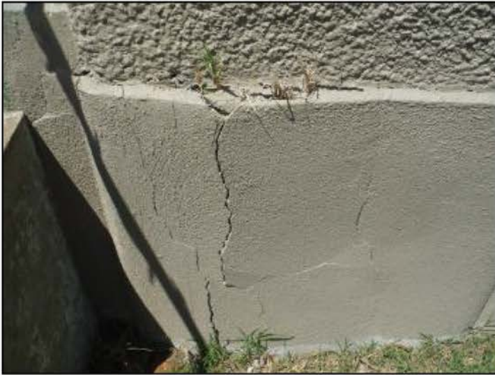
Common cracks relative to age
