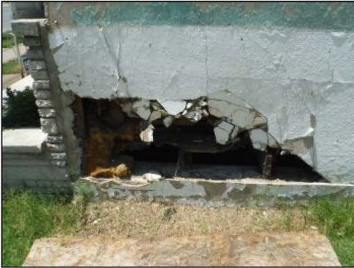
Vehicle damage is likely
