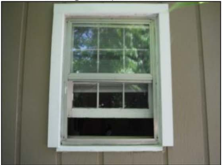
Keep screens in upstairs windows to reduce child fall out risk
