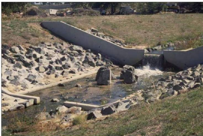
Photo 12. Vertical hard basin grade control structure.
