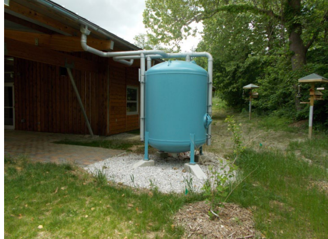
Photo 24. Aboveground cistern at the Watershed Center at Valley Water Mill.
