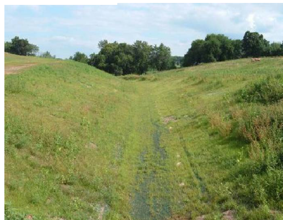
Photo 6. A steep, small grass-lined channel in a residential area reinforced by a TRM to maintain stability.
