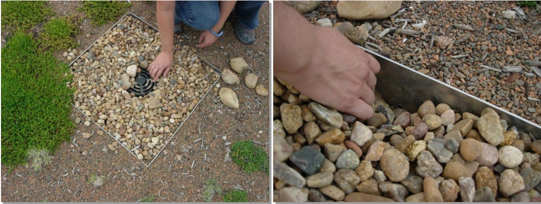
Photo 21. Separation of the roof drain from the growing media and plants using perforated metal edging and rock (Source: UDFCD, 2010).
