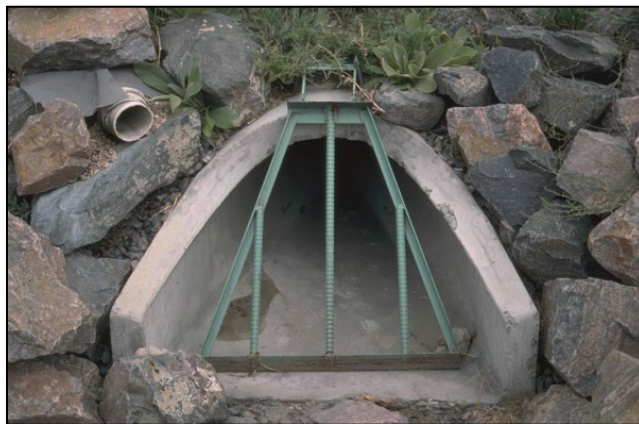
Photograph 4. A small trash rack at culvert entrance will increase the risk of entrance plugging.
