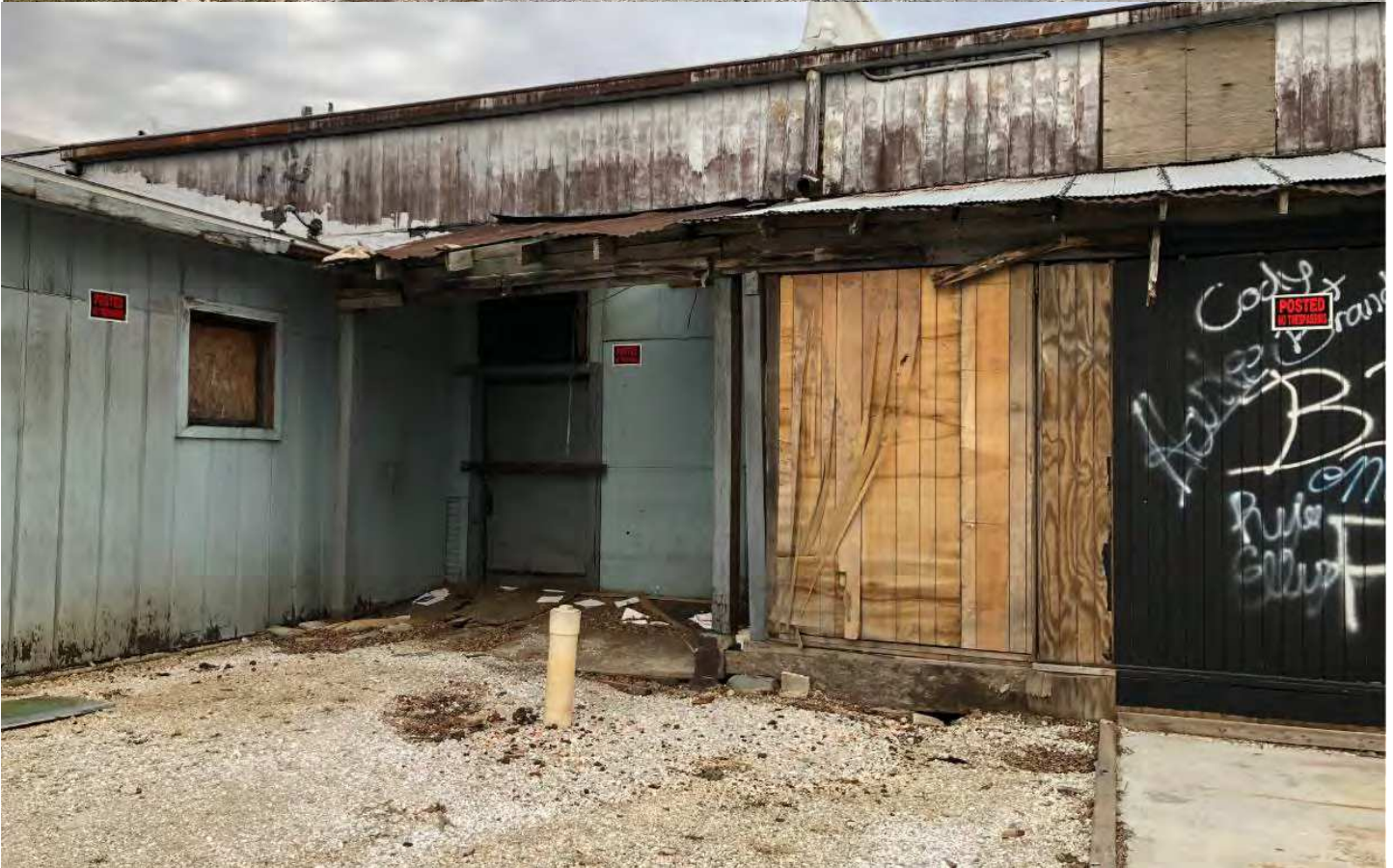
Rear Elevation of Nightclub / Saw & Tool Building: Corrugated metal roof attached to back of building is severely dilapidated and missing in places. The Corrugated metal roof previously extended further from the back of the building and covered the porch shown in the right-center of the top picture (as was observed on the April 11, 2019 site visit), but was mostly removed after multiple calls to police reporting homeless persons using the roofed areas, including the porch, as living areas. The pictures above represent the condition as of December 5, 2019, after the removal of roofing. Graffiti covers a significant portion of the rear wall of the building.
