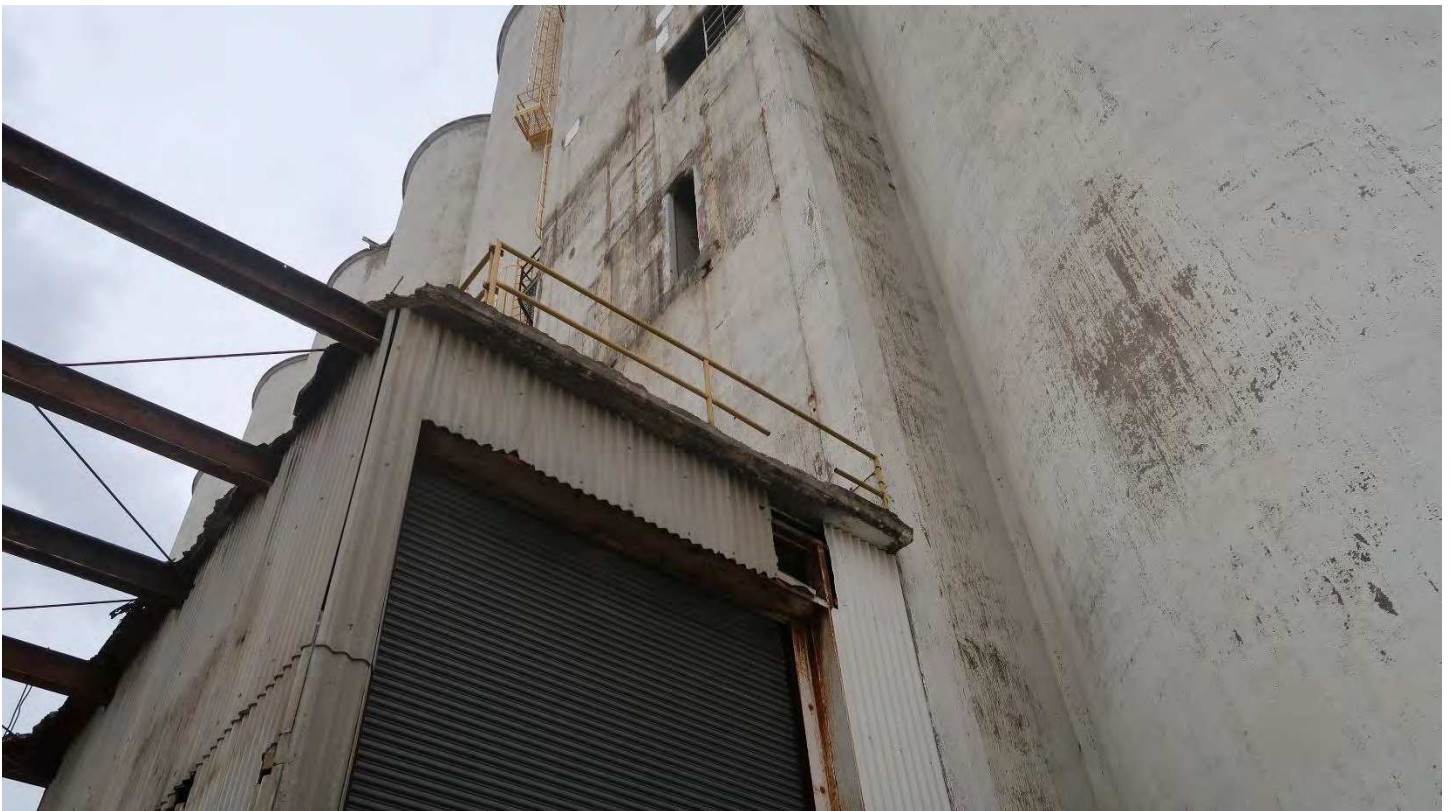
North Elevation of Area 3 Grain Tower: West side of corrugated metal structure rusted with one large piece of metal having partially fallen out leaving a sizeable hole. A portion of the protective railing on top of the corrugated metal structure is missing. Steel beams providing support for the roof of the corrugated metal structure are rusted. Roof edge appears from ground level to be significantly deteriorated.
