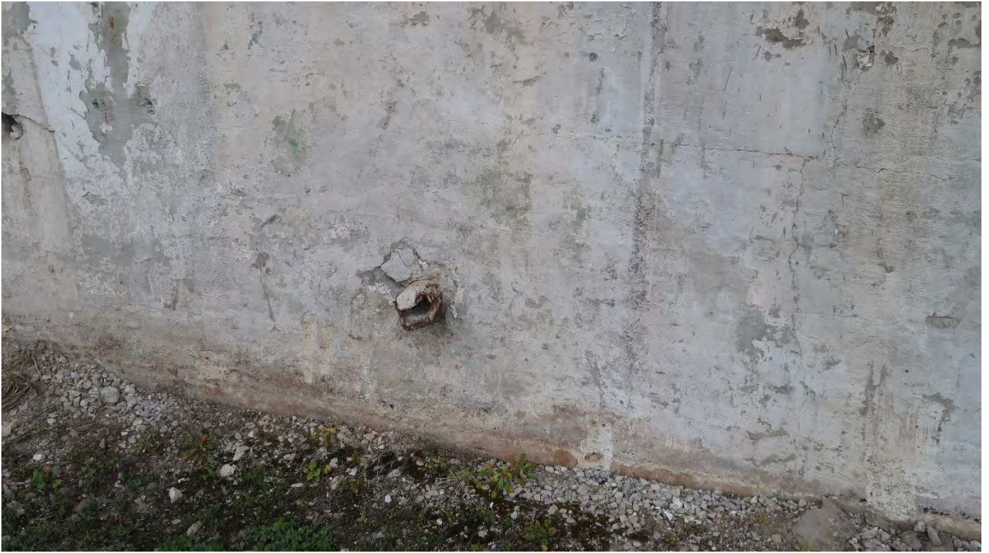
Front Elevation of JVIC Building: Rusty metal protrusions extend from loading dock wall, having been cut off years prior, present a danger of injury to passersby.
