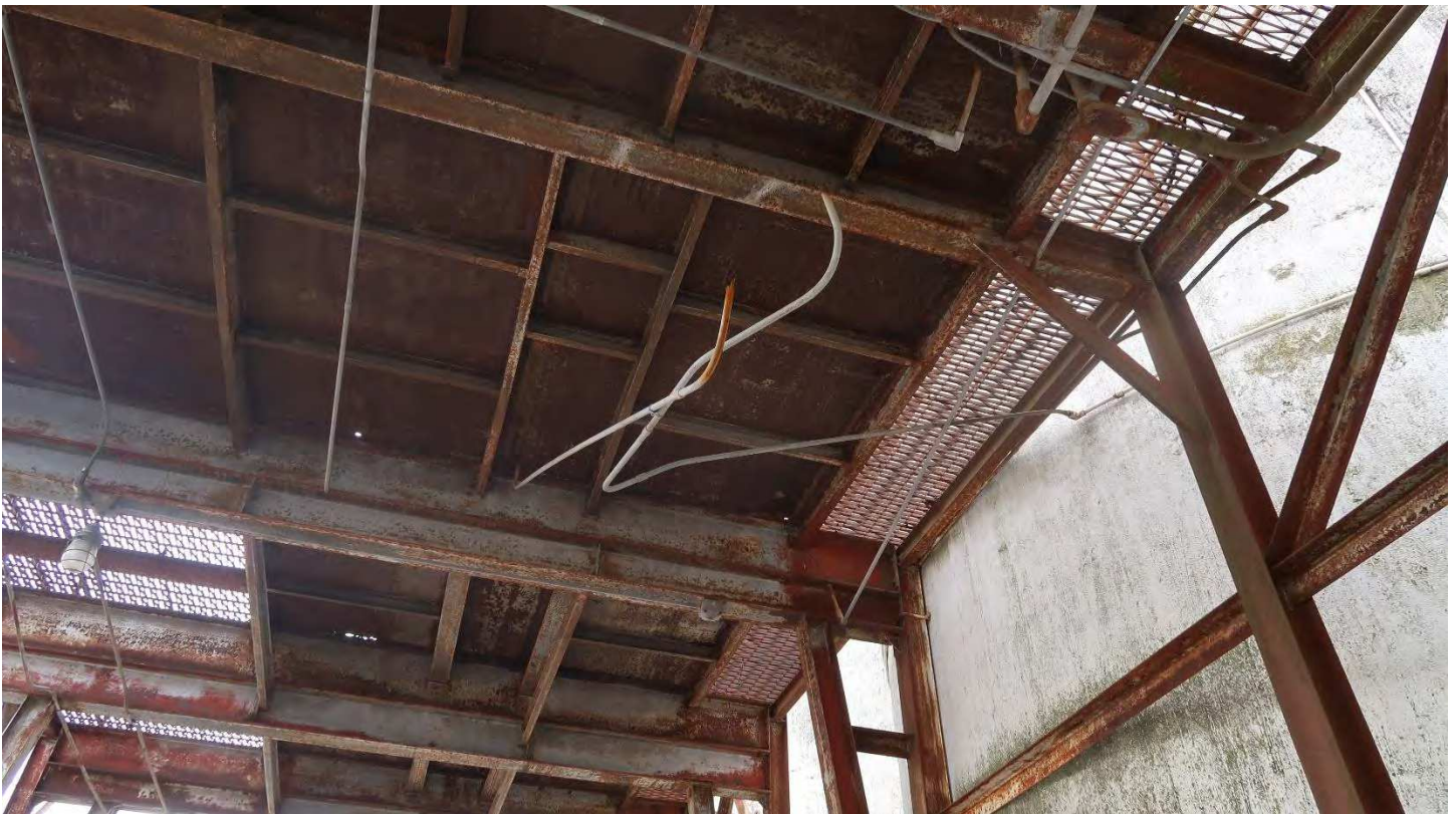
Underside of Steel Platform: All portions of steel structure, including vertical and horizontal support beams are significantly rusted. Underside of platform also shows significant rusting. Rusty pipes and open electrical conduits hang from the structure.
