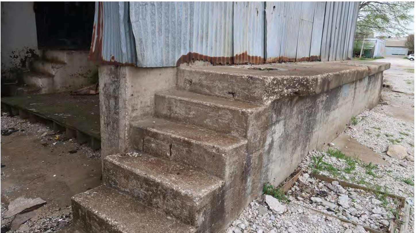
North Elevation of Area 3 Grain Tower: Concrete platform and stairs on front of structure are severely deteriorated with large pieces of concrete missing and significant spalling on the remaining structure. There is no handrail protecting the platform at the top of the stairs, which is approximately 40 inches high. Corrugated metal siding is rusted with sharp edges curled outward presenting injury risks. Large open hole in the top of the platform with sharp rusty metal objects inside presents injury risks.
