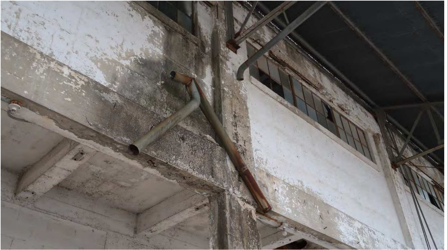
Front Elevation of JVIC Building: Broken windows are abundant with hanging shards of glass waiting to fall on loading dock / street area below. Components of previous downspout system hang from remaining mounting system, disconnected from main line from gutter. Concrete spalling is significant.
