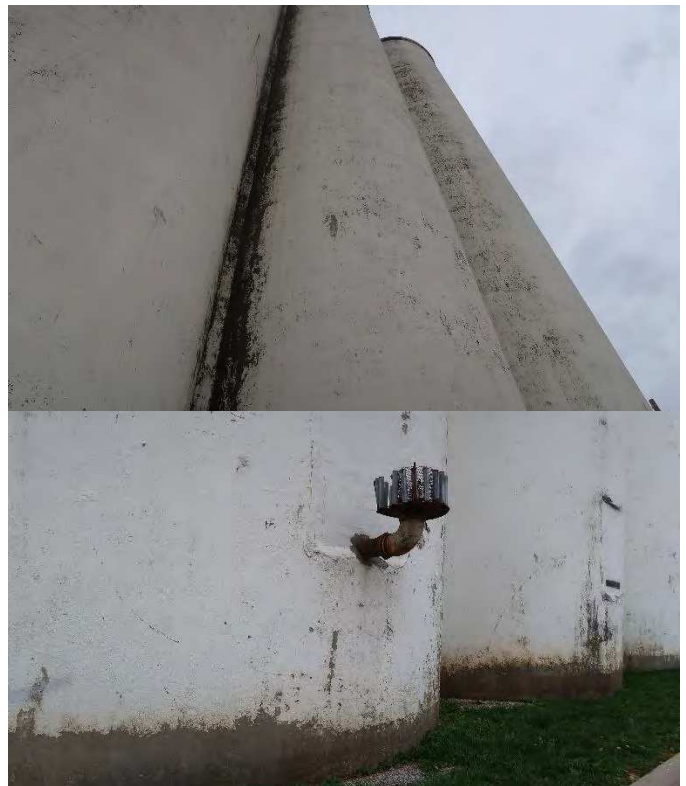
East Elevation of Area 2 Grain Tower: Exterior surfaces are dilapidated with peeling paint and evidence of spalling. Metal door and frame are rusted and held closed with an exterior latch and padlock. Concrete around the door frame is deteriorated, particularly below the door where rebar reinforcement is exposed to the elements and shows signs of significant rust. Rusted pipe protruding from structure at head/shoulder level presents a danger of injury to passersby.
