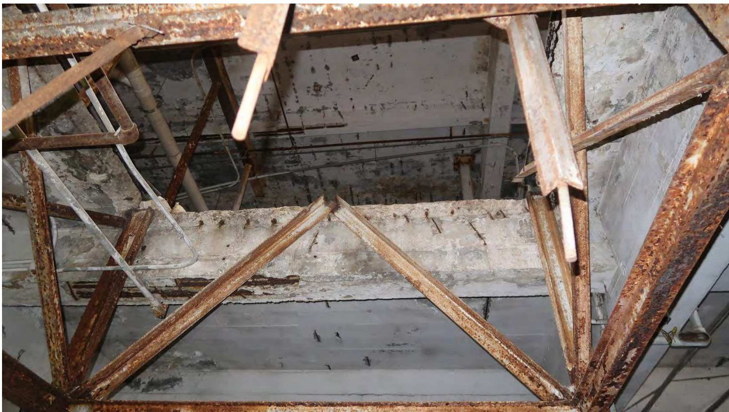
Inside JVIC Building: No access exists to second floor except for large holes in the deck between the first and second floors.
