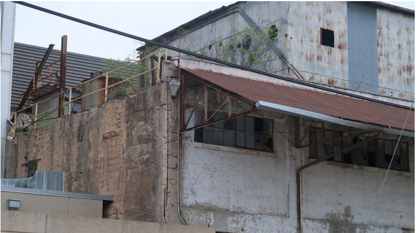
Front Elevation of JVIC Building: Concrete structure and finish is severely deteriorated. Gutter is bent to the point that water likely spills over the front instead of routing to downspouts. Remnants of unused structural components are significantly rusted and deteriorated.
