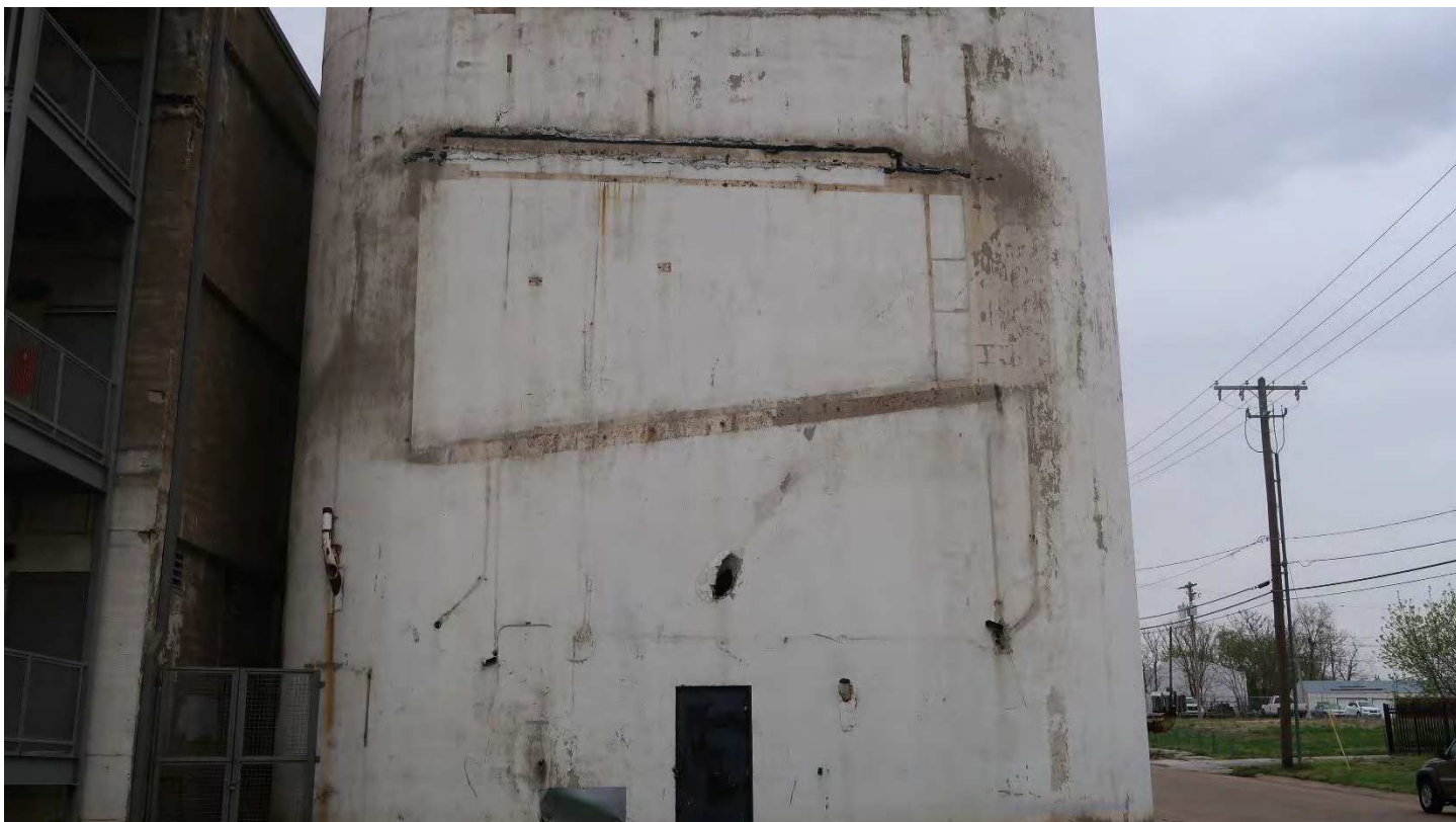
South Elevation of Area 2 Grain Tower: Dilapidated concrete structure with peeling paint and rusted metal pipes and brackets extending from the structure. Some evidence of the beginning of spalling of exterior surfaces. Cracks in the concrete structure are visible higher up on the south elevation.
