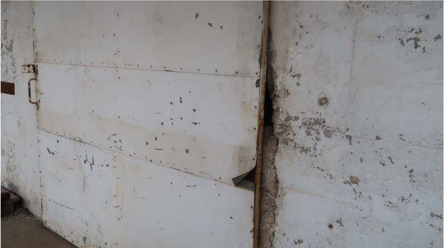
Front Elevation of JVIC Building: Makeshift door shows evidence of attempted break-in.
