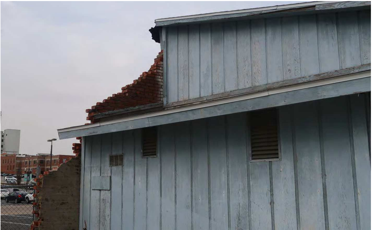
Rear Elevation of Nightclub / Saw & Tool Building: Portion of brick façade is missing. Wood siding is dilapidated with evidence of wood rot.
