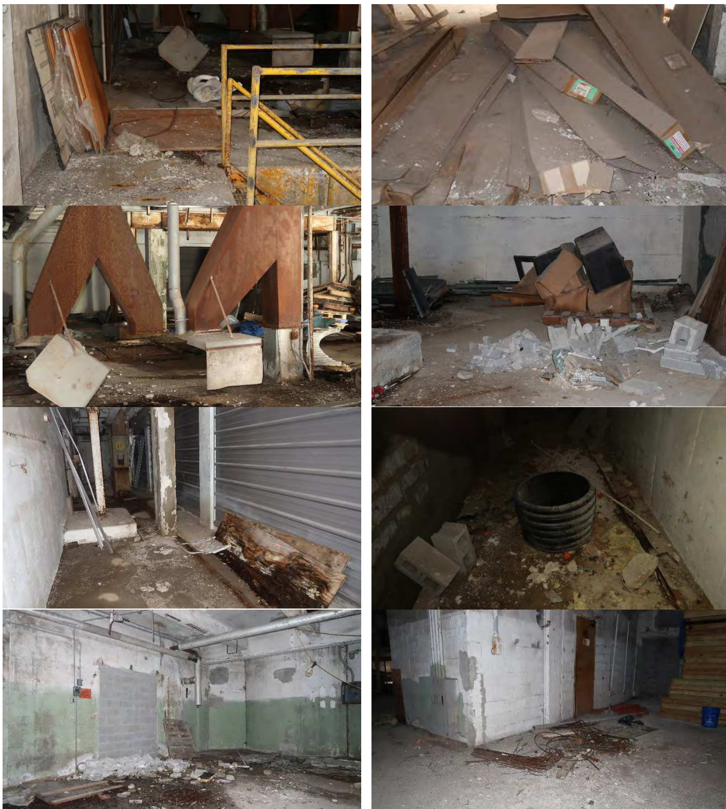
Inside JVIC Building: Significant accumulations of debris are pervasive through the interior of the first floor of the JVIC Building.
