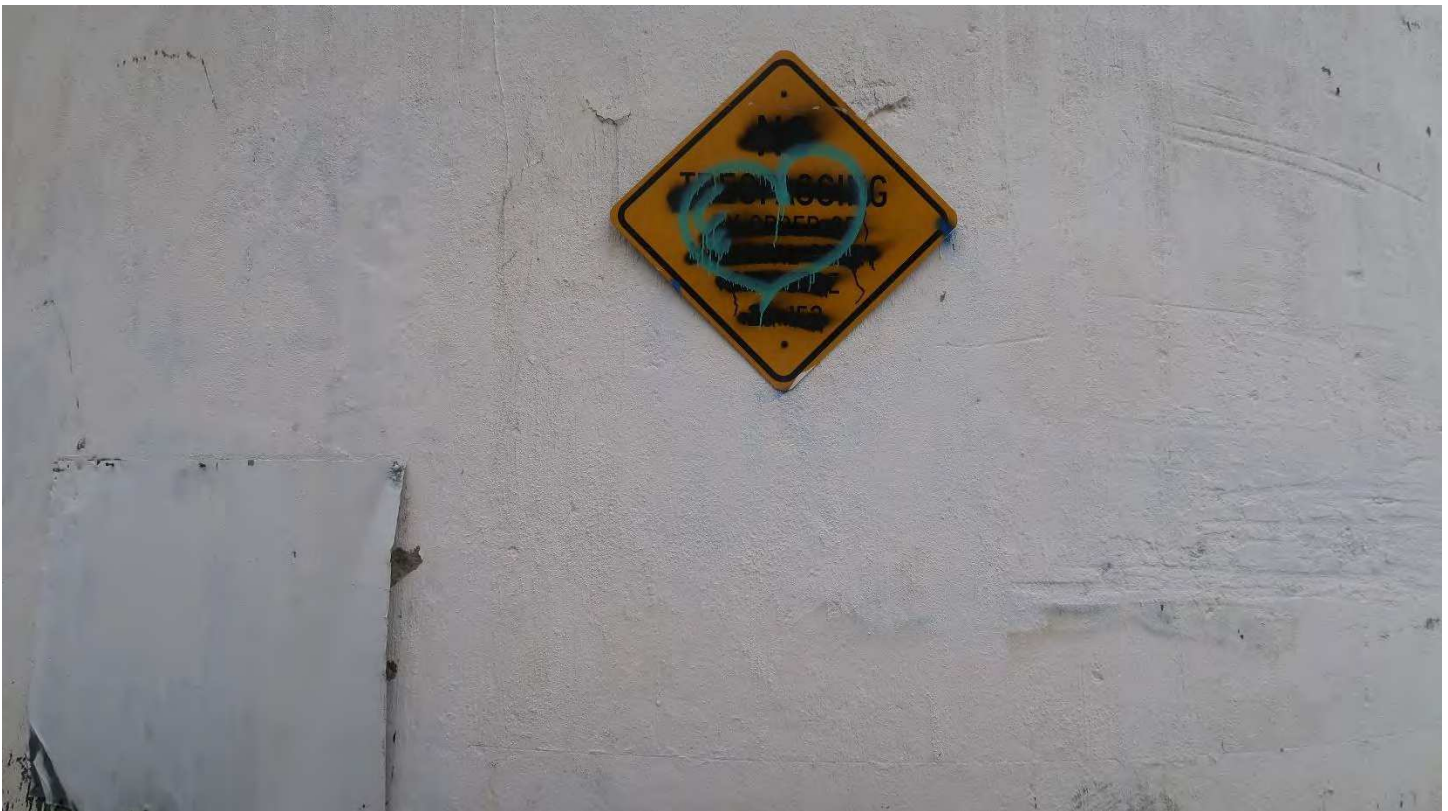
South Elevation of Area 3 Grain Tower: Sheet metal has been torn away from one of the openings, suggested an attempt to break in. Remnants of sheet metal covering are still attached to the building, creating a sharp protrusion that poses risk of injury to passersby. Portions of the concrete exterior are breaking off of the building and there is significant evidence of spalling. No trespassing sign is graffitied over.
