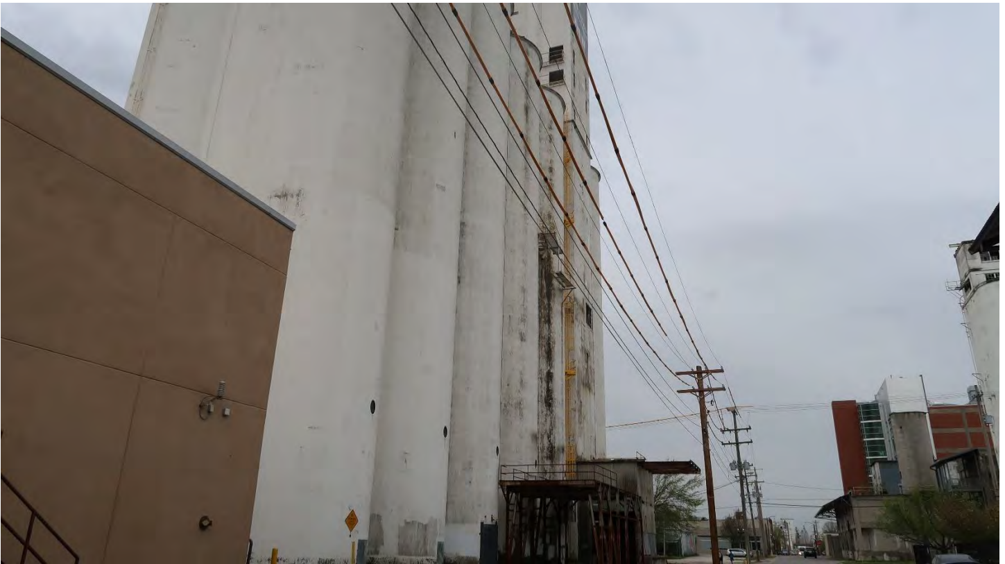
North Elevation of Area 3 Grain Tower: Exterior is dilapidated with peeling paint, cracks in exterior walls, and evidence of beginnings of spalling on exterior walls. Large openings in exterior walls with no glass, bars, or any other protective barriers are present to prevent falls.
