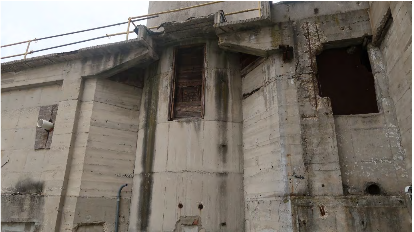
Side Elevation of JVIC Building: Significant concrete spalling and exposure of rebar reinforcement. Holes exist through exterior wall. Chunks of concrete have dislodged and fallen from overhanging roof. Numerous open perforations exist.
