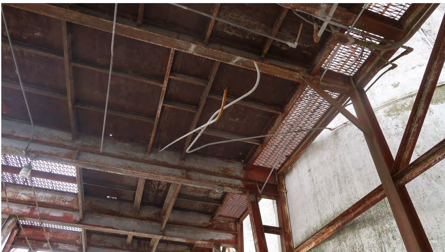
Underside of Steel Platform: All portions of steel structure, including vertical and horizontal support beams are significantly rusted. Underside of platform also shows significant rusting. Rusty pipes and open electrical conduits hang from the structure.
