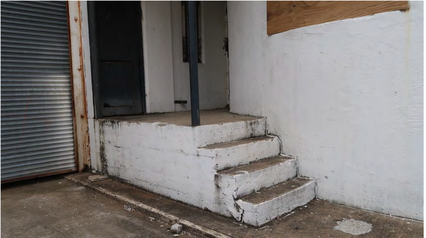
Northwest Entry Way to Area 3 Grain Tower: Concrete stairs and platform to main doors are significantly deteriorated with several cracks and evidence of spalling. Handrail missing from platform.
