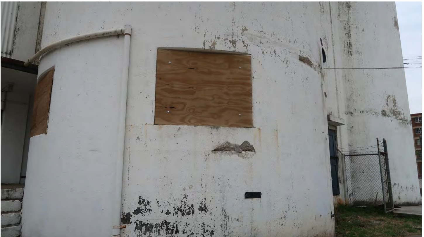
West Elevation of Area 3 Grain Tower: Exterior openings have been boarded up. Concrete surfaces are deteriorated with notable spalling. Chunks of concrete are missing from the exterior wall, exposing the underlying rebar reinforcement, which is rusted.
