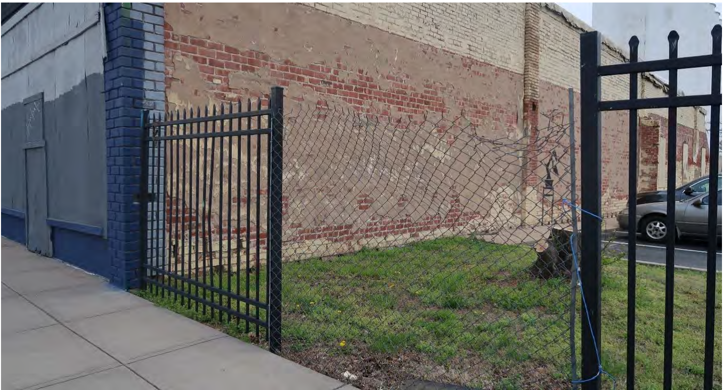
Side (South) Elevation of Nightclub / Saw & Tool Building: Portion of iron fence is missing and has been replaced by a piece of chain link fencing with sharp metal ends protruding at top creating a safety concern.
