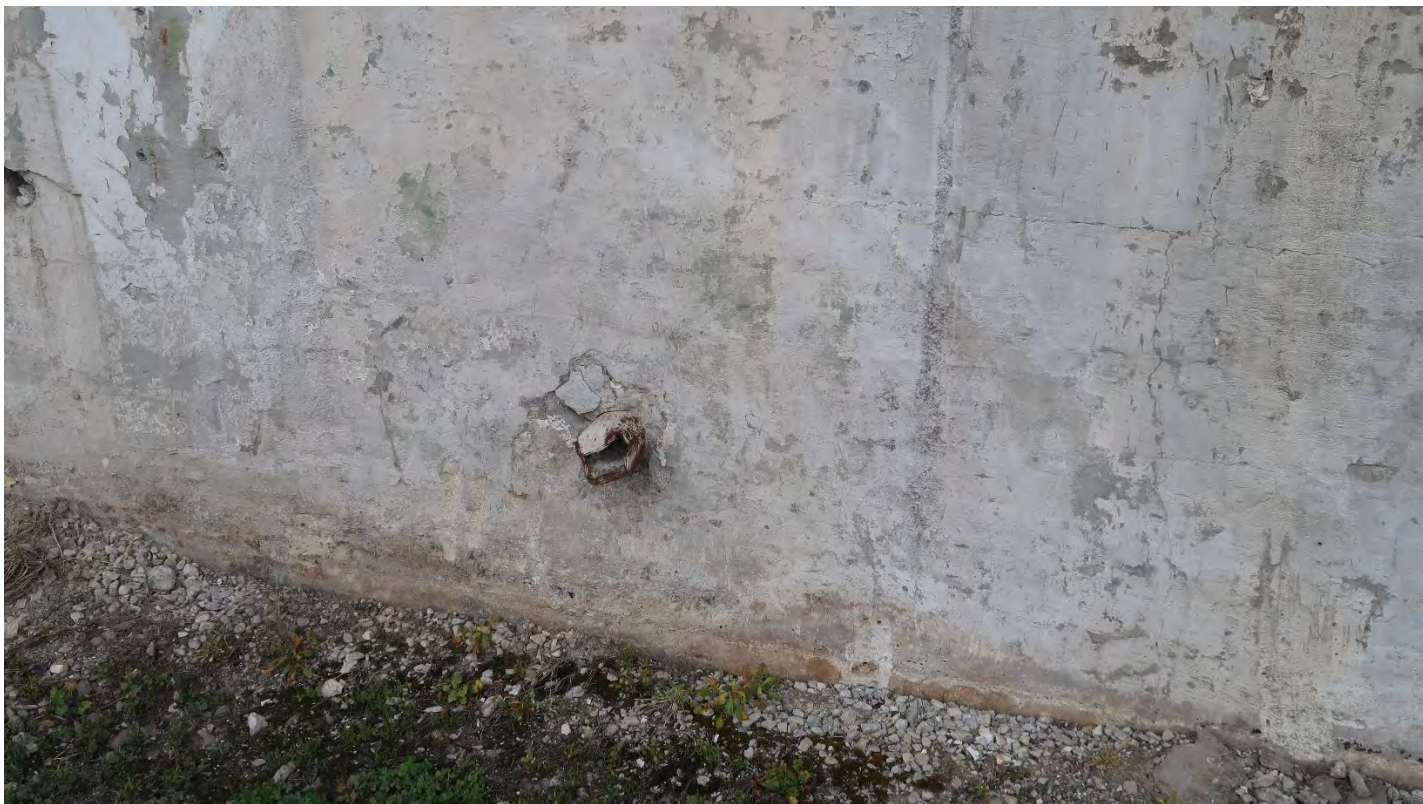
Front Elevation of JVIC Building: Rusty metal protrusions extend from loading dock wall, having been cut off years prior, present a danger of injury to passersby.
