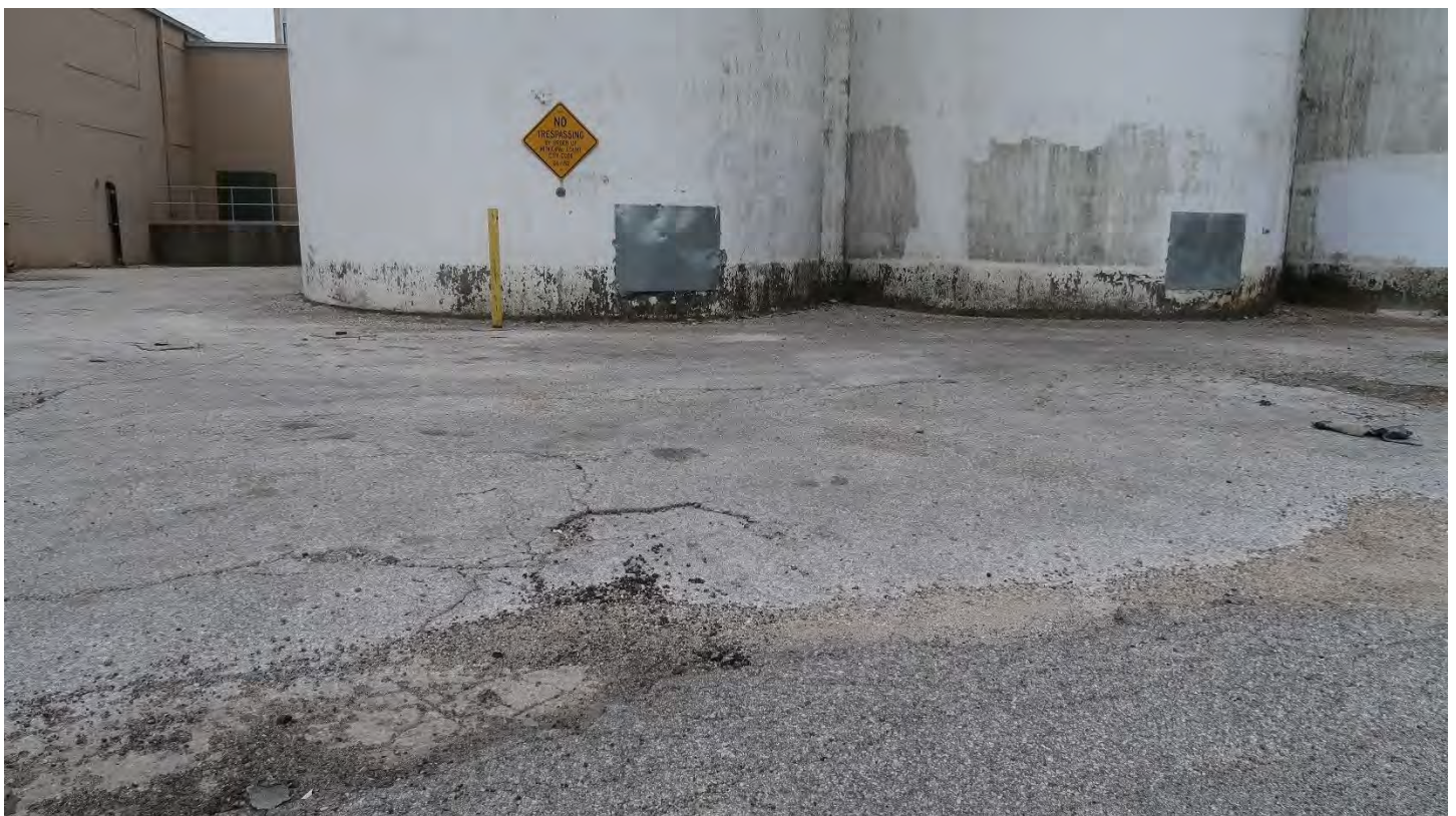
South Elevation of Area 3 Grain Tower: Exterior is dilapidated with peeling paint and evidence of spalling in the concrete surfaces. Exterior openings are covered with sheet metal. Corners of sheet metal attached to structure are damaged and/or peeling away from the structure, creating many sharp protrusions that present injury risks.
