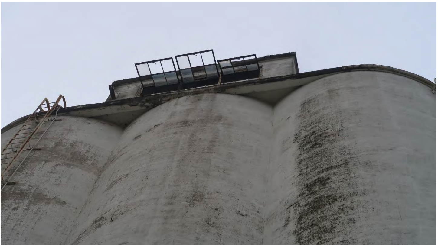
South Elevation of Area 2 Grain Tower (top picture) and North Elevation of Area 2 Grain Tower (bottom picture): Window frames at top of the grain tower are rusted with several panes of glass missing. Remaining glass panes will potentially fall to the grassy area on the south side and parking lot on the north side, as the windows continue to deteriorate. Evidence of spalling of concrete surfaces at the top of the grain tower.
