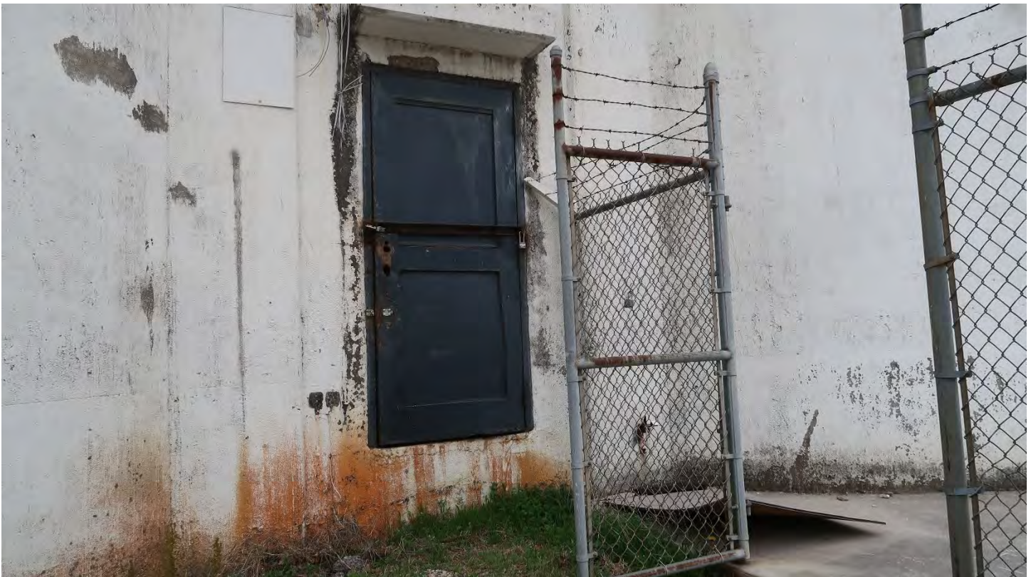
West Elevation of Area 3 Grain Tower: Exterior is dilapidated with peeling paint and evidence of spalling on concrete walls. Wires hang from the structure by the door. Concrete surfaces on the ground are deteriorated, and settling unevenly into the ground, creating trip and fall hazards. Chain link fencing is rusted and starting to fall down. Barbed wire at the top of the chained link fencing is also rusted and presents risk of injury. Missing and broken door hardware is evidence of prior break-in attempts.
