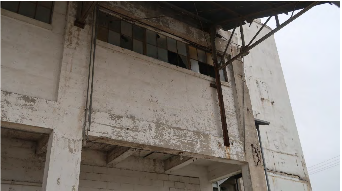
Front Elevation of JVIC Building: Electrical conduits simply cut off above loading dock ceiling. Structural components of awning covering loading dock / street area show significant rust and deterioration.
