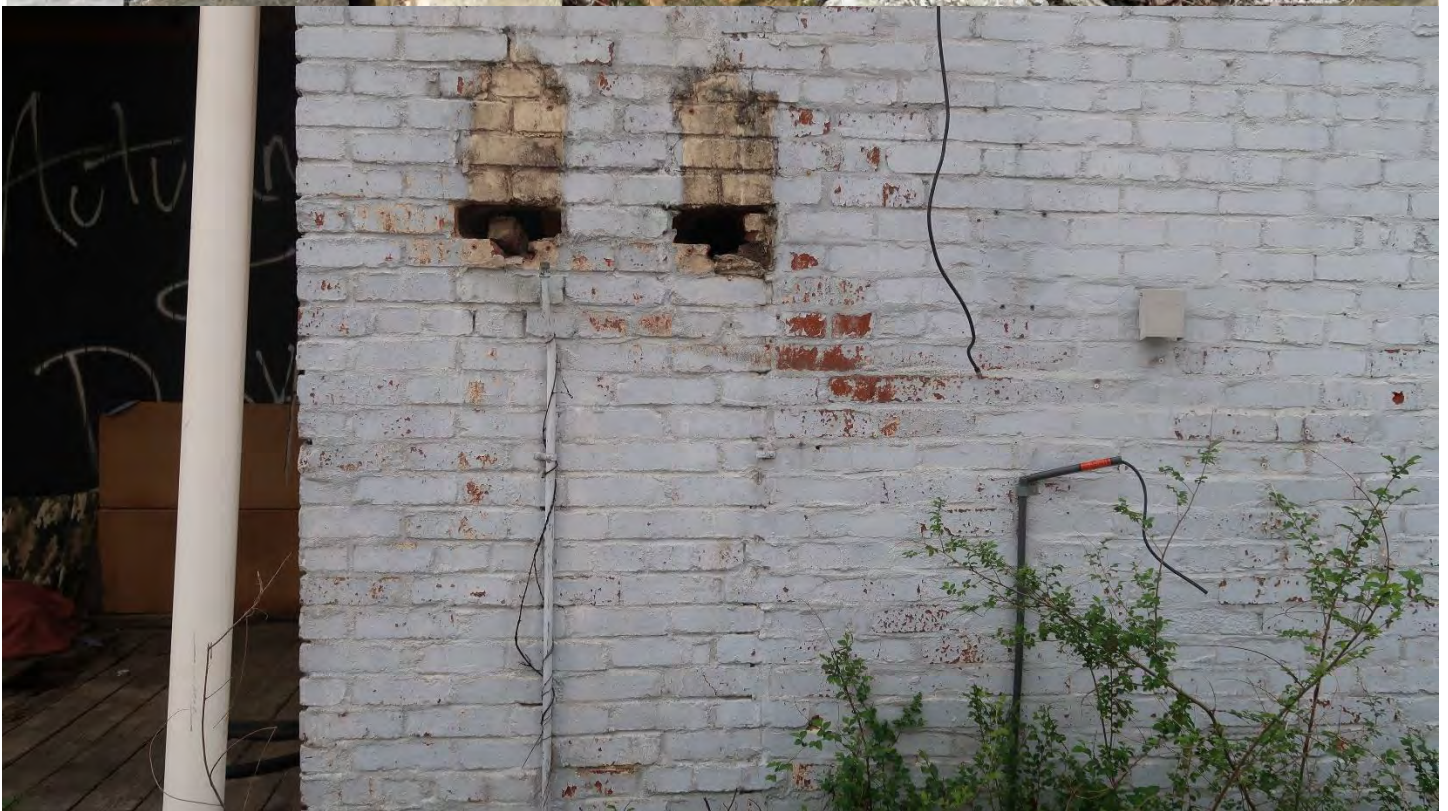
Side (North) Elevation of Nightclub / Saw & Tool Building: Holes in exterior wall. Wooden porch attached to building shows evidence of wood rot, with all or parts of certain boards missing. Loose wiring hanging from side of building and protruding from exposed conduit attached to building wall.
