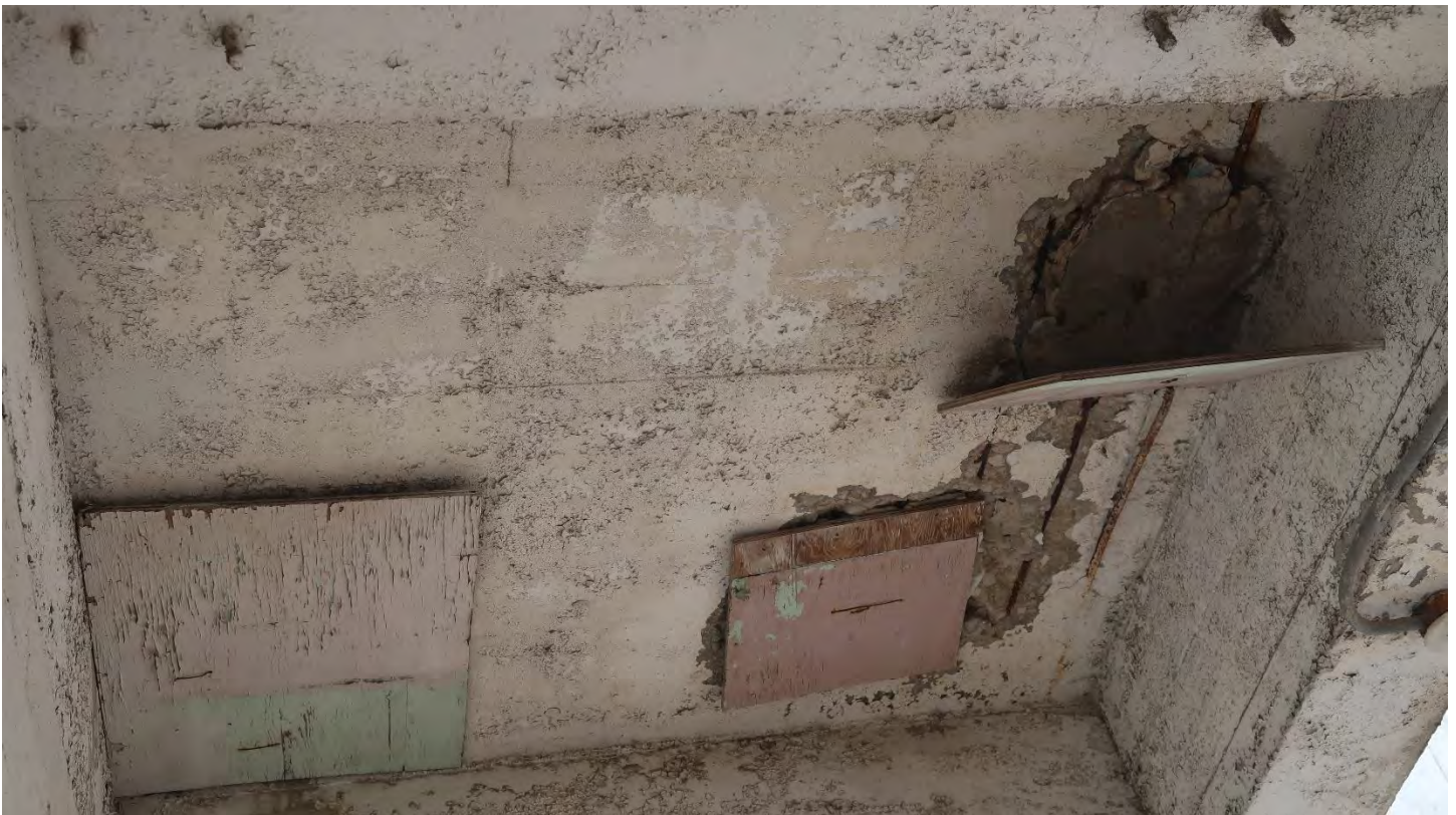
Front Elevation of JVIC Building: Portions of loading dock ceiling, including makeshift patches, falling onto loading dock area.
