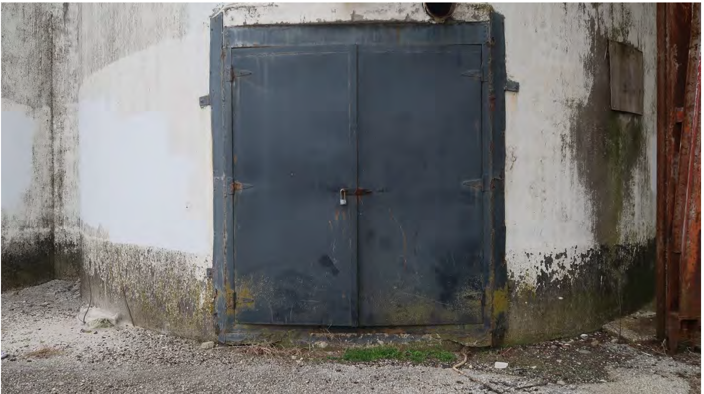
North Elevation of Area 3 Grain Tower: Steel structure at front of tower shows significant rust. Concrete footings into which the steel pillars supporting the structure are attached are deteriorated with evidence of spalling. Metal entry door and frame are rusted and door is minimally secured with exterior latch and padlock. There are holes in the exterior wall above the entry door.
