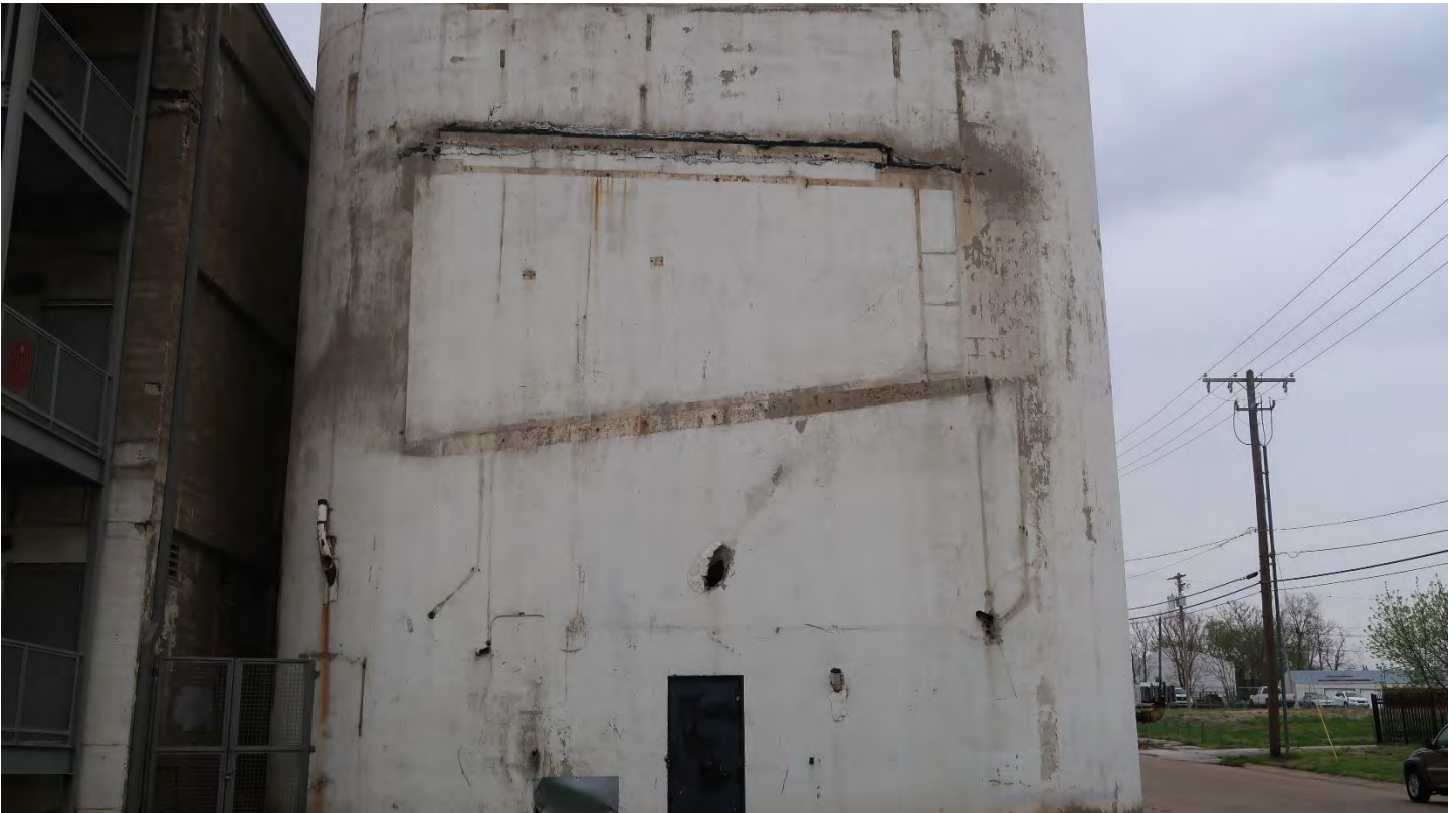
South Elevation of Area 2 Grain Tower: Dilapidated concrete structure with peeling paint and rusted metal pipes and brackets extending from the structure. Some evidence of the beginning of spalling of exterior surfaces. Cracks in the concrete structure are visible higher up on the south elevation.
