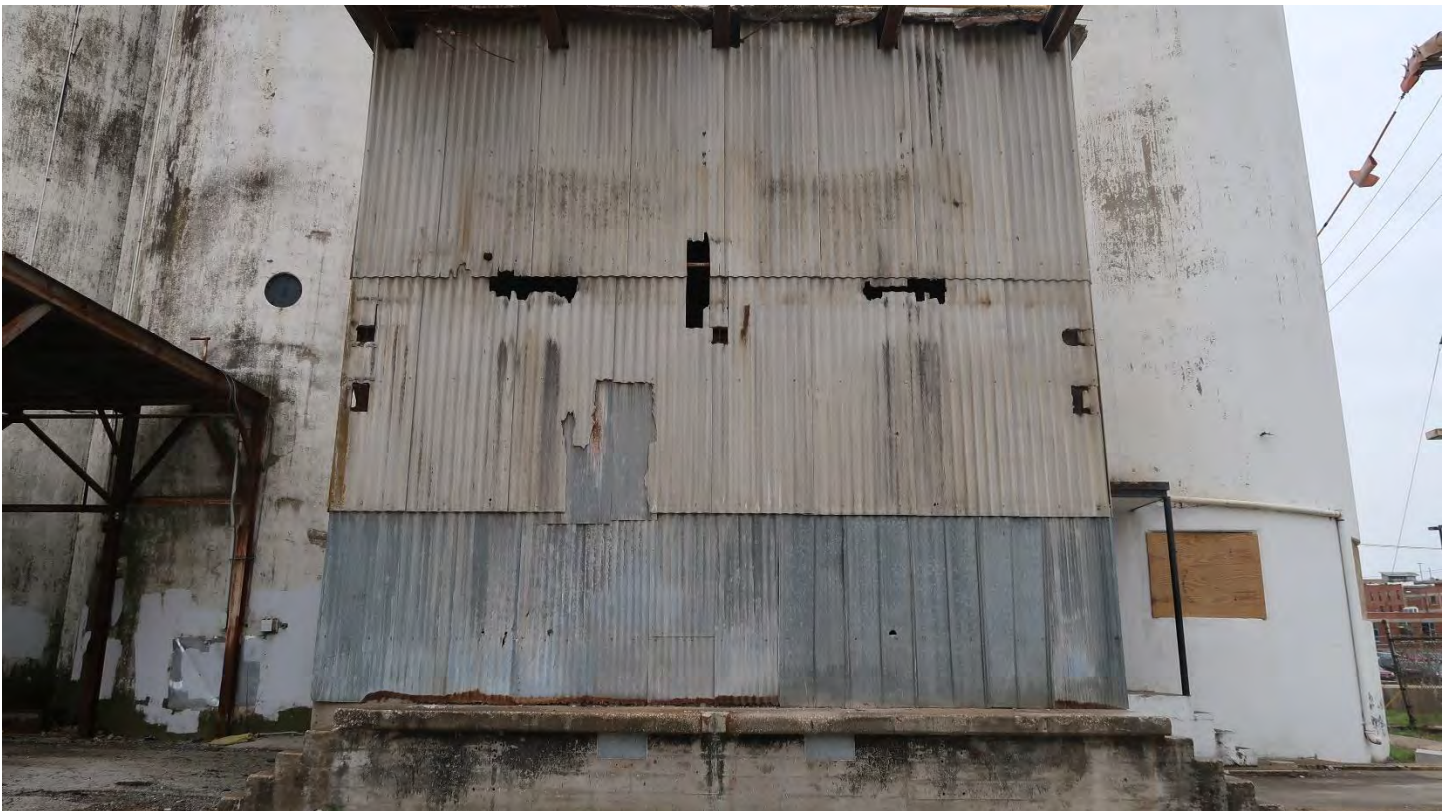
North Elevation of Area 3 Grain Tower: Corrugated metal structure attached to grain tower is severely dilapidated with holes in exterior of structure. Significant rusting (particularly along the base of the wall and steel support beams at the top of the structure) is present. Portions of the corrugated metal have been broken or torn off, leaving sharp rusted edges exposed which present a risk of injury. Concrete base upon which the structure sits is significantly deteriorated.
