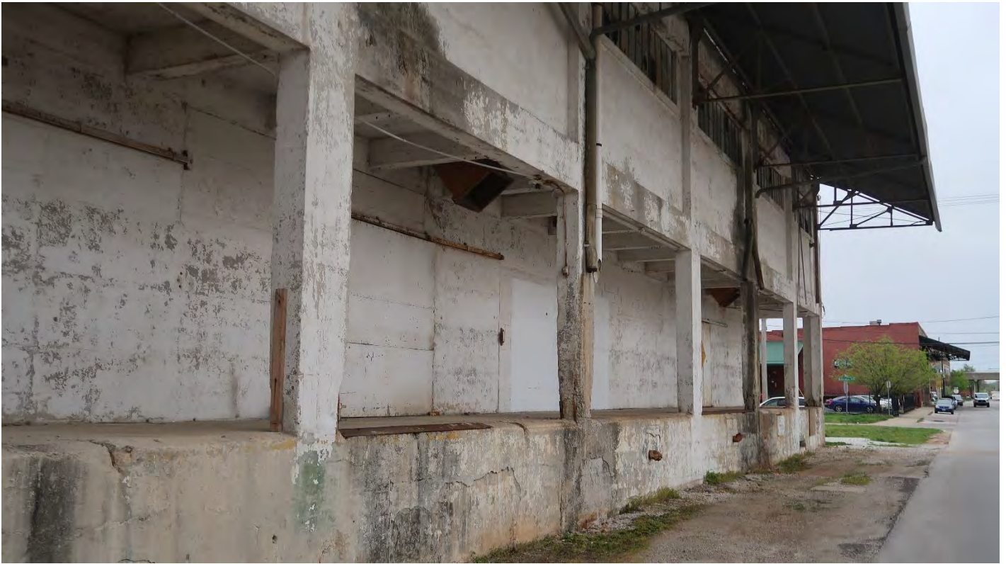
Front Elevation of JVIC Building: Concrete structure and finish is severely deteriorated. Downspouts are cut off over eight feet above ground level. Electrical conduits are cut off randomly. Pavement ends in a mix of gravel and weeds before reaching loading dock.
