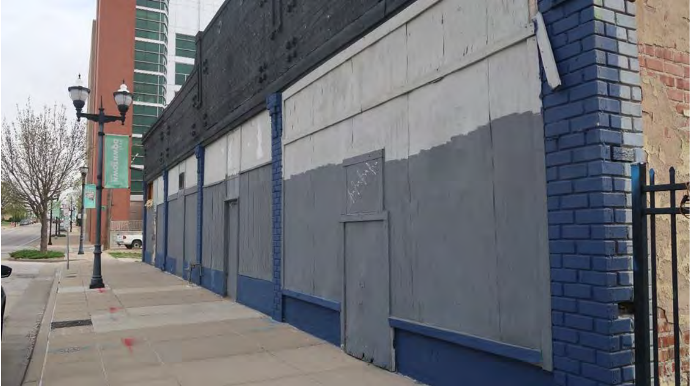
Front Elevation of Nightclub / Saw & Tool Building: Portion of exterior wall missing with insulation and framing exposed. Storefront has been removed and boarded up with plywood, which is dilapidated with some wood rot present. Upper brick facade is beginning to separate from sides of building and lean over sidewalk.
