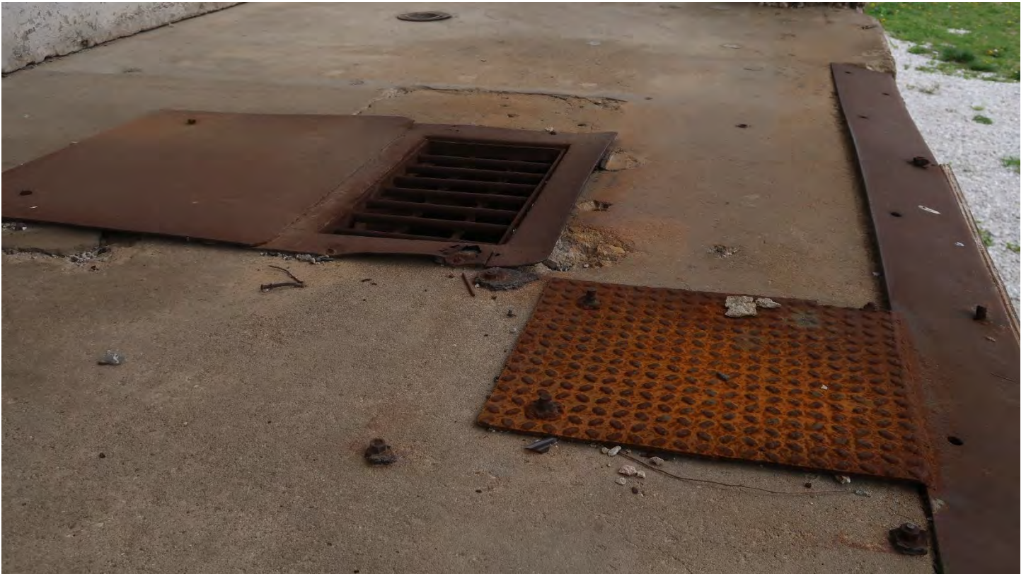
Front Elevation of JVIC Building: Loading dock area has numerous trip and fall hazards including deteriorated grating with edges curled up and rusty bolt anchors protruding above concrete surface.
