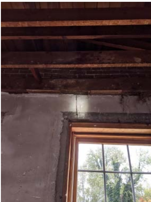
Crack in Masonry Wall of West Suite
