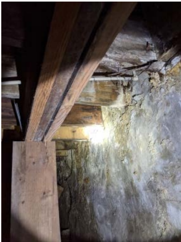
Moisture Damage in Basement
