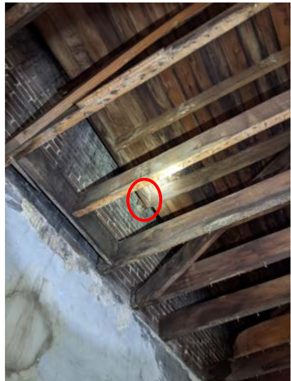
Roof Truss Sliding out of Support Pocket
