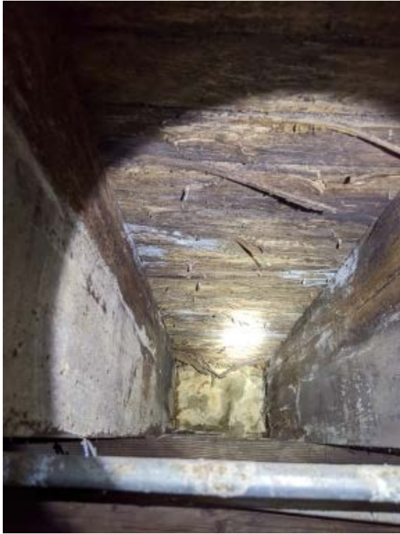
Moisture Damage in Basement
