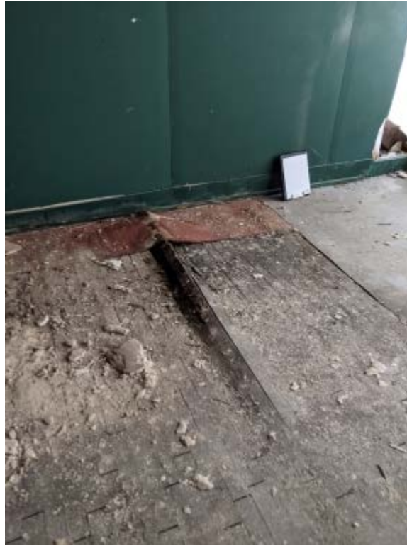
Buckled Floor Planks on First Floor of East Suite
