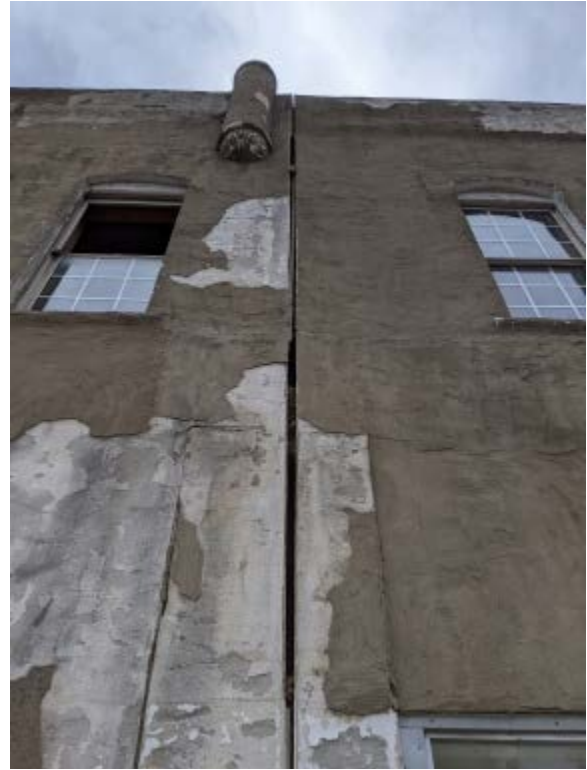
Vertical Crack in North Wall
