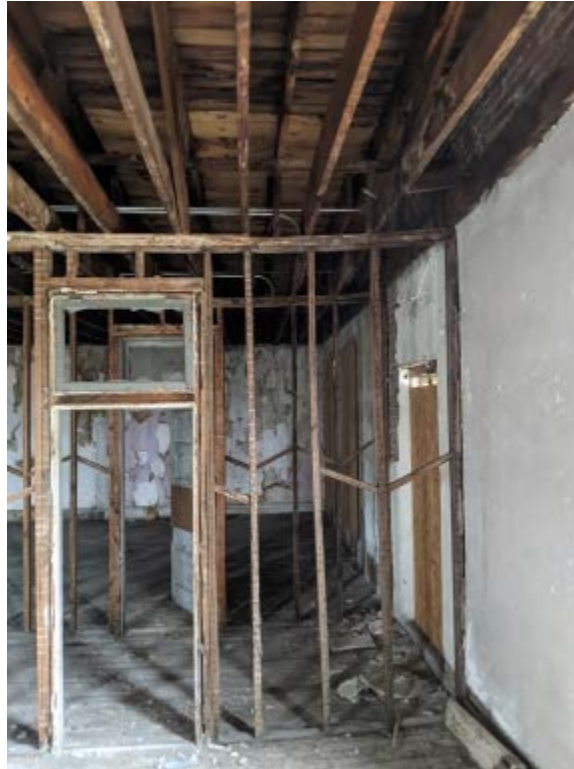
Damaged Load-Bearing Wall on Second-Floor of West Suite
