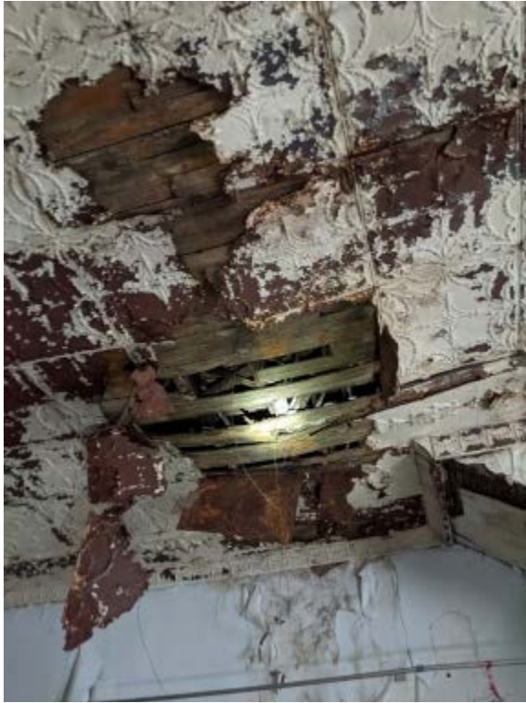
Hole in Second Floor of East Suite
