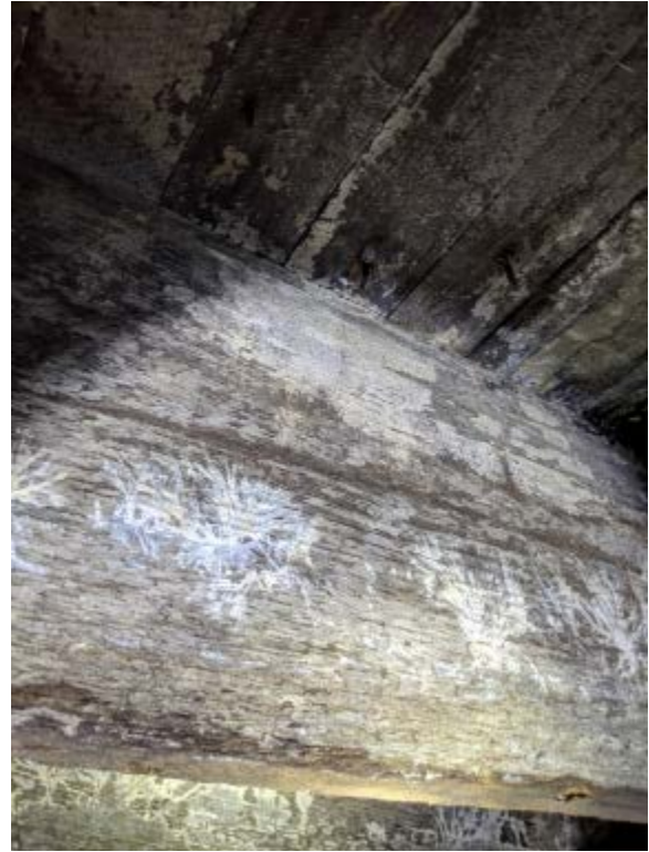
Organic Growth in Basement
