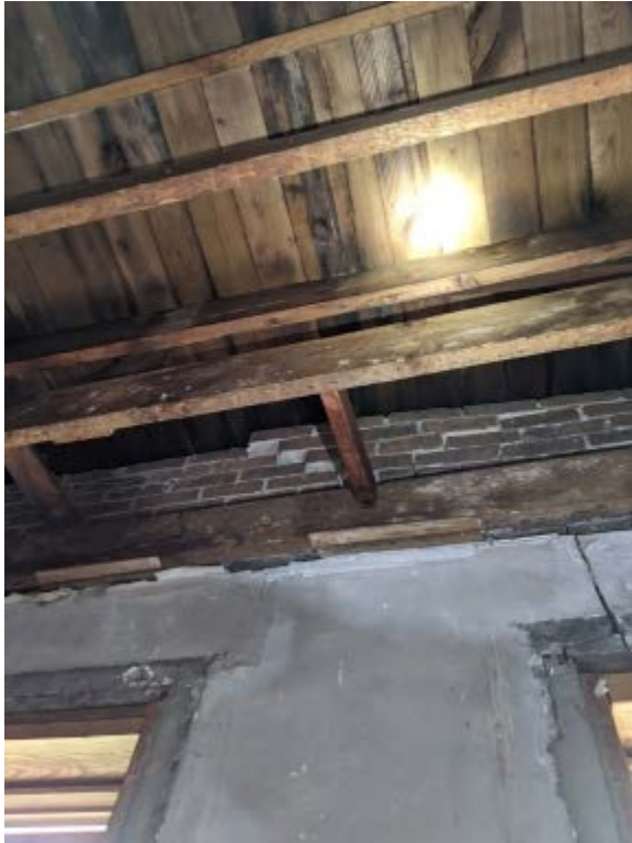
Displaced Bricks at Top of South Wall of West Suite
