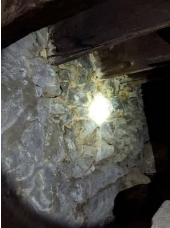
Eroded Basement Wall
