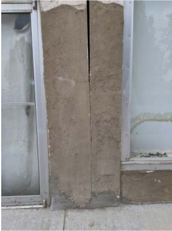
Vertical Crack in North Wall
