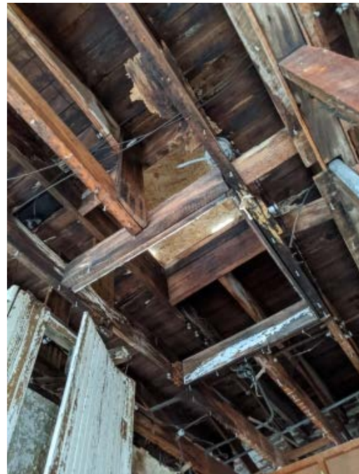
Deteriorated Roof Framing of East Suite
