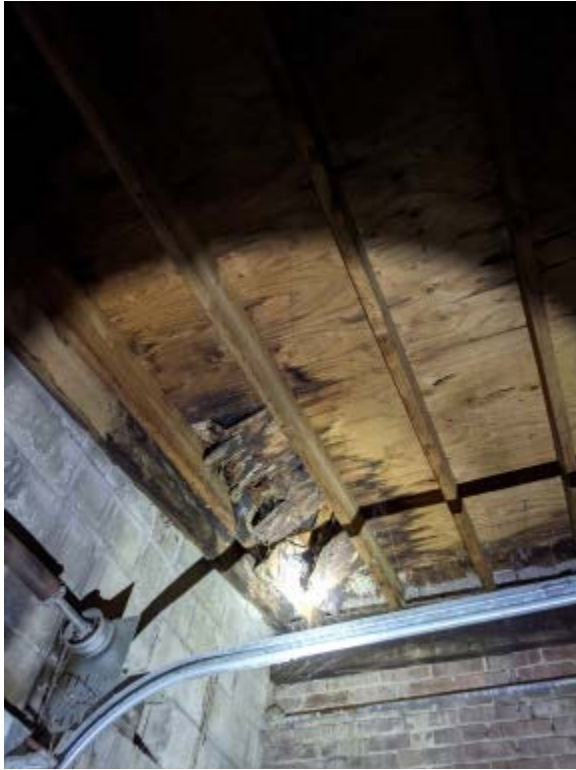
Deteriorated Roof Framing at Addition
