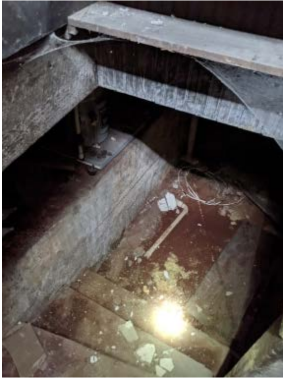
Muddy Basement Floor
