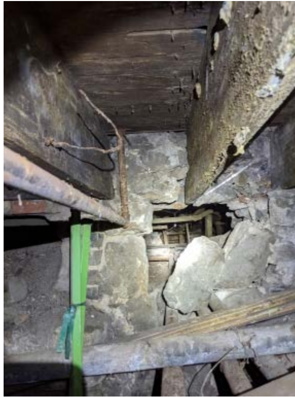
Hole in Basement Demising Wall
