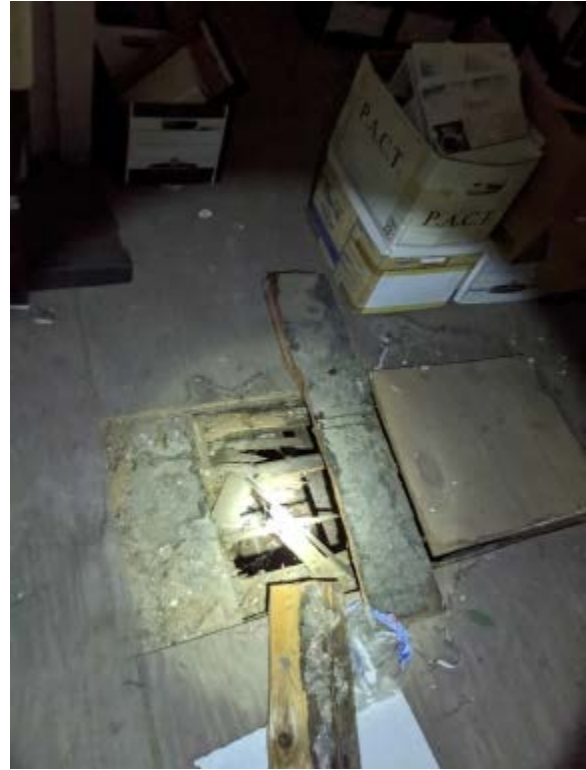
Hole in First Floor of West Suite
