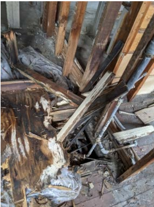
Pile of Debris on Second Floor of East Suite
