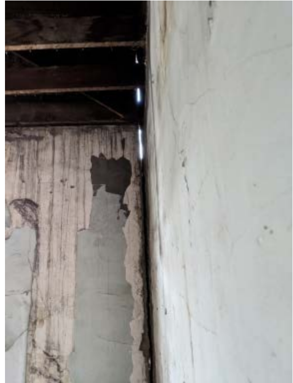
Vertical Gap at North Wall of West Suite
