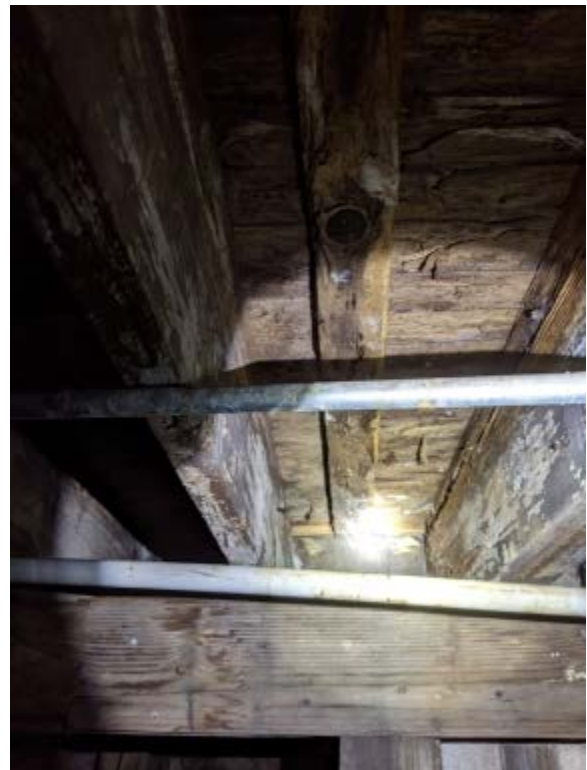
Moisture Damage in Basement
