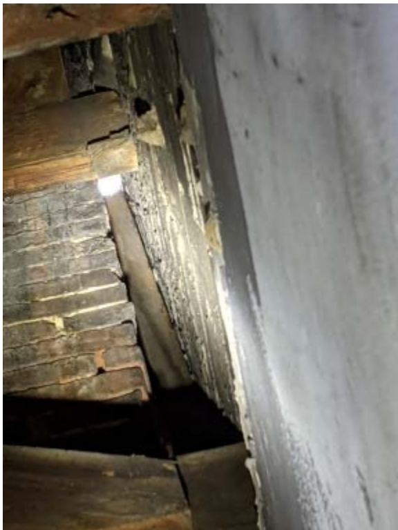
Vertical Gap at North Wall of West Suite
