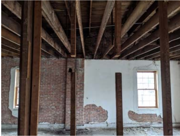
Load-Bearing Studs Cut Off at West Suite
