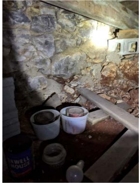
Eroded Basement Wall
