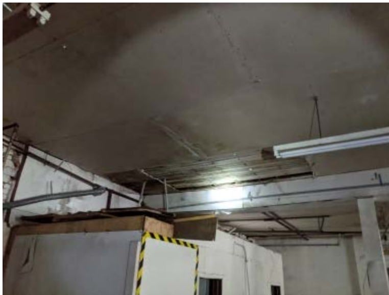
Deflected Beam at South End of Beam-Column Line at West Suite
