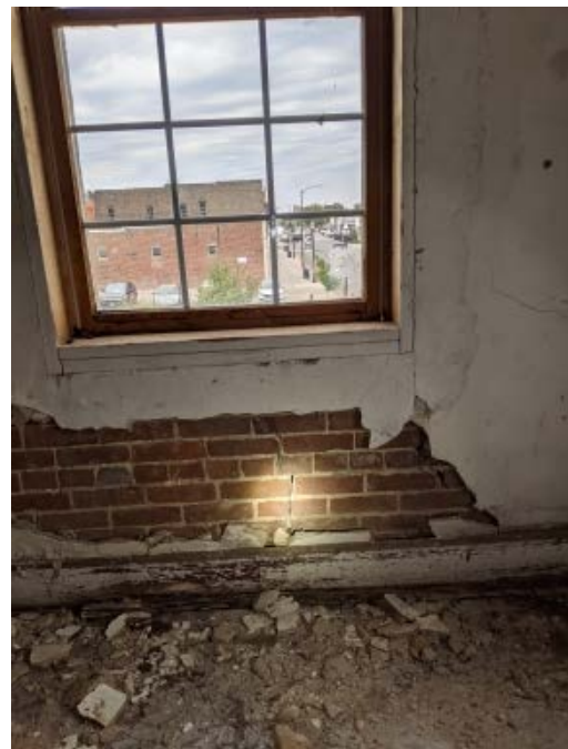
Crack in Masonry Wall of West Suite
