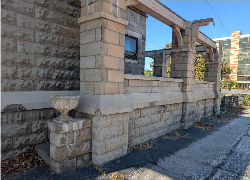
Photos 13-15 – Remaining porch columns and decorative brackets
