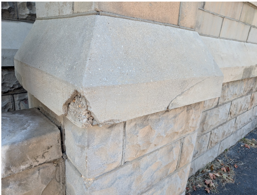
Photo 36-38 – Areas of concrete porch deterioration
