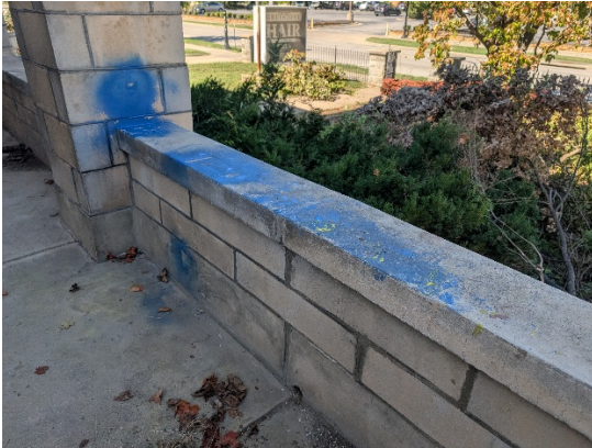
Photos 32-35 – Graffiti on masonry surfaces
