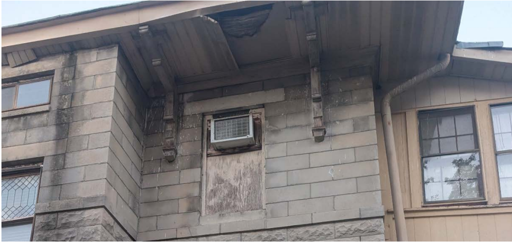
Photos 20-21 – Deteriorated soffit
