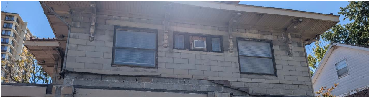
Photos 23-24 – Window trim rot
