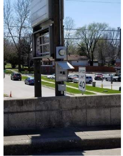
Figure 29 – Open breaker panel, 1000 block E Kearney St, north side
