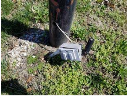
Figure 27 – Deteriorated signage w/ exposed wires, 800 block W Kearney St
