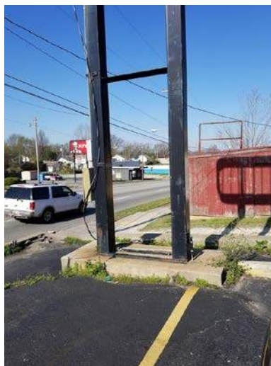
Figure 25 – Deteriorated signage w/ loose wires, 700 block W Kearney St, north side
