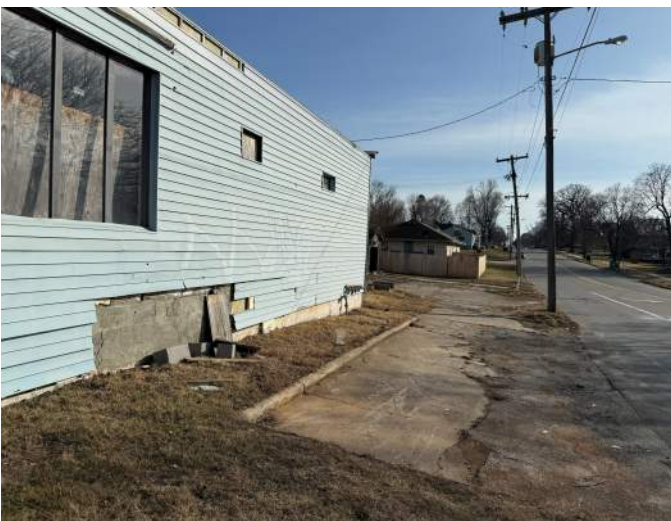
Located at 930 W Kearney, Building facade deteriorating. No sidewalk or curb. Non ADA Compliant.
