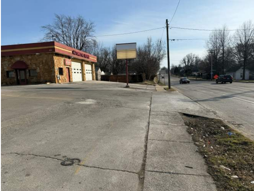
Located at 658 W Kearney, No sidewalk or curb. Non ADA Complaint.
