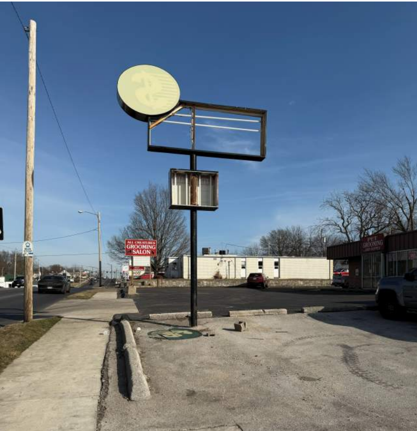
Located at 920 W Kearney, Signage is exposed and deteriorated.
