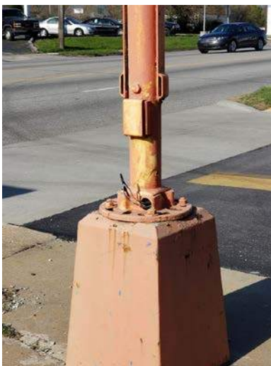
Figure 24 – Deteriorated signage w/ exposed wires, 1200 E Kearney St, north side
