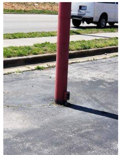
Figure 26 – Deteriorated signage w/ open junction box & exposed wires, 1200 block W Kearney St, north side
