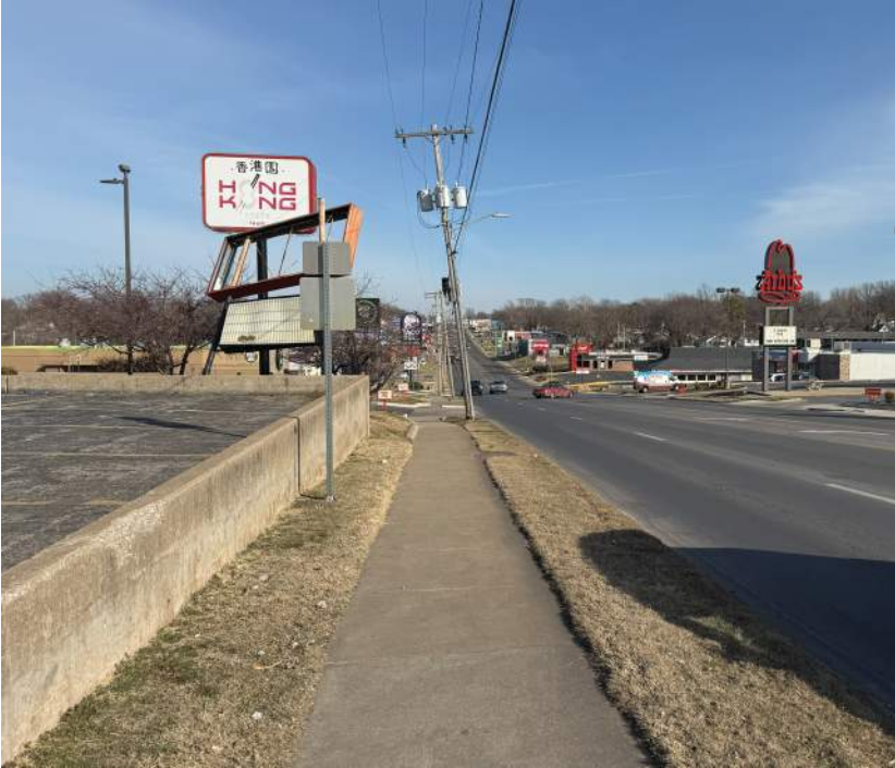
Located at 1445 and 1421 W Kearney, Signage with exposed wires falling onto adjacent property.
