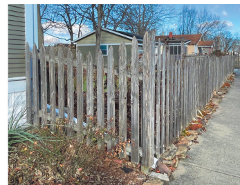
7 FENCE @ NORTHEAST CORNER OF HOUSE (SLOPE UP TO MATCH GRADE OF SOIL)
